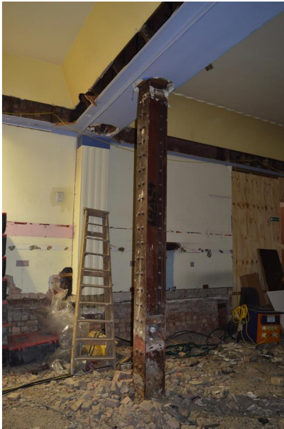
Plate 16: Ground floor, entrance hall, iron supports formerly encased in fluted plaster column, facing south-west (7533_0026)
