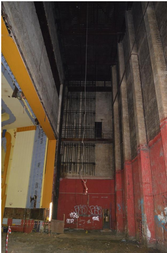
Plate 30: Ground floor, former stage area with loading gallery and counterweight scenery lines, facing west (7533_0044)
