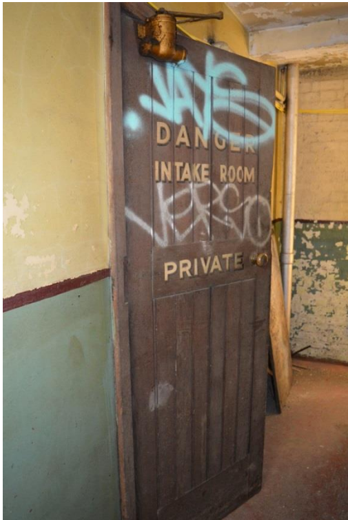
Plate 48: First floor, east wing, plenum and intake room door detailing, facing east (7533_0103)
