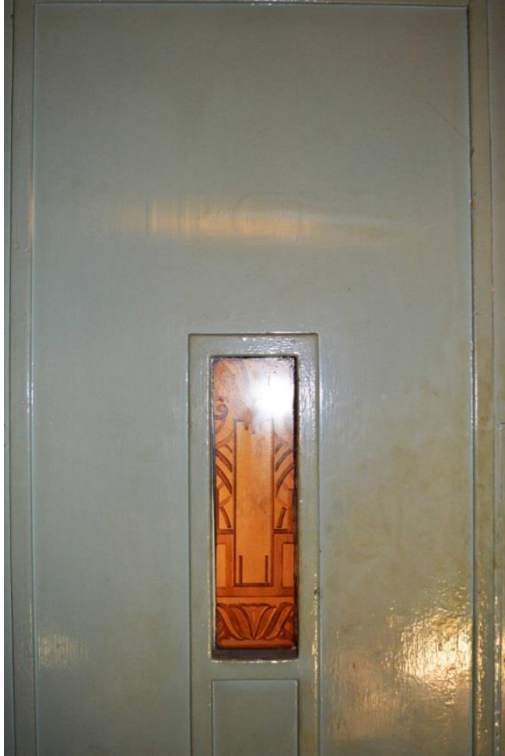
Plate 61: First floor, southern wing, eastern access corridor, glazed door detail and 'Circle' signage, facing north-east (7533_0096)
