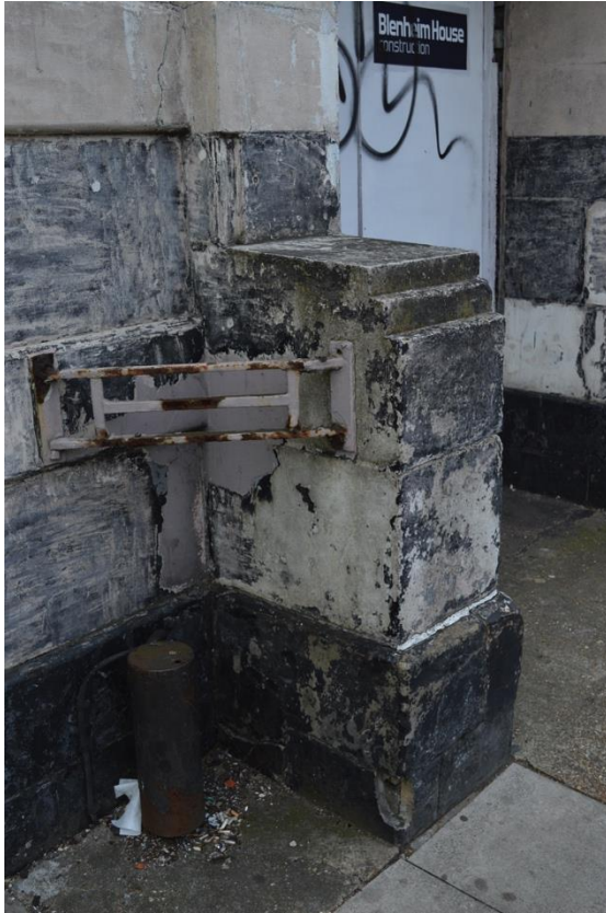
Plate 3: Exterior, west elevation, detail of door buttress and metal tie, facing south-east (7533-0004)
