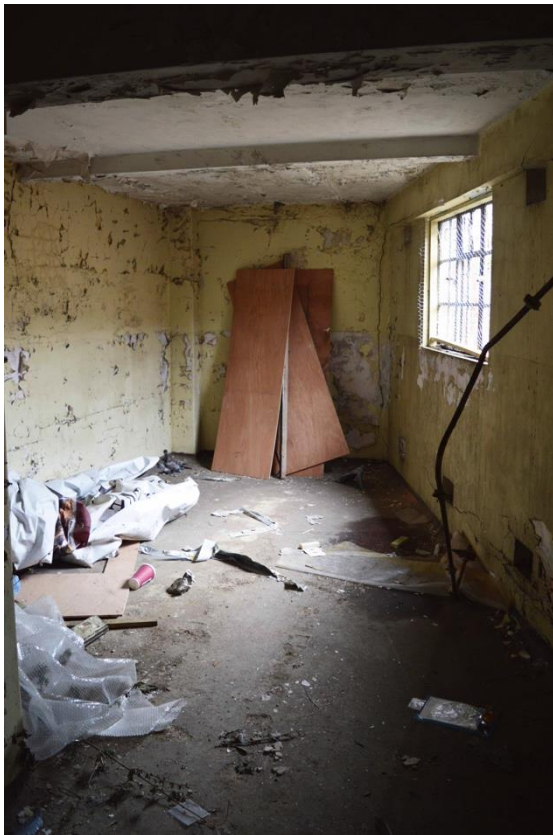
Plate 74: Fourth floor, southern wing, electrical/lighting and sound chamber, facing west (7533_0070)
