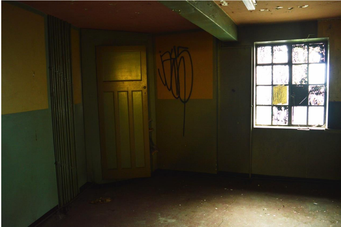
Plate 71: Third floor, southern wing, store room with exhaust chamber beyond, facing east (7533_0081)
