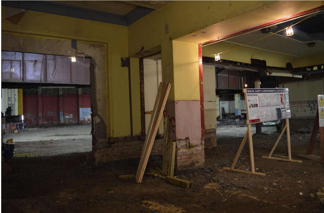
Plate 13: Ground floor, entrance lobby and location of former pay office, facing north-east (7533_0021)
