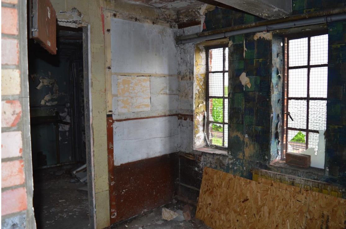
Plate 79: Fourth floor, southern wing, repair room and electrician's store beyond, facing south-east (7533_0073)
