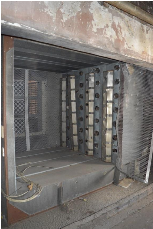
Plate 52: Third floor, east wing, detail of plenum chamber and intake room beyond, facing north-east (7533_0111)
