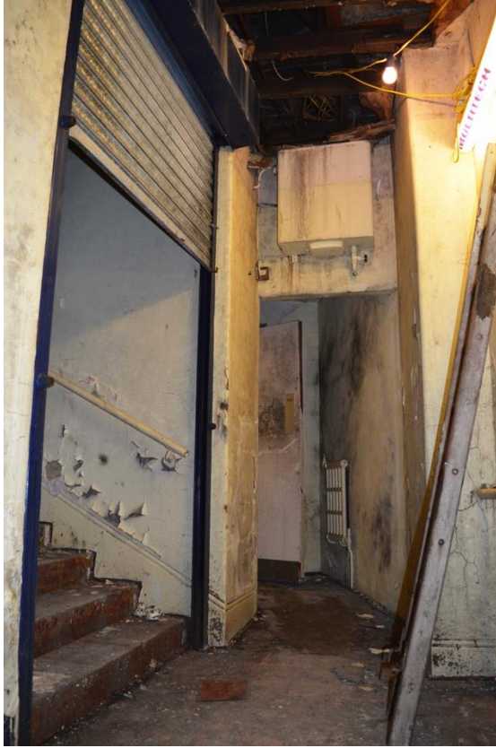
Plate 27: Ground floor, auditorium, western corridor with external door opening and WC, facing north (7533_0100)
