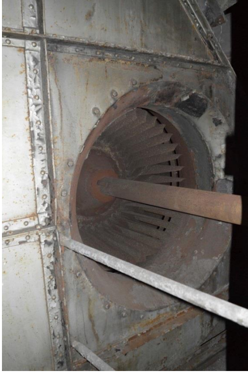
Plate 51: Third floor, east wing, detail of plenum chamber ventilation equipment, facing south-east (7533_0113)
