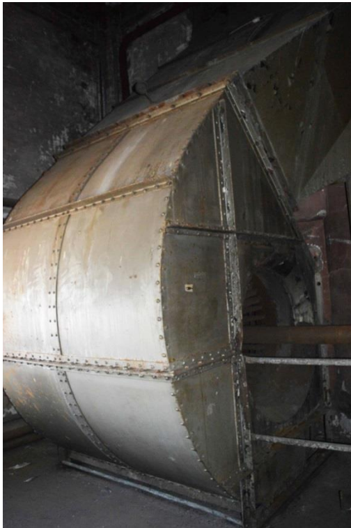
Plate 50: Third floor, east wing, plenum chamber and ventilation equipment, facing south-east (7533_0112)
