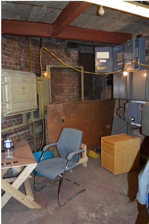
Plate 56: Ground floor, southern wing, electrical intake room, facing west (7533_0052)
