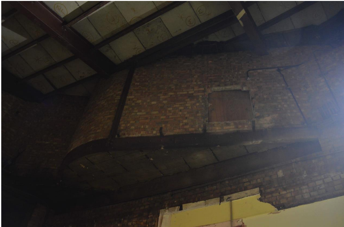
Plate 72: Ground floor, external view of exhaust chamber from the auditorium, facing south-east (7533_0034)
