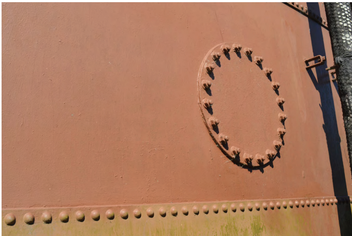
Plate 29: Detail of inspection hatch to the tank's eastern side, facing north-west (TYB15-0016)
