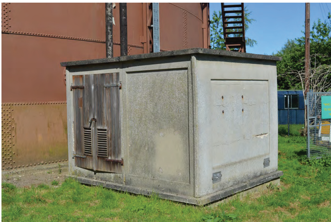
Plate 32: Detail of the concrete housing for the associated plant comprising modular heating pump forming part of the anti-freeze system and E&I equipment, facing north (TYB15-0021)
