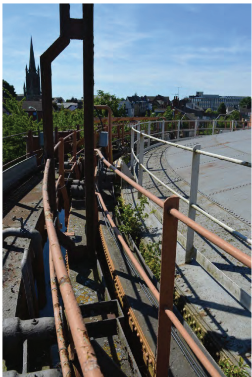
Plate 7: Detail of the three-lift arrangement of the gasholder bell, facing south (TYB15-0028)
