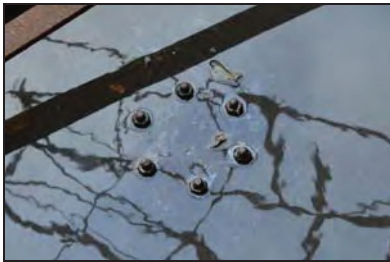
TYB15-0112 Part-submerged fitting. Facing south-west
