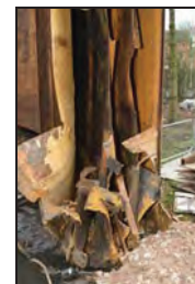
TYB15-0120 Section through lifts and tank wall, note lift cups. Facing south-west
