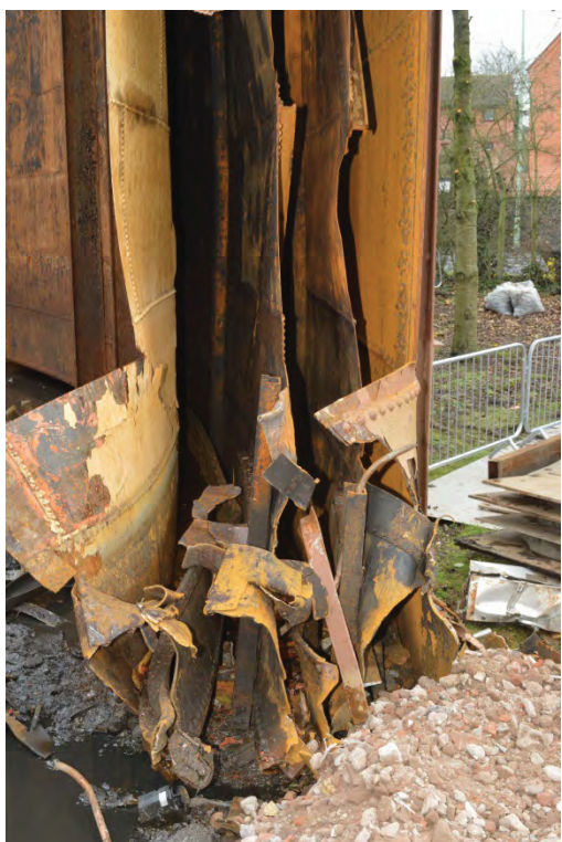
Plate 10: Section through lift and tank wall sheets – not lift cups, facing south-east (TYB15-0120)
