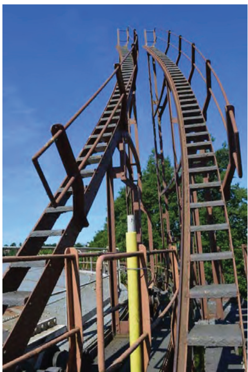
Plate 18: Detail of angled handrail to the first and third lift access stairs, facing north-west (TYB15-0039)
