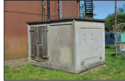
TYB15-0021 Concrete housing for associated plant. Facing west
