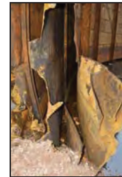
TYB15-0117 Section through lifts and tank wall, note lift cups. Facing north-west
