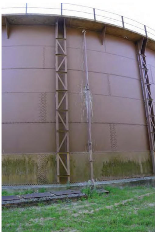
Plate 30: Detail of the water overflow pipework and associated ground drainage to the tank's northern edge, facing south (TYB15-0010)
