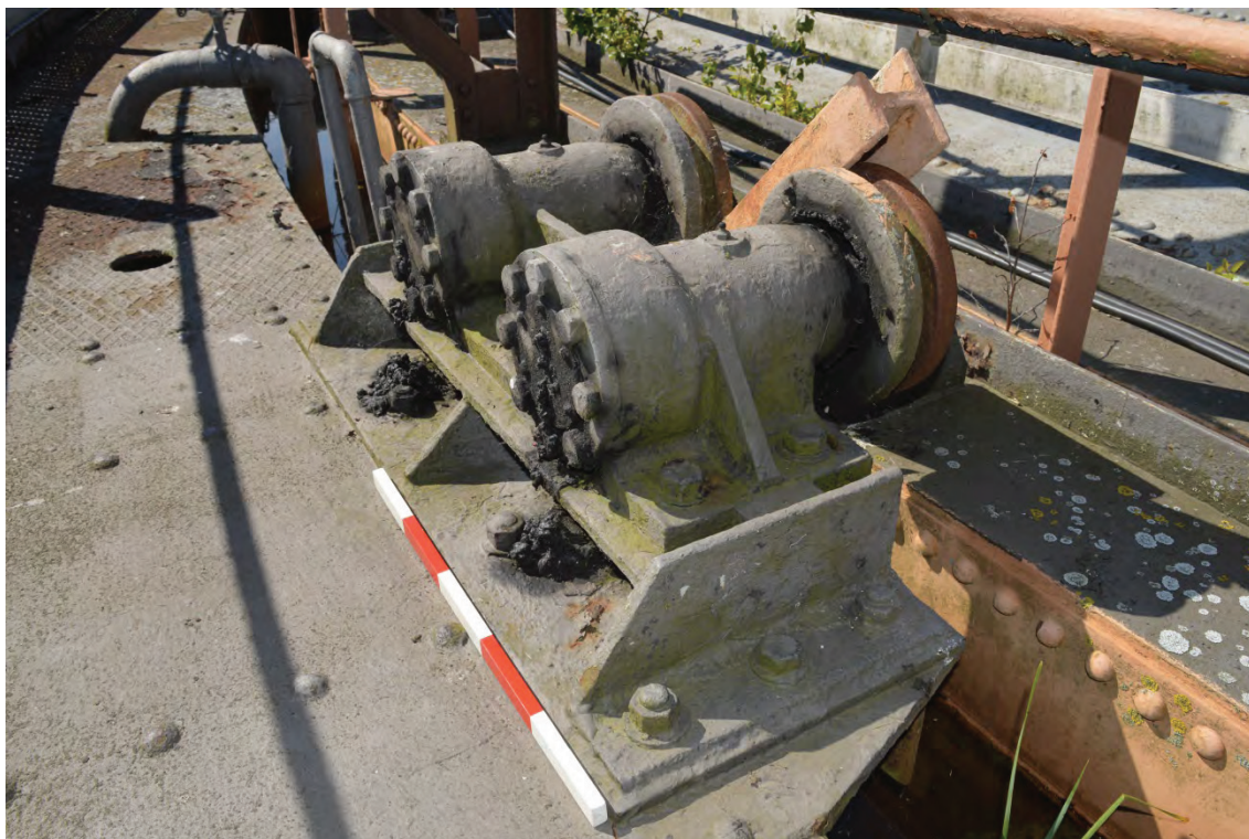
Plate 11: Detail of electrical anti-freeze pump system, dated 1988, located on the middle lift wall, facing west (TYB15-0032)
