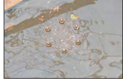
TYB15-0111 Part-submerged fitting. Facing south-west
