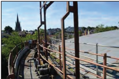
TYB15-0025 Tank platform. Facing south
