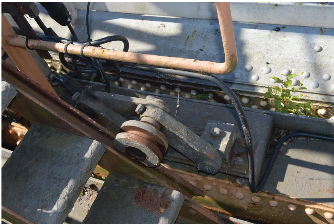
Plate 19: Detail of staircase guide carriage located on the middle lift, facing south-west (TYB15-0034)
