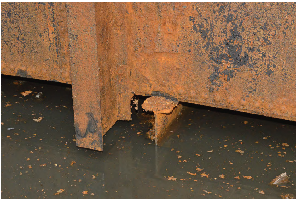
Plate 9: Detail of the inner lift resting on I-girder support, facing north-east (TYB15-0097)
