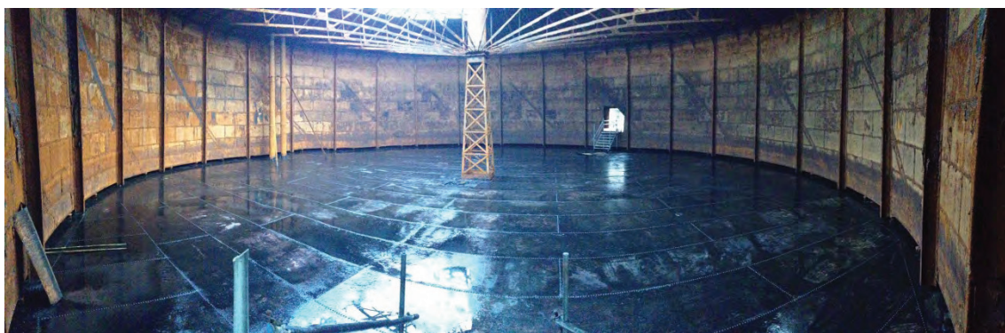
Plate 2: General view of the interior of the gasholder, facing west – provided by the client (TYB15-0128)
