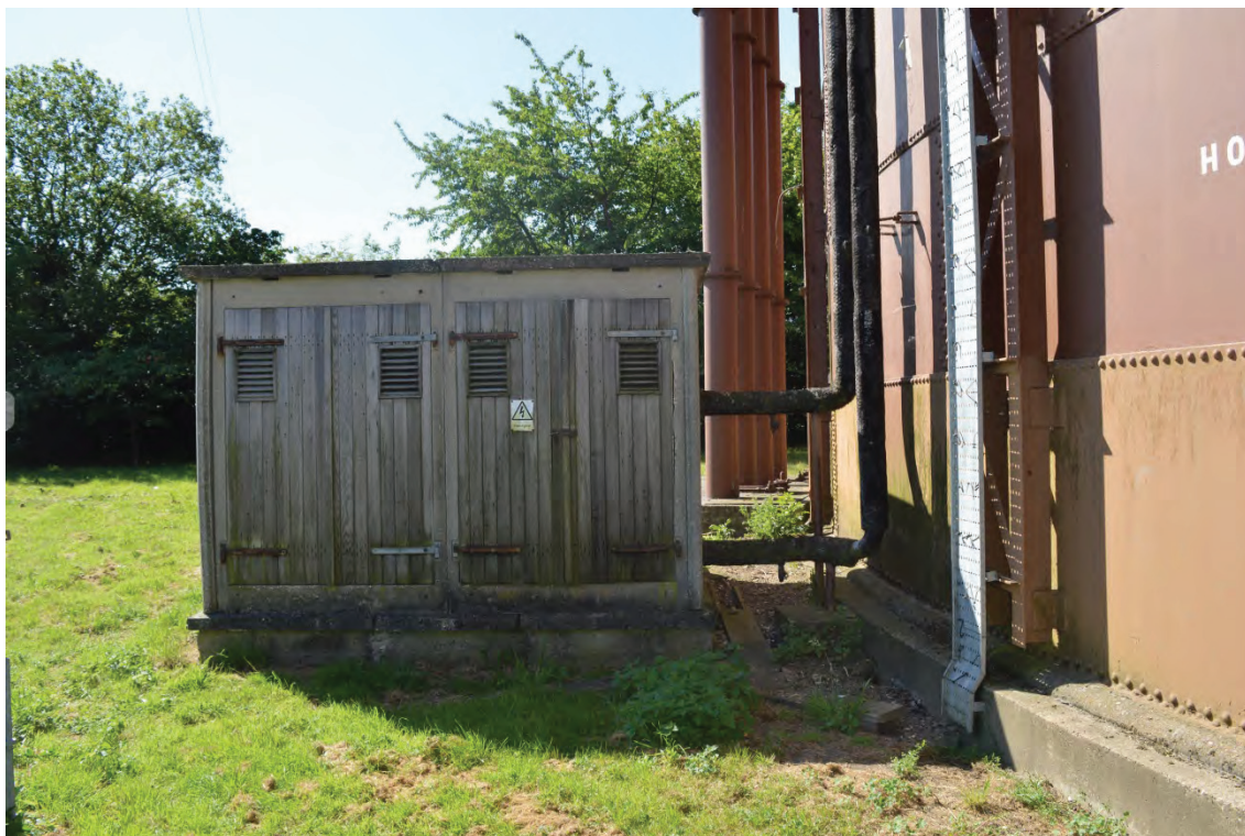
Plate 31: Detail of the concrete housing and pipework for the modular heating pump forming part of the anti-freeze system, facing south (TYB15-0020)
