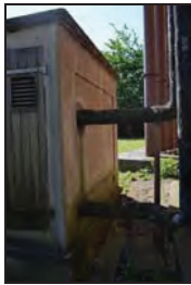
TYB15-0022 Concrete housing and pipework for modular heating pump. Facing south
