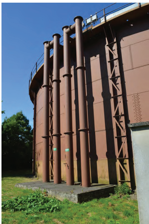
Plate 28: Detail of the inlet and outlet gas mains pipework to the tank's eastern side, facing south-west (TYB15-0017)
