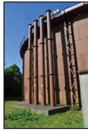
TYB15-0017 Inlet/outlet gas mains pipework. Facing south-west
