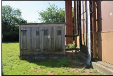
TYB15-0020 Concrete housing for associated plant. Facing south
