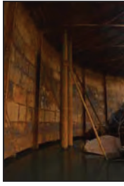
TYB15-0106 Pipes within gasholder. Facing south-east
