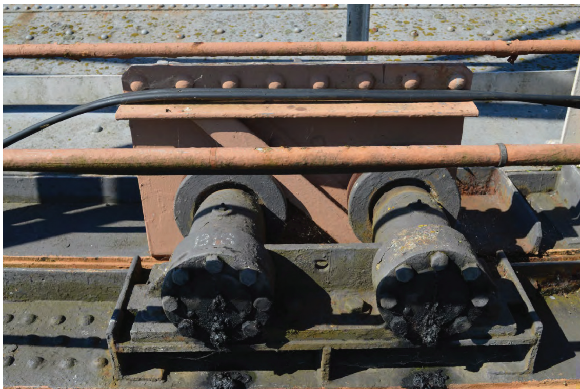
Plate 13: Detail of carriage wheel and guide rail construction fixed to the second (middle) lift, facing west (TYB15-0031)
