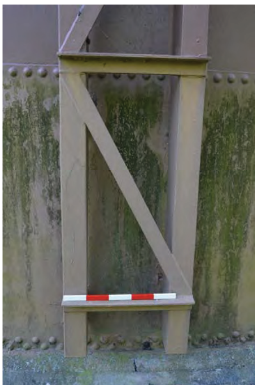
Plate 22: Detail of vertical reinforcements situated around the tank's outer edge, facing south (7374_0015)
