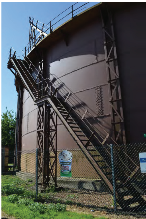
Plate 23: Detail of staircase providing access to the tank platform from ground level, facing south-west (TYB15-0002)
