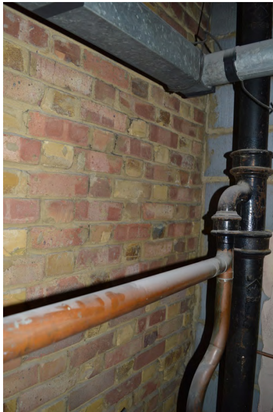
Plate 42: Fabric of the original building within void in room 130, 154 Bayswater Road (Photo 13).
