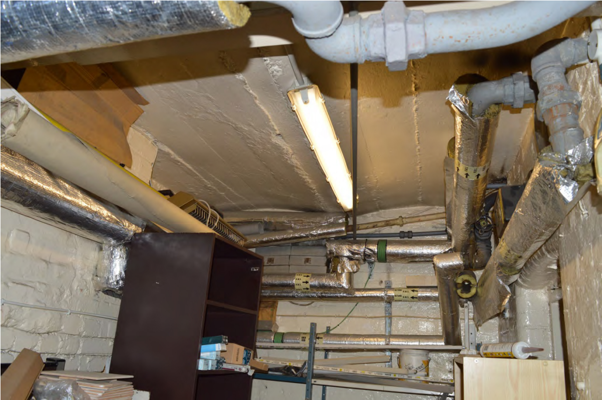
Plate 14: Reinforced concrete vaulting in a store within the basement, 154 Bayswater Road (Photo 180).
