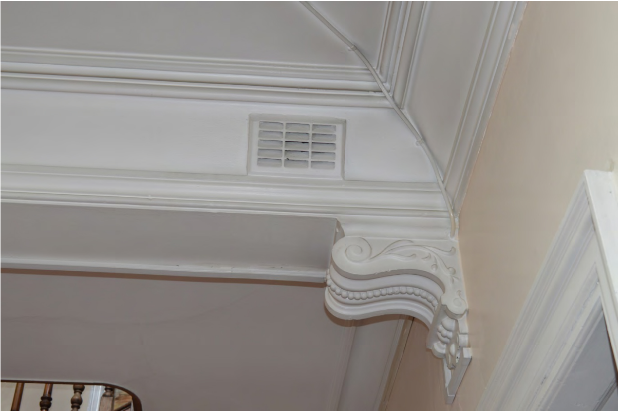
Plate 54: Console brackets on girder on the second floor landing, 6 Palace Court (Photo 284).
