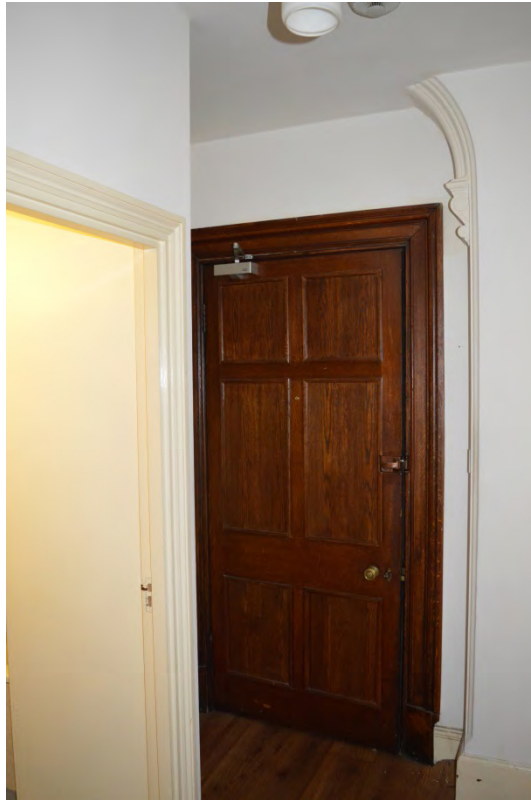
Plate 52: Blind arch truncated by an inserted ceiling in room 138, 6 Palace Court (Photo 334).
