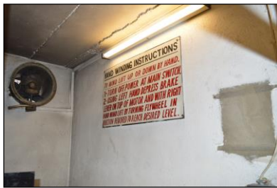
7330-0004 7330_Lift Motor Room. Facing south-east
