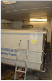
7330-0001 7330_Tank Room. Facing west
