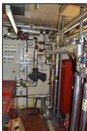
7330-0403 7330_Boiler Room. Facing east
