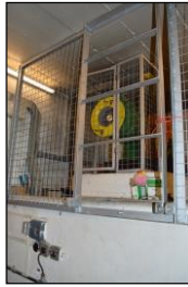
7330-0002 7330_Lift Motor. Facing north
