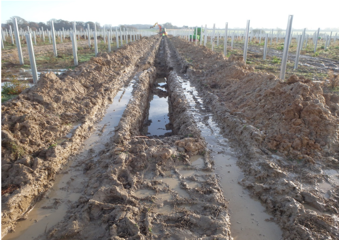
Figure 5: General view of cable trench under excavation illustrating poor ground conditions – November 2014.
