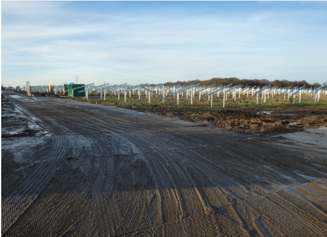
Figure 2: Temporary roads formed from mesh matting laid directly on the existing ground surface.
