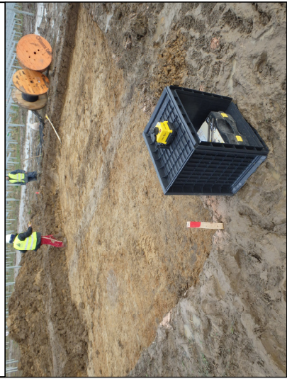
Gully 006, 1m scale
