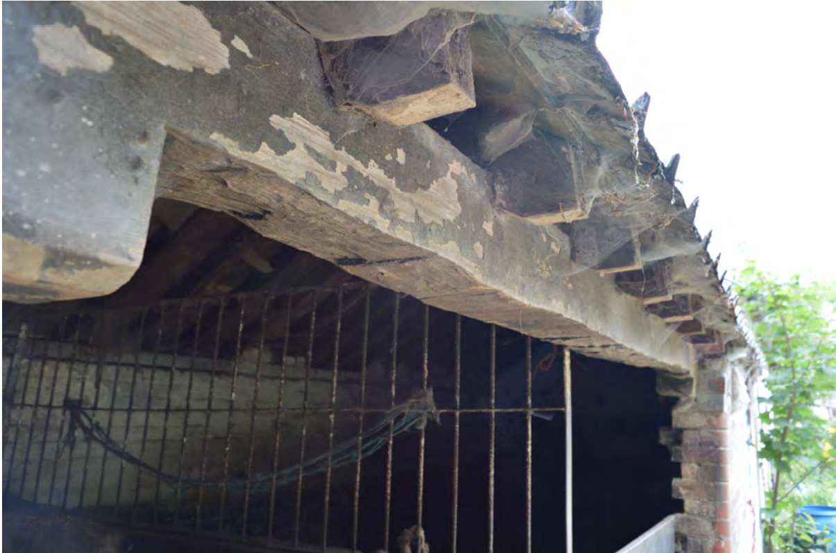
Plate 31: Timber beam above the entrance to the southern half of the central building (Photo #14).
