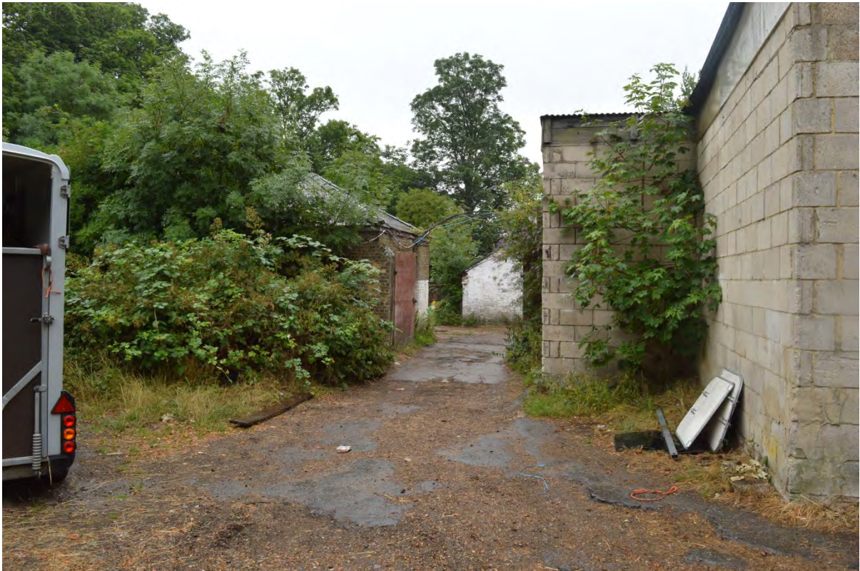
Plate 1: Principal elevation of the piggery – largely masked by vegetation and later development (Photo #128).
