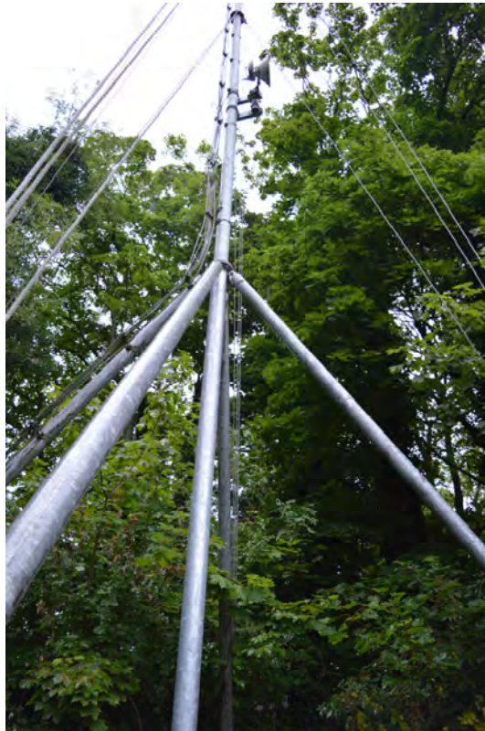
Plate 41: Communications mast (Photo #87).
