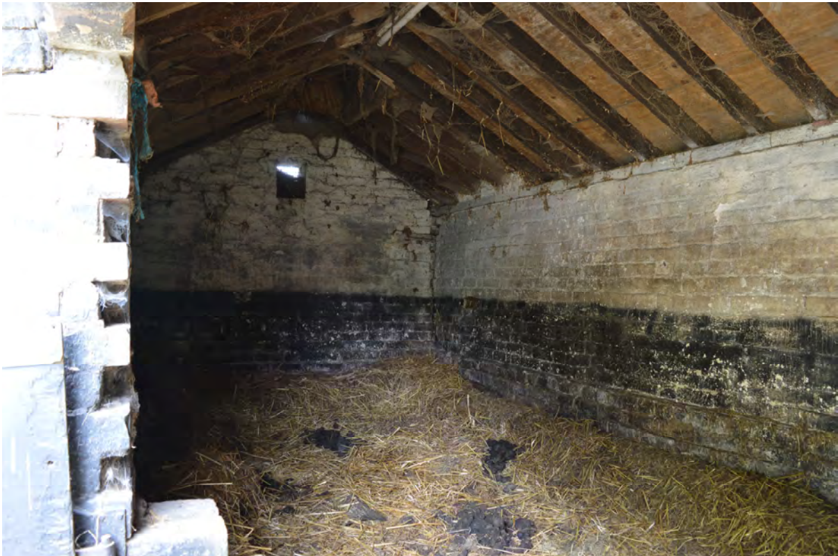
Plate 33: Stable in south of the central building – note the roof and upper walls (Photo #10).
