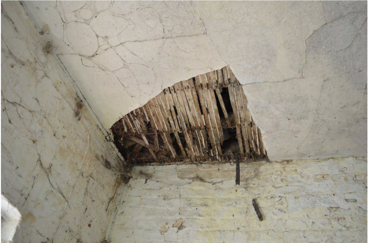
Plate 9: Exposed lath and plaster ceiling (Photo #29).
