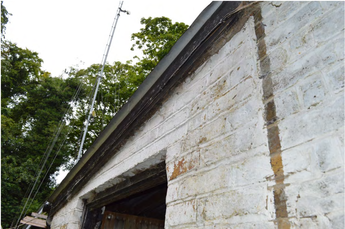
Plate 11: Inserted shed roof and brickwork at the west end of the western storage/tack building (Photo #55).
