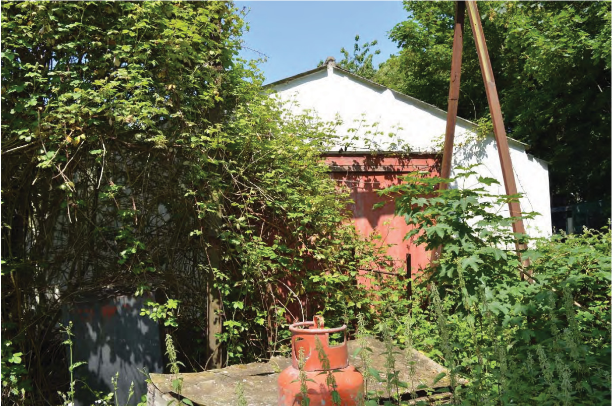
Plate 13 Large doorway at south-eastern end of rear range of Building 1, viewed externally (11)
