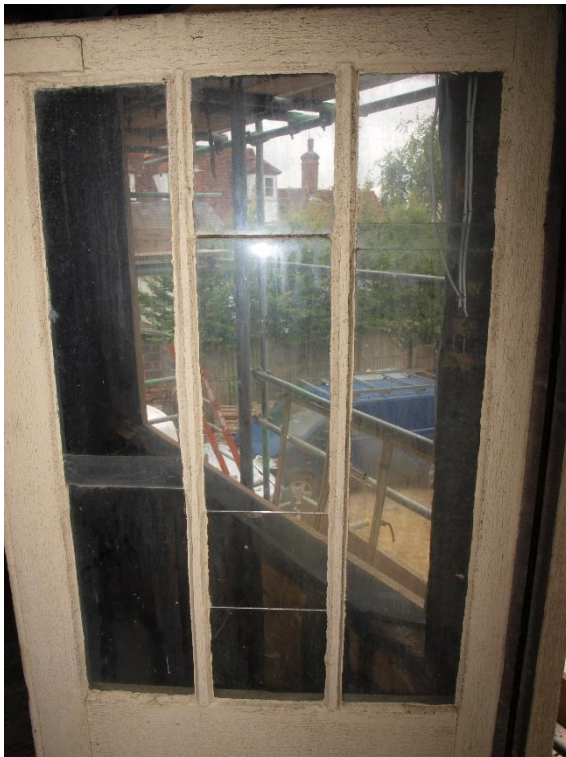
Plate 4: Detail of the overlapped glazed light arrangement found throughout the building, facing north-west (7790_025)
