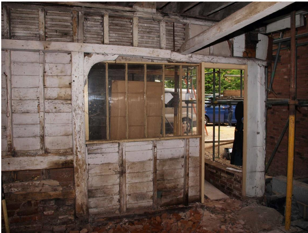
Plate 12: Detail of the north end of the partition wall (east side) with retained arch brace, facing north-west (7790_045)
