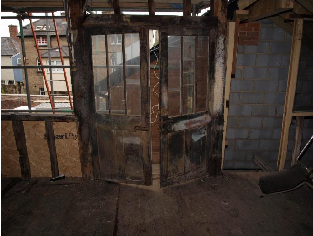
Plate 9: Detail of the northern loading door at first floor level, facing north (7790_014)
