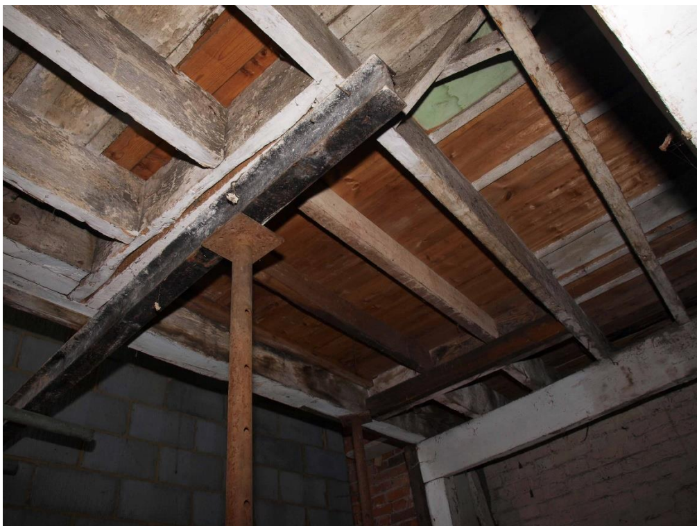
Plate 20: Detail of the location of an earlier internal stair within the north-east corner, facing north-east (7790_053)
