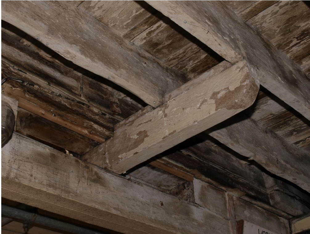
Plate 27: Detail of the cantilever to the former loading platform at first floor level, facing north-east (7790_032)
