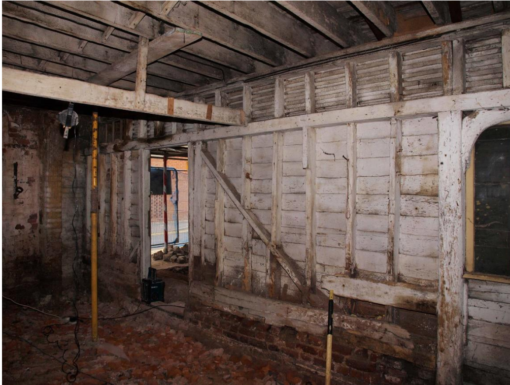
Plate 13: Detail of the east side of the partition wall construction at ground floor level, facing south-west (7790_044)
