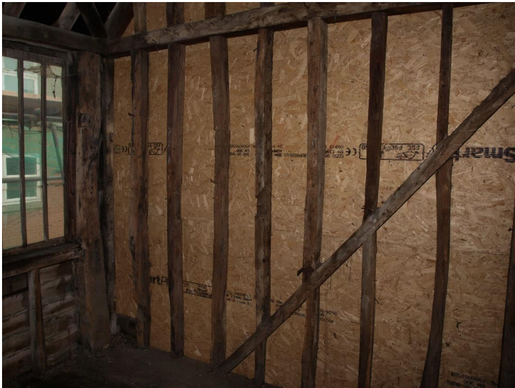
Plate 30: Detail of the timber framing of the western wall at first floor level, facing south-west (7790_027)
