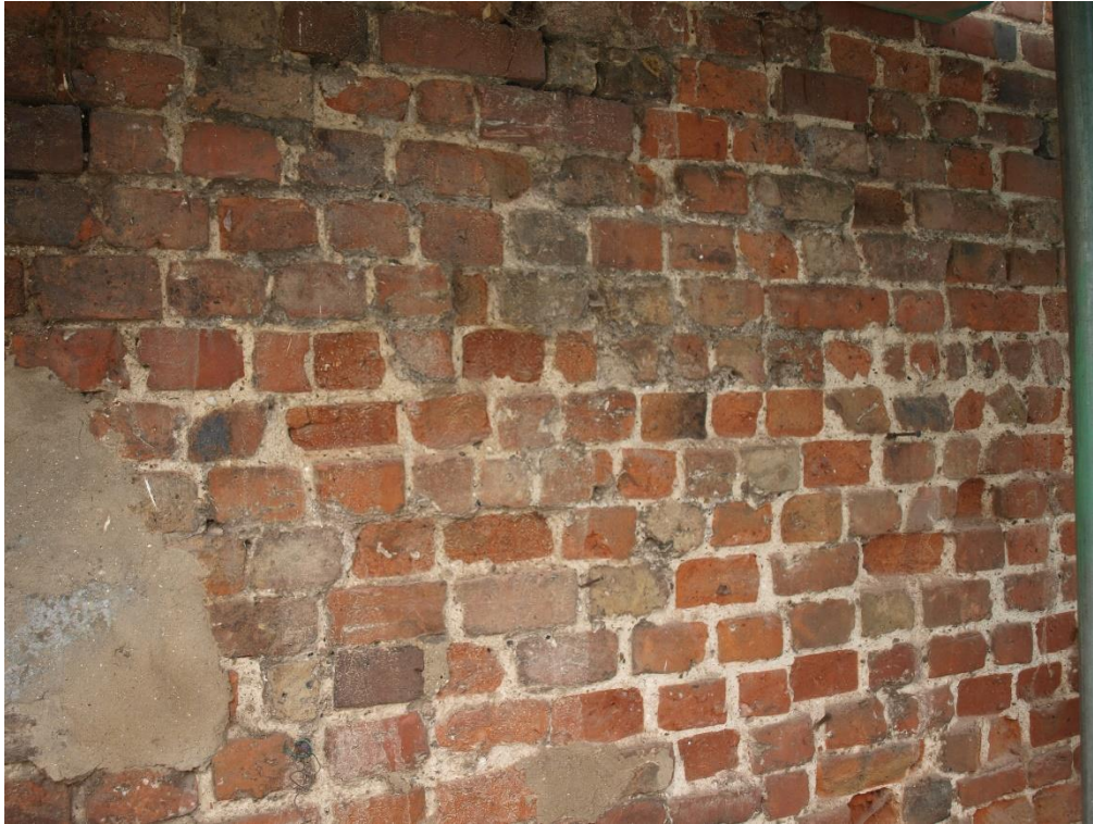
Plate 5: Exterior, detail of the two phases of brickwork to the lower level of the west elevation, facing south-east (7790_006)
