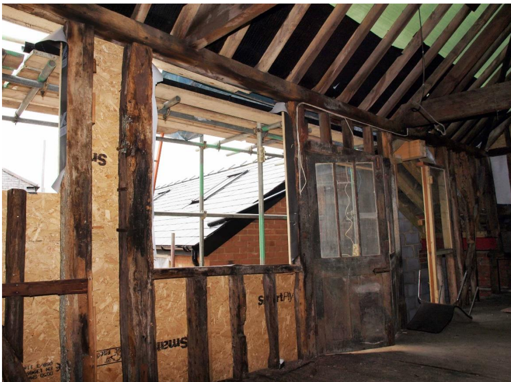
Plate 34: Detail of the door and window arrangement within the north elevation at first floor level, facing north-east (7790_022)
