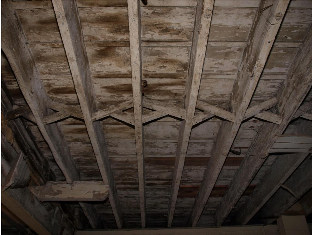
Plate 19: Detail of the floor joists supporting the first floor level, facing east (7790_031)
