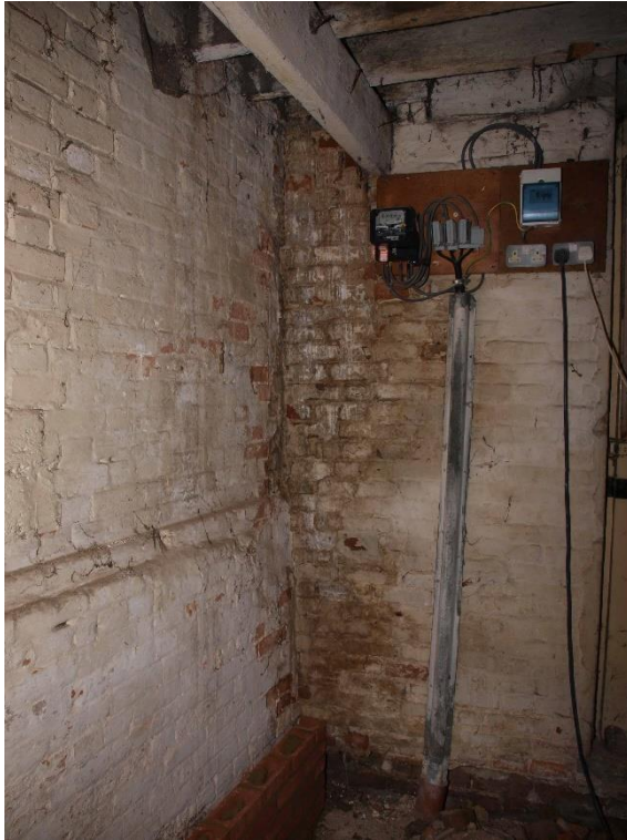
Plate 17: View of the brickwork construction on the eastern wall at ground floor level, facing south-east (7790_046)
