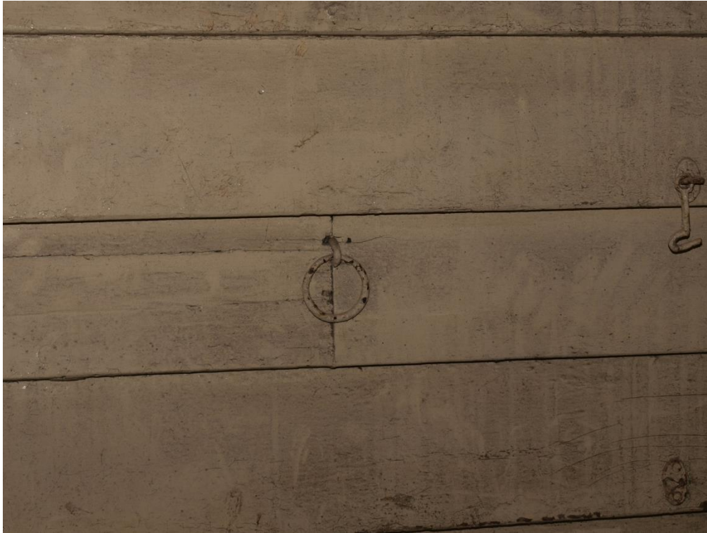
Plate 23: Detail of the retained tethering ring on the partition wall (west side), facing east (7790_035)
