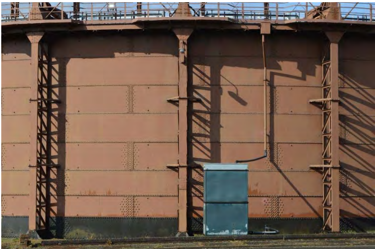
Plate 58: Gasholder No. 3, detail of the above-ground steel tank and water overflow pipe, facing west (71)
