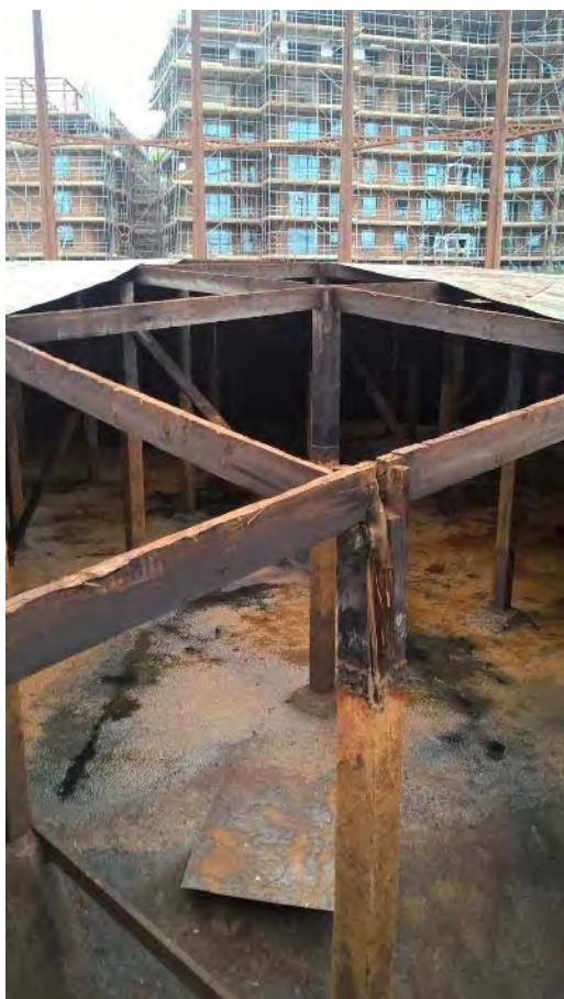
Plate 23: Gasholder No. 1, internal detail of the timber frame supporting the underside of the crown, facing west (476)
