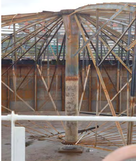
Plate 41: Gasholder No. 2, detail of the central stanchion and tension ties, facing north-east (294)
