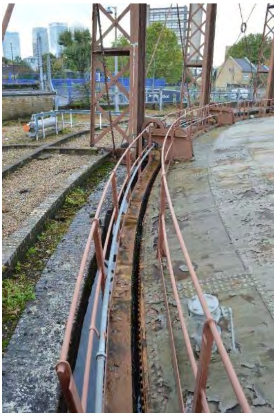
Plate 28: Gasholder No. 1, arrangement of the two lifts with associated lute, served by guard rails, facing south (174)
