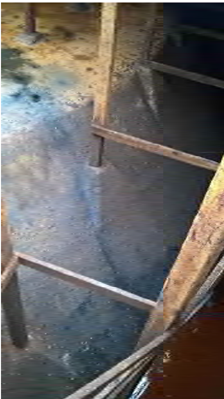
Plate 26: Gasholder No. 1, detail of the beam bracing supporting the outer rim of post supporting the underside of the crown, facing north-west (479)
