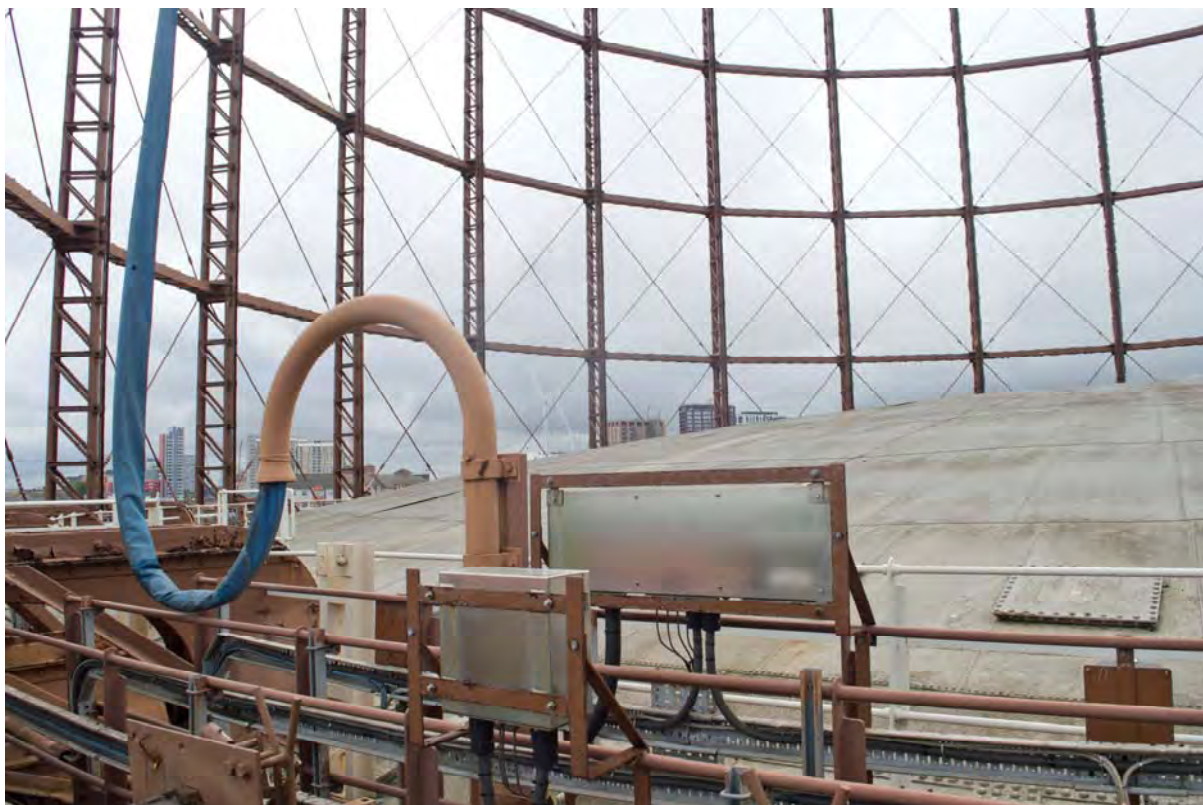
Plate 89: Gasholder No. 3, detail of the shepherd's-crook cable guides for the pressure alarm monitoring equipment, facing north-east (332)
