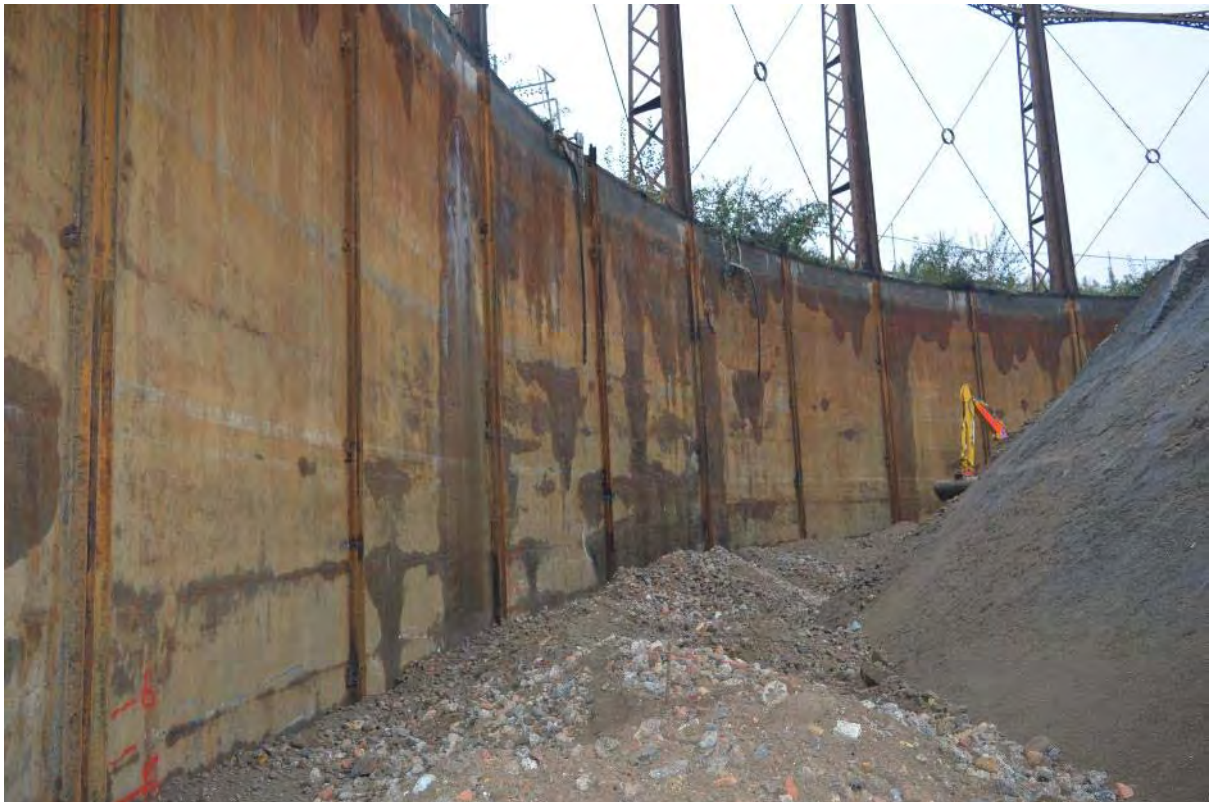
Plate 17: Gasholder No. 1, detail of the inner face of the inner lift wall, note the stanctions used to house their associated lift rollers, facing south (401)
