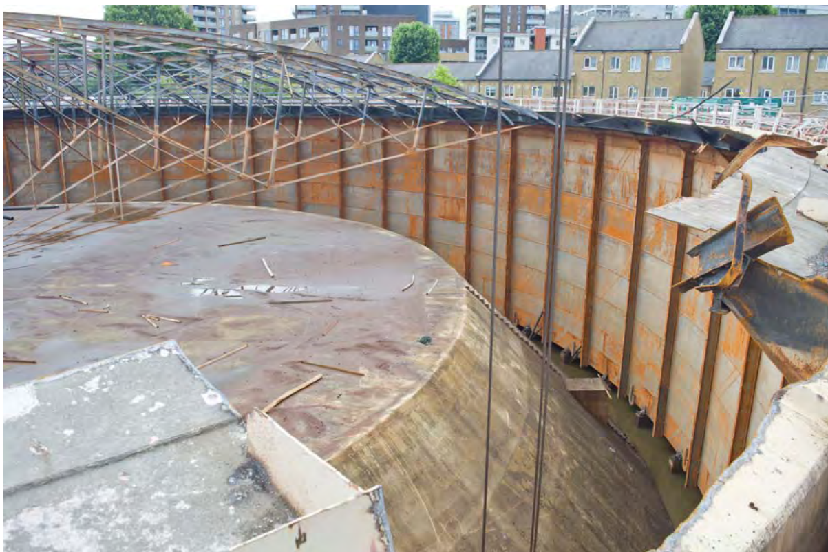
Plate 42: Gasholder No. 2, interior view of the inner lift wall stanchions and bell trusses, facing south-west (309)
