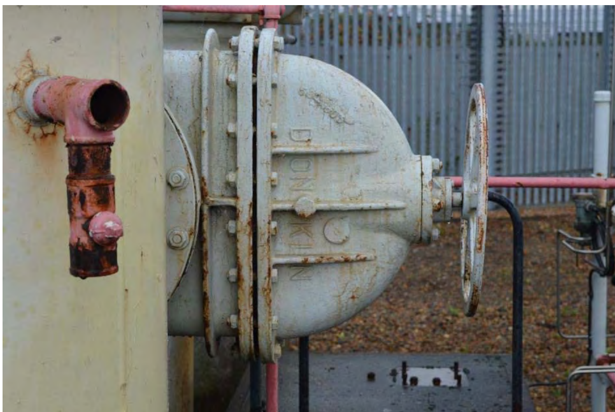
Plate 56: Gasholder No. 2, detail of the 'Donkin' gas distribution pipework to the north-east of the holder, facing north (20)
