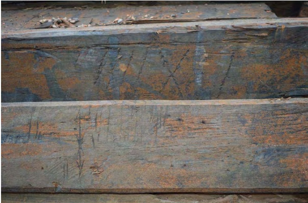
Plate 27: Gasholder No. 1, carpentry marking upon a selection of timber posts formerly supporting the underside of the crown (post-deconstruction), facing north (451)
