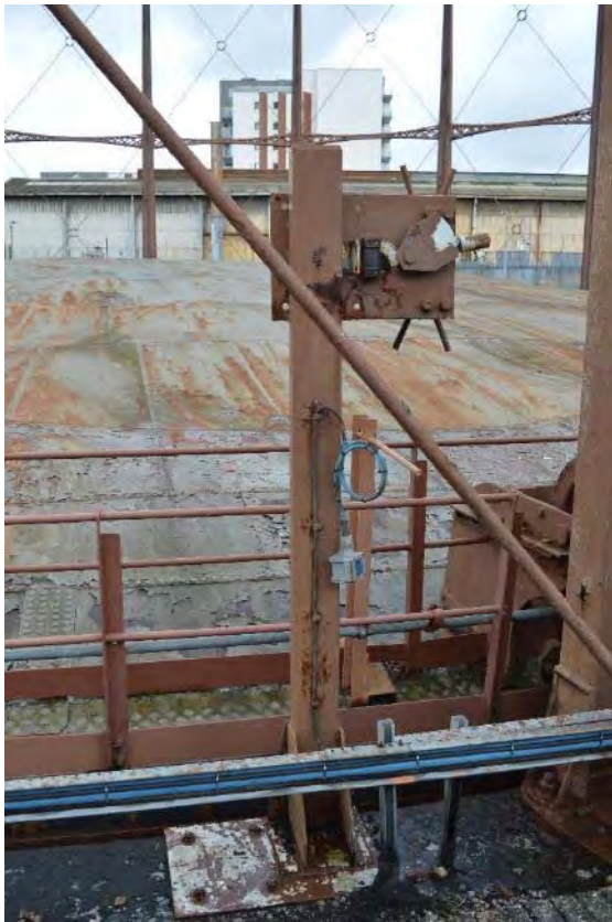
Plate 33: Gasholder No. 1, detail of the upright supports for the pressure alarm system, facing south-west (181)
