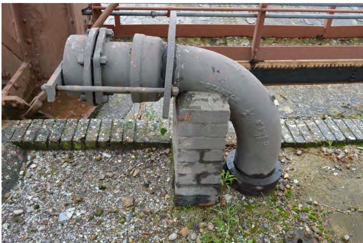
Plate 20: Gasholder No. 1, ancillary pipework located to the northern edge of the gasholder (presumably gas inlet/outlet valve), facing south (197)
