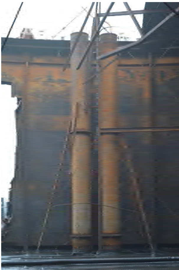
Plate 62: Gasholder No. 3, view of the paired pipes set within the tank interior to the west side, facing north-west (374)
