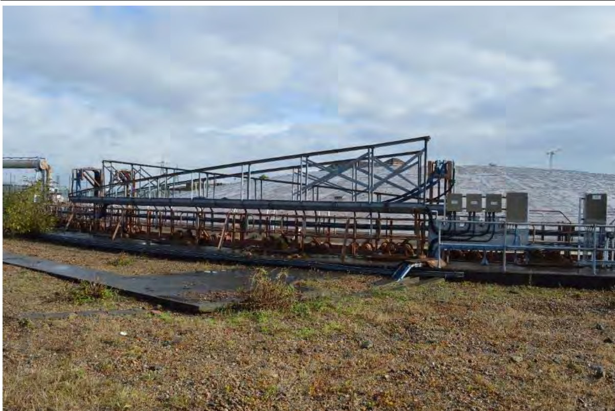
Plate 47: Gasholder No. 2, extendible steel supports serving the water monitoring equipment, facing north-east (40)
