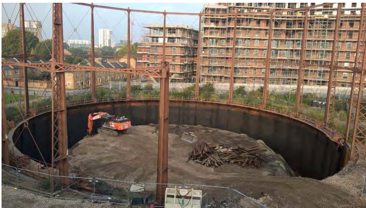
Plate 14: Gasholder No. 1, view of the tank dumping following deconstruction works, facing south-west (491)
