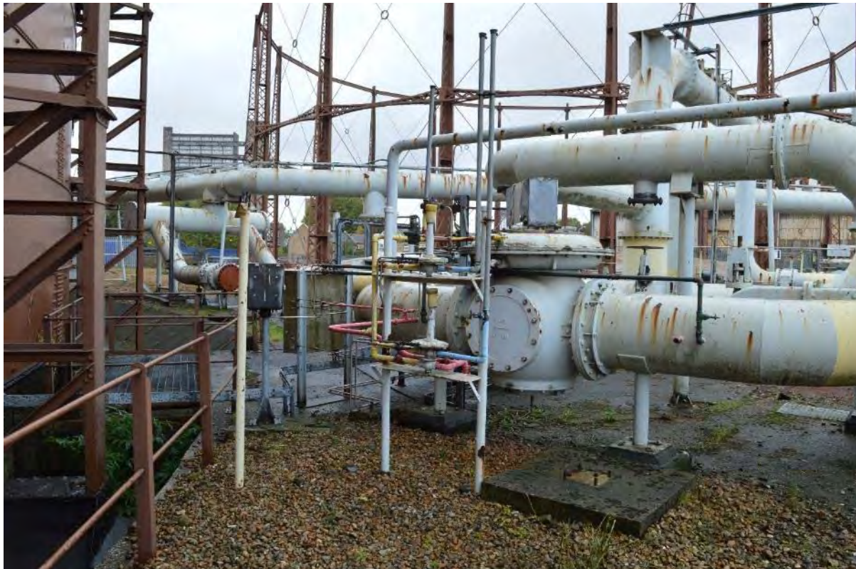
Plate 90: General view of the retained 'Donkin' gas distribution pipework located between Gasholders 1 & 3, facing south-west (104)
