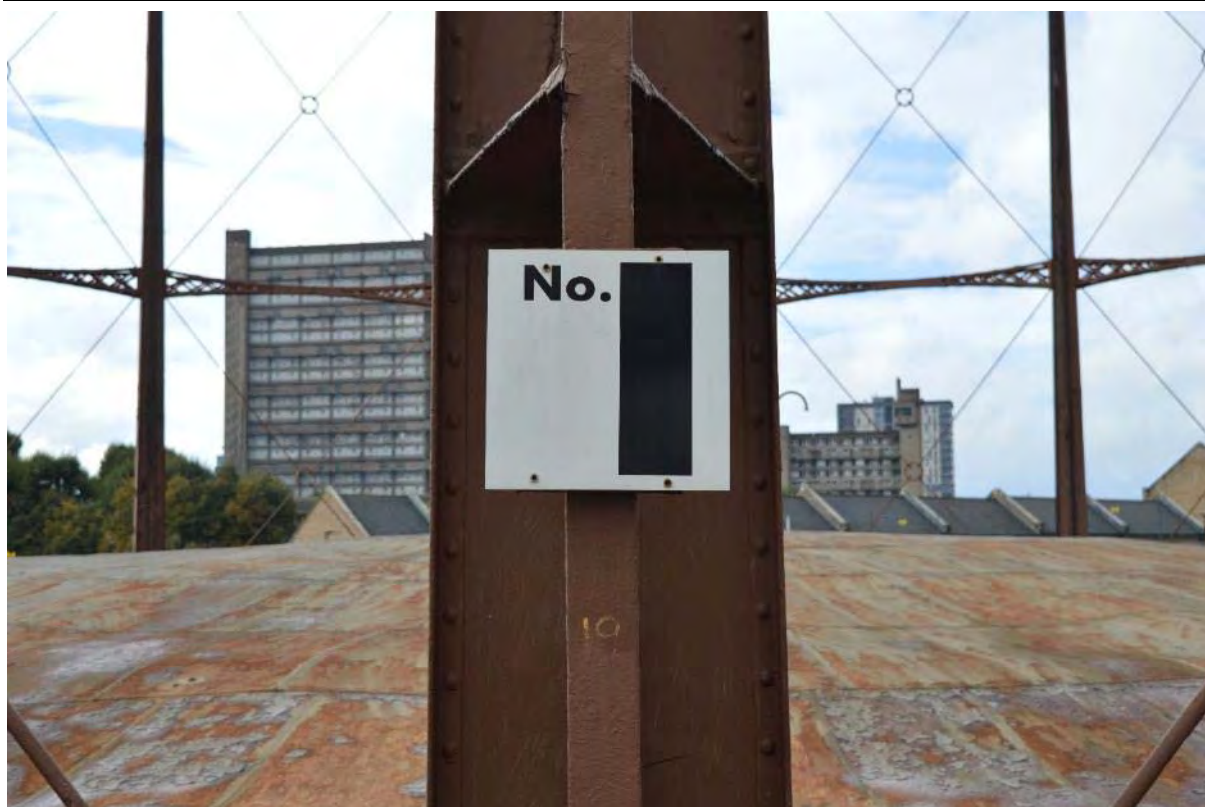
Plate 11: Gasholder No. 1, modern identification signage located to the north of the structure's edge, facing south-west (193)
