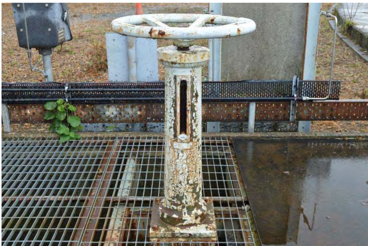
Plate 55: Gasholder No. 2, detail of the gas mains manual valve wheel to the north-west of the holder, facing north (19)
