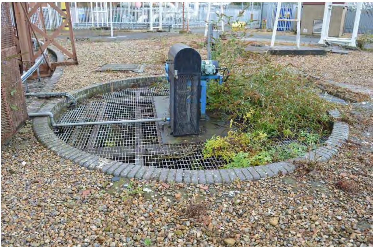
Plate 18: Gasholder No. 1, dry-well with operational syphons located to the north-east edge of the gasholder, facing north (184)
