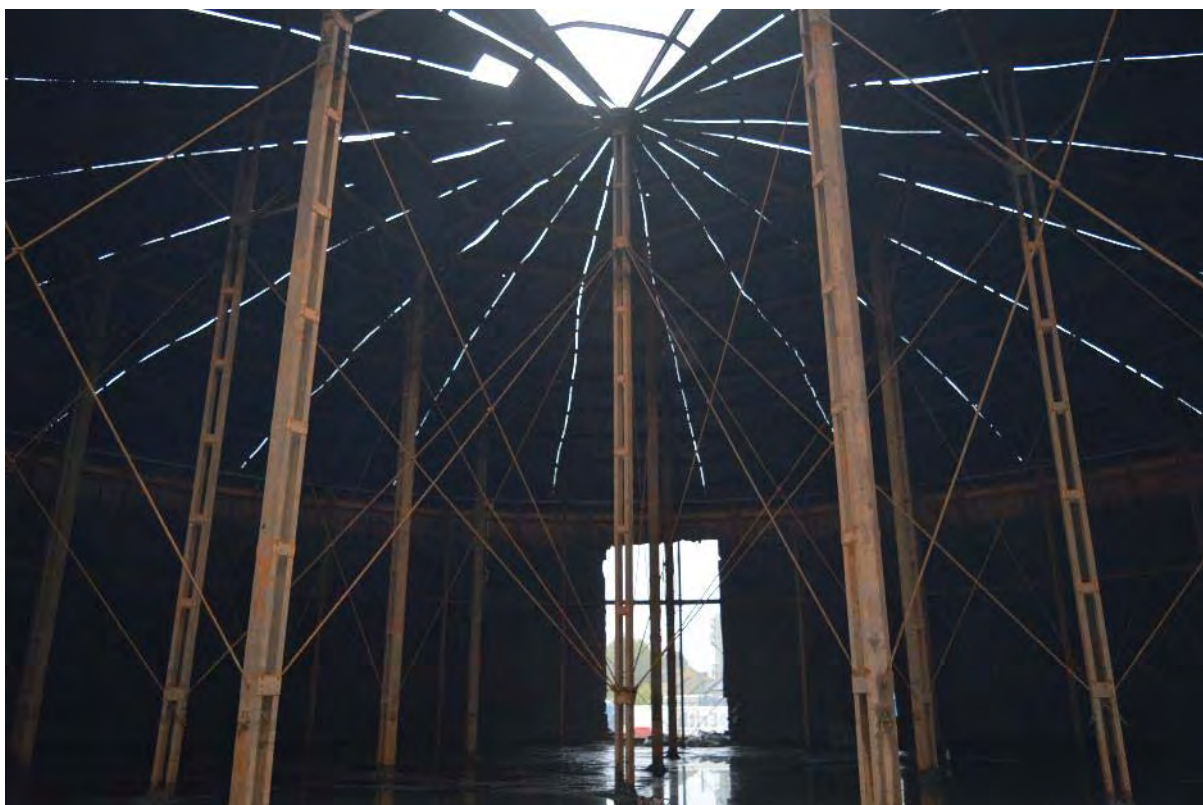
Plate 81: Gasholder No. 3, view of the steel framework which supports the underside of the crown, note hole in tank created for access during deconstruction, facing east (357)
