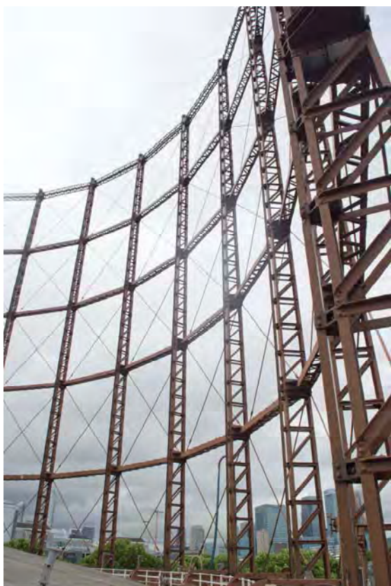
Plate 73: Gasholder No. 3, view of the guide frame stanchions and tension ties, facing north-west (330)
