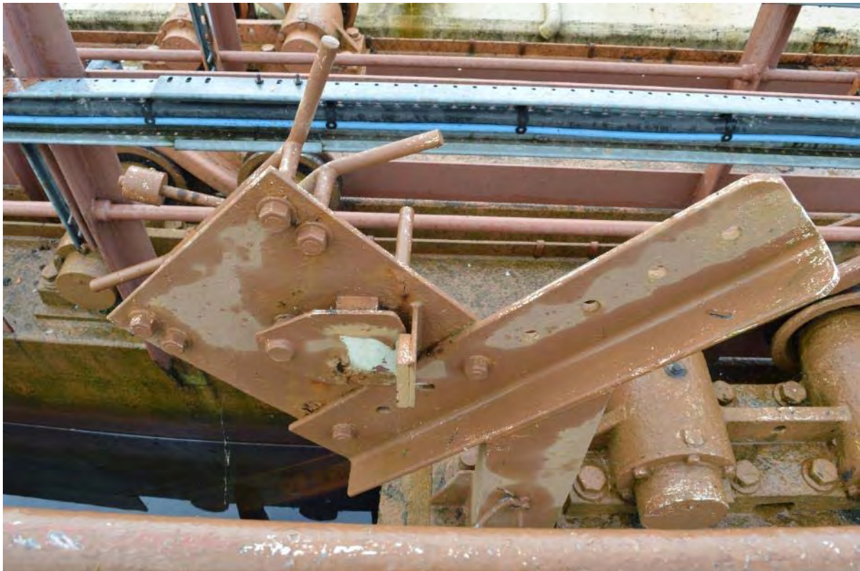
Plate 45: Gasholder No. 2, detail of pressure alarm system supports, facing south (26)
