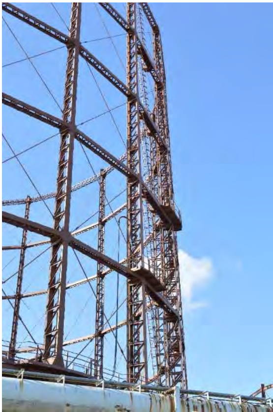
Plate 72: Gasholder No. 3, detail of the tapered guide frame standard panels, facing south-west (62)
