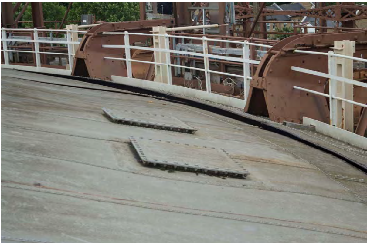
Plate 80: Gasholder No. 3, detail of the sheeting and inspection hatches within the northern side of the crown, facing west (243)
