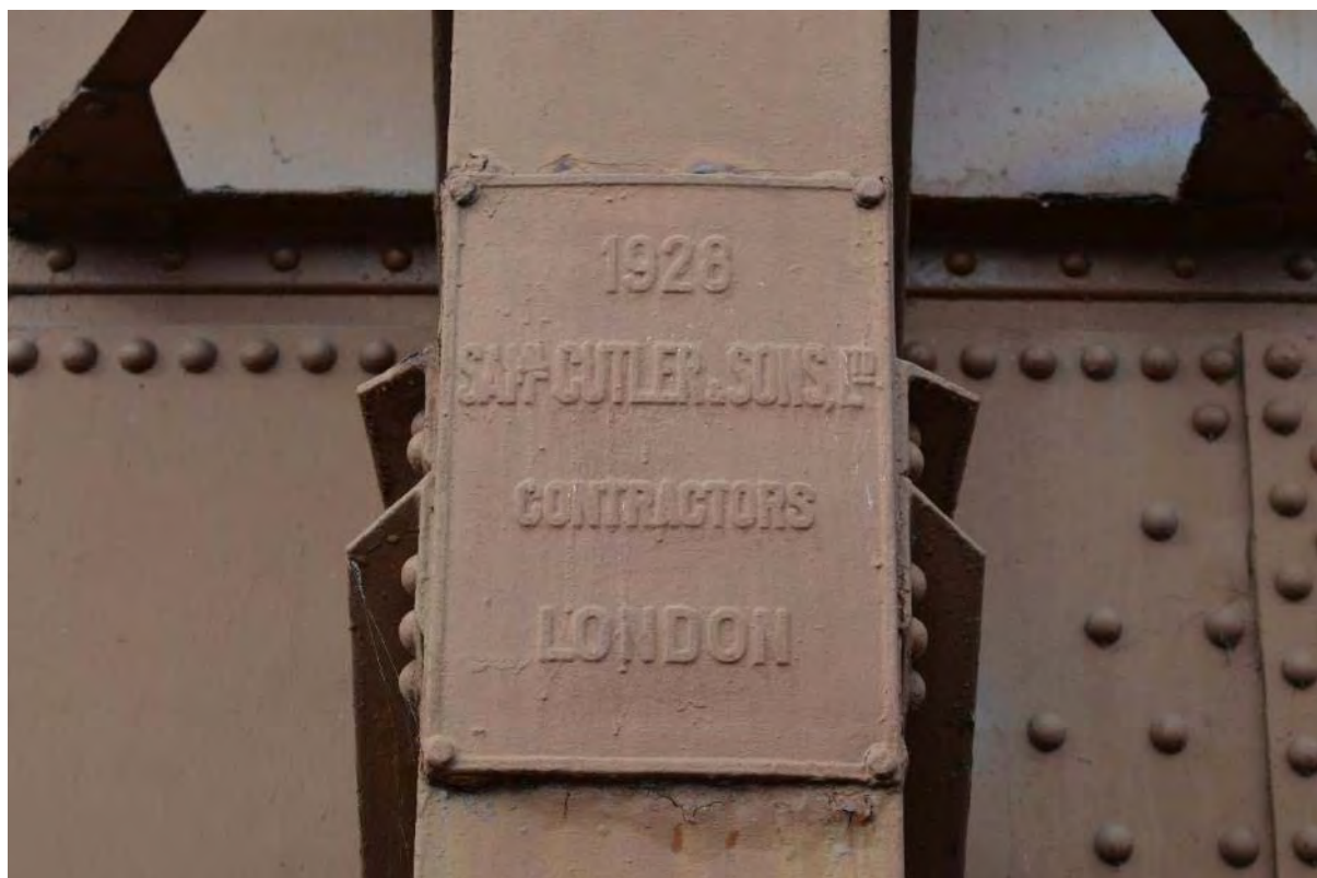
Plate 65: Gasholder No. 3, detail of the eastern edge Cutler identification plaque, facing west (85)
