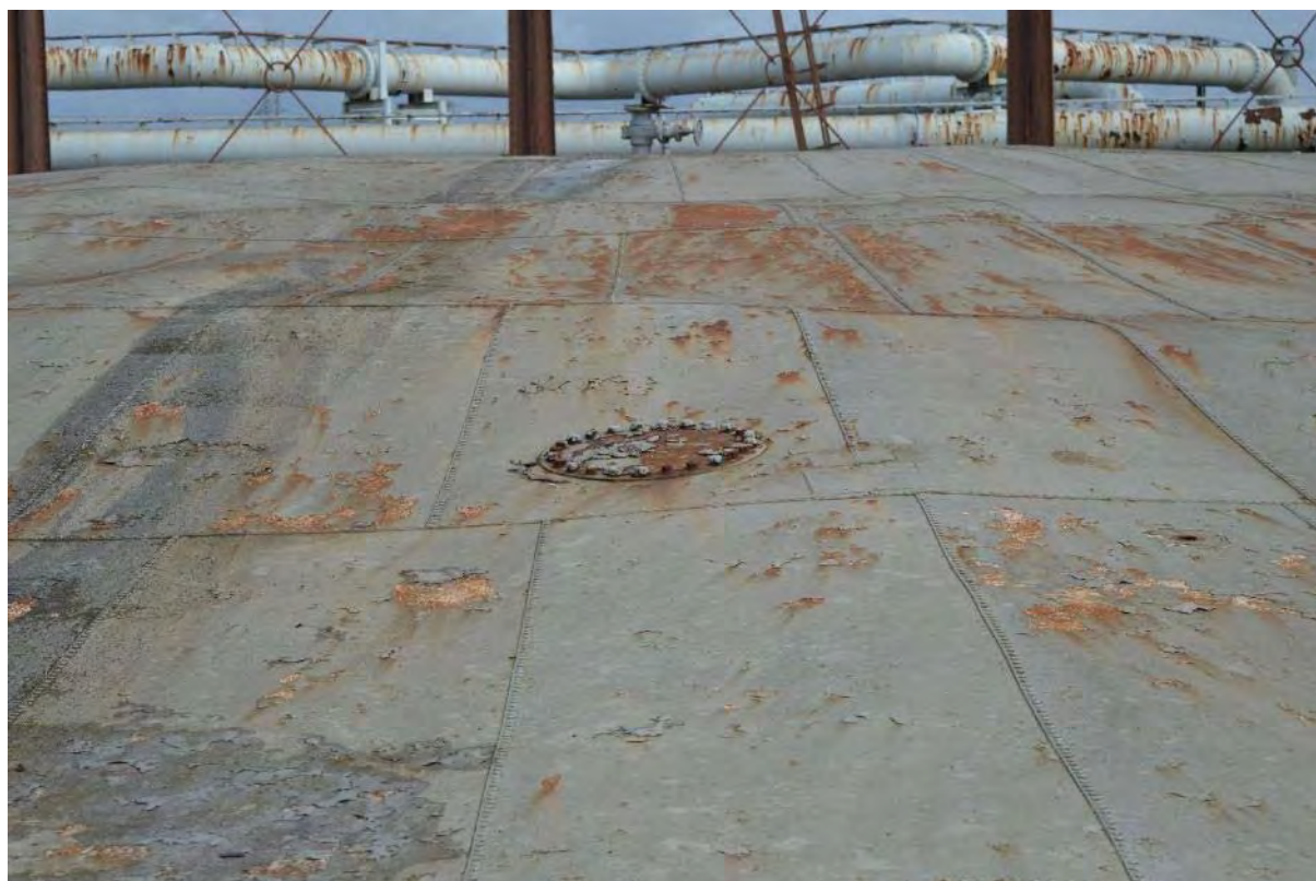
Plate 22: Gasholder No. 1, riveted circular hatch located on the gasholder bell, facing north-east (210)
