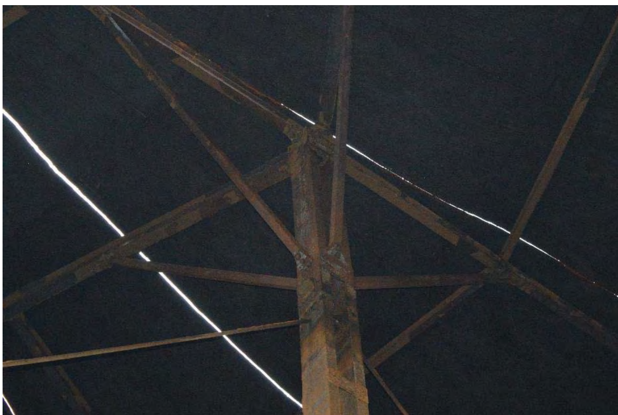
Plate 82: Gasholder No. 3, detail of the raking struts connecting the uprights to the L-section girders, which create the support framework to the underside of the crown, facing south-east (376)
