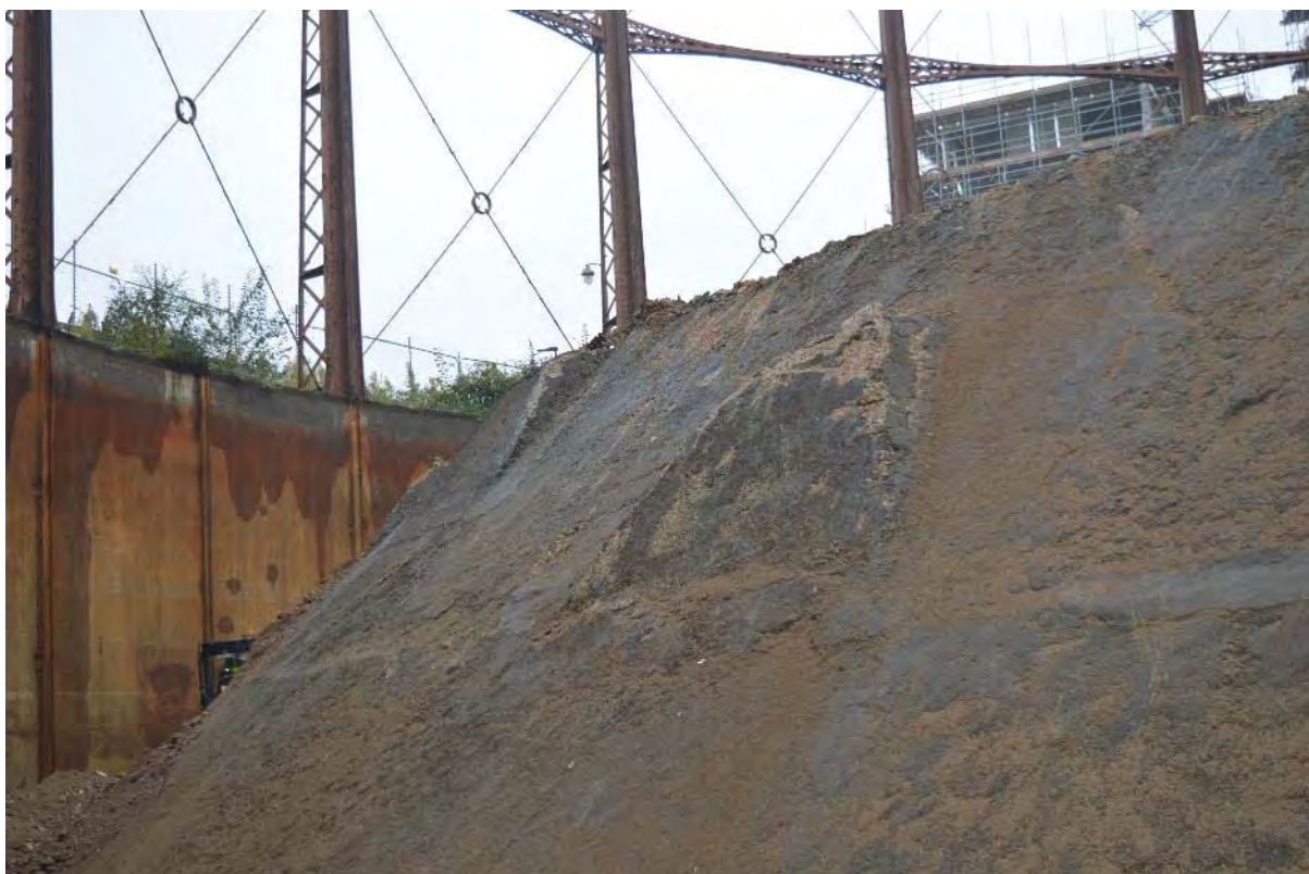
Plate 16: Gasholder No. 1, detail of the dumping concrete platforms used to secure the former timber framework supporting the underside of the crown, facing south (406)
