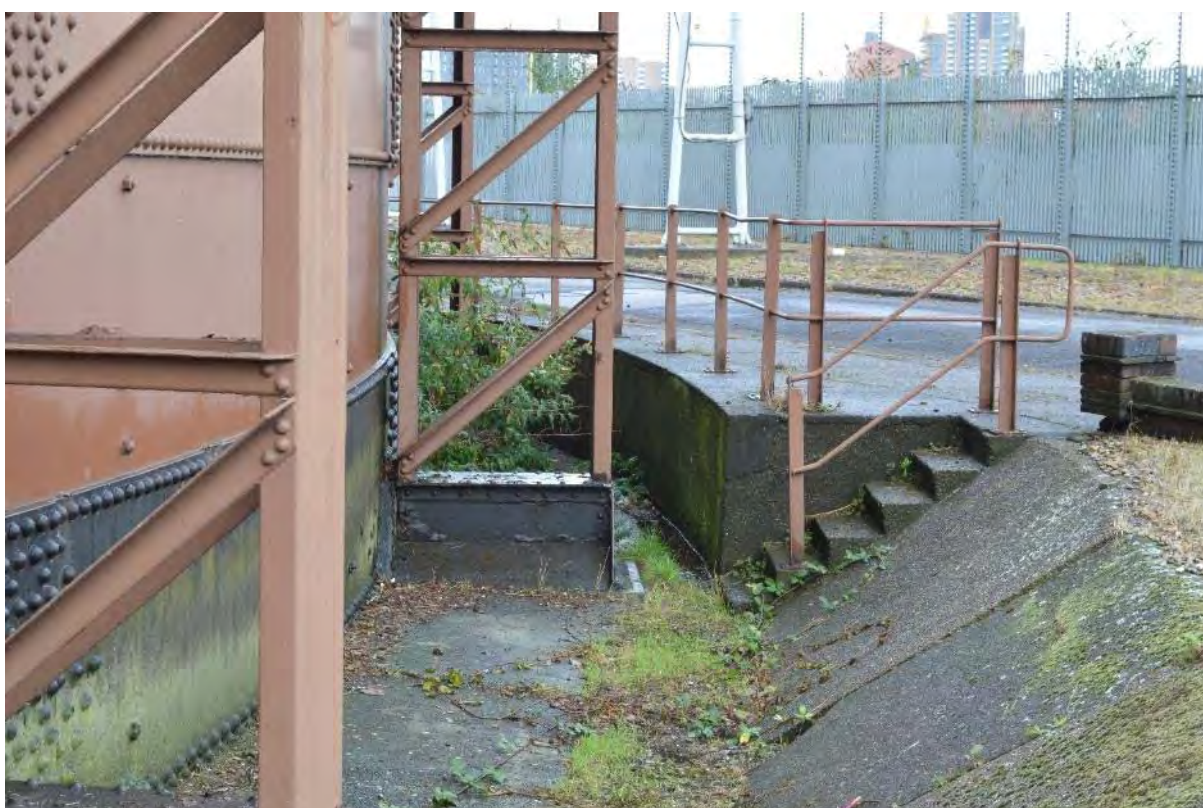
Plate 64: Gasholder No. 3, tank surround and raised curb level to the northern edge, facing north-west (90)
