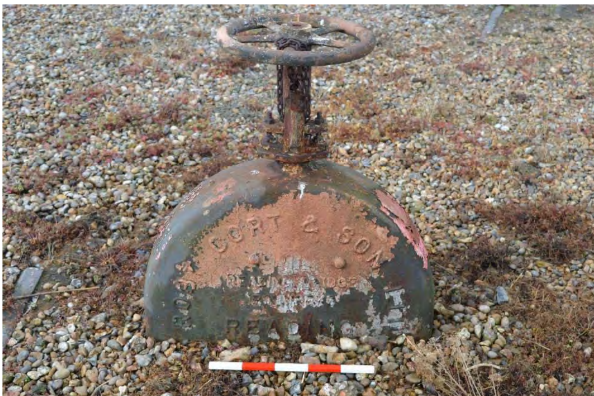
Plate 19: Gasholder No. 1, manual operational wheel associated to the dry-well equipment, facing west (190)
