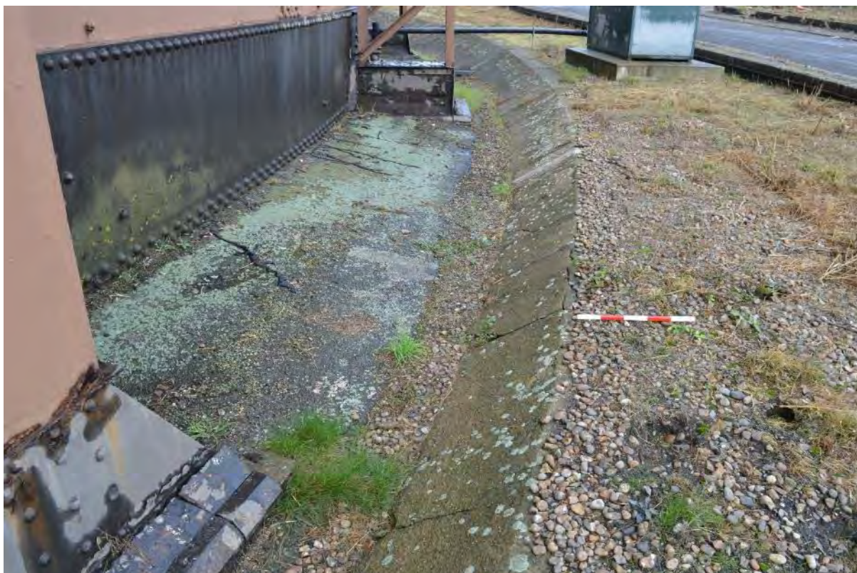
Plate 63: Gasholder No. 3, view of the concrete tank surround and curb, facing north-east (82)
