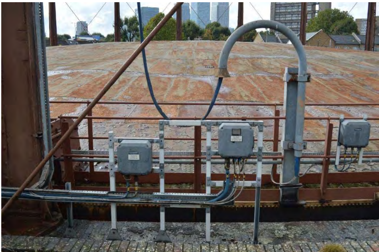
Plate 32: Gasholder No. 1, electrical anti-freeze system with water level measuring equipment located to the north-eastern edge of the gasholder, facing south-west (194)
