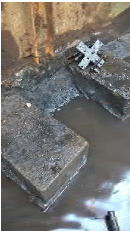
Plate 30: Gasholder No. 1, detail of the concrete plinths which support the base of each lift wall, facing south-east (480)
