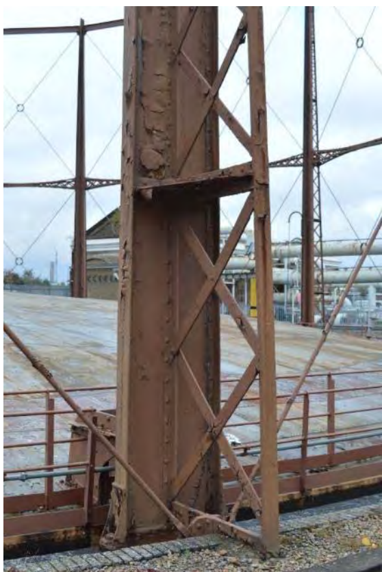
Plate 5: Gasholder No. 1, detail of the webbing and horizontal diaphragms attached to the standards, facing north-west (159)
