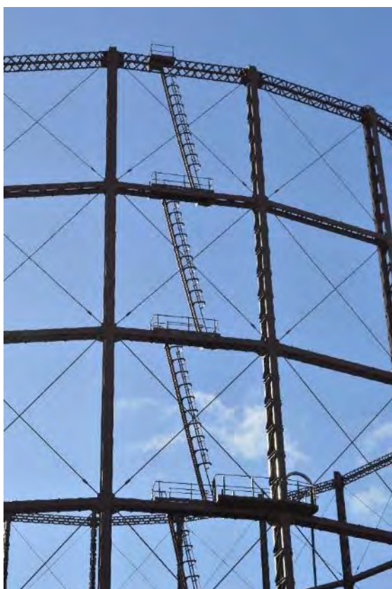
Plate 88: Gasholder No. 3, detail of the lift access ladders, platforms and guard cages, facing south-east (60)
