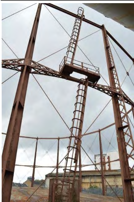
Plate 35: Gasholder No. 1, detail of the access ladders situated to the north-eastern edge of the gasholder, facing south-west (188)
