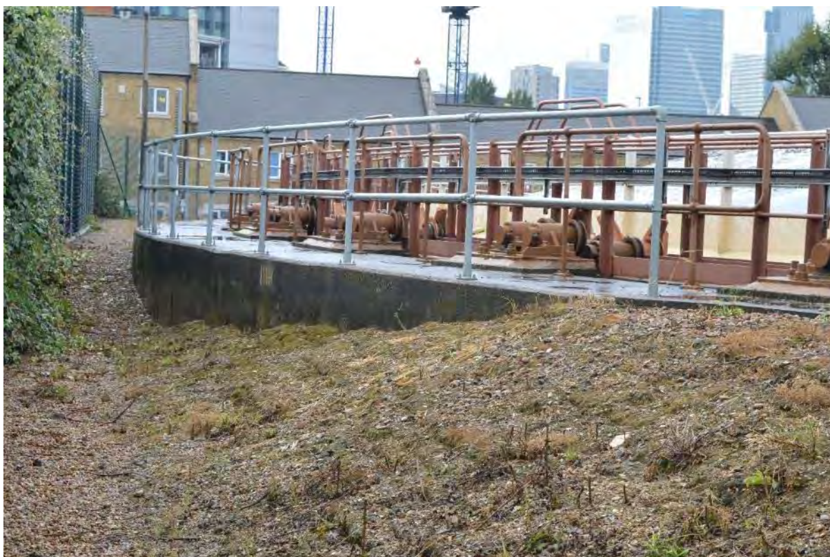
Plate 54: Gasholder No. 2, view of the concrete tank curb to the eastern edge, facing south-west (32)
