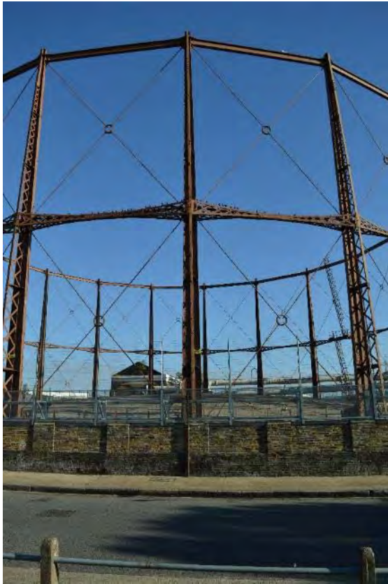
Plate 3: Gasholder No. 1, girder and standard arrangement of the guide frame, facing north (125)
