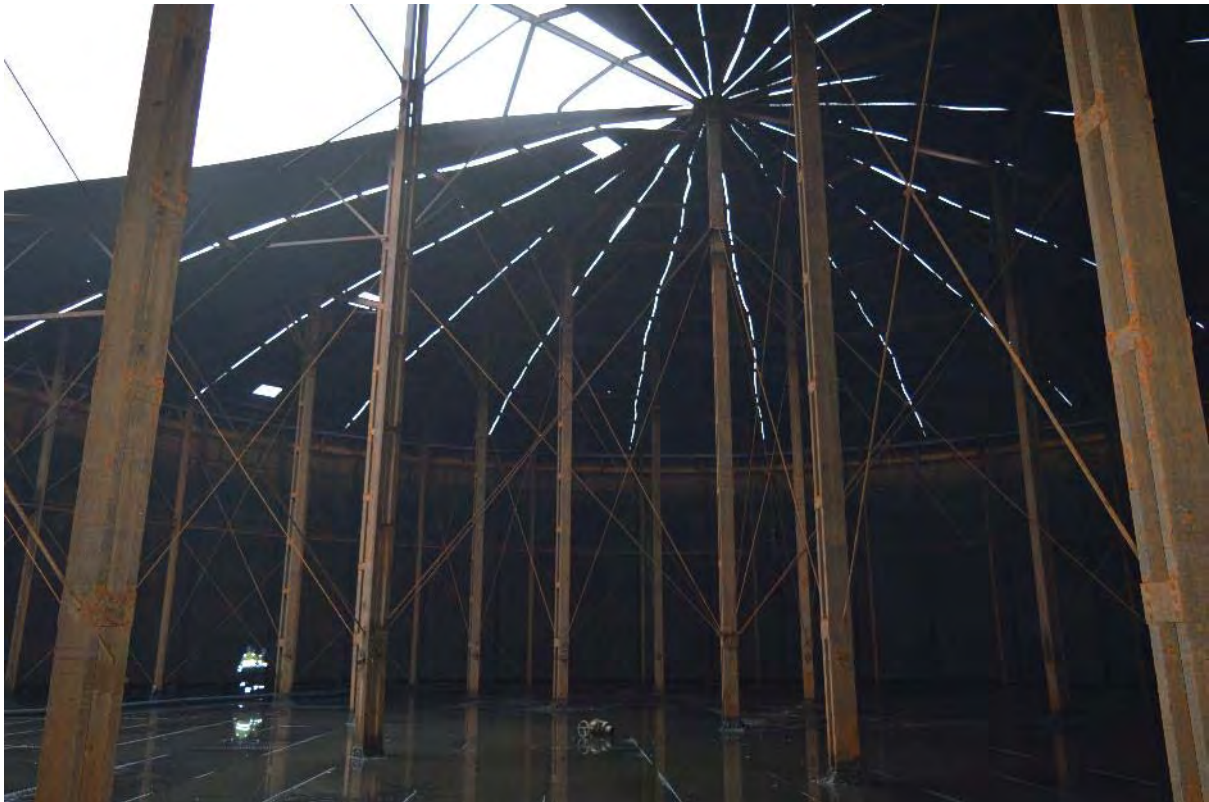
Plate 83: Gasholder No. 3, view of the steel trusses which create the framework supporting the underside of the crown, note the outer rim cross-bracing and central girder arrangement, facing north (385)
