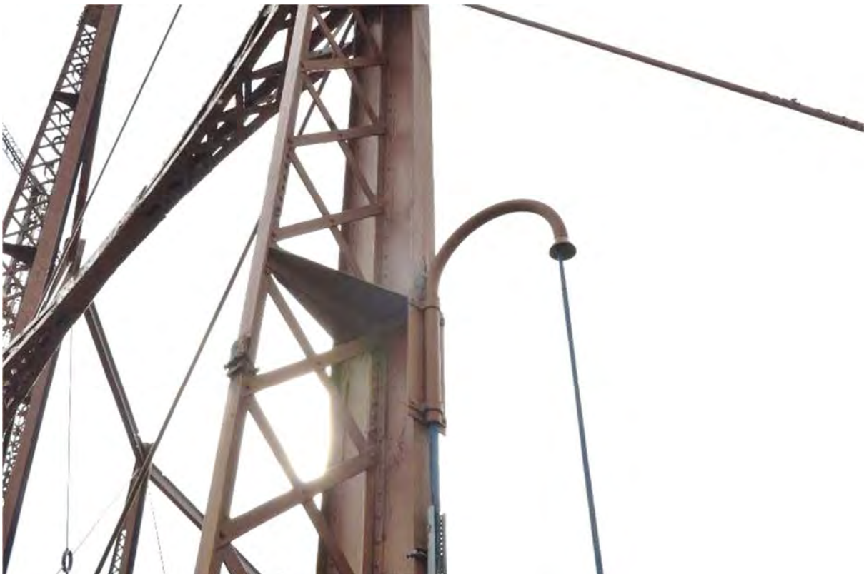
Plate 34: Gasholder No. 1, detail of the shepherd's-crook cable guides for the pressure alarm monitoring equipment, facing north-east (195)
