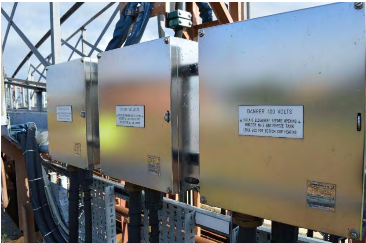
Plate 46: Gasholder No. 2, circuit boxes for the electrical anti-freeze and cup-level water monitoring systems, facing north-east (37)
