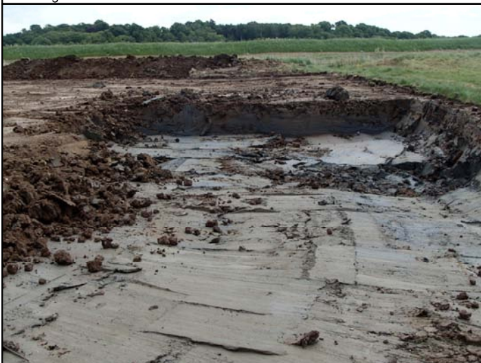
Fig. 3e. Excavation of the borrow pit, Area 3, showing the thin topsoil and the clay, looking east
