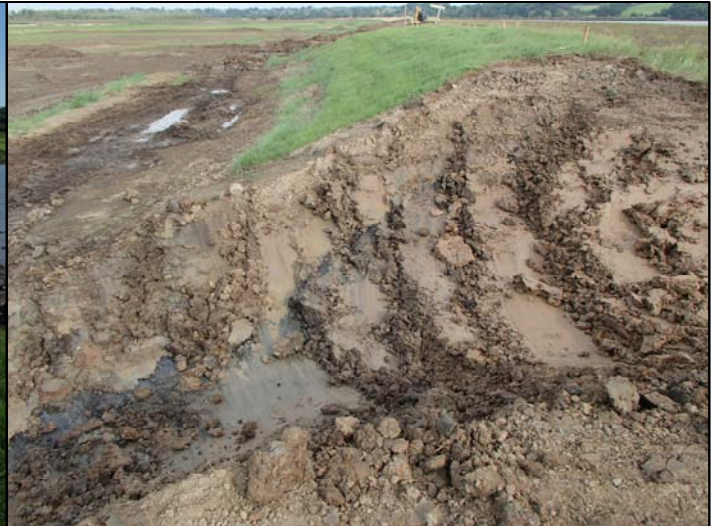
Fig. 5b. Section through the sea wall at the north end of the south breach Area 9, showing the two stages of construction separated by a black layer of rotting vegetation, looking north
