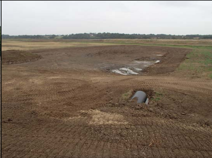
Fig. 4d. Extent of the south borrow pit Area 7, looking north-east. The sluice pipe for the new pond in Area 6 is in the foreground.
