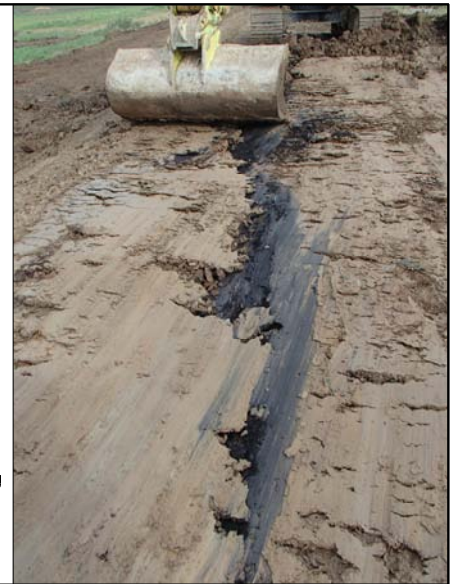
Fig. 6b. The layer of decayed vegetation dividing the sea wall stages of construction as it appeared during the sea wall works, looking north
