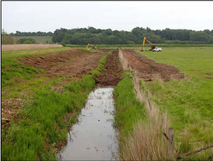
Fig. 3a. Stripping the topsoil and backfilling the ditch in Area 1, looking east
