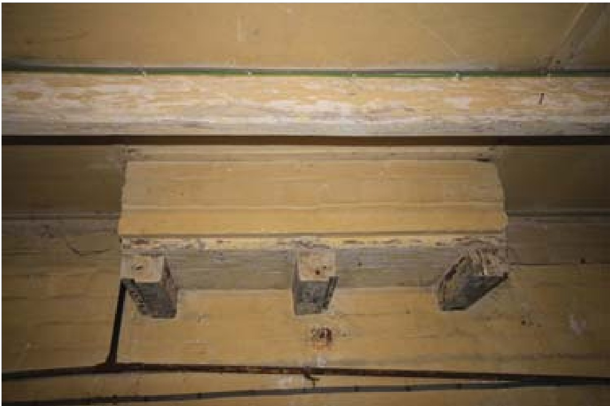
Plate 133: Base of the first floor fireplace within the cart room, Block D. (#406)
