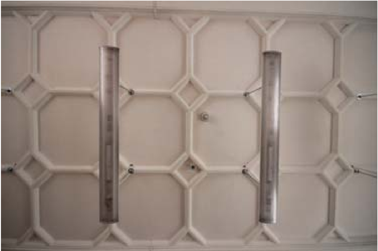
Plate 82: Overview of the ceiling, Room 13. (#221)
