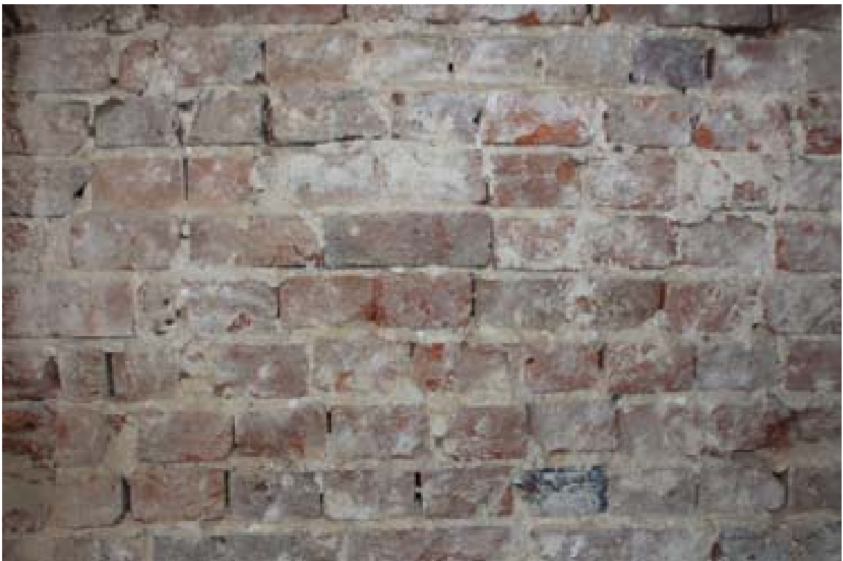
Plate 27: Example of the brickwork on the east wall of the hall, Room 2. (#105)
