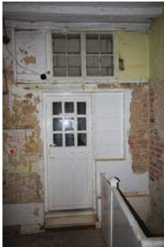
Plate 47: Half-timbered door, south wall, Room 6. Note the barrier to the basement stairs. (#149)
