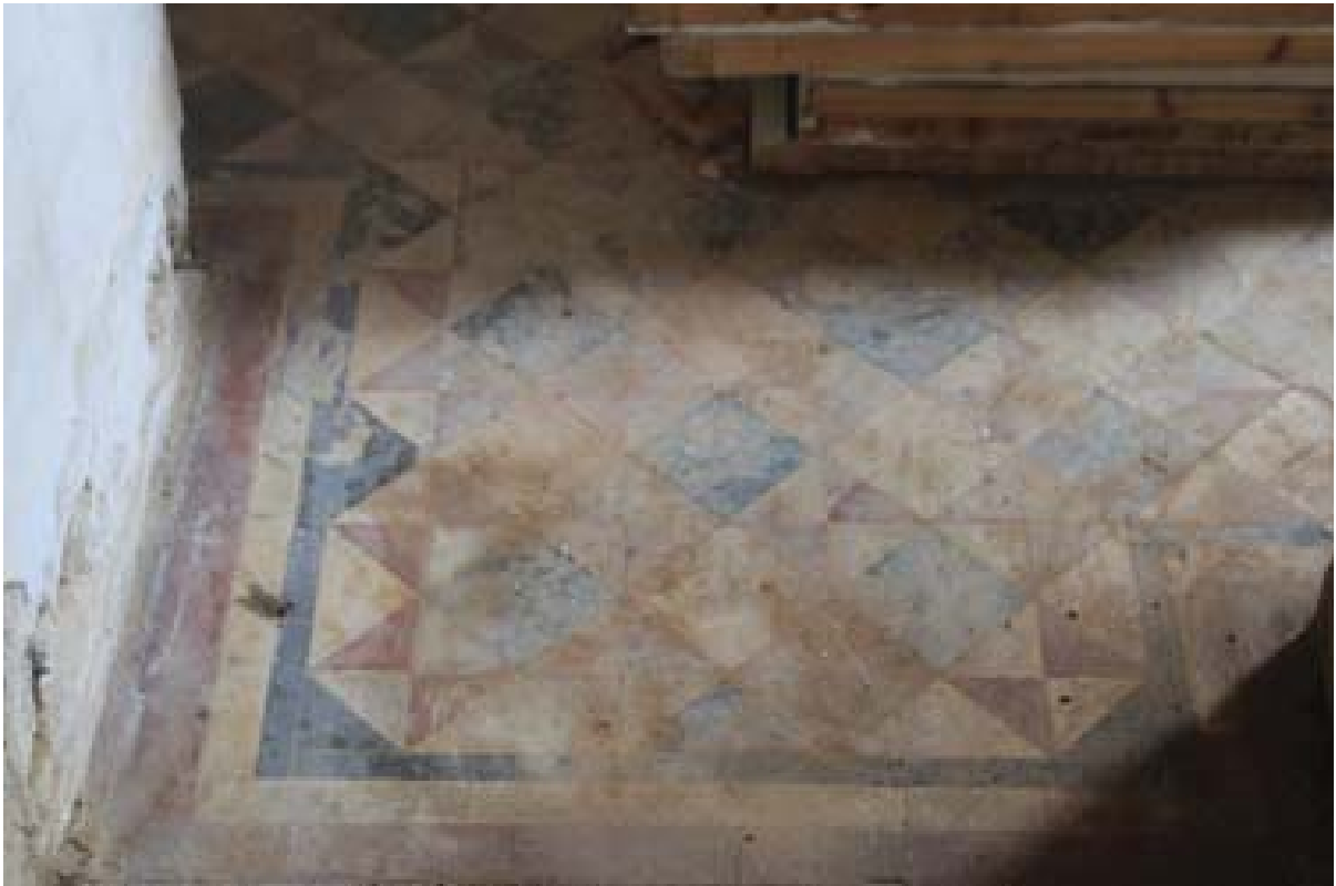
Plate 39: Edwardian tiles, Room 4. (#107)
