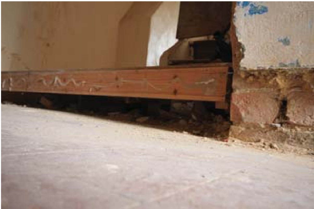
Plate 63: remnant section of inserted floor at the base of the stairs, Room 9/10. (#180)
