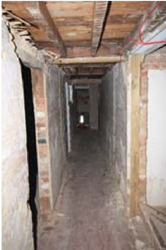
Plate 65: Overview of the servants' corridor (Room 9) showing the construction of the ceiling at its east end. (#142)
