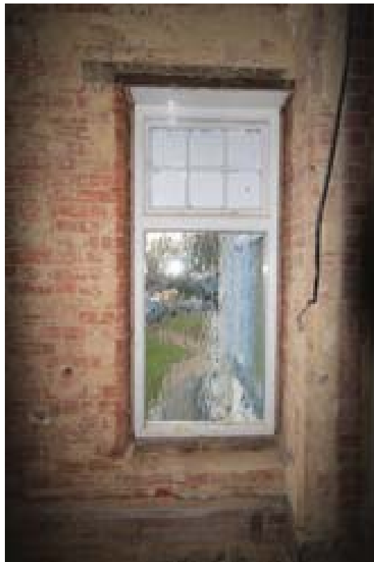
Plate 111: Window in north wall of Room 21 forming part of a wrap-around window to the stair and Room 16 to the north. (#284)
