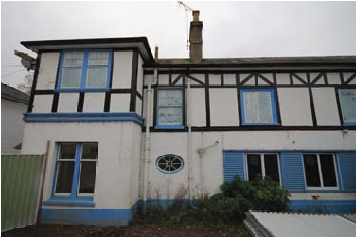
Plate 2: Presumed original horned sash and oeil-de-boeuf windows (centre) in north elevation of Block A. (#53)
