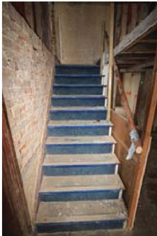
Plate 29: Overview of the stairs, Room 2. Note the bond timber at the base of the wall to the left. (#98)
