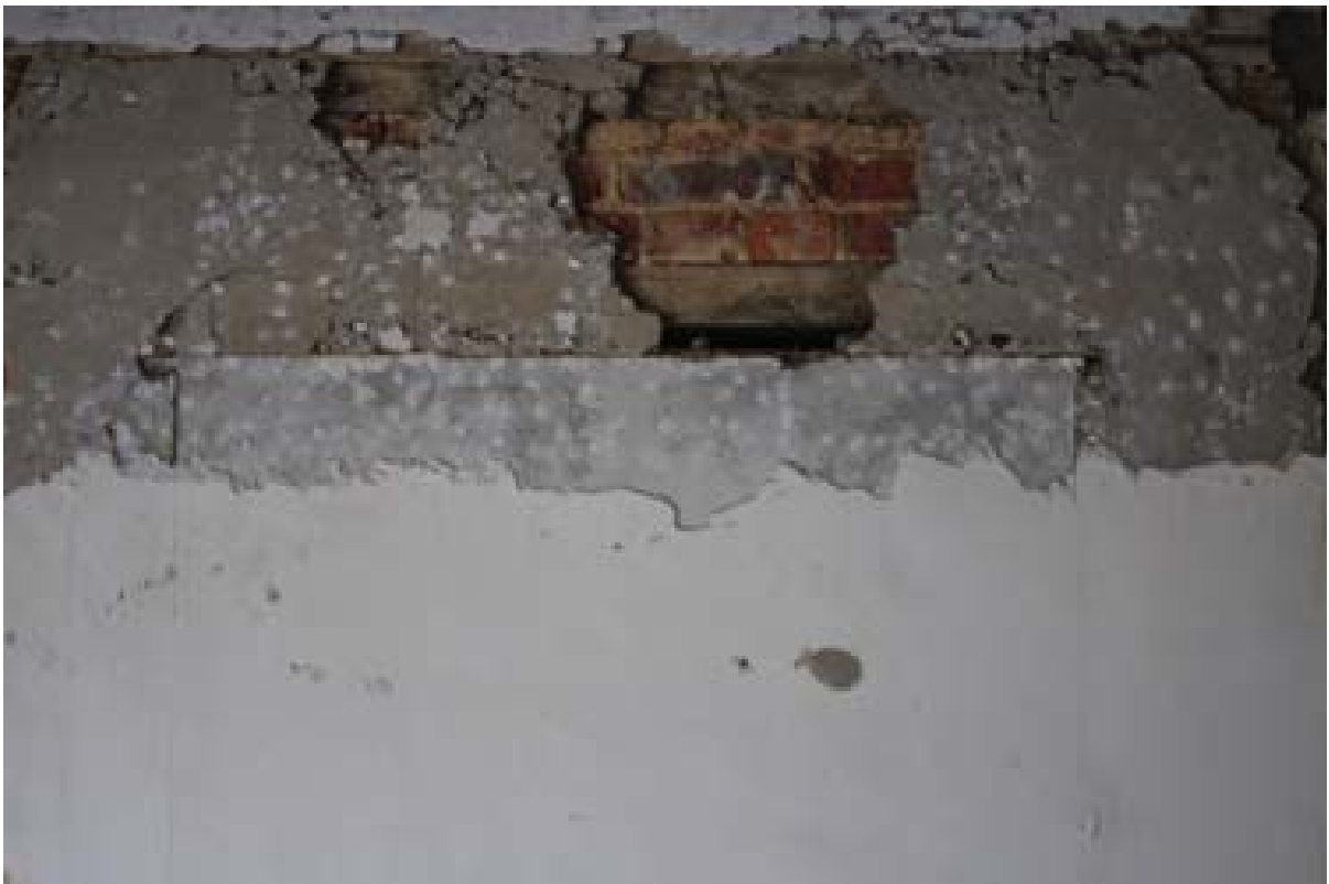
Plate 45: A blocked doorway to the Old Hall is revealed by a timber lintel in the west wall of Room 5. (#129)
