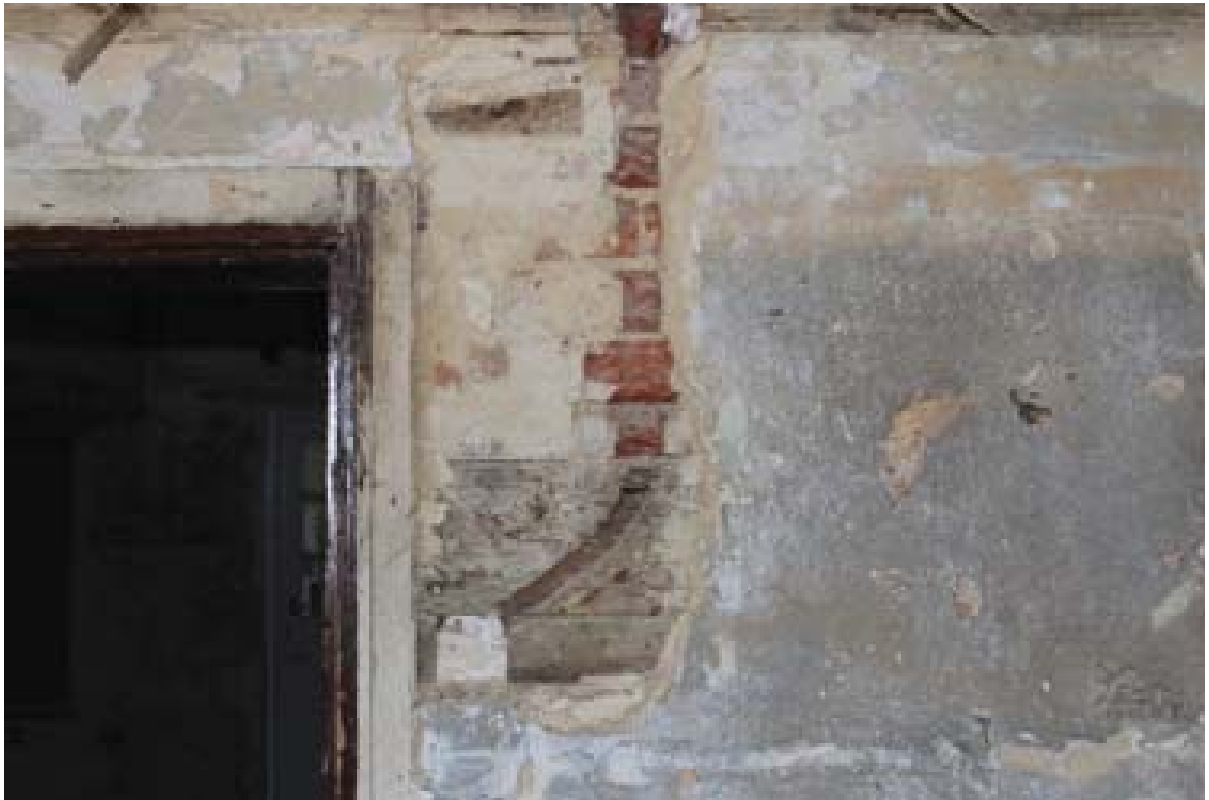
Plate 21: Bond timber in north wall of Room 1 – note the void peg hole implying a reuse of timber. (#71)
