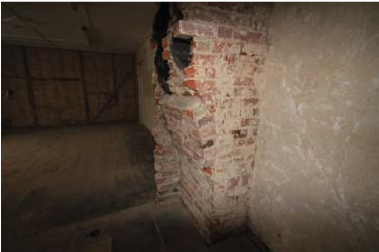
Plate 99: Remnant chimney stack and wall, Room 17. (#265)
