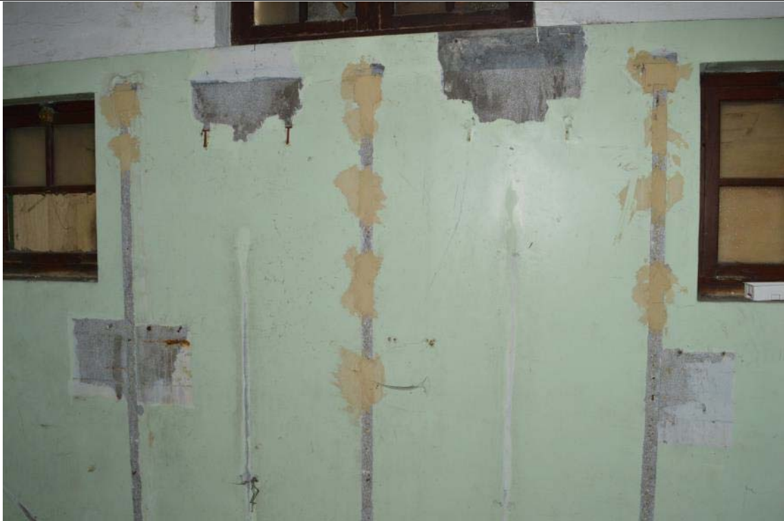
Plate 7: Room 5, looking east at former cubicle partitions and patches of original plasterwork (52)
