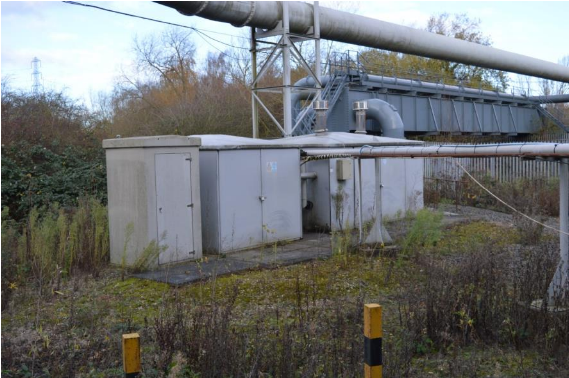
Plate 40: Pump House, Boiler House, and MEG Tank situated within the southern compound, facing north-west (ARG15-0116)
