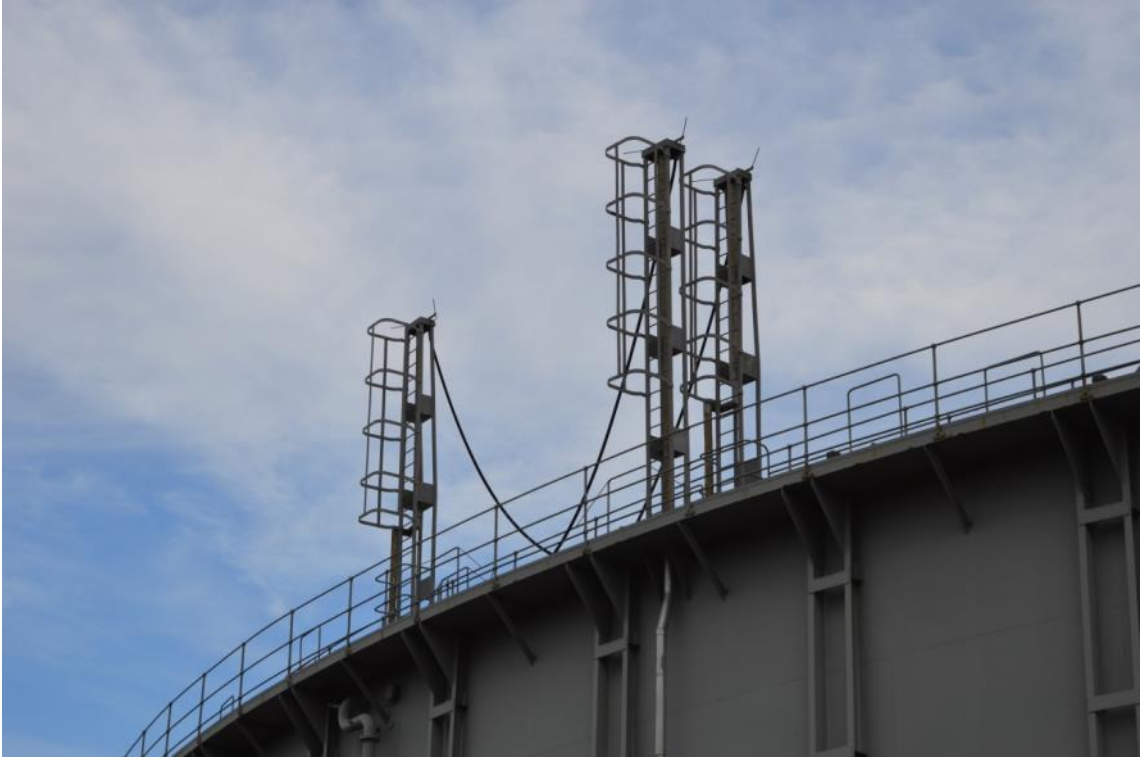
Plate 46: Gasholder No. 7, detail of enclosed access ladders and ancillary hoses, facing north (ARG15-0011)
