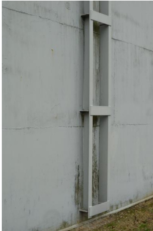
Plate 52: Gasholder No. 7, detail of the welded tank sheeting and vertical support stanchions, facing north-west (ARG15-0006)
