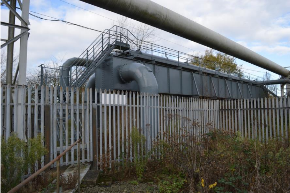
Plate 41: Gasholder No. 5, southern compound access bridge with associated gas mains pipework below, facing north (ARG15-0118)
