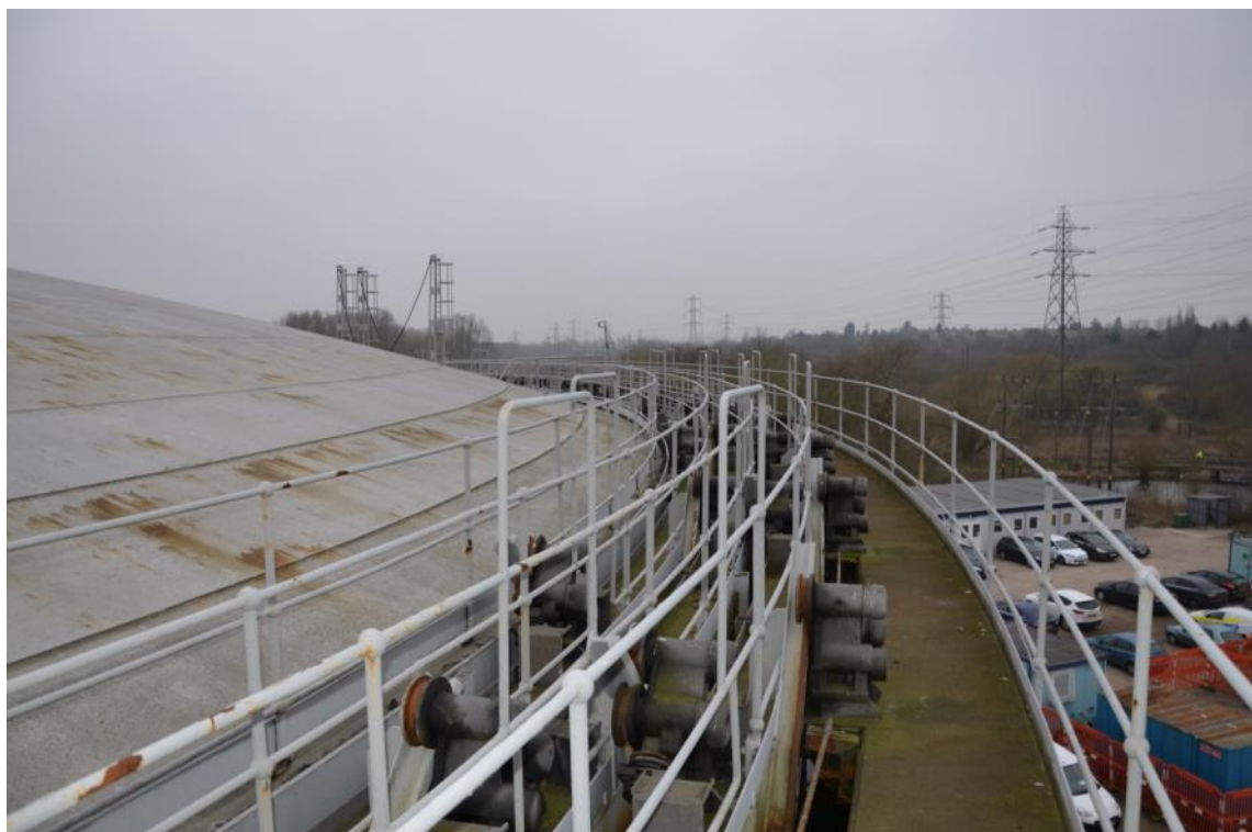
Plate 49: Gasholder No. 7, detail of the guide carriage arrangement, facing south-west (ARG15-0137) (Supplied by National Grid)
