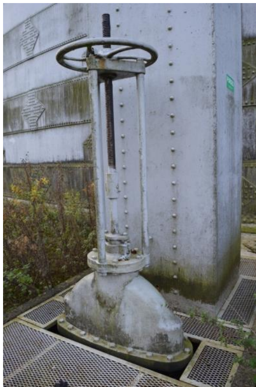
Plate 37: Gasholder No. 5, detail of manual operation valve serving the northern gas inlet/outlet syphon, facing south-west (ARG15-0128)
