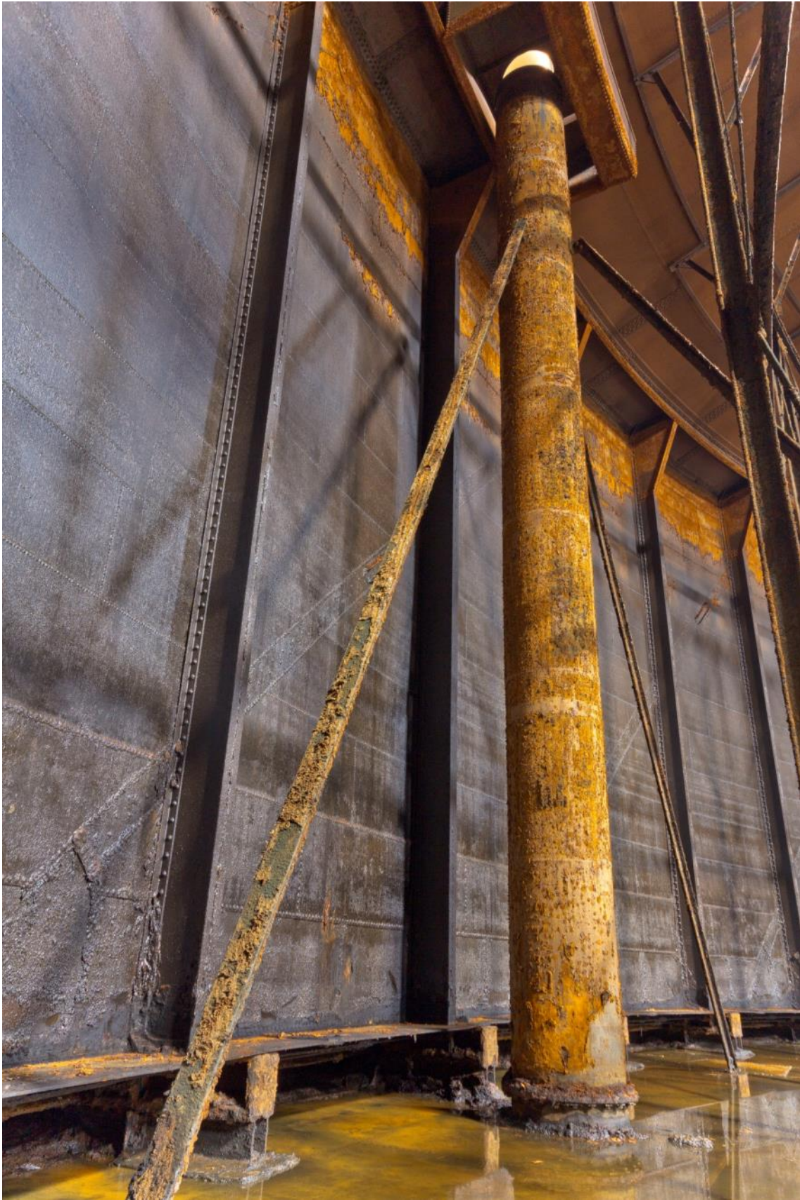
Plate 35: Gasholder No. 5, standpipe for gas supply within the gasholder (ARG15-0272)
