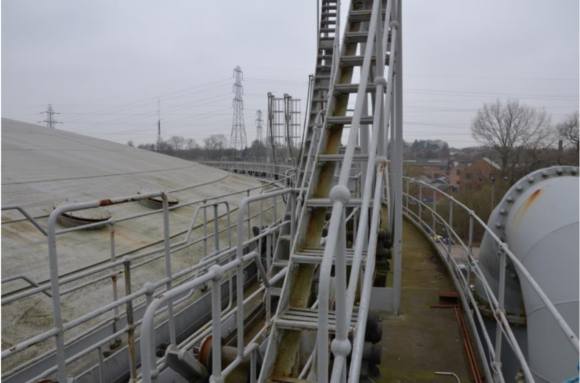
Plate 43: Gasholder No. 7, view of tank bell, platform, lift, access stair and handrail arrangement, facing west (ARG15-0136) (Supplied by National Grid)
