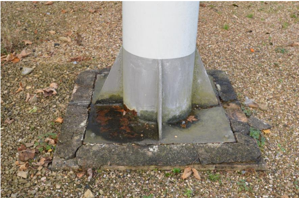
Plate 59: Detail of the column base supporting the gas mains pipework around the site, facing south-east (ARG15-0042)
