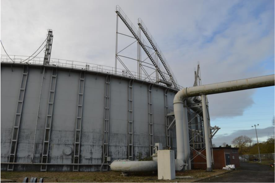
Plate 50: Gasholder No. 7, view of the lift access stair design, facing south-west (ARG15-0052)
