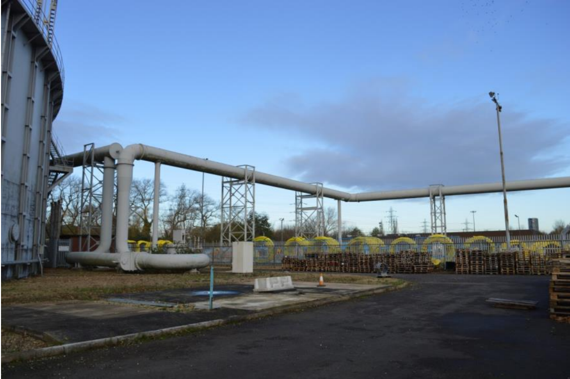
Plate 58: Gasholder No. 7, view of the gas mains 'Donkin' pipework extending to the site's southern compound, facing north-west (ARG15-0053)
