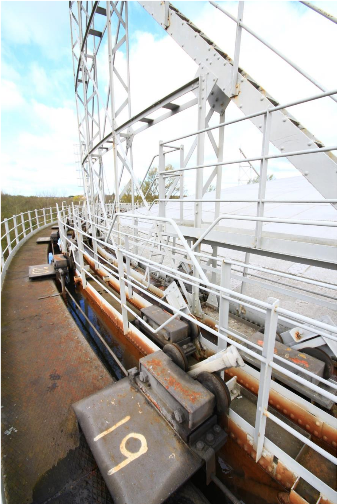
Plate 21: Gasholder No. 5, view of the guide carriage, tank platform and lift arrangement (ARG15-0184)
