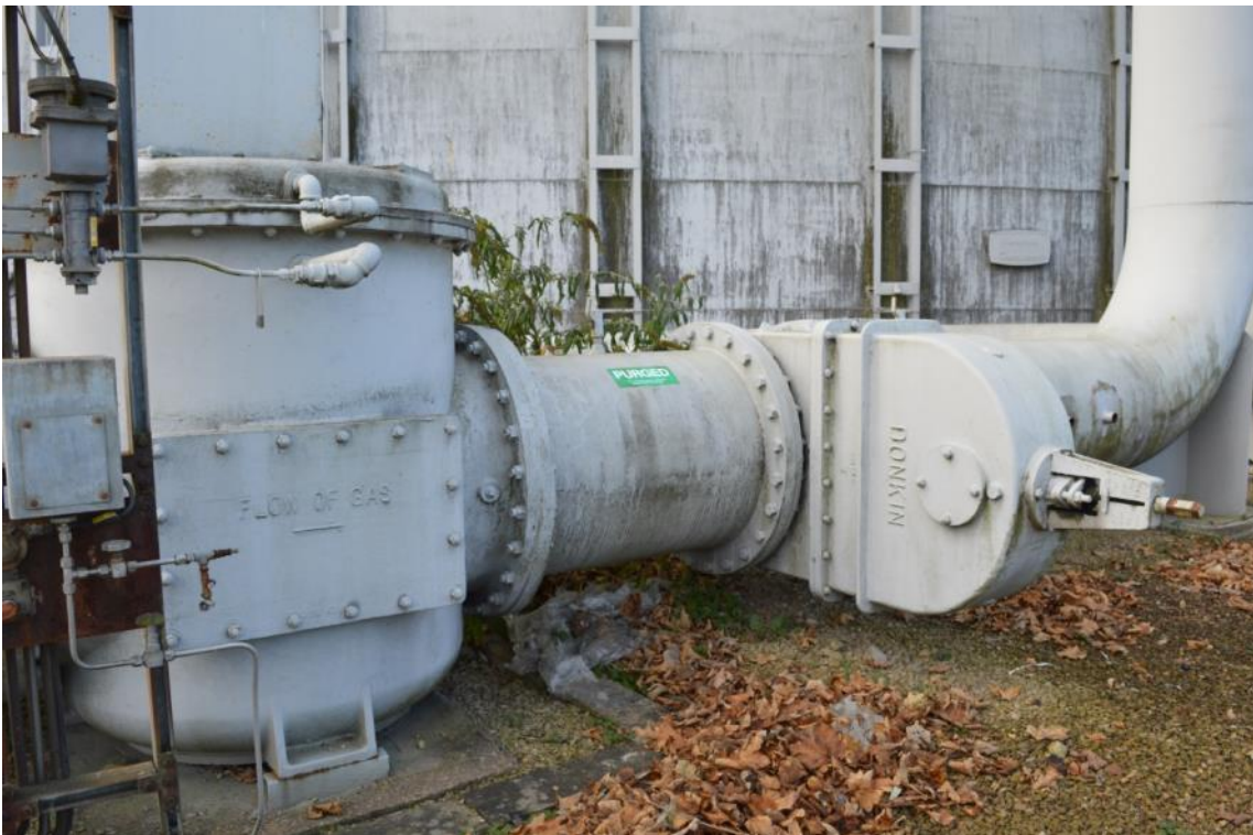
Plate 57: Gasholder No. 7, detail of the gas mains 'Donkin' pipework serving the northern compound, facing south-west (ARG15-0040)
