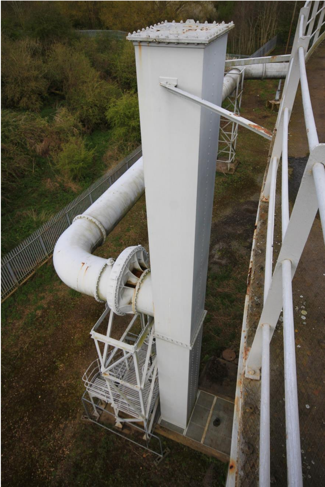
Plate 33: Gasholder No. 5, view of southern gas inlet/outlet syphon pipework, facing north-west (ARG15-0189)
