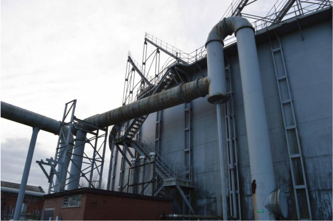
Plate 54: Gasholder No. 7, view of three tier tank access stair, facing south-east (ARG15-0036)
