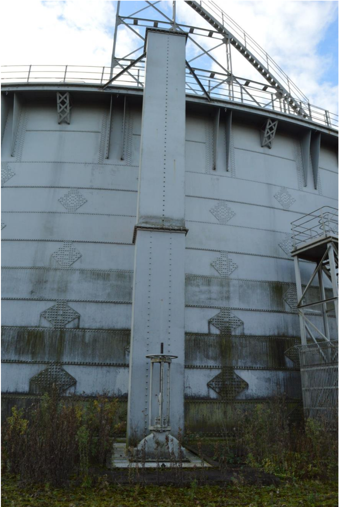
Plate 34: Gasholder No. 5, view of northern gas inlet/outlet syphon pipework, facing north-east (ARG15-0070)
