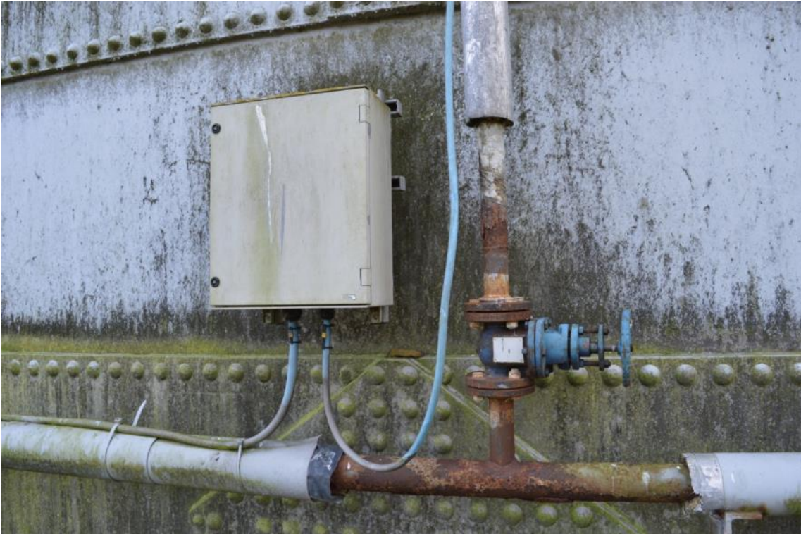
Plate 19: Gasholder No. 5, detail of the switch boxes serving the anti-freeze monitoring equipment and ring main, facing east (ARG15-0113)
