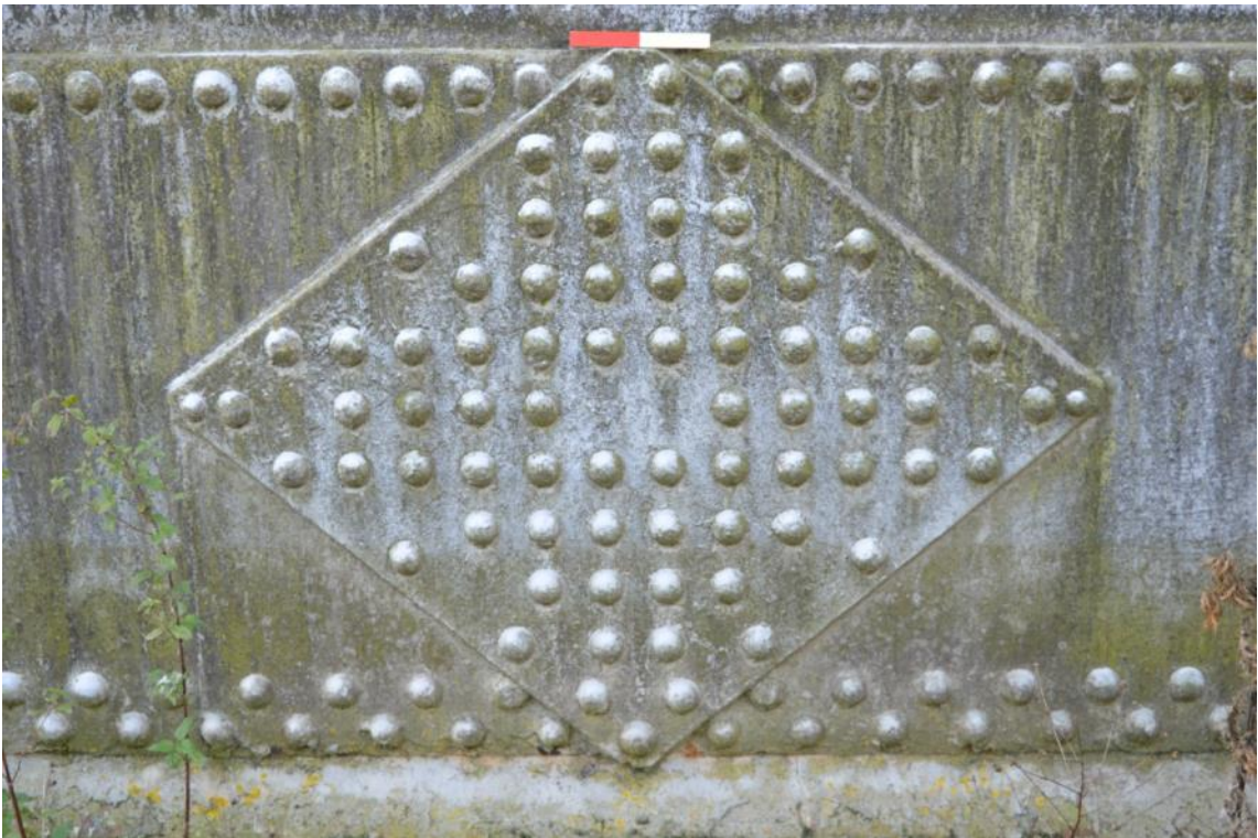
Plate 26: Gasholder No. 5, detail of support plates within the tank's first tier of sheeting, facing south (ARG15-0078)
