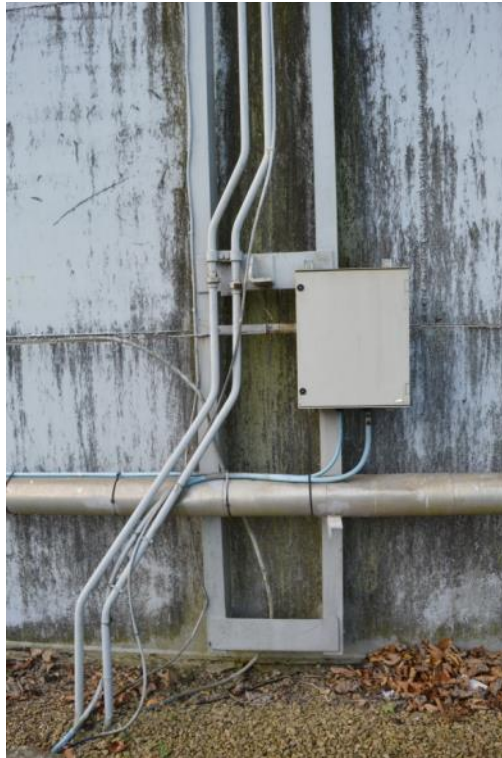
Plate 48: Gasholder No. 7, switch box pertaining to the antifreeze system (ARG15-0045)
