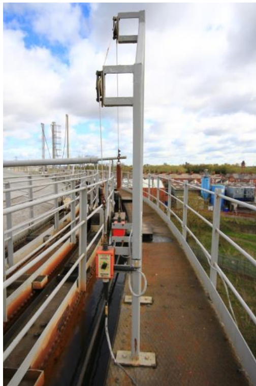
Plate 16: Gasholder No. 5, detail of the grabwire emergency switches (ARG15-0181)
