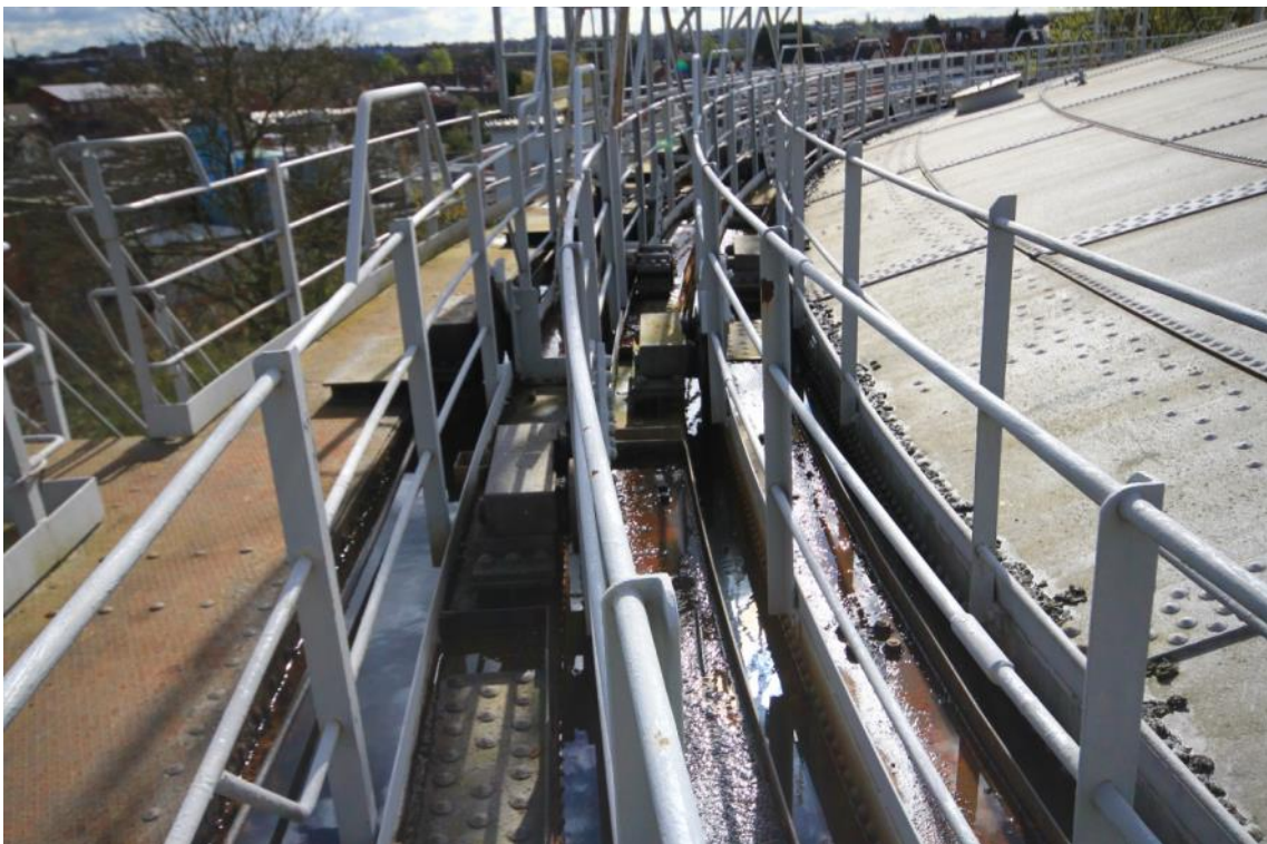
Plate 20: Gasholder No. 5, view of the guide carriage, tank platform and lift arrangement (ARG15-0157)
