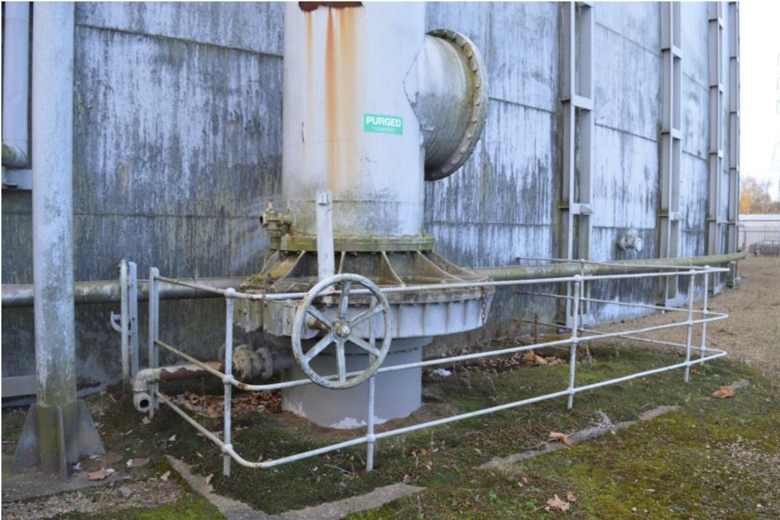
Plate 56: Gasholder No. 7, detail of northern gas mains inlet/outlet syphon pipework and manual operation valve, facing south-west (ARG15-0033)
