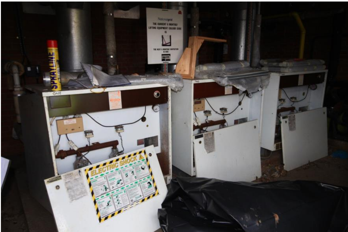
Plate 61: Apparatus within the boiler house (ARG15-0229)
