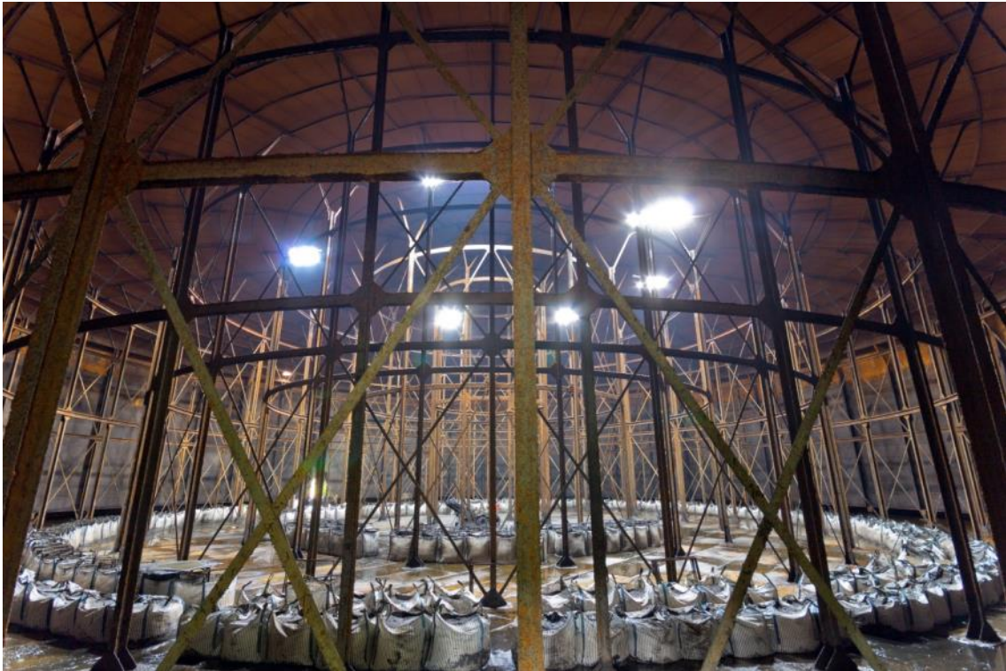
Plate 7: Gasholder No. 5, Interior framework – the bags are filled with sludge from the desludging process following the draining of the holder (ARG15-0275)
