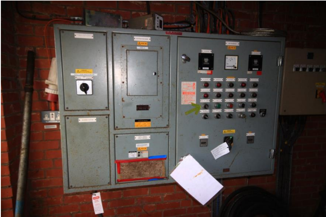
Plate 62: Alarm systems within the boiler house (ARG15-0230)
