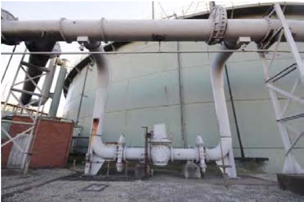
Plate 18: Volumetric governor, Gasholder 6 (PPD16-0020)
