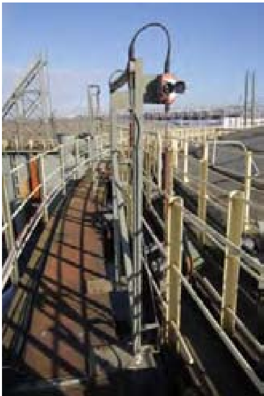
Plate 6: Craig & Derricott Ltd I-grab Grabwire emergency switches on tank platform, gasholder 6 (PPD16-0126)
