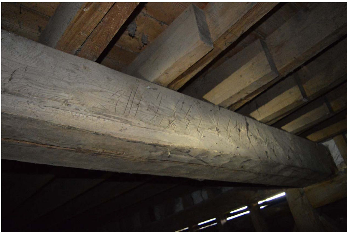
Plate 11: Merchant's marks on barn binding joist between Bays 1 and 2, looking south-west (HRWF_035)
