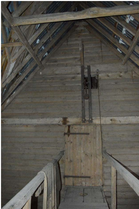
Plate 16: First floor of barn, gantry trap door and hoist in Bay 3, looking north (HRWF_052)
