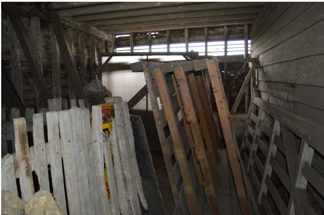
Plate 14: Ground floor of barn, Bay 6. Converted to cow-house or animal shelter, looking east (HRWF_044)
