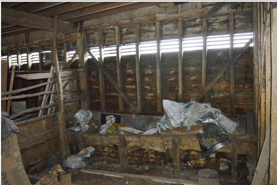
Plate 13: Ground floor of barn, Bays 4 and 5. Space converted to cow-house with manger and stall divider intact, looking east (HRWF_039)
