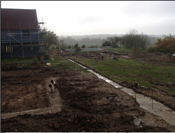
The garden retaining wall foundation Area 9, after filling with concrete looking south-west
