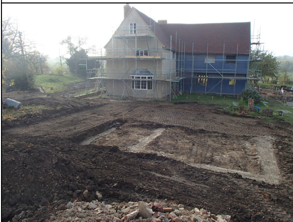
The hall, the garage foundations (Area 12) after filling with concrete and general landscaping, looking south
