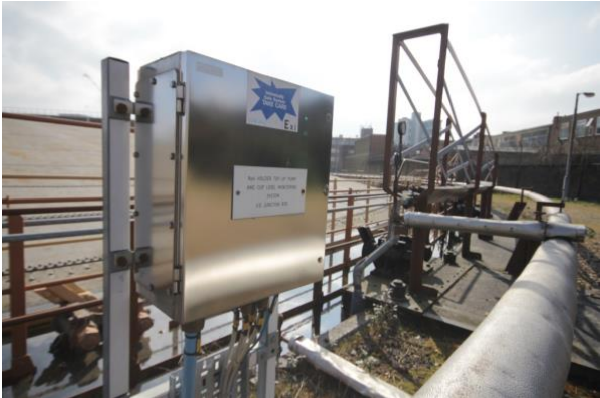
Plate 21: Water level monitoring system (MRA16-0092)
