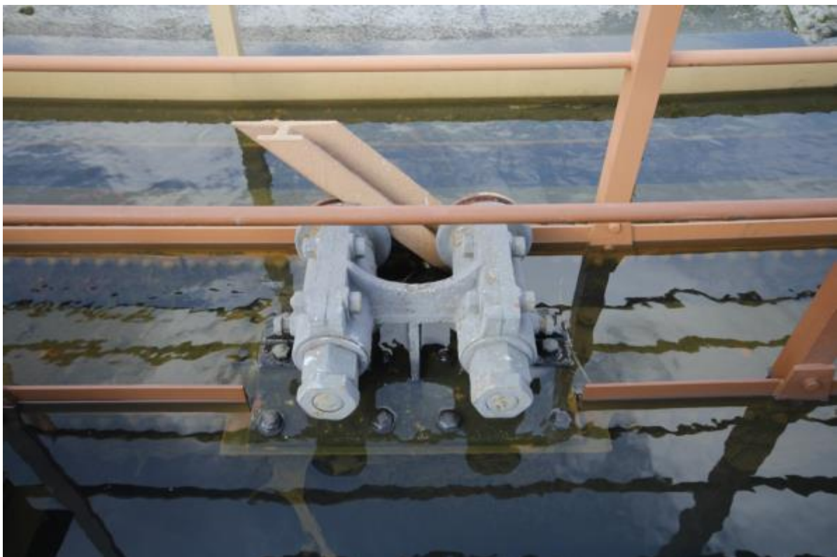
Plate 22: Guide carriages to inner lifts (MRA16-0078)
