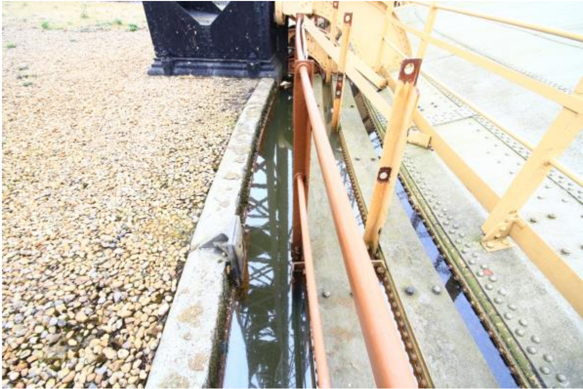
Plate 42: Concrete tank edge, Gasholder No. 5 (MRA16-0271)
