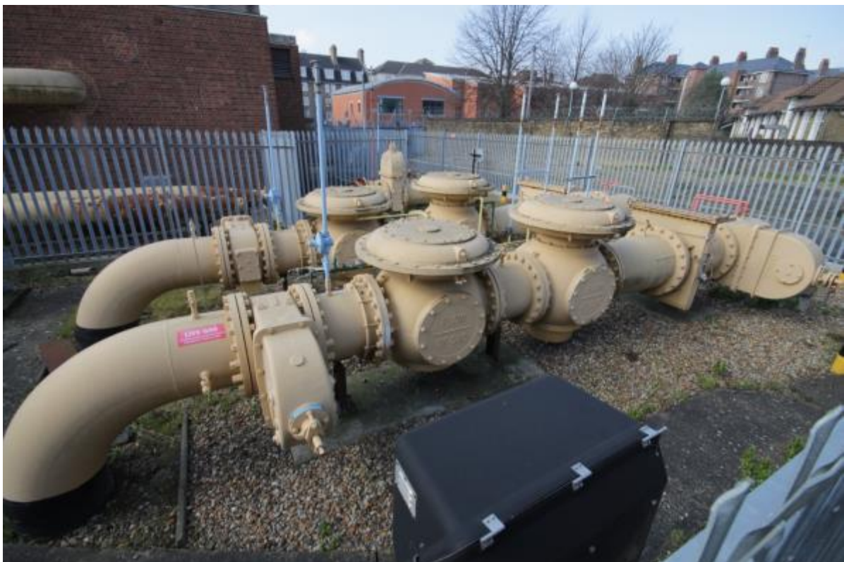
Plate 54: Live gas pipes (MRA16-0117)
