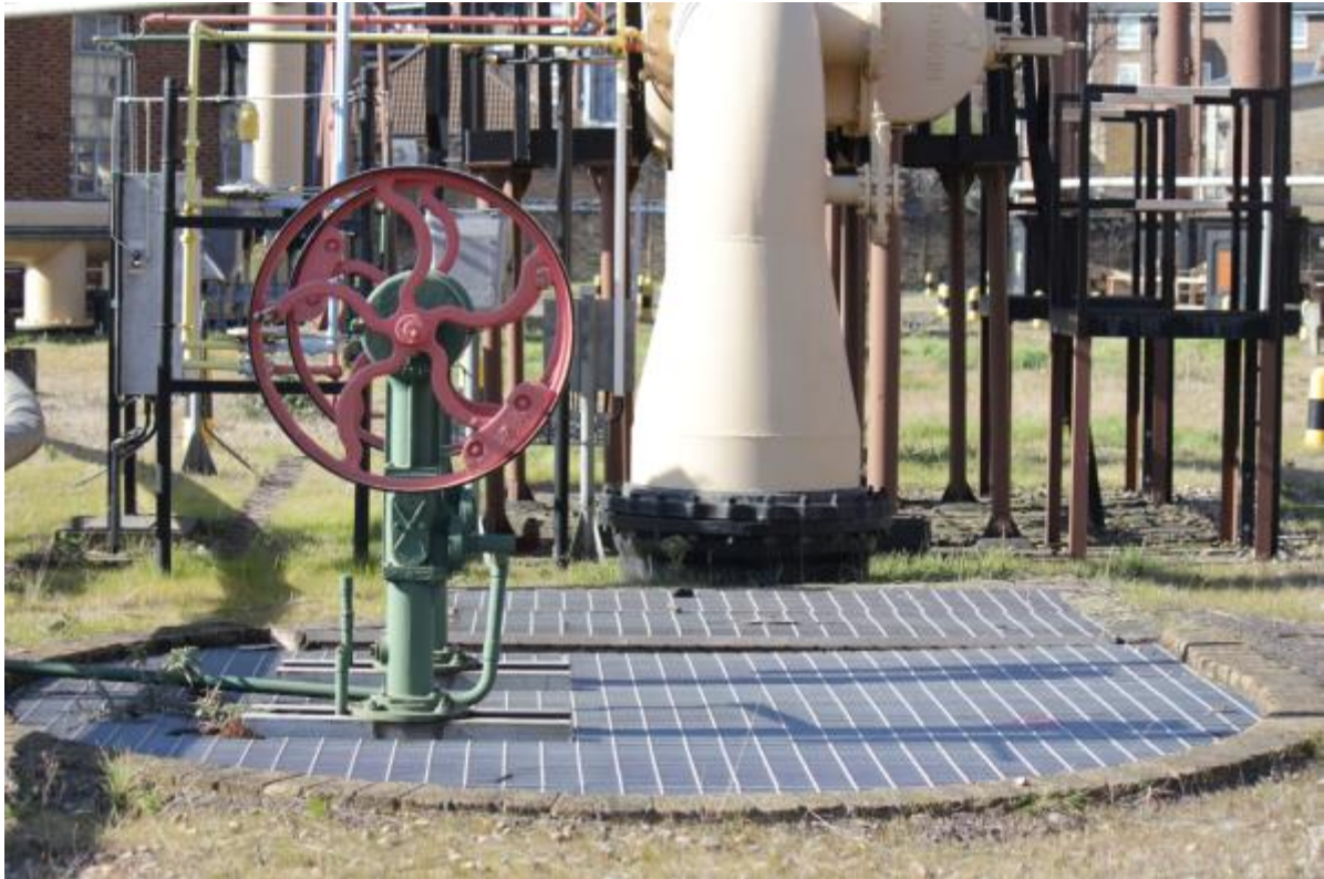
Plate 27: Siphon pit and Governor (MRA16-0219)
