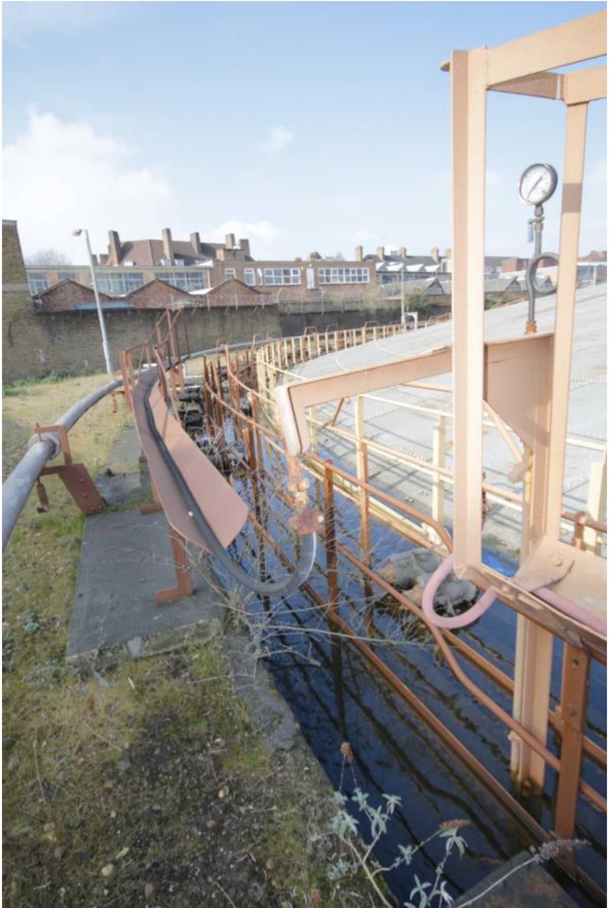
Plate 20: Hose guides with Boss 10 bar pressure gauge (MRA16-0088)
