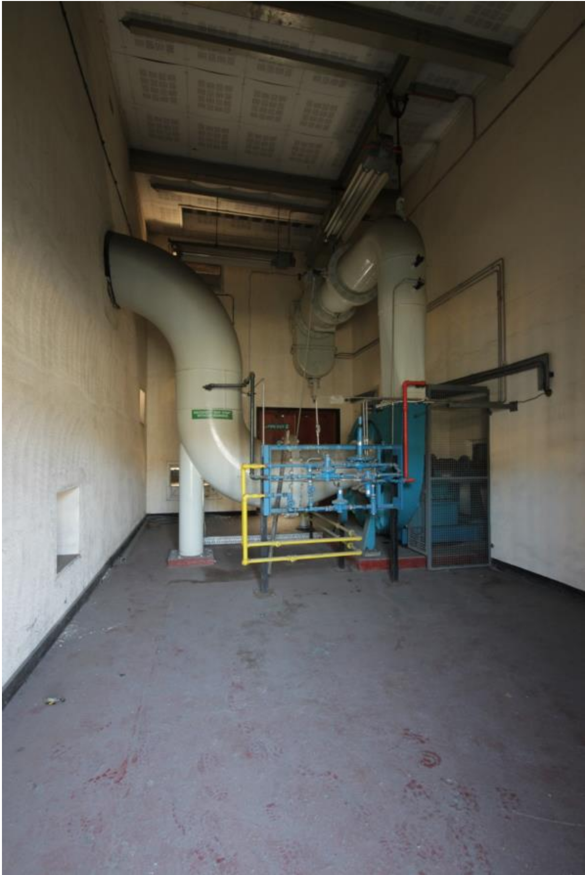
Plate 62: Booster Room (MRA16-0142)
