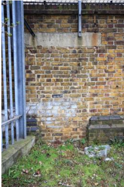
Plate 71: Blocked former exit to the canal right of way (MRA16-0293)
