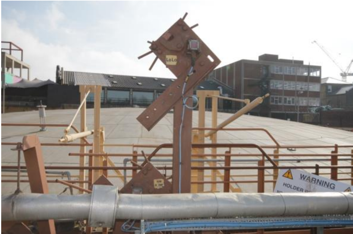
Plate 8: Pressure alarm system (MRA16-0043)
