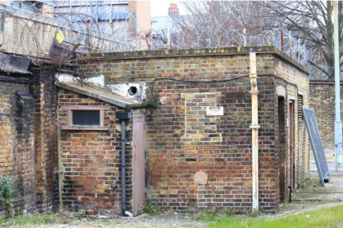
Plate 64: Electrical Substation and toilet (MRA16-0372)
