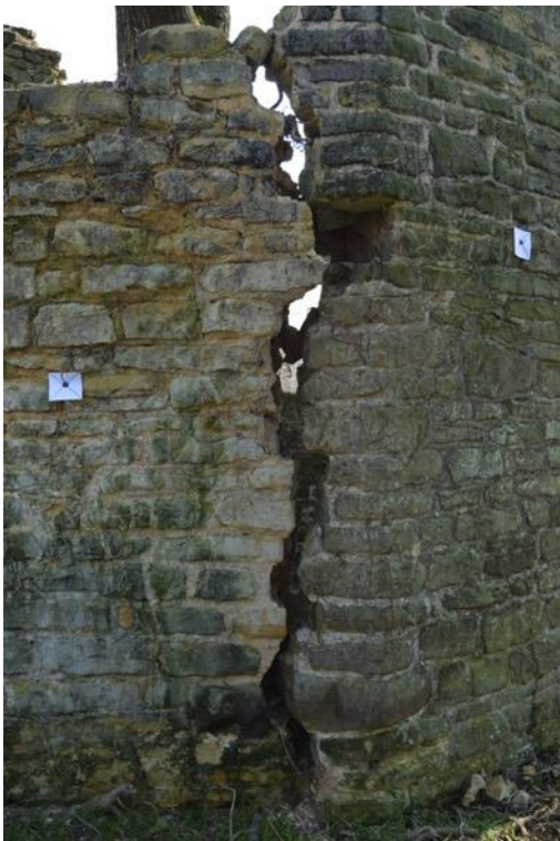
Plate 2: Example of the structural cracks with the base, Elevation 4 (6948_0054)
