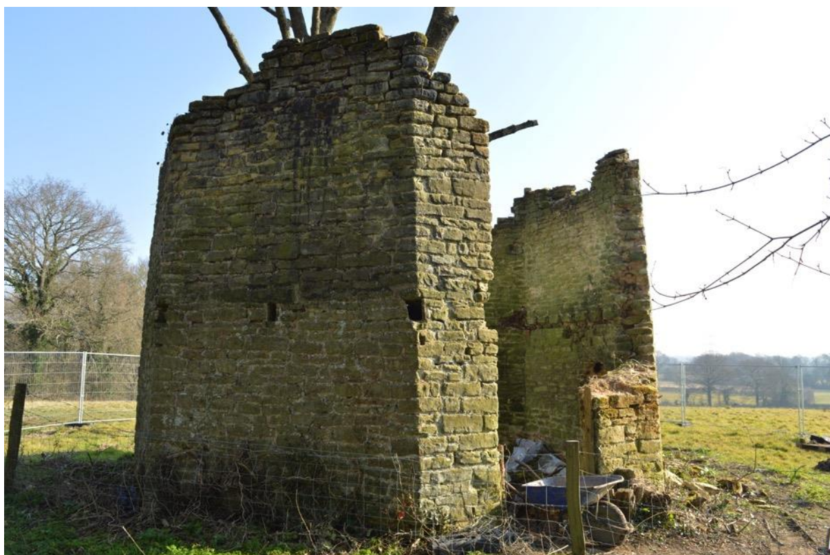
Plate 6: Detail of the tar staining of the upper level of the stone base, Elevation 2 (6948_0014)
