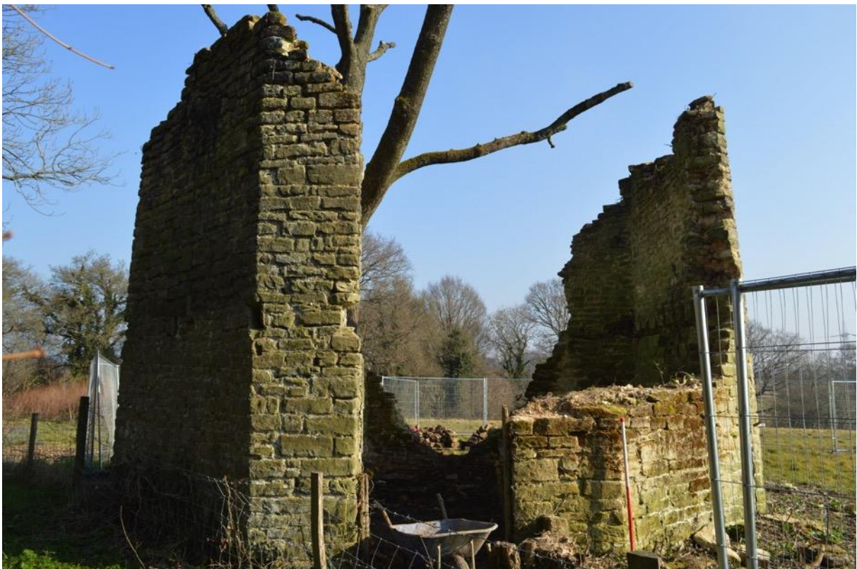
Plate 8: Retained ground floor level entrance, stone lintel and date stone formerly situated above not removed, Elevation 1 (6948_0017)
