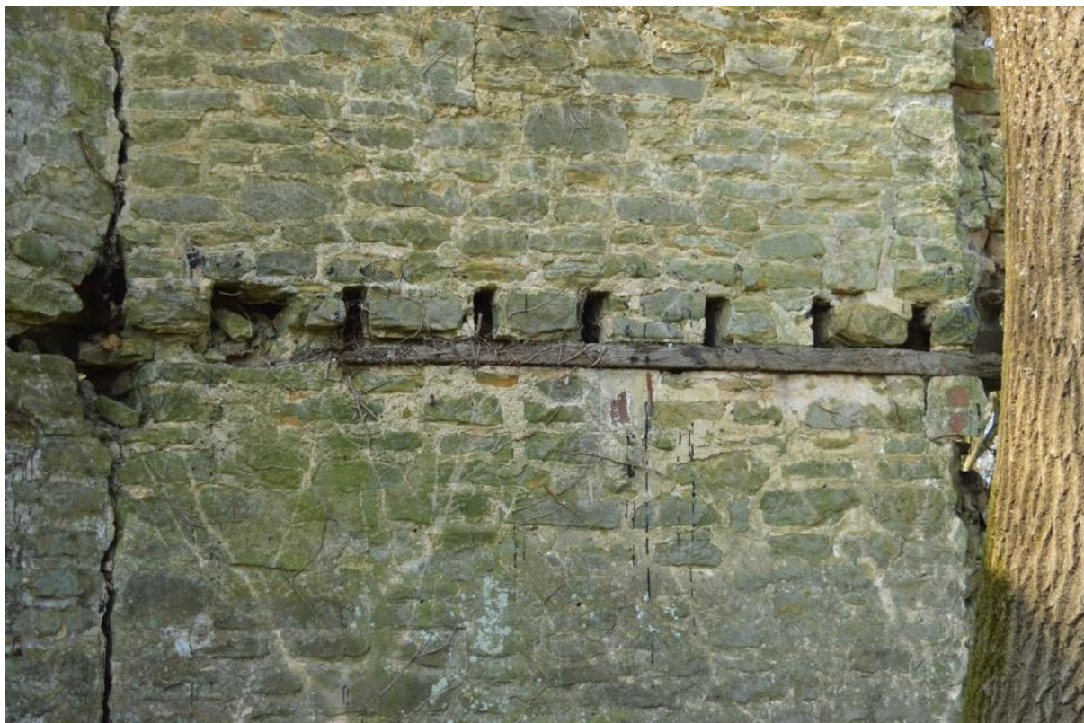
Plate 17: Detail of a wall set horizontal timber beam and floor joist sockets, Elevation 3 interior (6948_0041)
