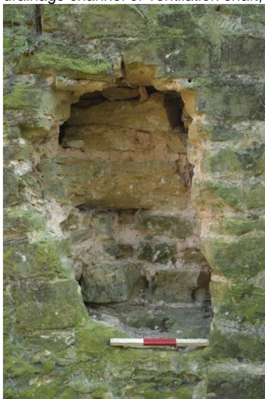
Plate 20: Detail of the large recess within the stone base internal wall face, Elevation 7 (6948_0043)
