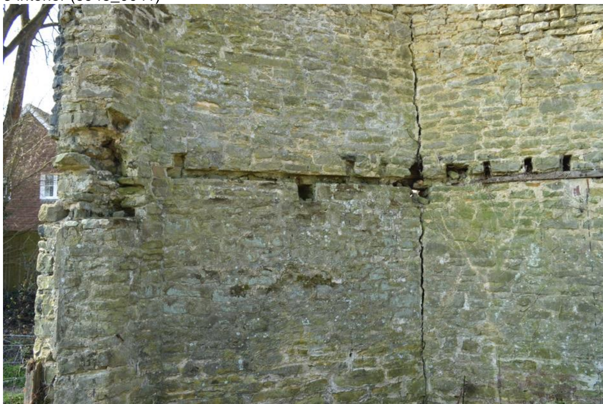
Plate 18: Detail of the redundant incision left by the location of a former horizontal beam, note the fewer floor joist sockets, Elevation 2 interior (6948_0039)
