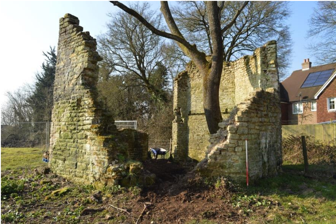
Plate 1: Stonework displacement caused by vegetation and overgrowth, Elevation 5 (6948_0015)
