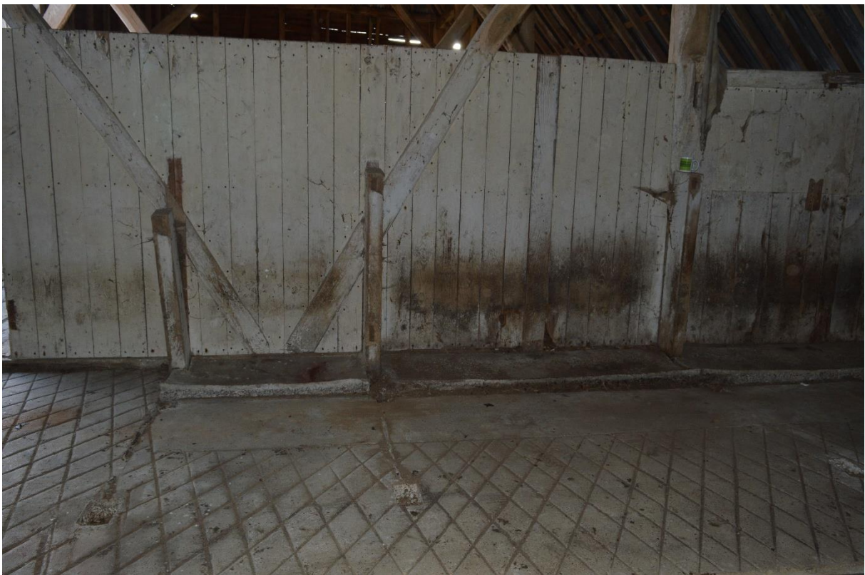
Plate 24: Evidence of cow stalls on floor and boarding of Truss 4, looking east (97)
