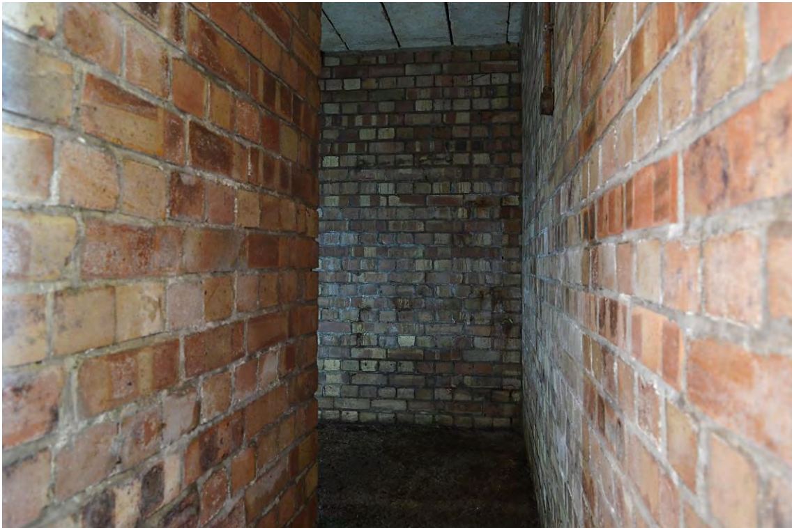
Plate 45: Shelter 4, view of the central circulation area within the southern end of the shelter, facing south (60)
