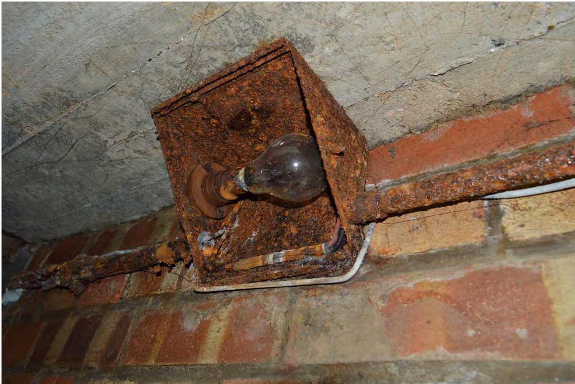
Plate 49: Shelter 4, detail of the light fittings within the eastern range of the shelter, facing south-east (76)
