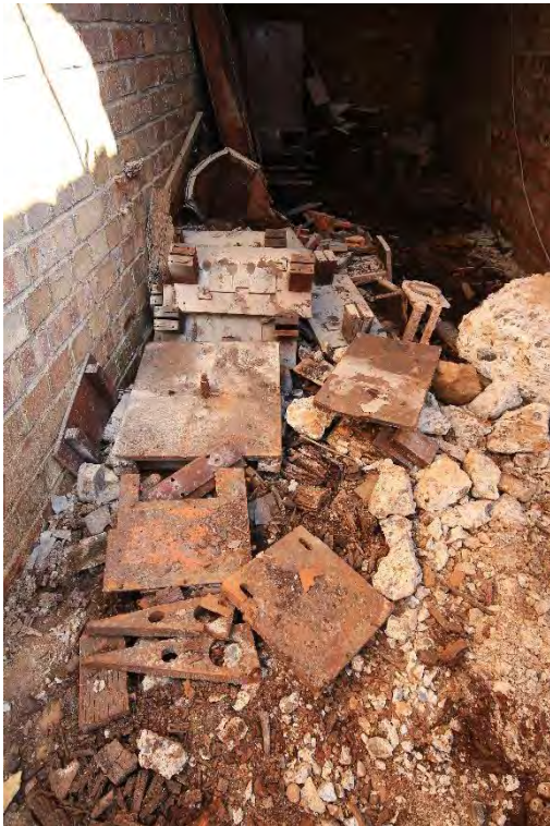
Plate 19: Shelter 4, collection of objects/materials and degraded timber planks found within the western gallery prior to asbestos removal works, facing north (28)
