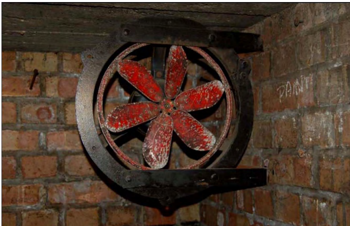
Plate 38: Shelter 2, example of the fan system providing air movement throughout Shelter 2, it is possible that Shelter 4 utilised the same system (FAU 2008, 52)
