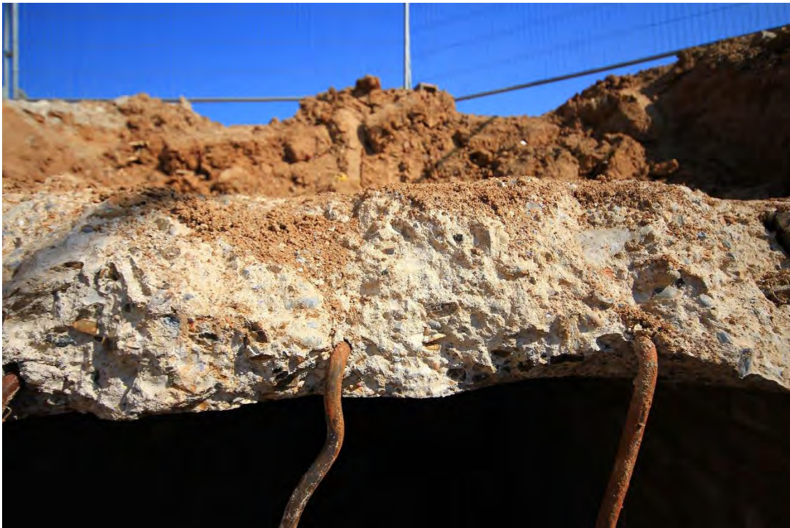
Plate 14: Shelter 4, detail of the reinforced concrete ceiling above the west gallery, facing north (30)
