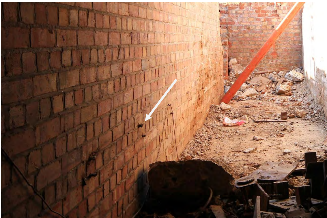
Plate 16: Shelter 4, detail of the redundant brackets formerly supporting the west gallery bench seating (no longer in-situ ), facing south-east (23)
