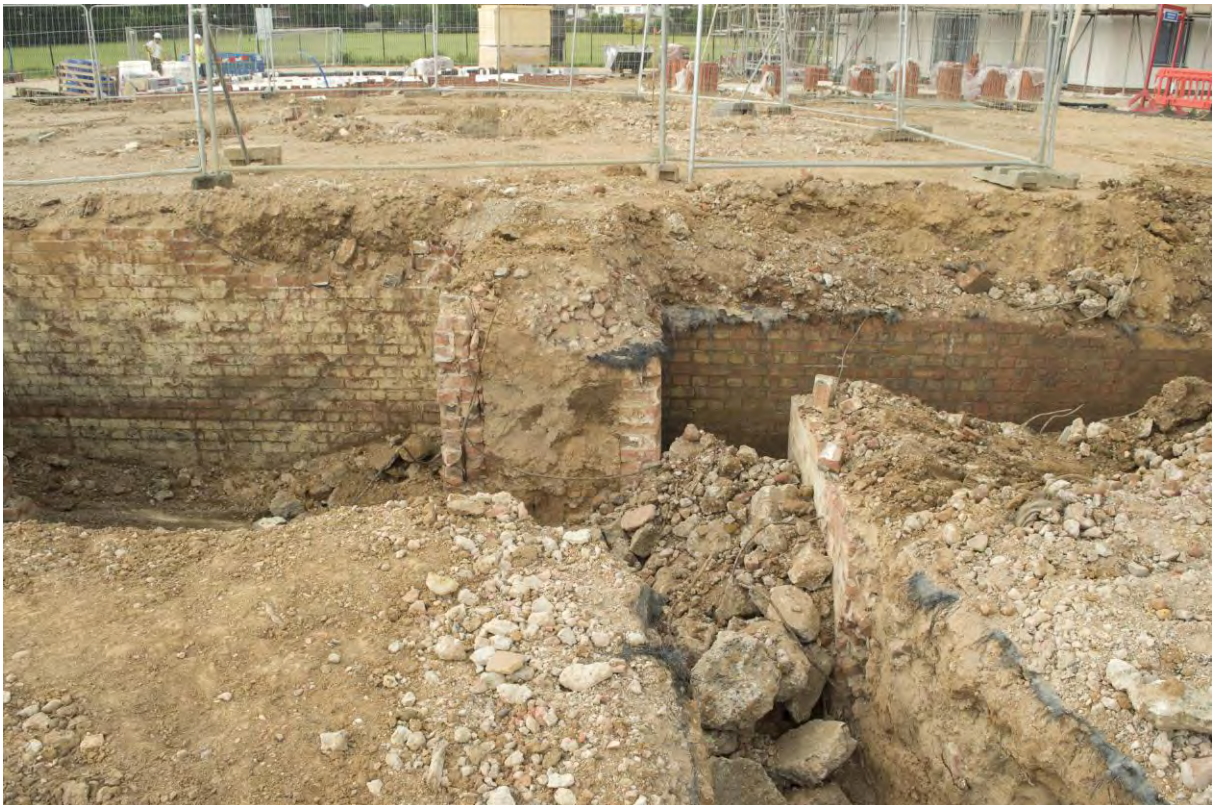
Plate 24: Shelter 4, excavated east gallery (left), baffle (middle) and entrance passage (right), facing west (162)
