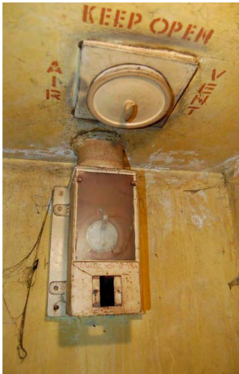
Plate 39: Shelter 1, example of the stink trap valve unit within the chemical closets in Shelter 1 (FAU 2008, 41)
