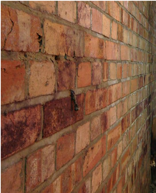
Plate 31: Shelter 4, protruding round headed steel pin (possible door pintle) located adjacent to the north-west chemical closet, facing north-west (13)
