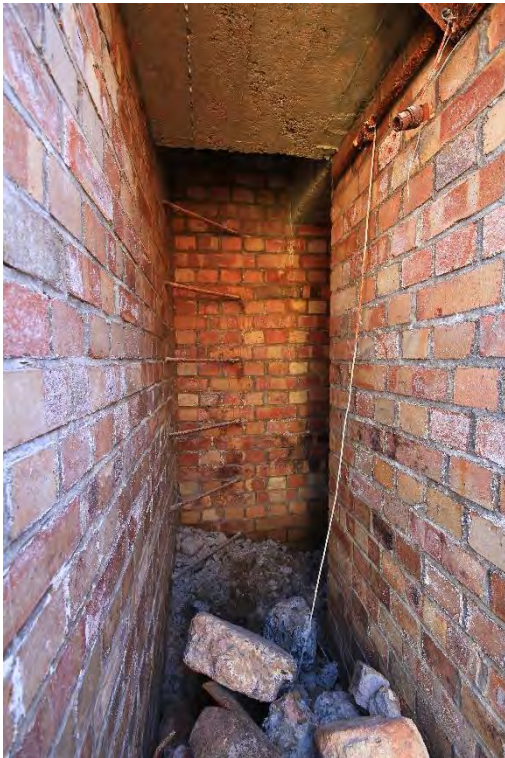
Plate 41: Shelter 4, southern passage providing access to the south-west escape hatch, facing east (33)
