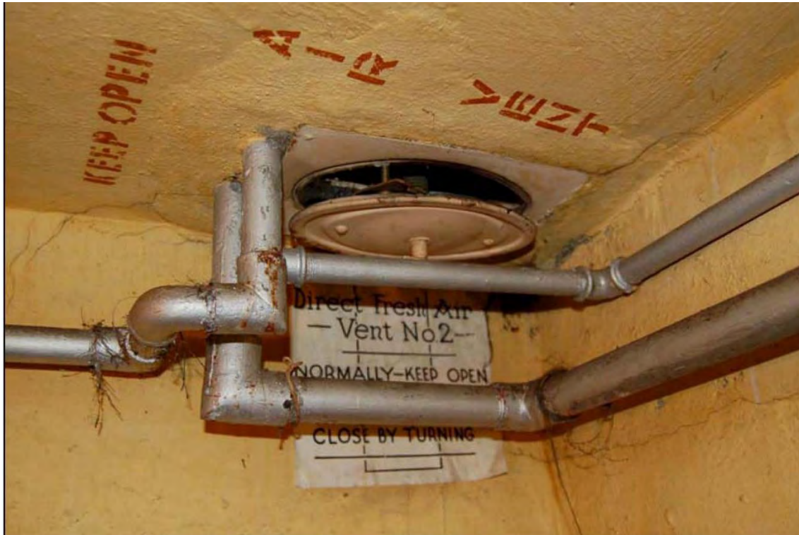
Plate 37: Shelter 1, well preserved example of a spring-loaded air vent within the changing area of Shelter 1. Note the instruction notices (FAU 2008, 37)
