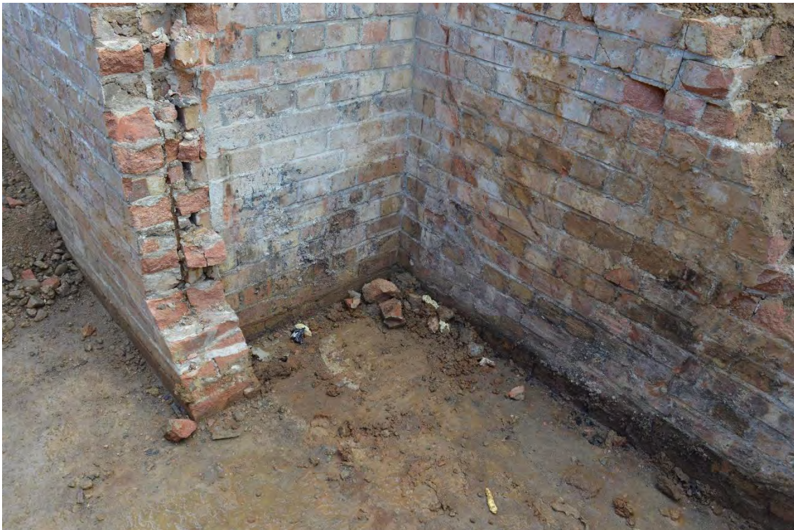
Plate 30: Shelter 4, detail of the scarring left by the former chemical toilet (removed) within the concrete screed flooring within the south-west closet, facing north-east (55)
