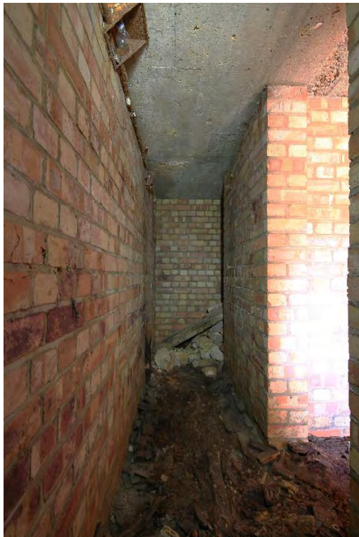
Plate 34: Shelter 4, view of the narrow passage opposite the north-west chemical closet, facing north (13)
