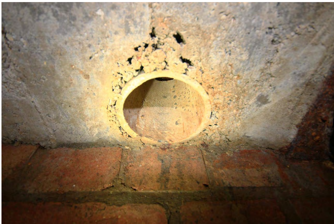
Plate 40: Shelter 4, redundant ceiling valve opening found within the north-west chemical closet that formerly held the stink trap unit, facing south (18)
