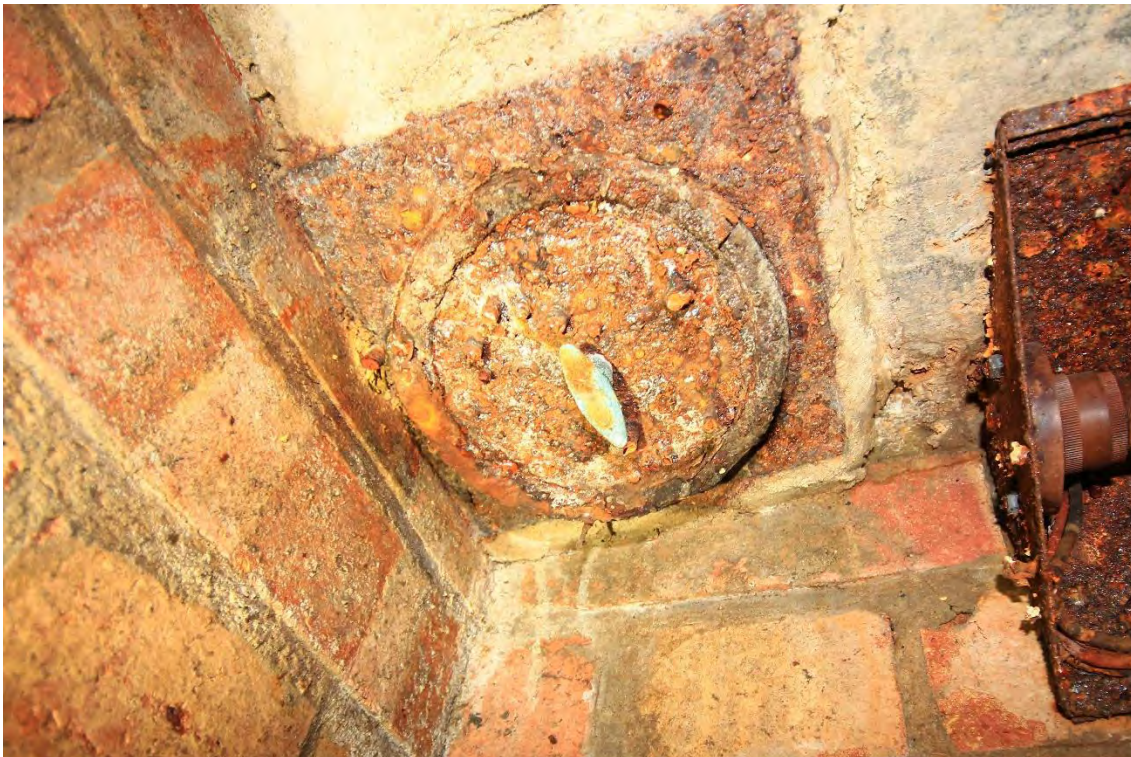
Plate 36: Shelter 4, spring-loaded air-vent located in the corner of the north-west chemical closet, facing south-west (16)
