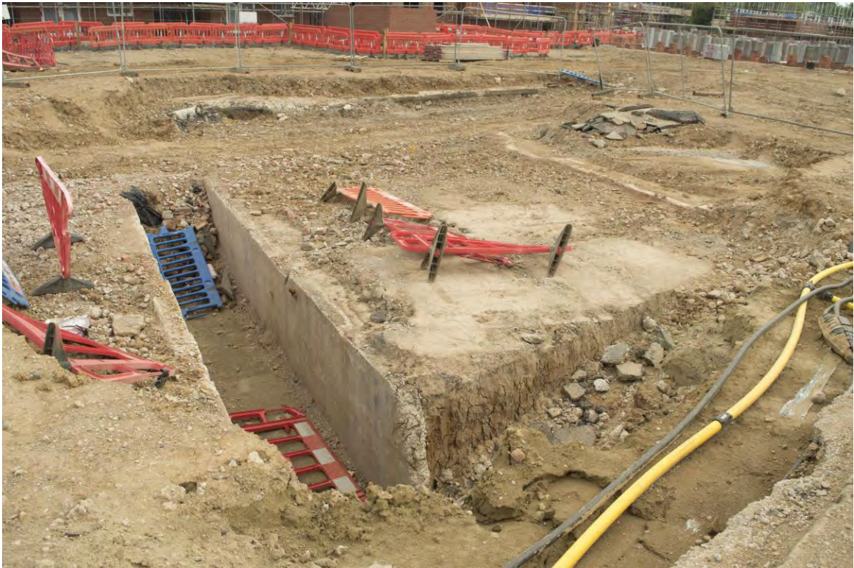
Plate 53: Service tunnel, east kerb of road to the top right of the frame, facing north-east (114)
