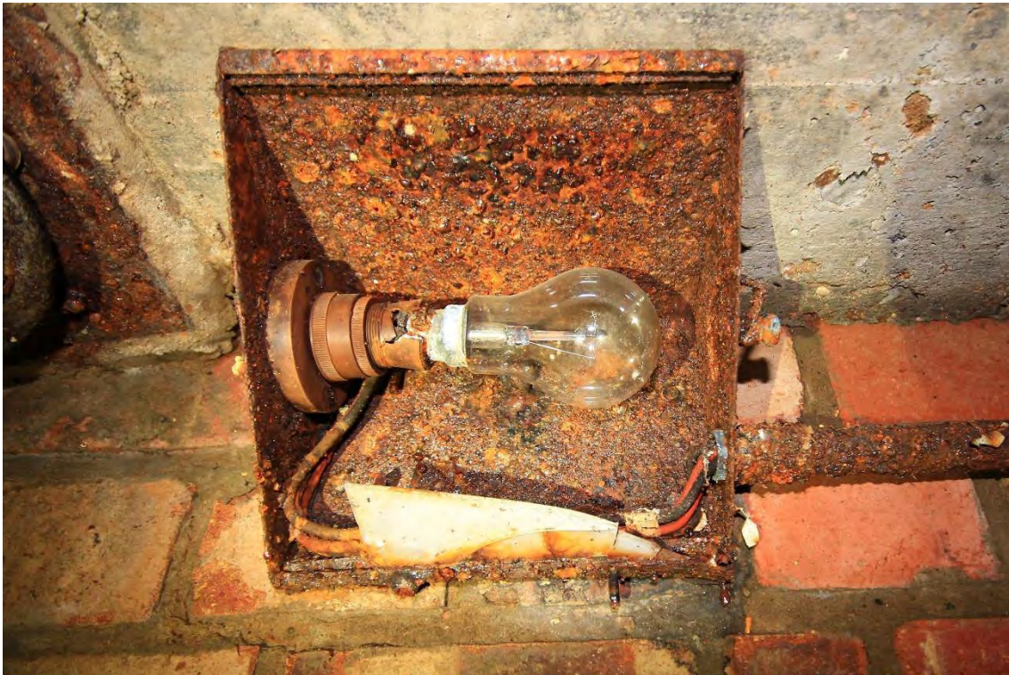
Plate 15: Shelter 4, typical example of the light fittings found throughout the structure, facing west (15)
