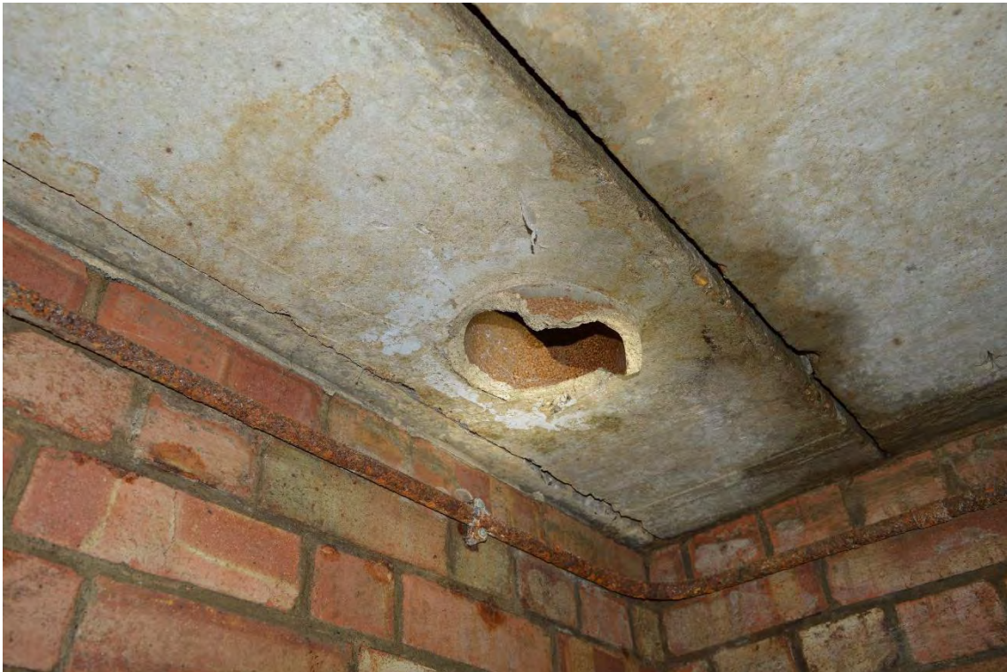
Plate 47: Shelter 4, detail of the redundant valve opening within the central circulation area, formerly serving ventilation purposes, facing south-east (63)
