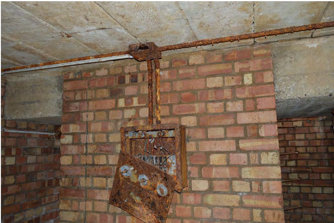
Plate 48: Shelter 4, detail of the electrical switch unit within the southern central circulation area, facing north (64)
