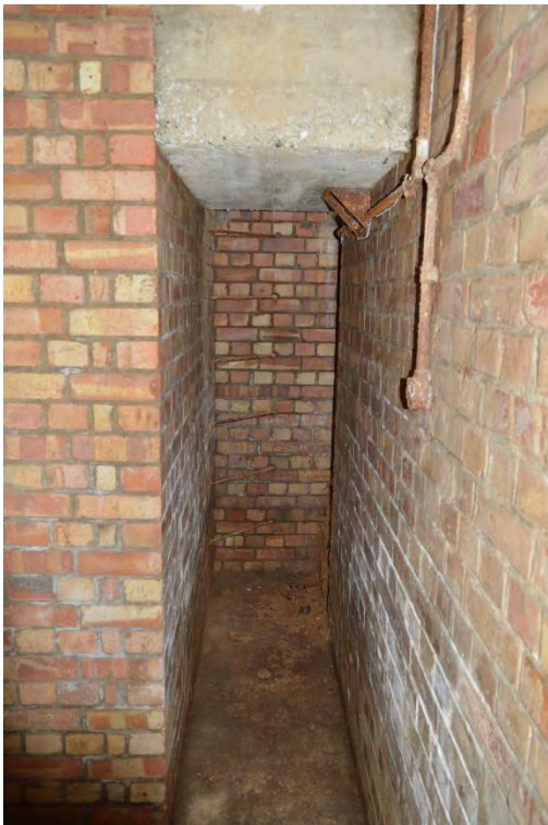
Plate 44: Shelter 4, view of the passage connecting the south-east escape hatch and central circulation area, facing north (67)
