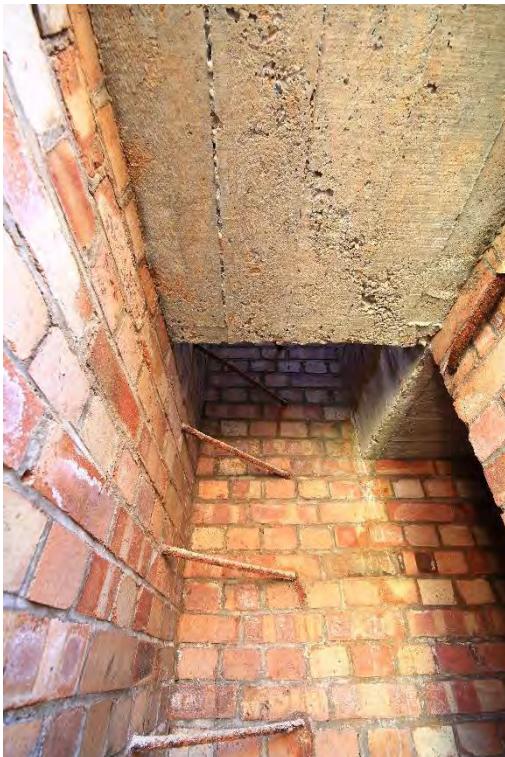
Plate 42: Shelter 4, south-west escape hatch with embedded metal rung access, facing east (up) (35)
