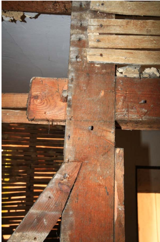
Plate 11: Detail shot of notched joint and carpentry marks on the exposed studwork, facing south (TRE16-0257)
