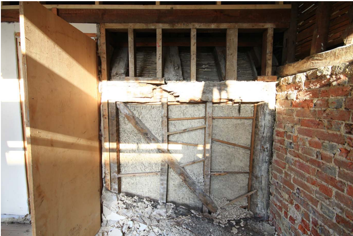
Plate 6: Exposed 19 th -century studwork and 20 th -century timbers and plaster within the 14 th -century framework of the hall range, looking west (TRE16-0243)
