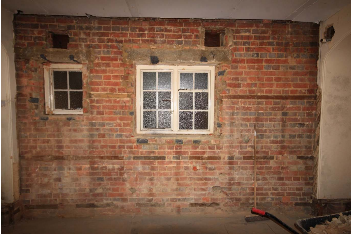
Plate 13: Exposed fabric of the east wall of the 1839-74 extension constructed in English bond with bond timbers, and two inserted windows, looking east (TRE16-0290)
