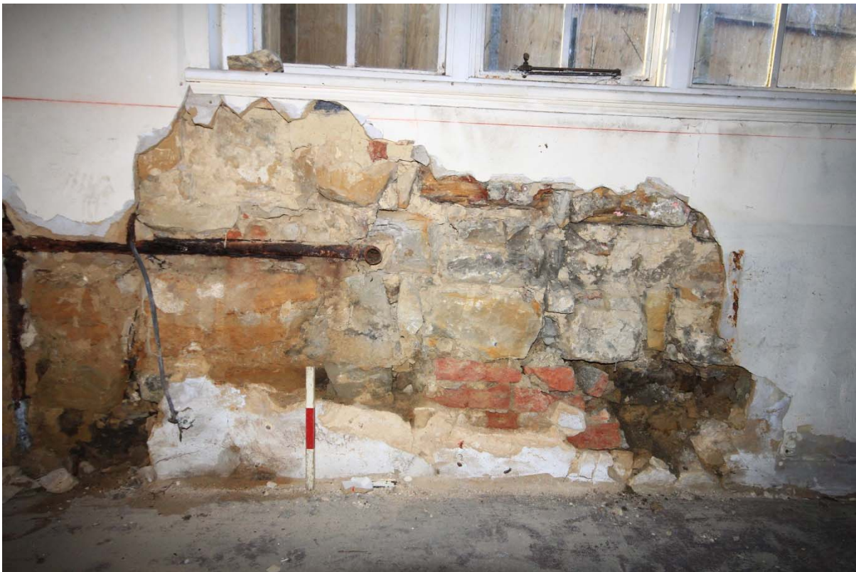
Plate 2: Exposed fabric of the south wall of the 18 th -century extension to the south-east of the crosswing, looking south (TRE16-0283)
