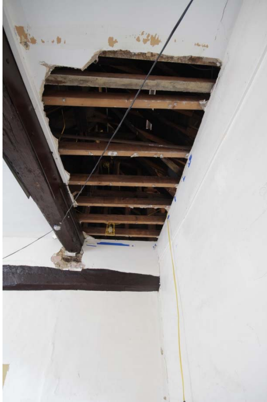
Plate 5: Exposed fabric of the inserted ceiling on the first floor of the hall range, looking north (TRE16-0218)
