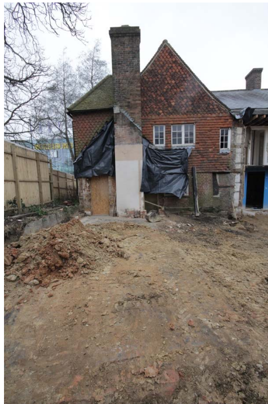
Plate 14: Exposed slab of the east extension to the cross wing, facing west (TRE16-0183)
