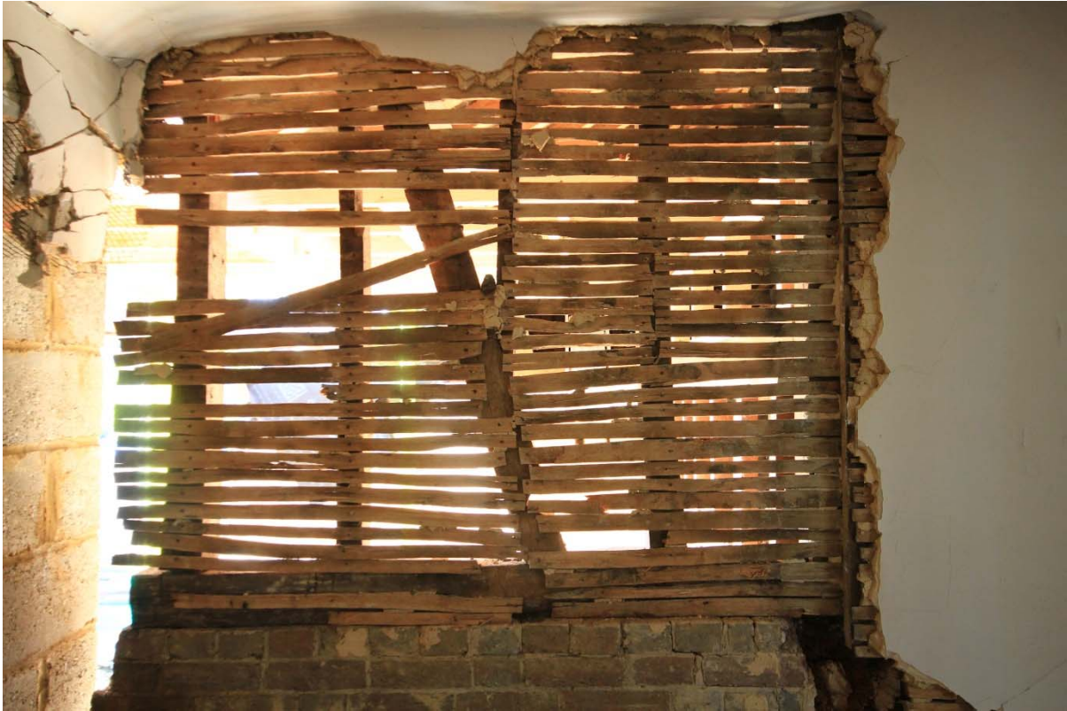
Plate 7: North wall of the east extension to the hall range, revealing 19 th -century studwork beneath lath-and-plaster, looking south (TRE16-0274)
