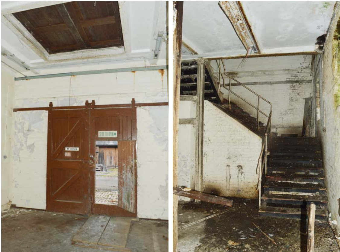
Plate 20 – Equipment store (Building 28), ground floor. Left: main doorway and goods hatch, looking north (SGA15-174). Right: main stair, looking east (SGA15-179)
