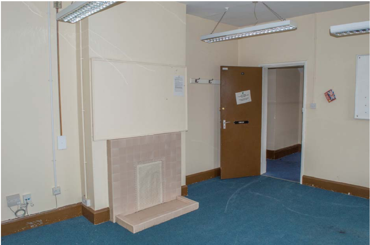
Plate 82 – Building 20: first floor, western servants' quarters, looking south-west. Note the replacement ceramic chimney-piece, matching those within the officers' rooms (SGA15-529)
