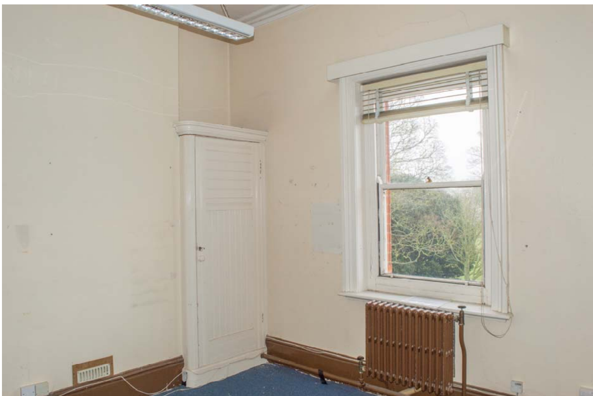
Plate 78 – Building 20: first floor, tertiary bedroom to commanding officer's quarters. View looking north-east (SGA15-506)
