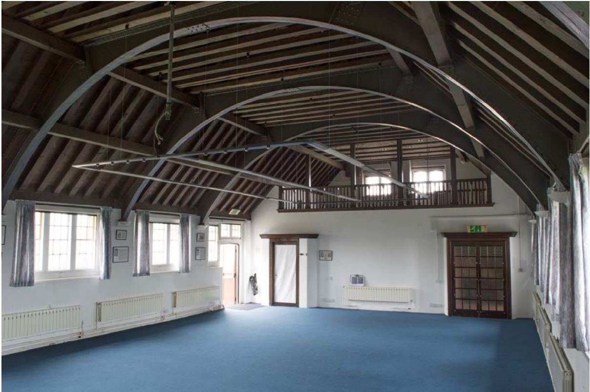
Plate 21 – Building 17: Sir John Moore Library, view of the hall, looking east towards the balcony (SGA15-232)
