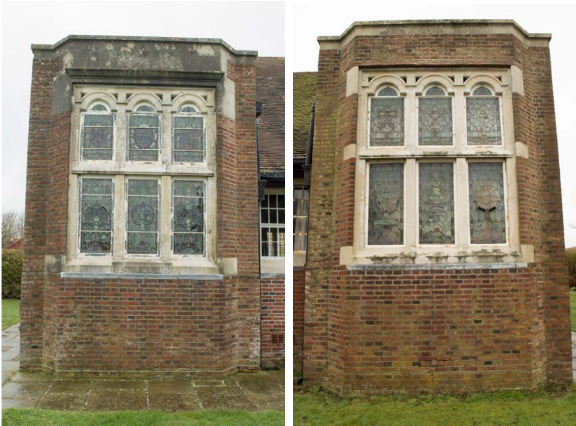
Plate 15 – Building 17: Sir John Moore Library, external view of stained glass to western bay windows (SGA15-303 & 310)
