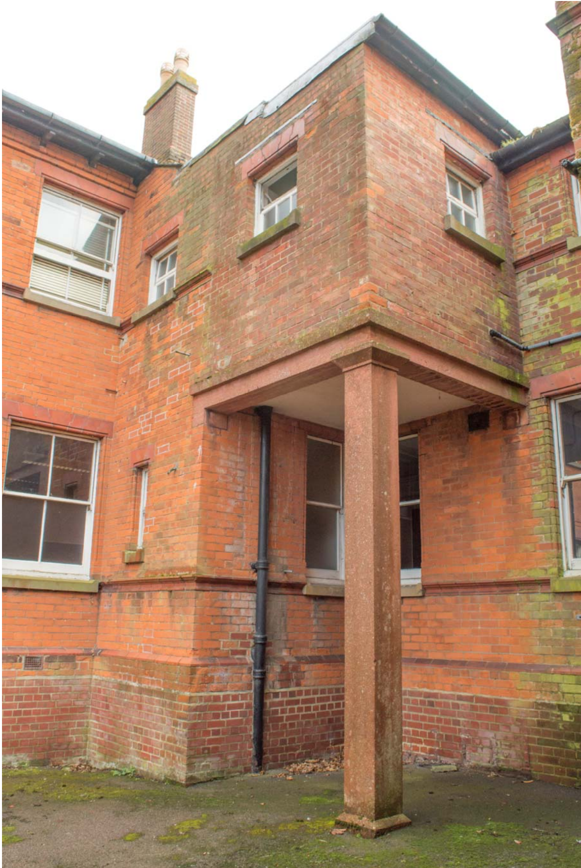
Plate 53 – Building 20: post-War sanitary extension to rear of commander's residence. View looking south-east (SGA15-395)
