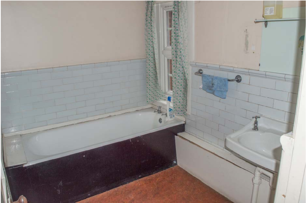
Plate 45 – Building 19: western house, first floor, bathroom to western extension. View looking south-west (SGA15-607)
