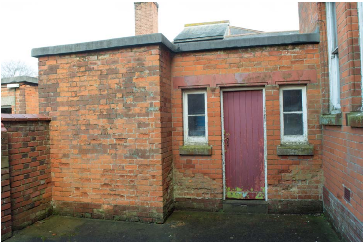
Plate 52 – Building 20: officers' mess, western service wing, example of servants' WC to rear yard. View looking east (SGA15-410)
