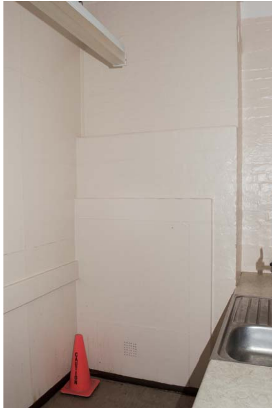
Plate 75 – Building 20: ground floor, fireplace to servants' room in field officers' wing (SGA15-493)
