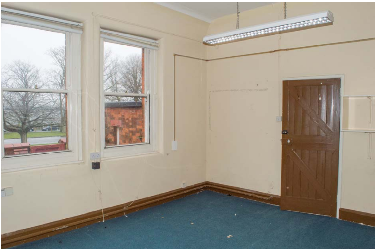
Plate 62 – Building 20: ground floor, servants' quarters to eastern side. View looking north-east (SGA15-446)
