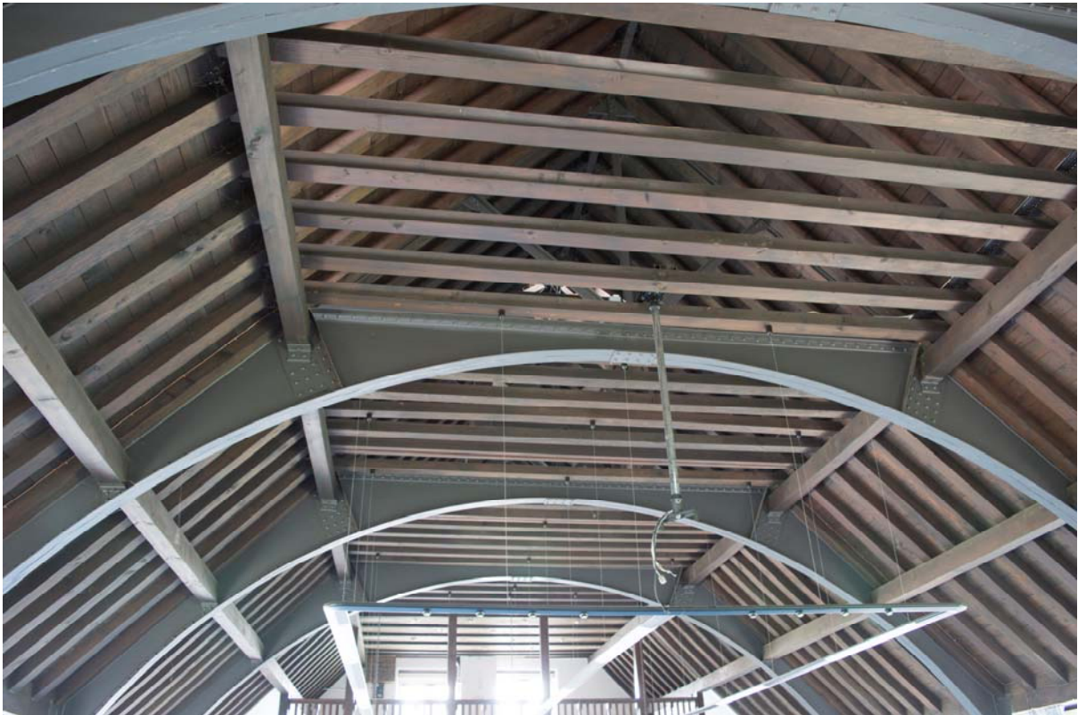
Plate 22 – Building 17: Sir John Moore Library, detail of the hall's roof, looking east (SGA15-244)
