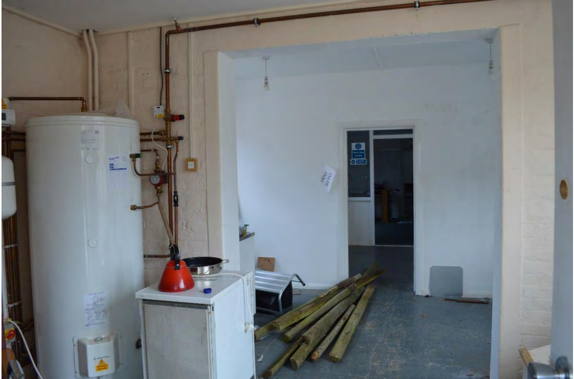
Internal view of the south-east projection of the rear range. Note the opening up of the original room proportions to accommodate an open-plan layout. View facing north-west (73)
