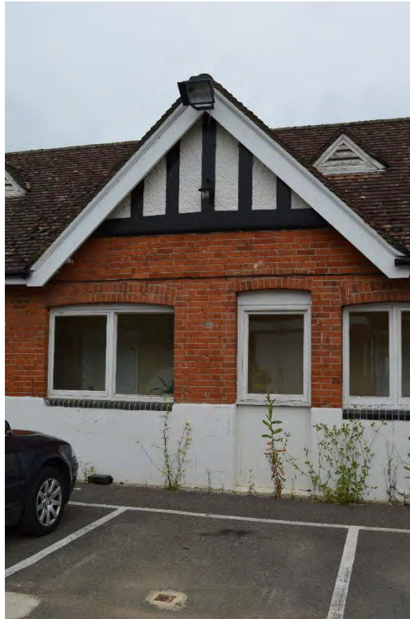
Detail of the window and door rearrangement present on all elevations of the rear block. Note the pebbledash and concrete render (south-east elevation), facing north-west (38)
