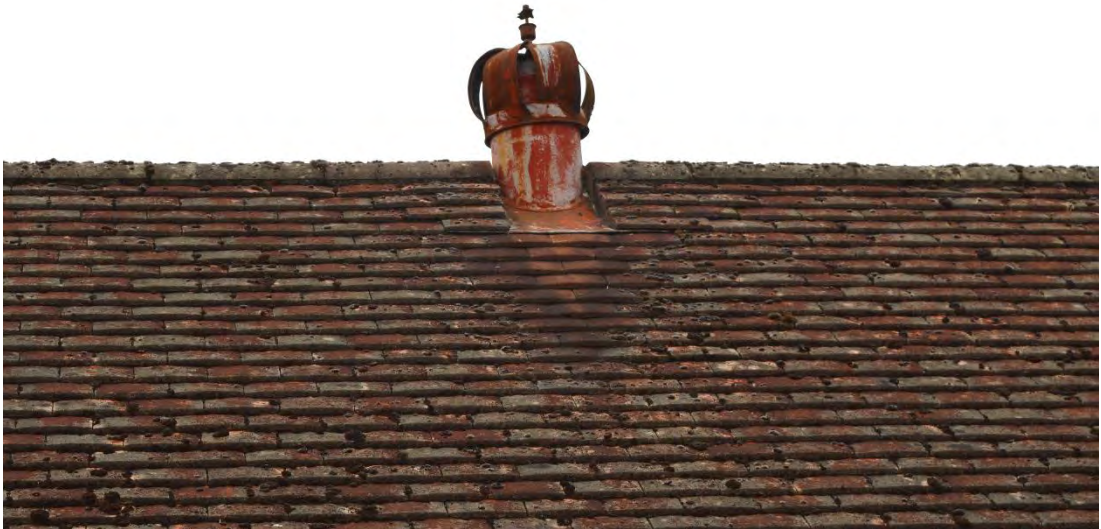
Crown shaped roof vent located on the north-east elevation of the rear block, facing south-west (44)
