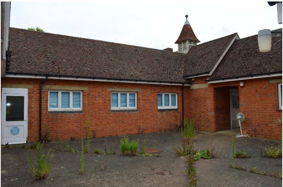
View of the south-west elevation of the rear north-east range of the rear block, facing north-east (30)
