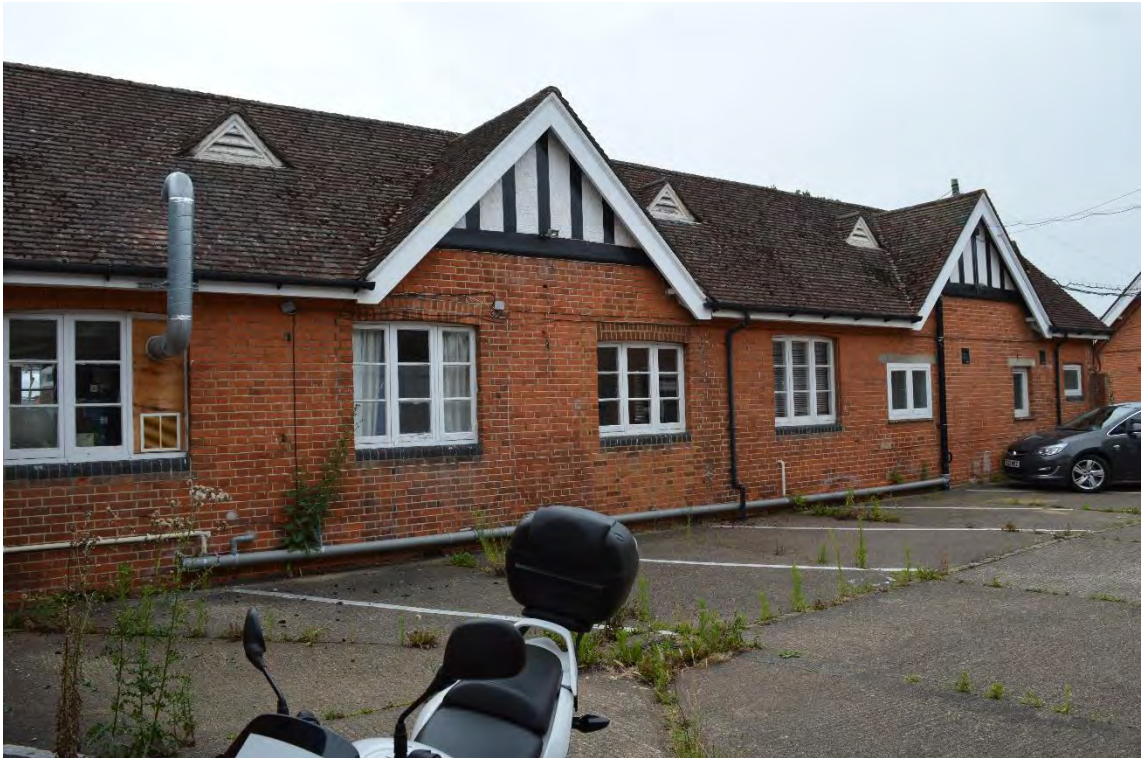
View of the north-west elevation of the rear block's south-east projection, facing north (32)
