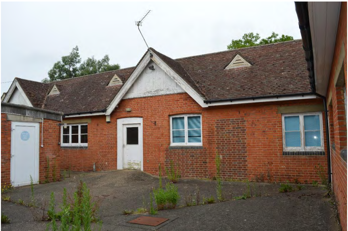
View of the south-east elevation of the north-west wing of the rear block, facing north-west (29)
