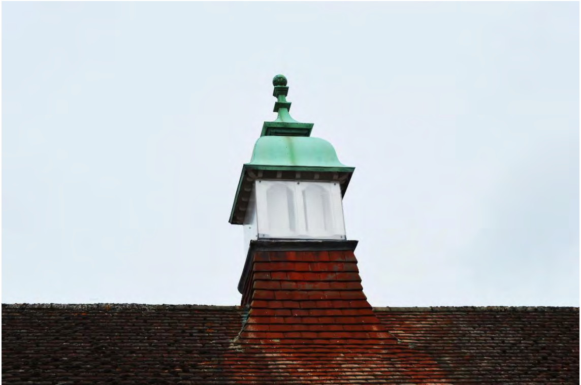
Copper-roofed lantern situated centrally upon the south-east range of the main college building, facing north-west (10)
