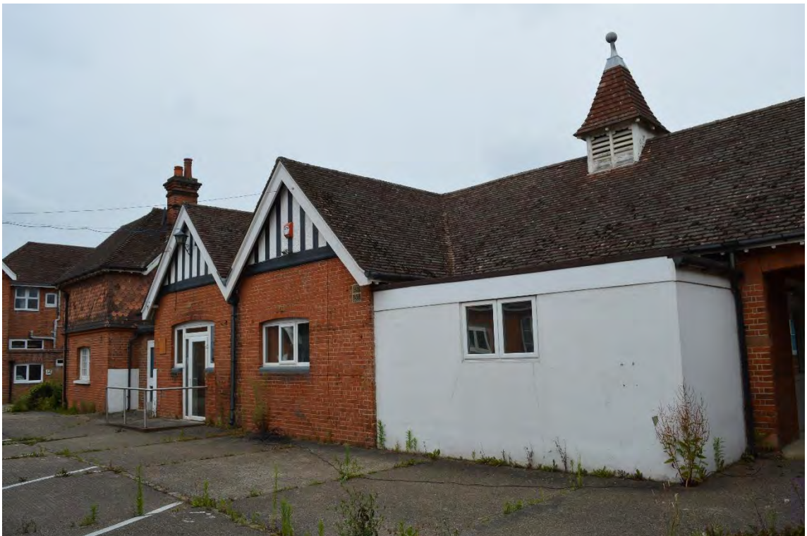
View of the south-east elevation of the central projection of the rear block, facing west (33)
