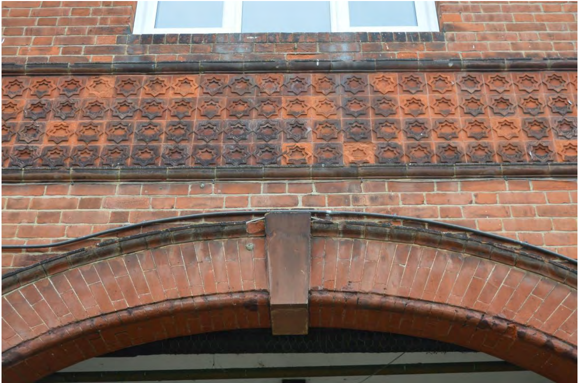
Detail of the gauged brick arch and decorative frieze above the north-east passageway providing access into the courtyard, facing north-east (18)
