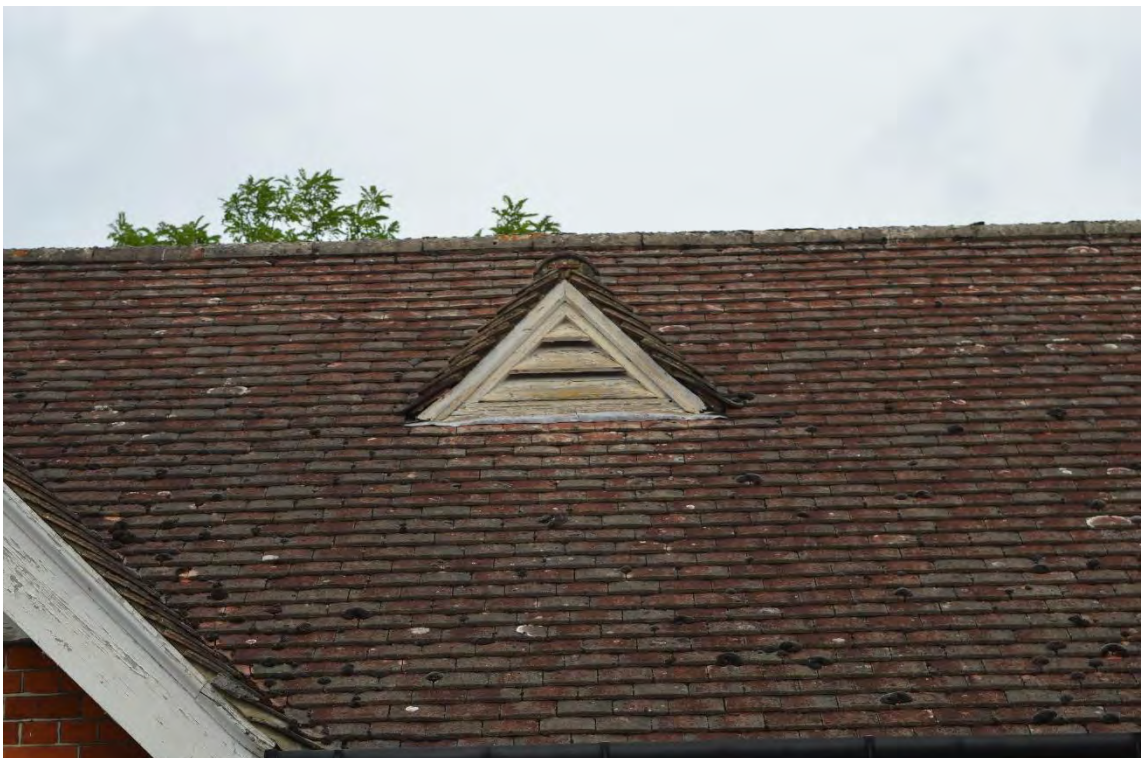
Detail of the timber slated air vents located throughout the rear block, facing north-west (31)
