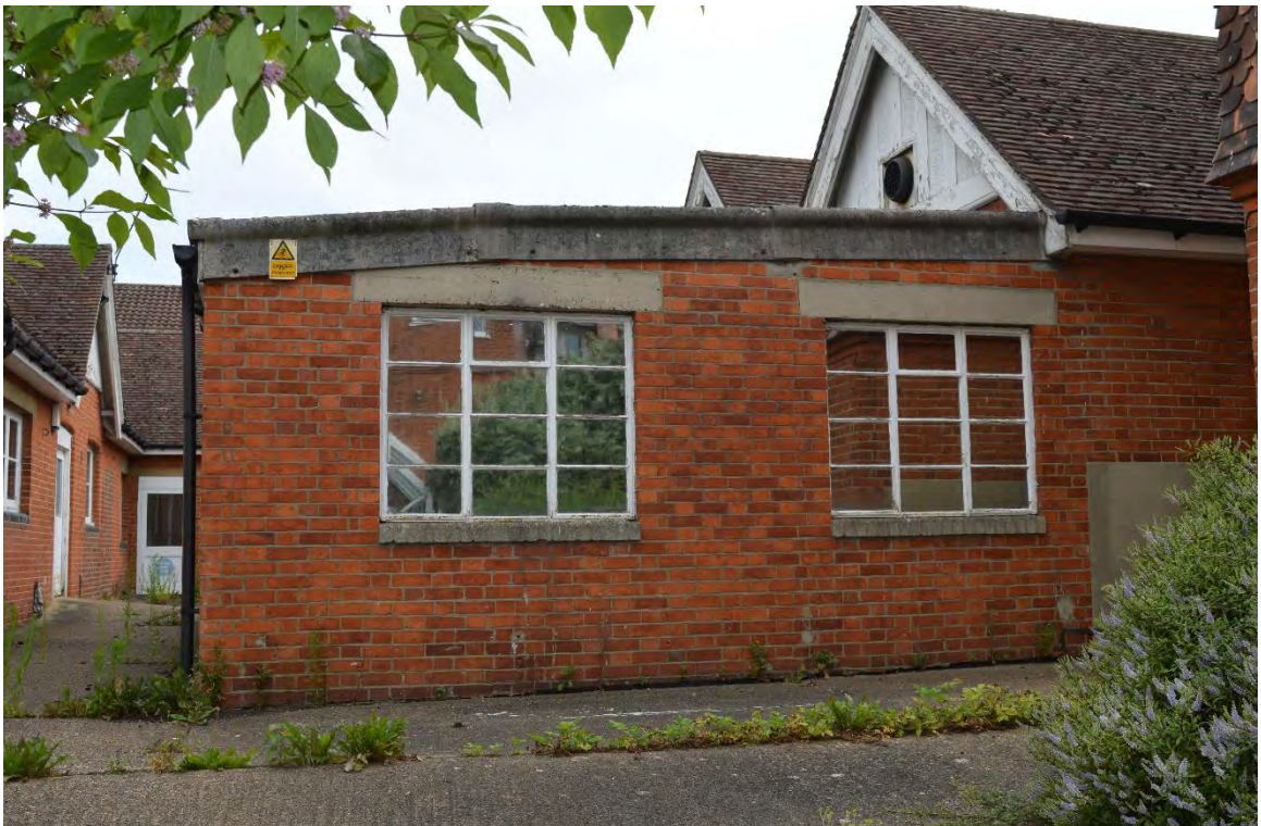
View of the north-west yard, infilled with a mid/late 20 th century extension (in situ by 1949), facing north-east (26)
