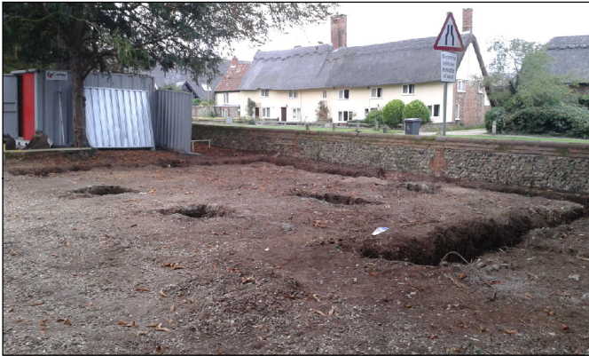
C. View of the site following excavation of the footing trenches (looking south-west)
