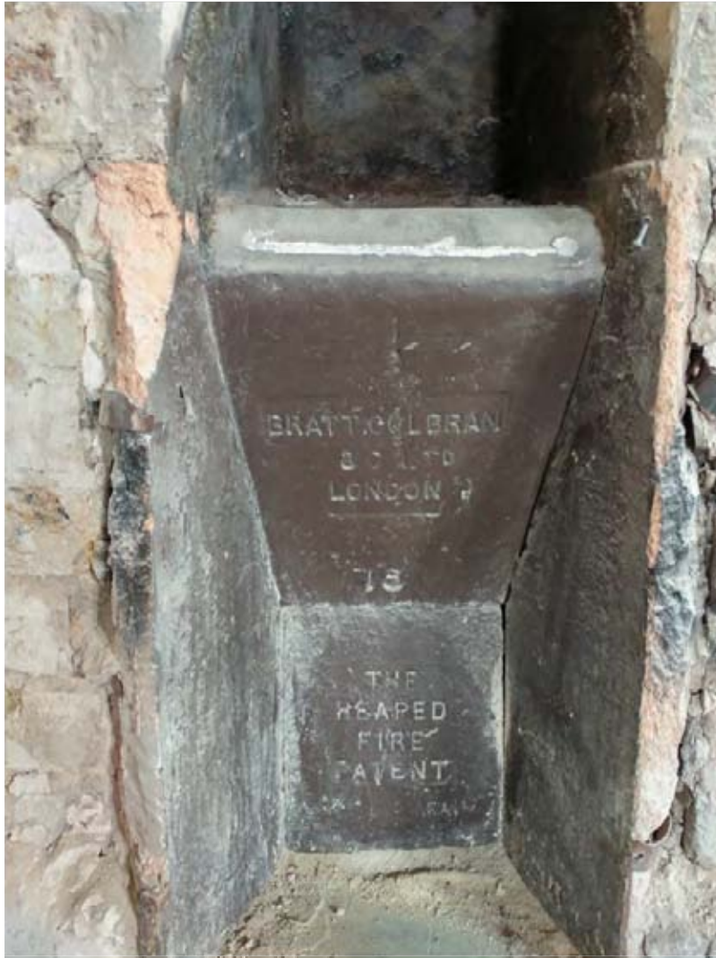
Plate 63: Heaped Fire gas fire in servant's quarters (#BCA16-0017)
