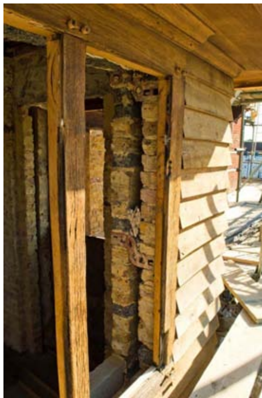
Plate 4: Window frame and cavity wall at first-floor level showing cavity-wall bricks, concrete bricks, and buff stock bricks (#BCA16-0121)
