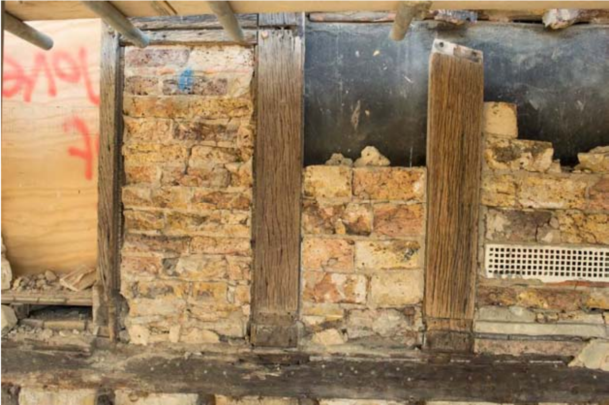
Plate 5: Half-timbering exhibiting morticing, with irregular brick infill to panels (#BCA16-0071)
