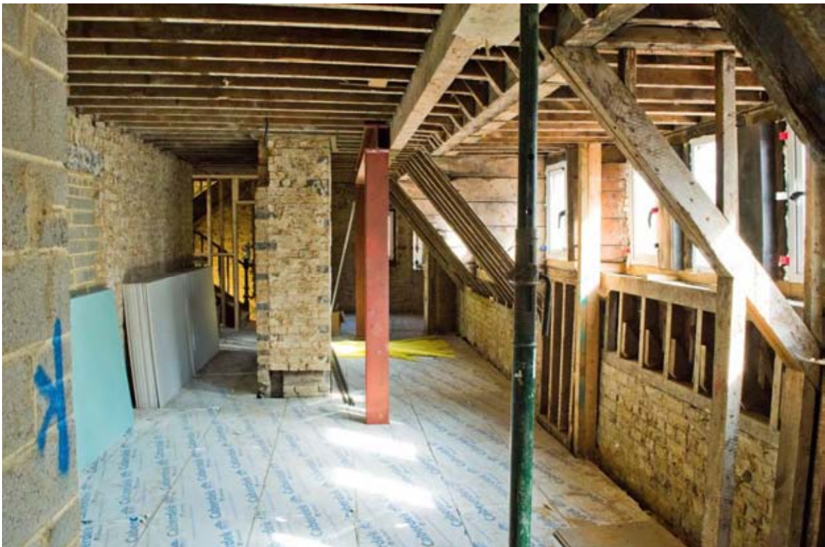
Plate 58: Looking north along the former spinal corridor at first-floor level – Note that previous room divisions along the east side of the corridor have been removed (#BCA16-0198)
