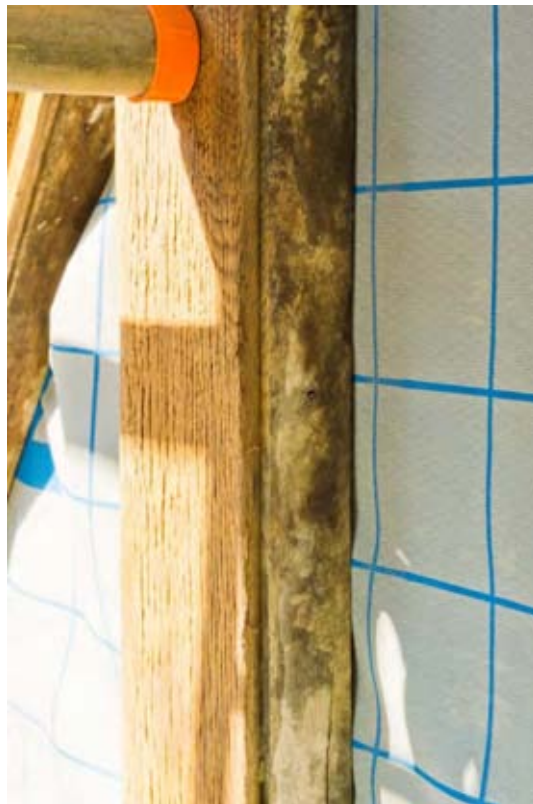
Plate 6: Section through half-timbering in the east gable of the east wing (#BCA16-0128)
