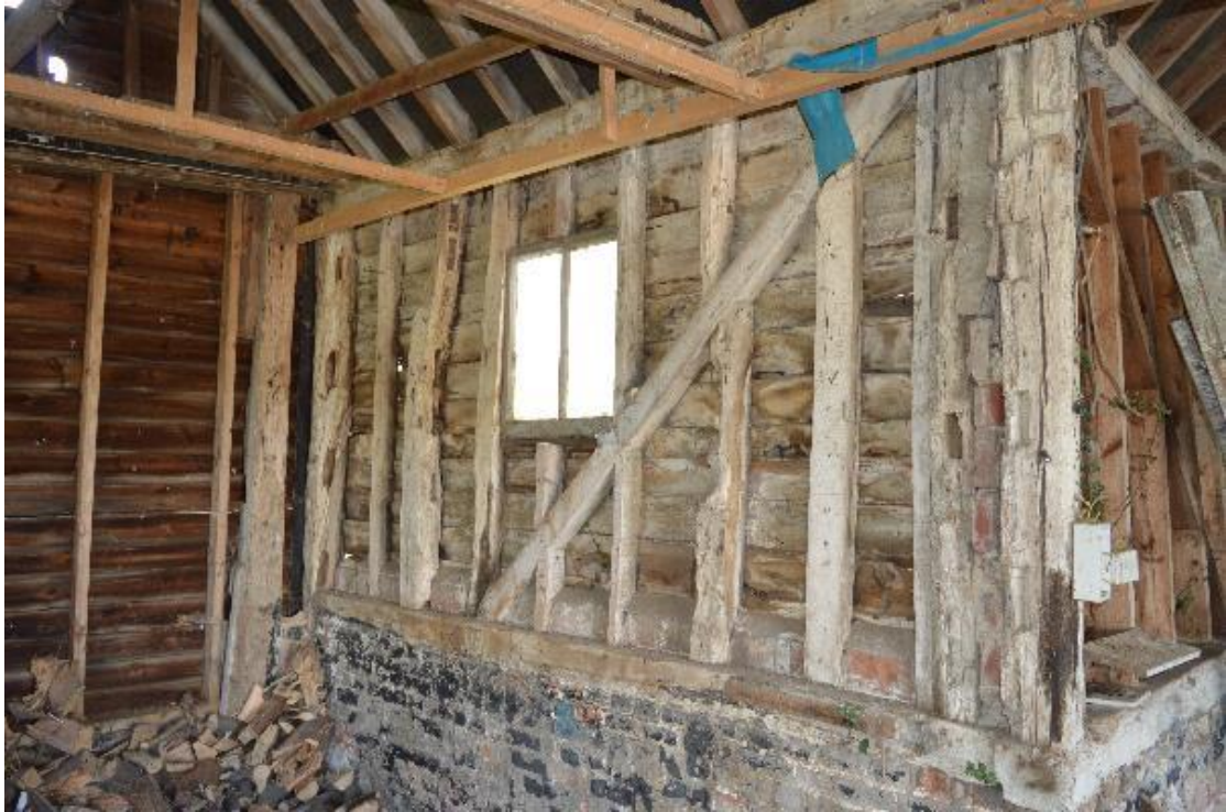
Plate 17 View of the mixed stud arrangement within the wagon porch, note original and modern timber use, facing south-west (32)
