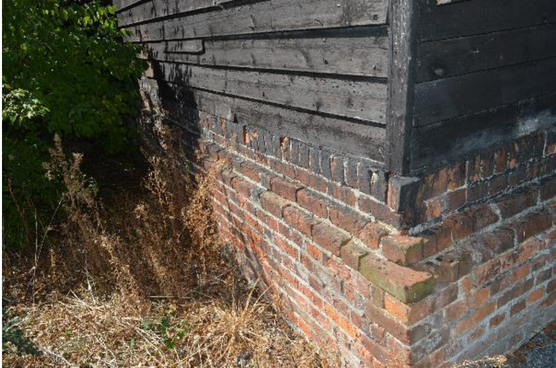
Plate 3 View of the brick dwarf wall supporting the barn's timber frame, facing south-west (39)
