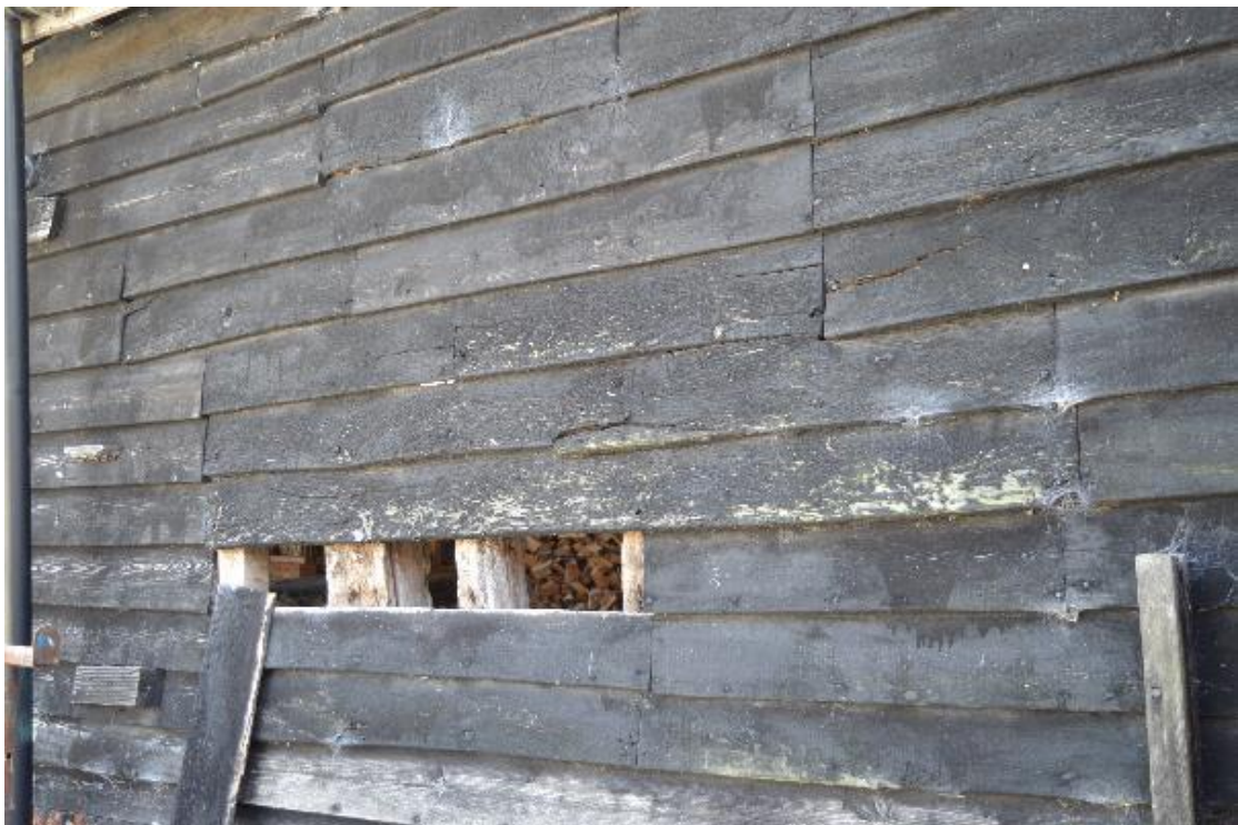
Plate 2 Detailed view of the retained weather boarding located within the barn's north elevation, facing south-east (25)
