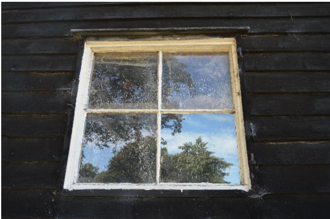
Plate 6 Detail of the window and redundant pintels retained within the east elevation, facing west (38)
