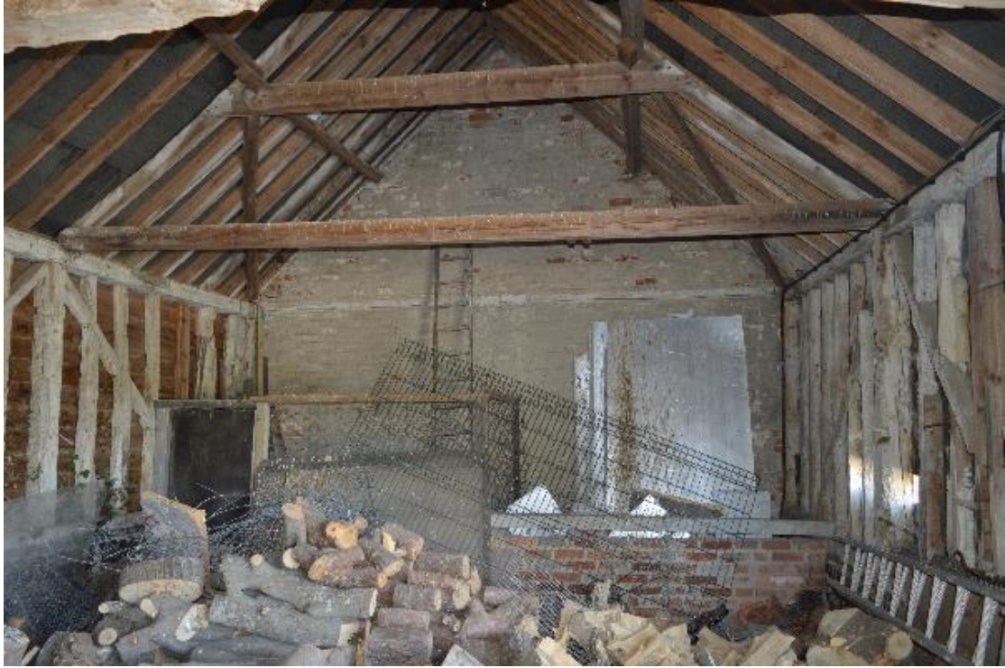
Plate 23 Western end (Bay 5) of the main body of the barn, inserted dog pen, facing west (34)
