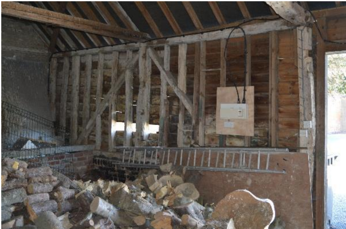
Plate 18 Detailed view of the north side of Bay 4 showing replacement studs, facing north-west (right) (32)
