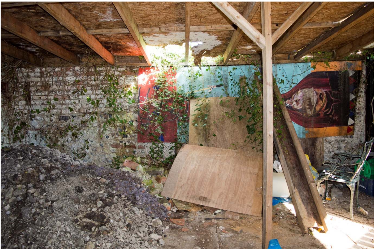
Plate 16: North wall of northern shelter, showing original enclosure walls at base, with later, probably early 20 th century brickwork above (63)
