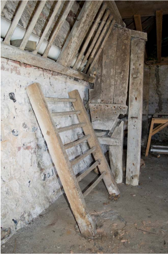
Plate 13: Detail of hay-rack. Note the brick ledge which is integral to the wall, thus indicating the hay-rack to be an original feature (49)
