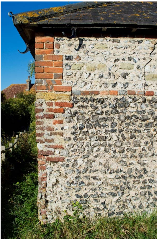
Plate 2: Variation in the wall construction, showing early fabric below and later fabric above (10)
