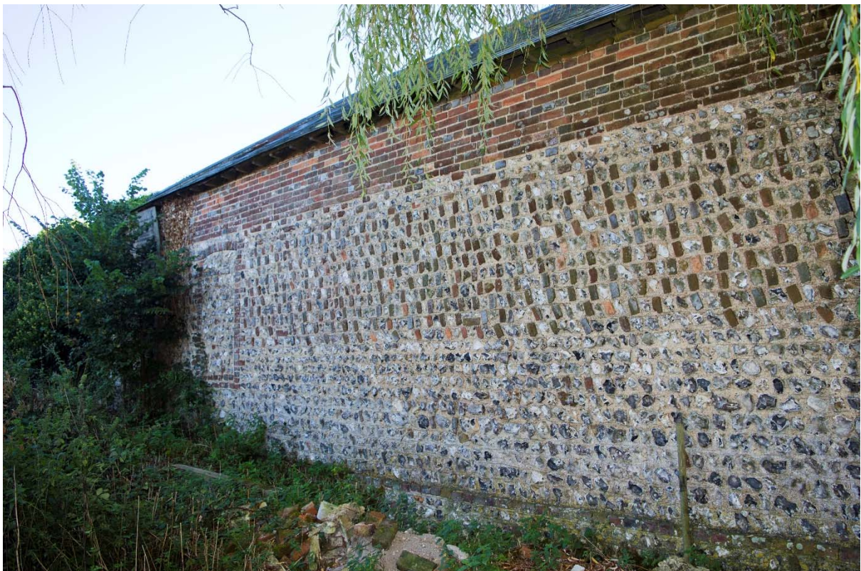
Plate 4: West elevation of the building, showing the different materials used in its construction. Note the blocked opening towards the north end (18)
