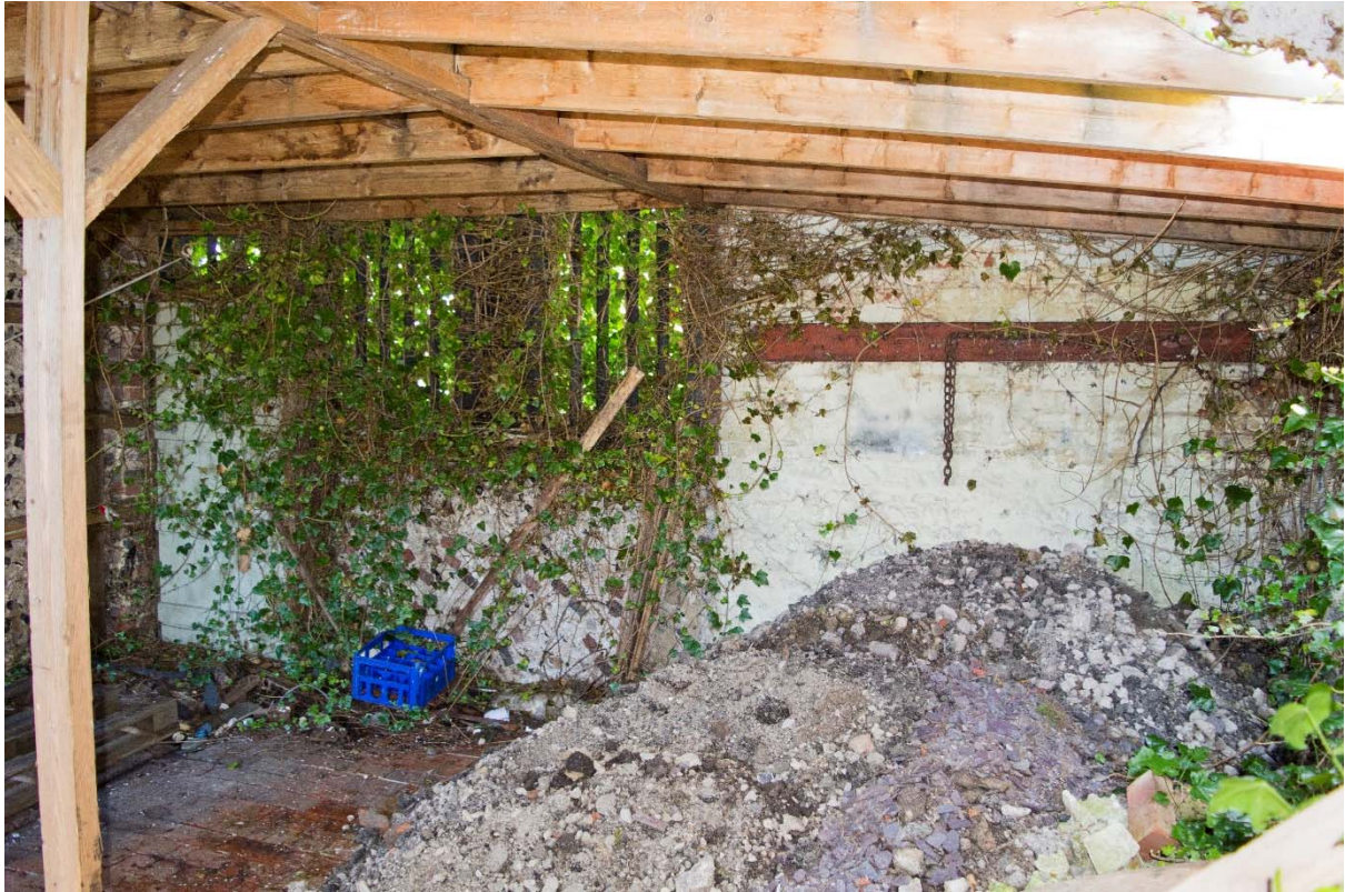
Plate 17: West wall of northern shelter, showing original enclosure walls at base, with later brickwork (right) and timber mullions (left) above. Note the early/mid-20 th century door to far left (62)
