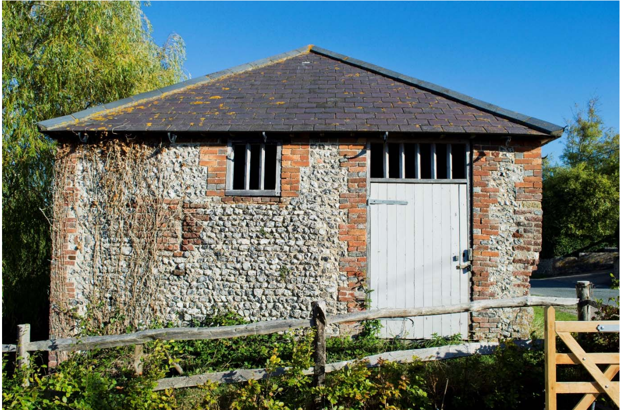
Plate 3: South elevation of the building, showing early fabric contained within the lower portion. Note the blocked window towards the left-hand side (11)
