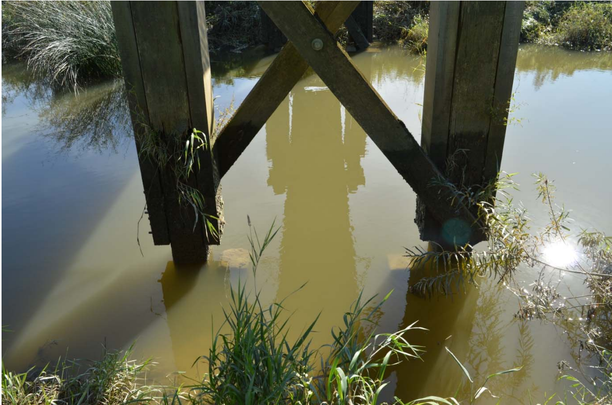
Plate 4: Submerged possible former piles visible just beneath the water below the existing bridge (#EFO16-0060)
