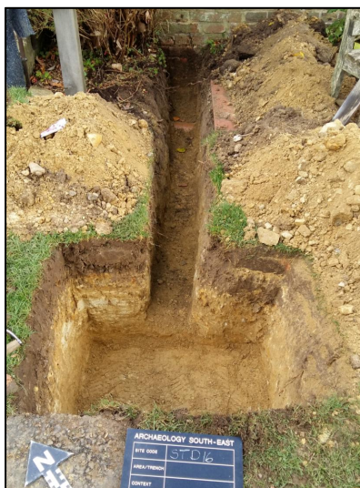
View of junction box pit beside potting shed
