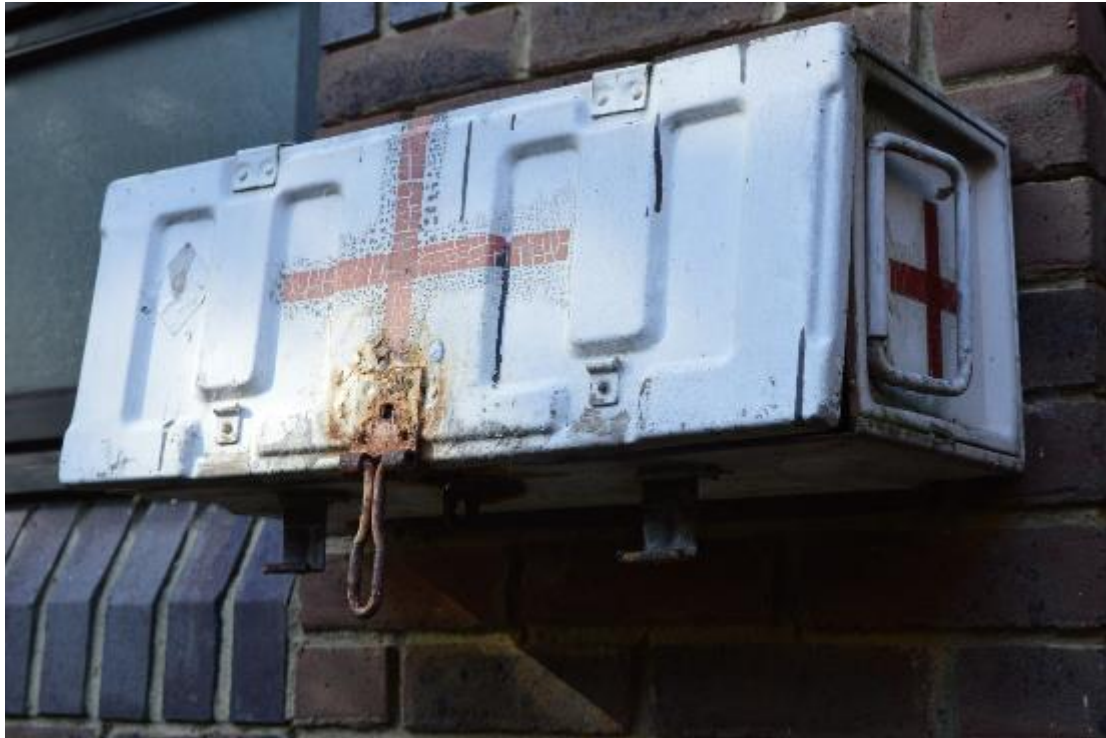
Plate 201: Building 25, south elevation passage, first aid box (863)
