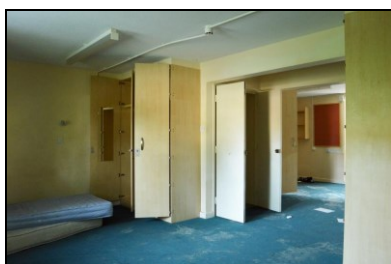
HOB16-0835 Building 25, typical communal bedroom / lounge interior at ground, first and second
