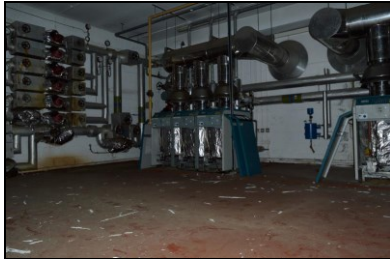
HOB16-0856 Building 25, plant room
