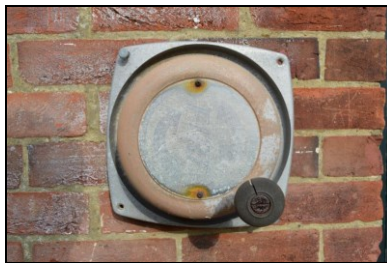
HOB16-0446 Building 11, north elevation, fire alarm
