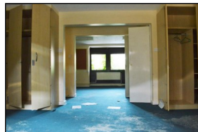
HOB16-0834 Building 25, typical communal bedroom / lounge interior at ground, first and second floor levels within all blocks
