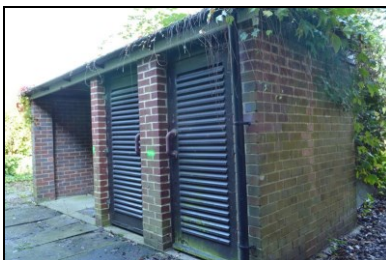
HOB16-0290 Building 4, electricity sub-station (east)
