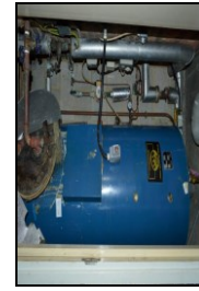
HOB16-0855 Building 25, typical stairwell boiler
