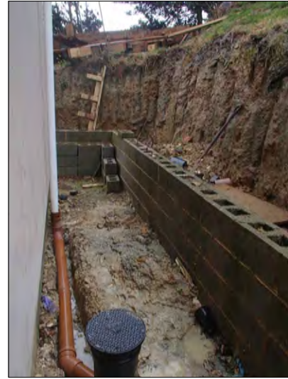
Location of drainage trenches. Note that the entire area is terraced into the hillslope to a depth of over 2m
