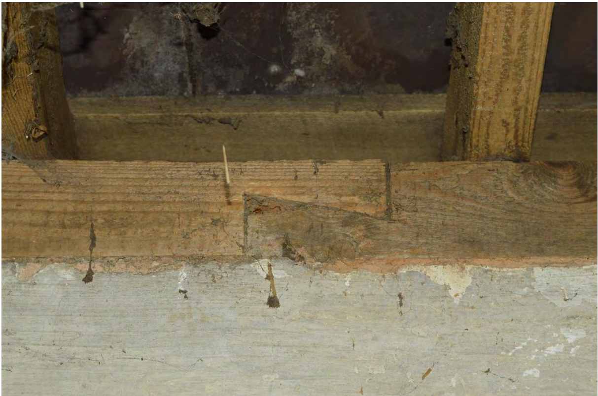
Plate 24: Building D, north unit, first floor level hay loft, detail of scarf joint to wall plate, facing east (171)
