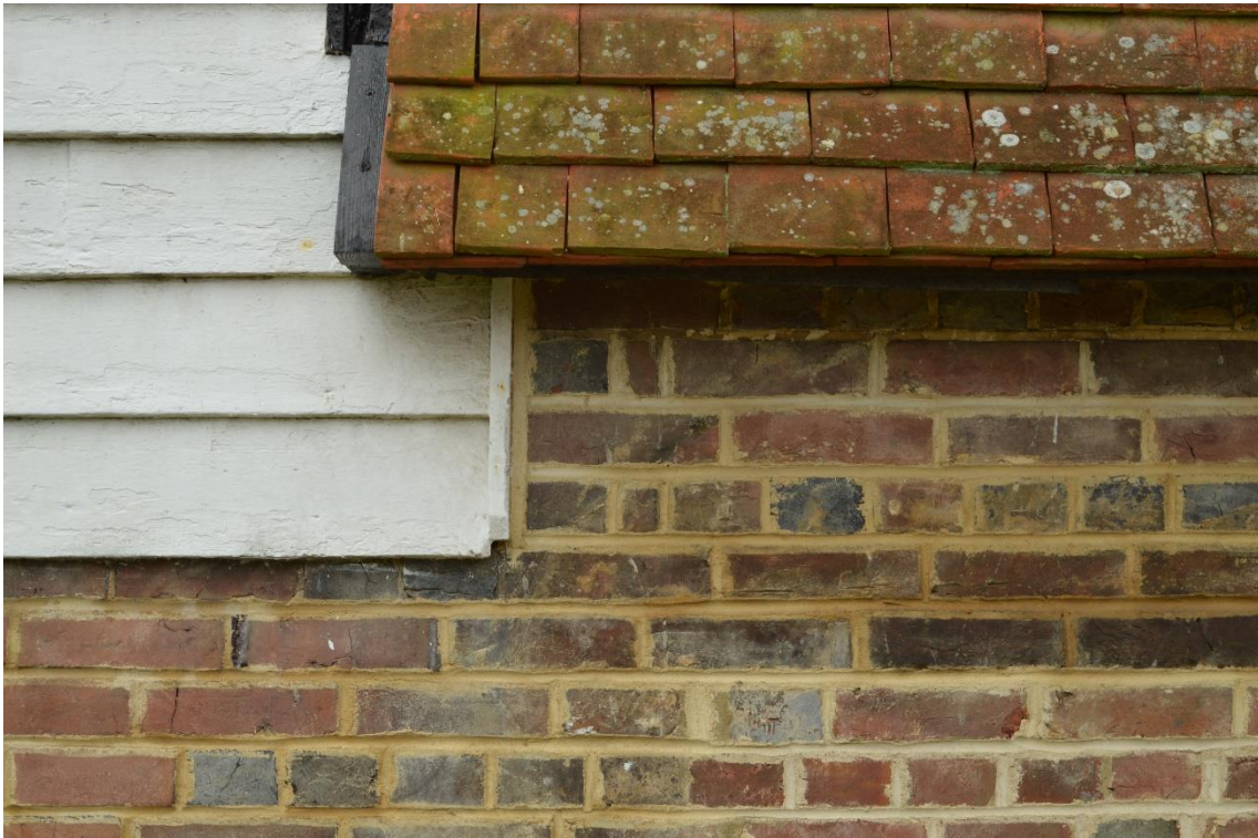
Plate 4: Queen closers at junction of east wall of farmhouse and lean-to, facing west (PEL17-0009)
