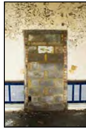
RER16-0053 G2 - Blocked opening to G13. Facing south
