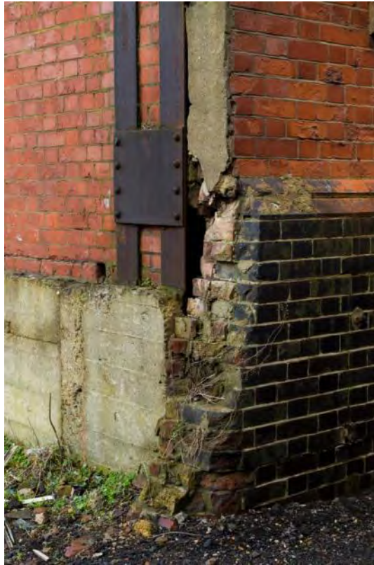
Plate 20: Crudely truncated brickwork on the south side of the west elevation (#RER16-0020)
