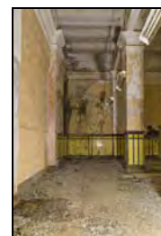
RER16-0129 Control Room F15 - Overview. Facing south
