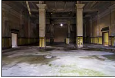
RER16-0239 Control Room F15 - Overview. Facing east
