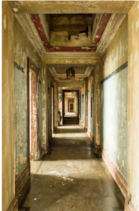
Plate 82: View east along second-floor corridors – note the blocked skylight (#RER16-0201)
