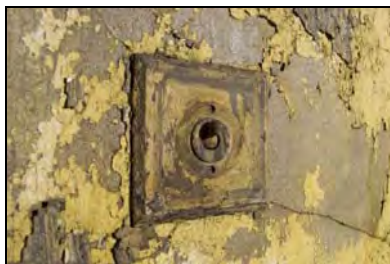
RER16-0221 Typical light switch. Facing south-west
