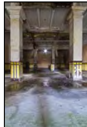
RER16-0245 Control Room F15 - Overview. Facing east
