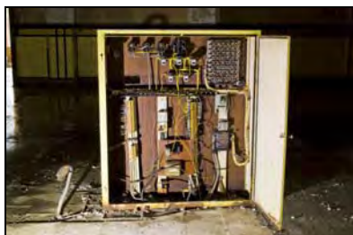
RER16-0124 Control Room F15 - Rear of panel. Facing north
