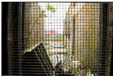
RER16-0220 Blocked doorway to roof space. Facing south
