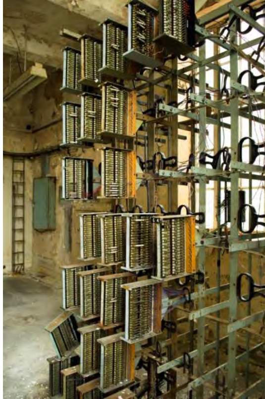
Plate 33: Telephone exchange panel, Room G5 (#RER16-0092)
