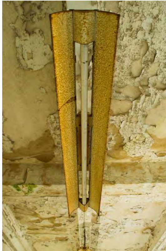
Plate 86: Light fixture in Room S1 (#RER16-0222)
