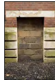
RER16-0024 South Elevation - Blocked opening. Facing north
