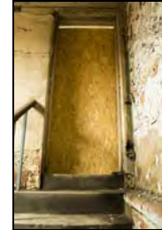
RER16-0183 Secondary Stair blocked egress to roof space. Facing north
