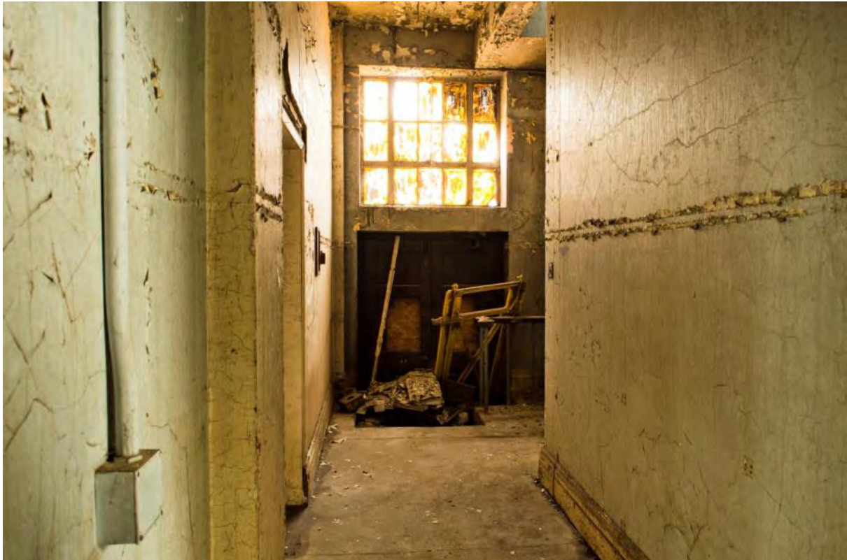
Plate 43: Corridor south of Room G8, facing a blocked egress to the east side of the building (#RER16-0076)
