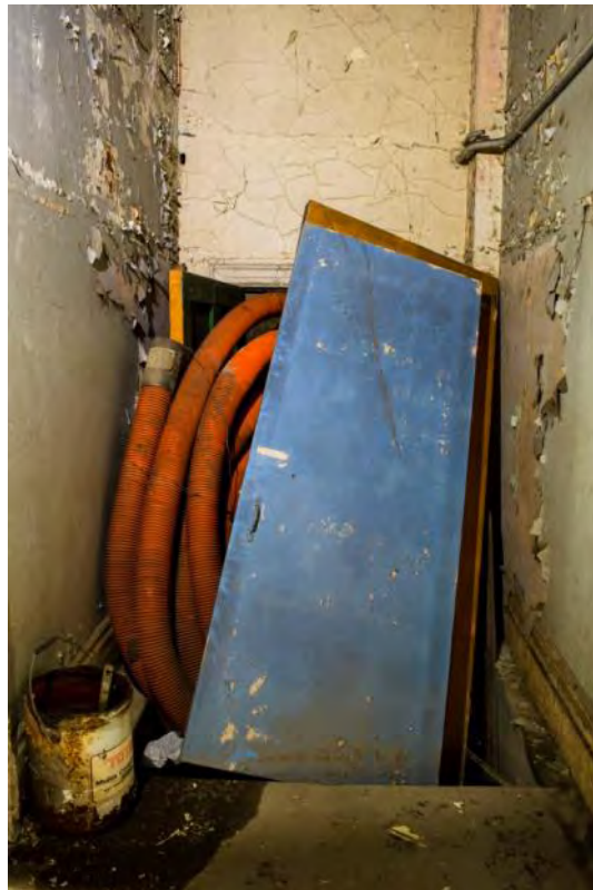
Plate 42: Blocked entrance to Room G12 (#RER16-0086)
