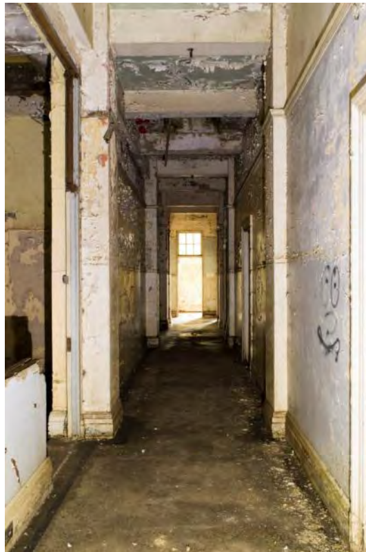
Plate 64: Looking north along the corridor towards Room F7. Note Room F11 to the left (#RER16-0170)
