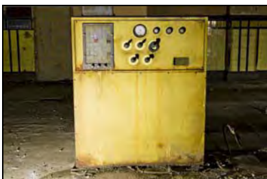
RER16-0125 Control Room F15 - Control Panel. Facing south
