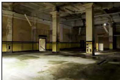
RER16-0121 Control Room F15 - Overview. Facing north-east
