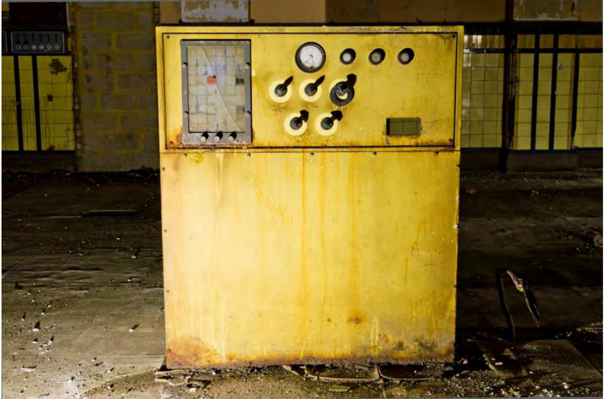
Plate 79: Control Room control panel (#RER16-0125)
