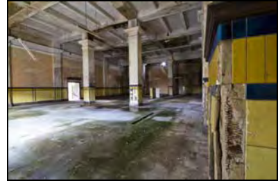
RER16-0240 Control Room F15 - Overview. Facing north-east
