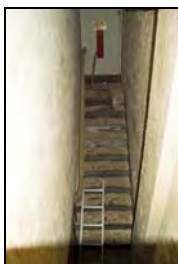
RER16-0145 Blocked stair. Facing west
