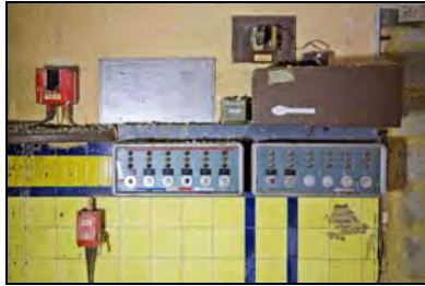
RER16-0242 Control Room F15 - Control Panels. Facing south
