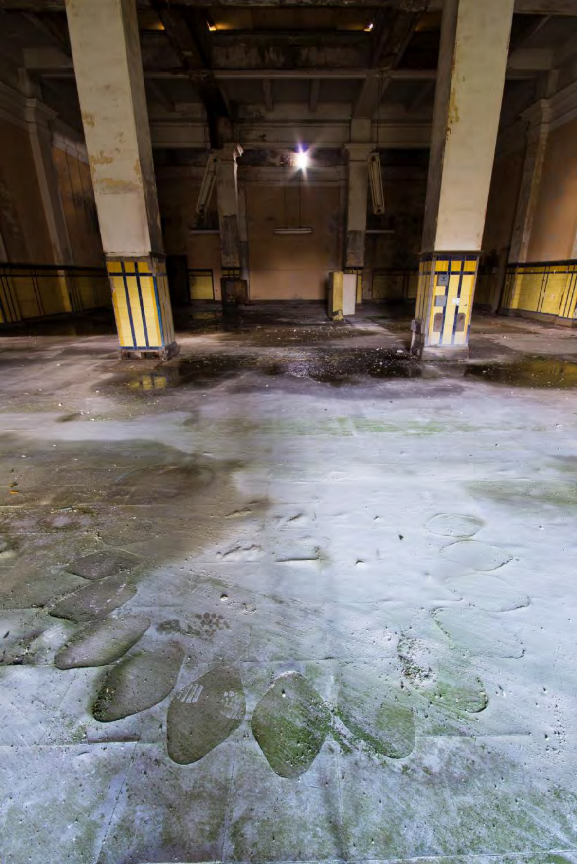
Plate 81: Extant impressions left from the removed governor control pedestals and telephone pedestals within the Control Room (#RER16-0246)
