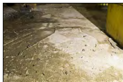
RER16-0132 Control Room F15 - Plant impression. Facing east
