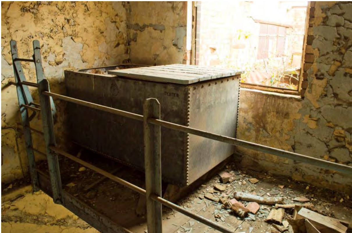
Plate 48: Water tank and platform at the top of the secondary stair (#RER16-0182)
