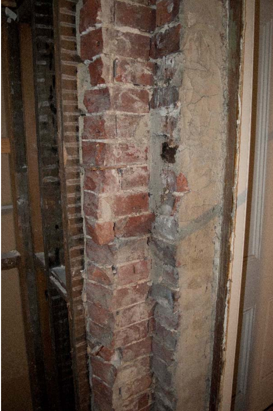
Plate A3.3: Truncated brick wall, which replaced a stud partition beneath the Phase-1 girder. Attached to the right-hand side is part of a brick wall which separated the kitchen from the passageway to the south (RLB-0096)
