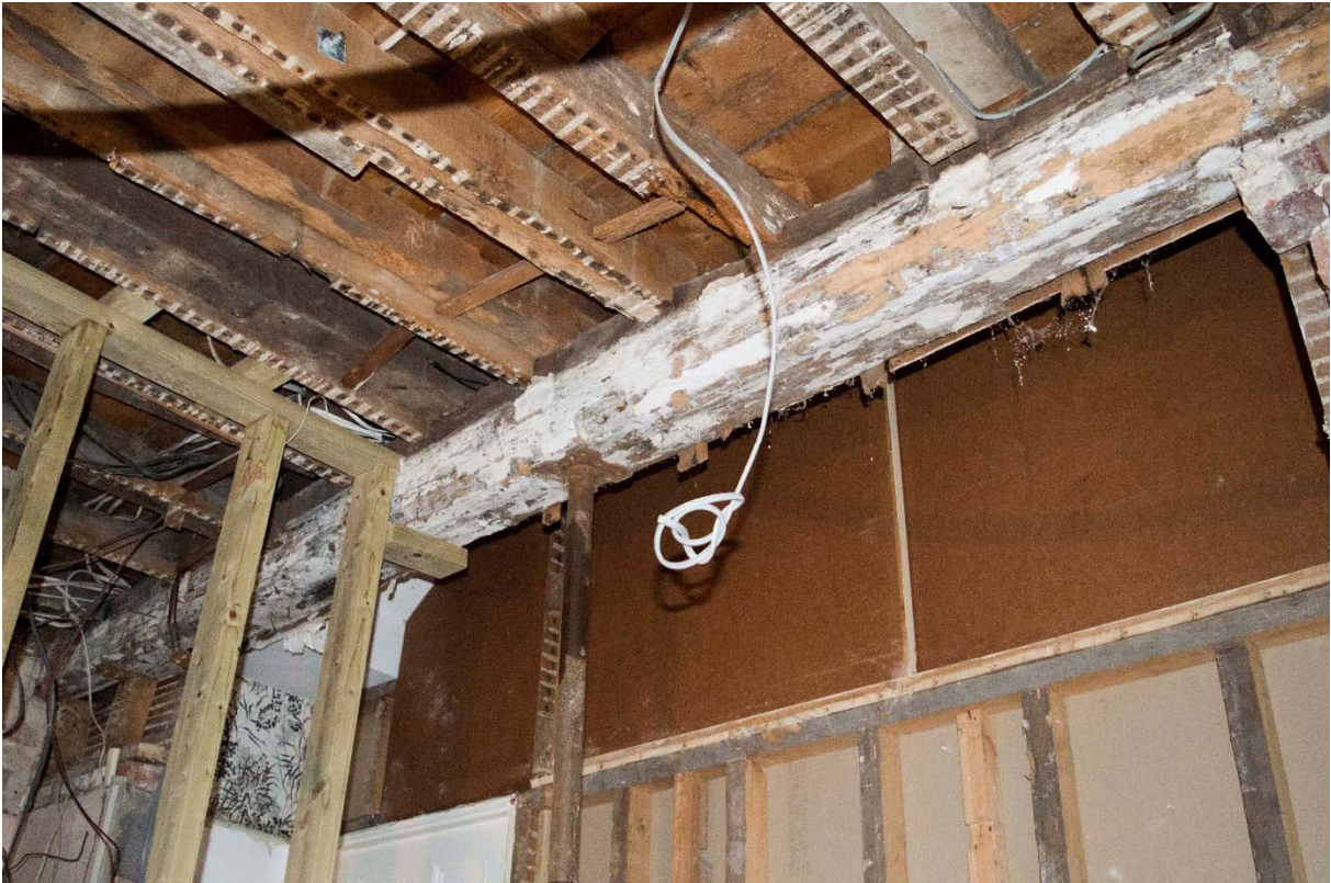
Plate A3.1: Phase-1 chamfered ceiling girder. Note the redundant joist mortises in the face of the girder where the joists have been raised. (RLB-0085)
