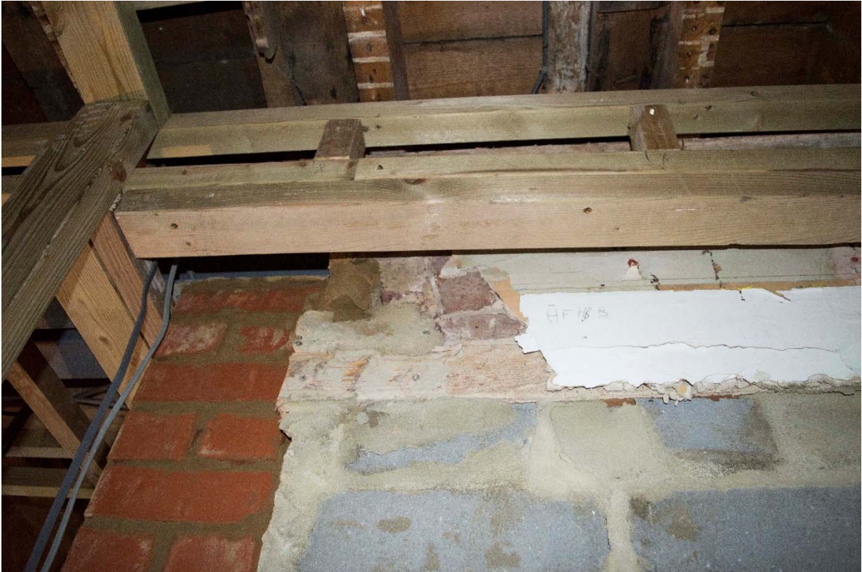
Plate A3.7: Partially visible brick arched head to former pantry doorway on western side of kitchen (RLB-0094)
