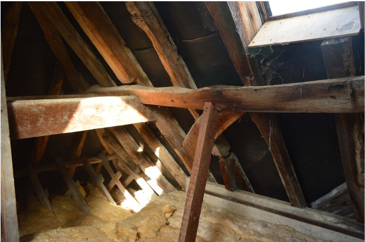
Plate 2: Junction of purlin, collar, principal rafter and windbrace of Truss 3, facing north-west (RLB17-0004)
