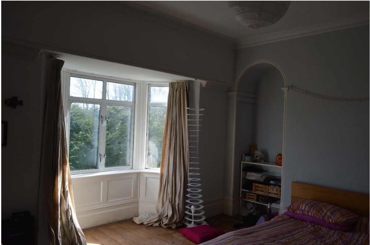
Plate 17: Interior of first floor north-west room with late 17 th or 18 th century moulded cornice, facing south-east (RLB17-0051)
