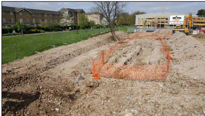
View north-west showing Trench 2 and the adjacent groundworks area. The concrete beams for Eagle Wharf are displayed quite prominently.
