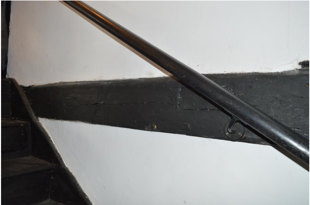
Plate 3: Redundant mortices on hall side of low end cross-beam, facing west (BES-0008)
