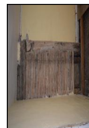
BES17-0090 Blocked door, post and truncated wall plate in 1F NW room. Facing west
