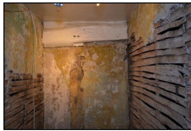
BES17-0077 Shutter groove on wall plate above stairs. Facing east
