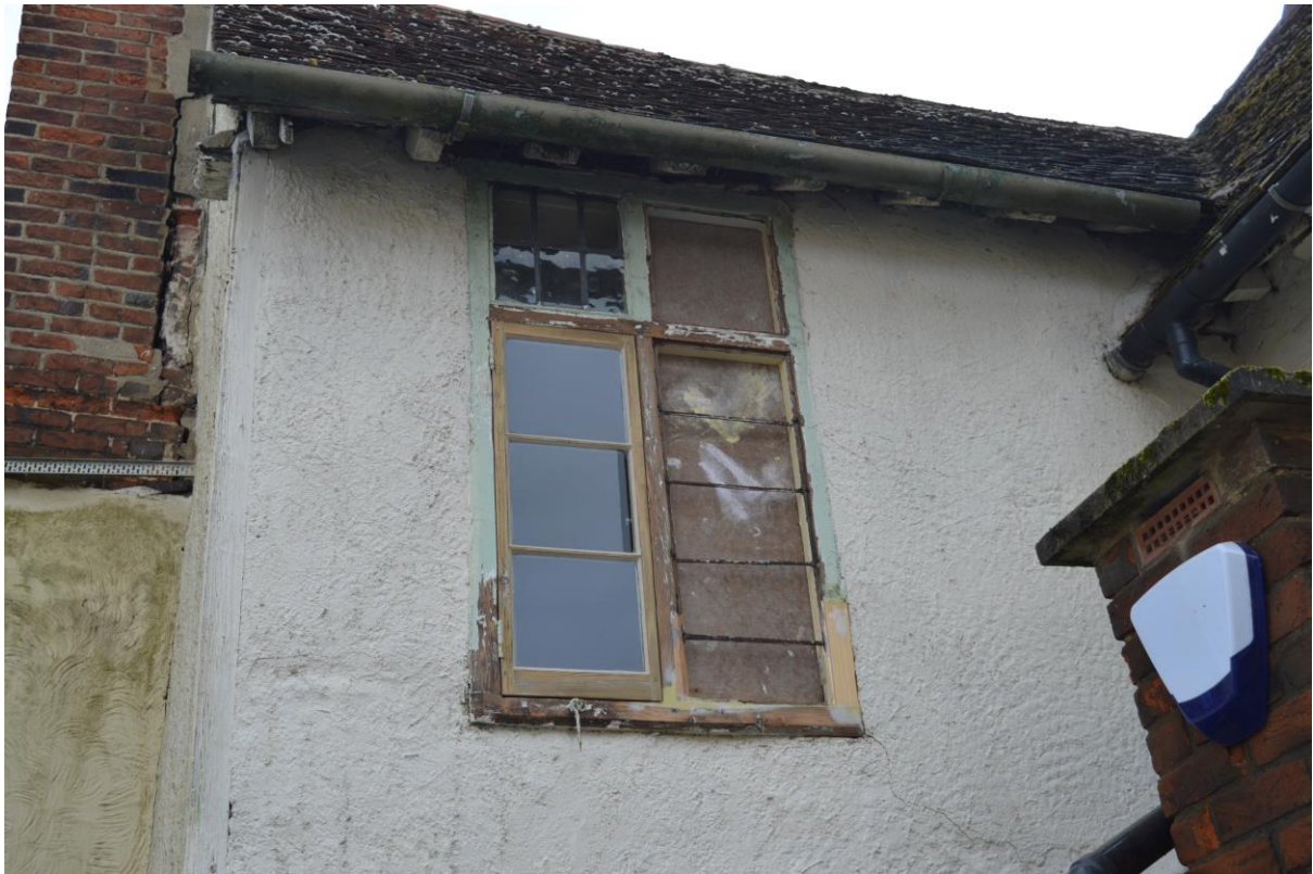
Plate 14: Cross type window on west wall of rear wing, facing east (BES-0027)
