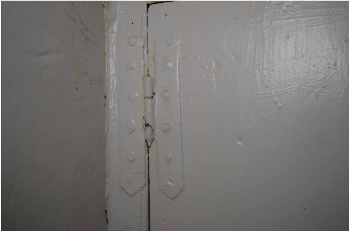
Plate 16: H-hinge on plank and batten door in first floor room, facing west (BES-0082)
