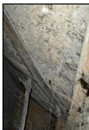
BES17-0115 Void under attic stairs. Facing west
