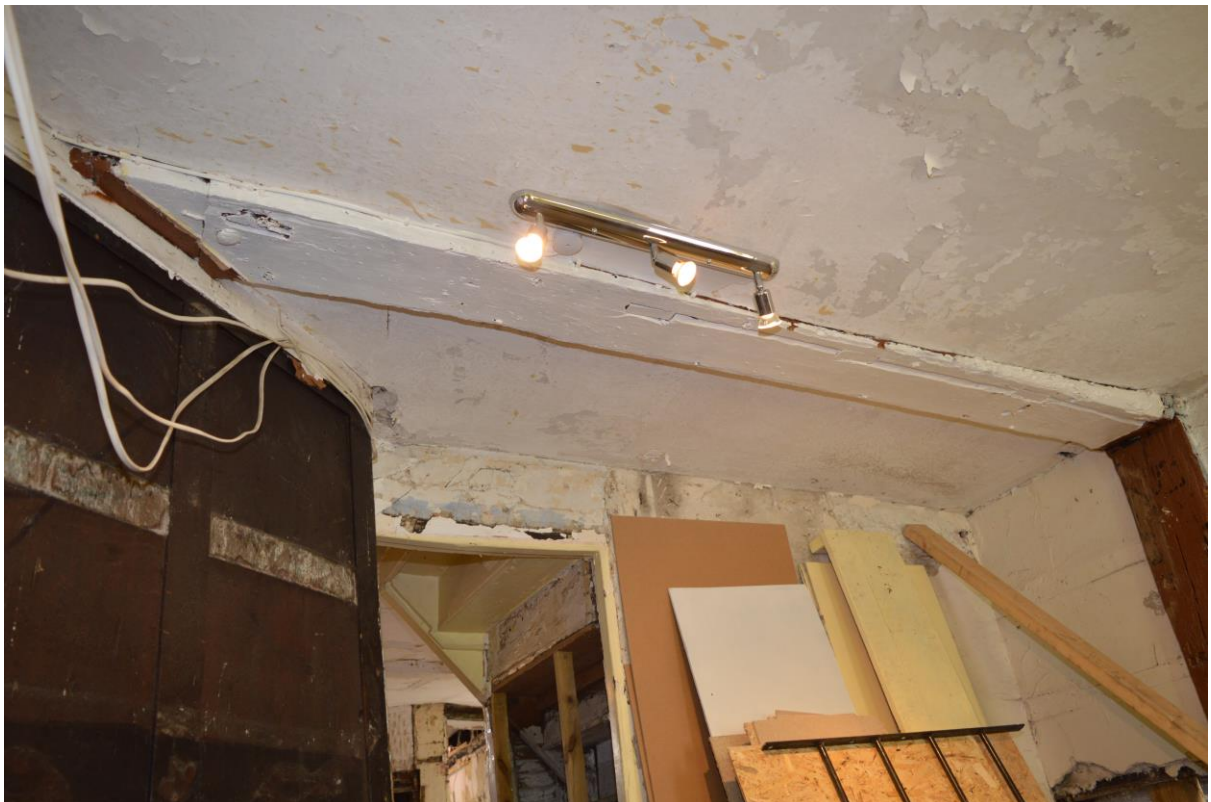
Plate 4: Bridging joist in high end bay with evidence of partition and doorway, facing north (BES-0050)
