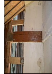
BES17-0051 Bridging joist and post in ground floor south room. Facing east
