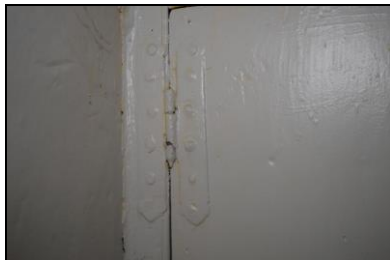
BES17-0082 H hinge on cupboard door in 1F south room. Facing west
