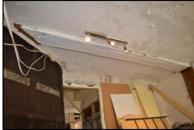
BES17-0050 Bridging joist in ground floor south room with evidence of partition and door. Facing north
