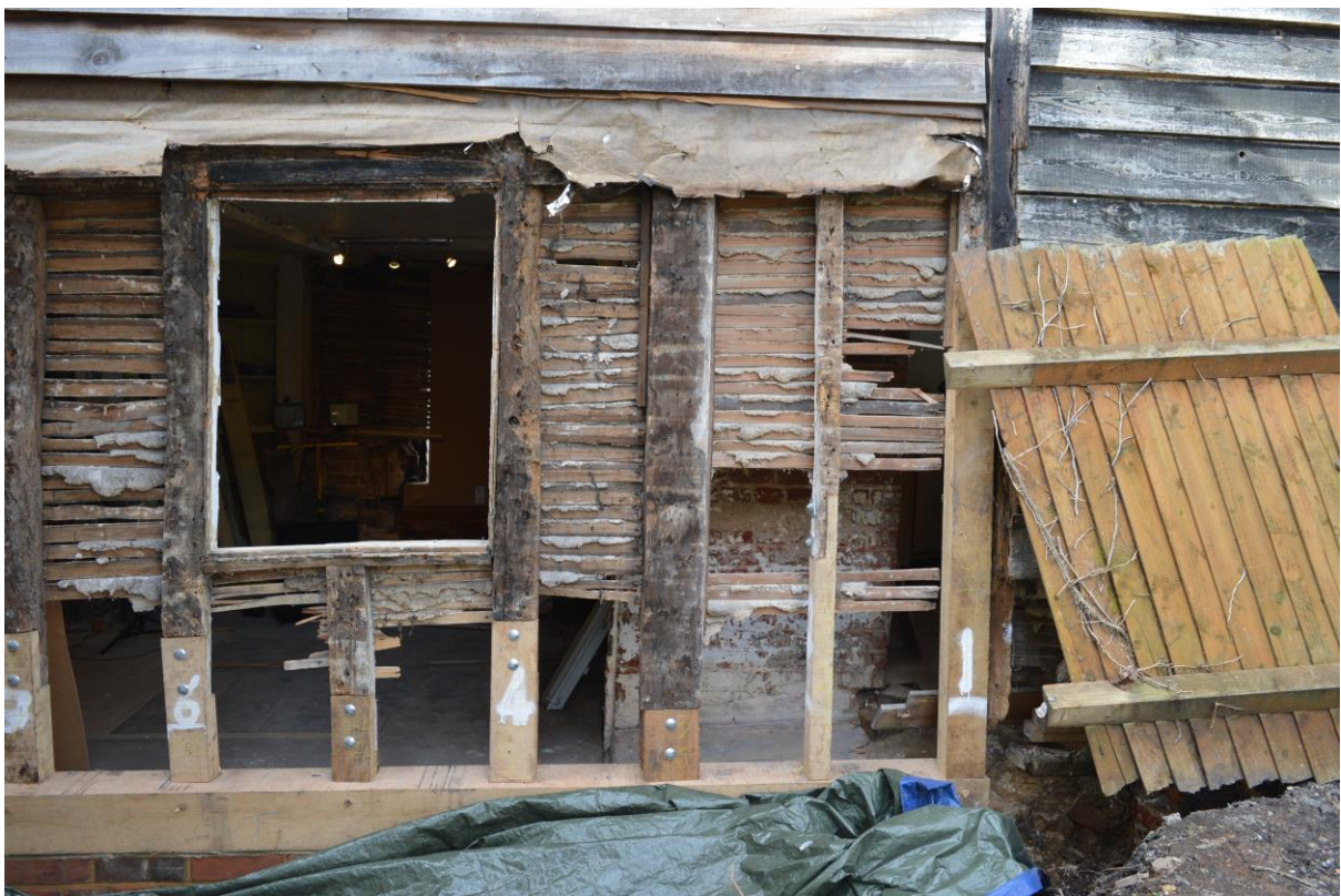
Plate 11: Phase 2 wall framing on east wall and inserted window, facing west (BES-0036)
