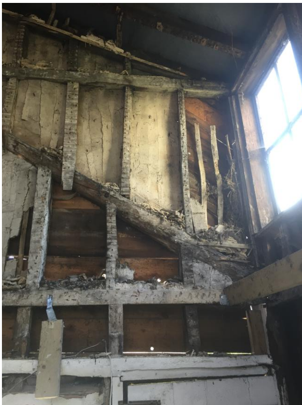
Plate 23: Phase 3 extension, original principal rafter preserved in heightened wall, facing west (BES-121)
