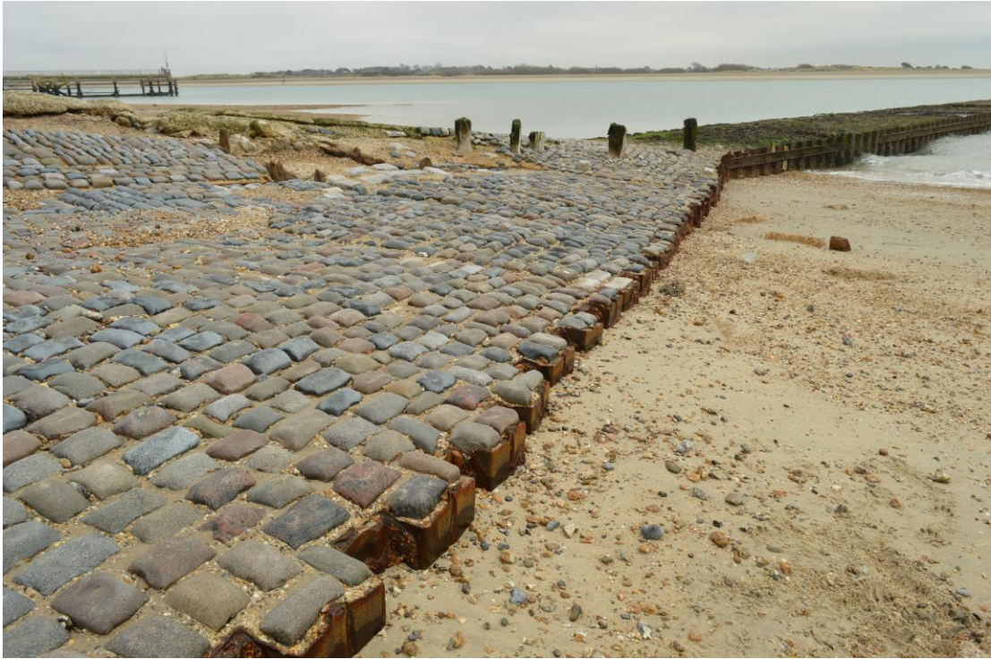
Plate 4: Stone setts and iron shuttering as part of the sewage outfall (looking north east)
