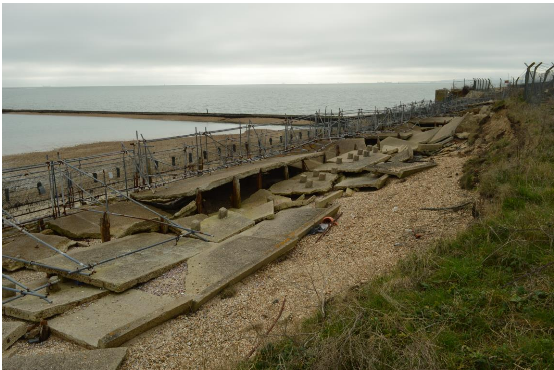
Plate 7: The damaged concrete revetment looking south east
