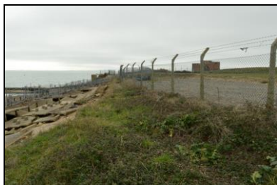
FCS17-0037 The damaged concrete revetments. Facing south-west
