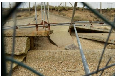
FCS17-0044 The damaged concrete revetments. Facing north-west
