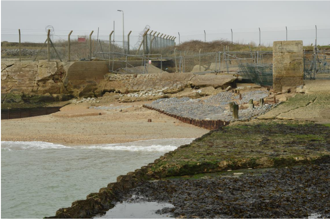
Plate 2: Detail of the concrete slabs and defences nearest the fort (looking south west)
