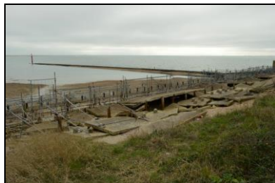
FCS17-0036 The damaged concrete revetments. Facing south
