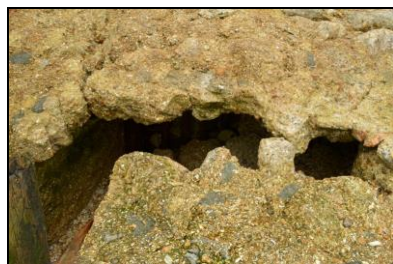
FCS17-0013 Voids in the concrete structures on the shore
