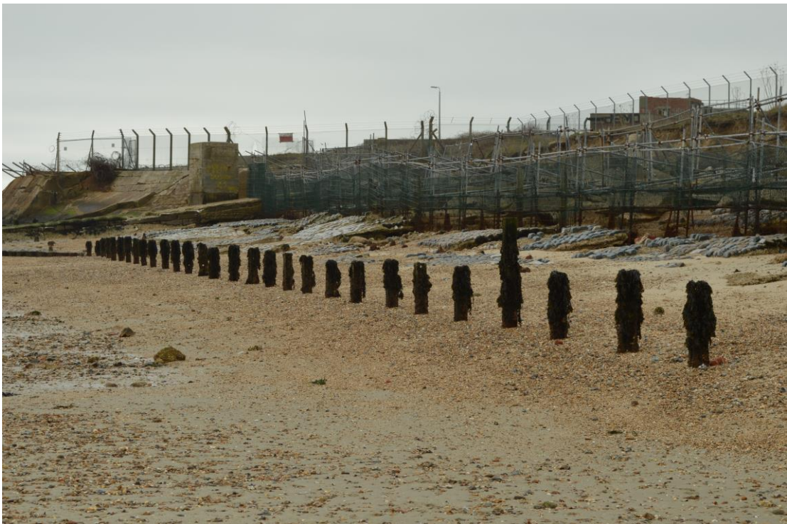
Plate 5: The iron I-posts with the fort in the background (looking south west)
