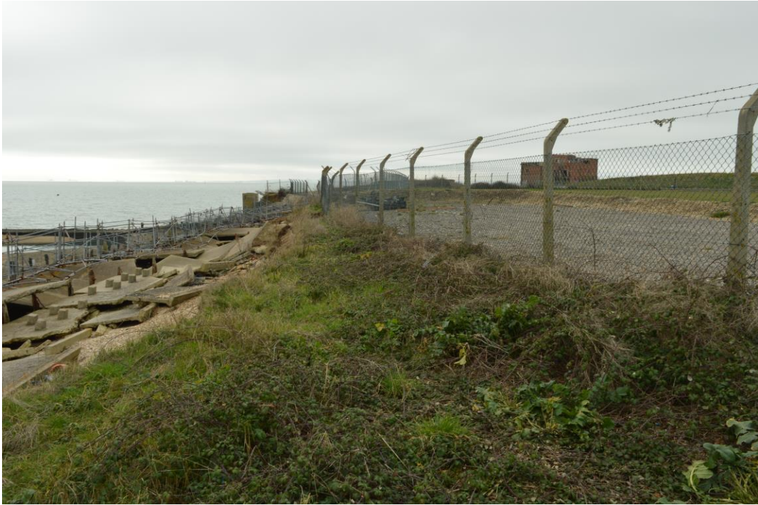
Plate 8: Showing the proximity of the damaged revetment to the fort (looking south west)
