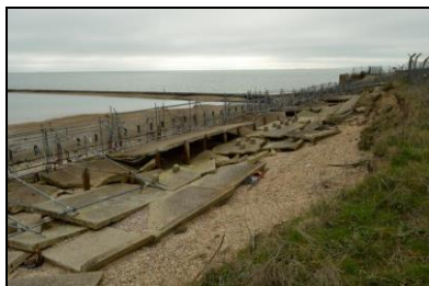
FCS17-0040 The damaged concrete revetments. Facing south
