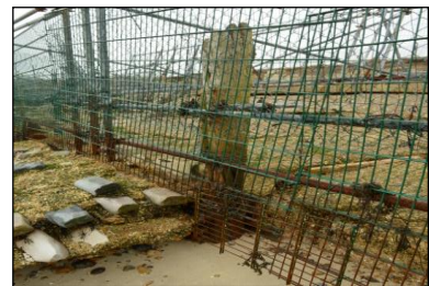
FCS17-0045 Post in the damaged concrete revetments. Facing west
