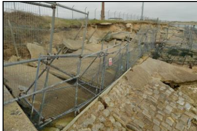
FCS17-0053 The damaged concrete revetments. Facing north-east
