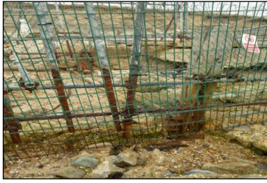
FCS17-0046 Post in the damaged concrete revetments. Facing north
