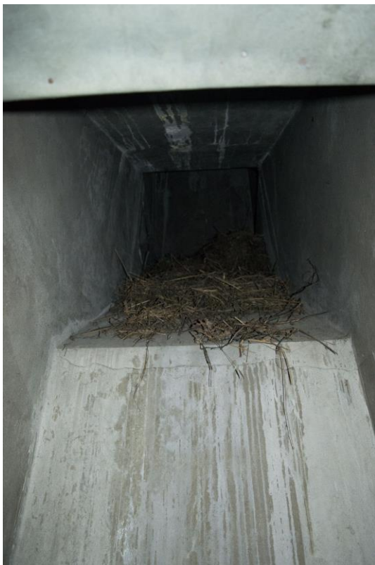
Plate 28: Interior of shaft, viewed from a hatch in the first floor south range cupboard (WOD17-0094)
