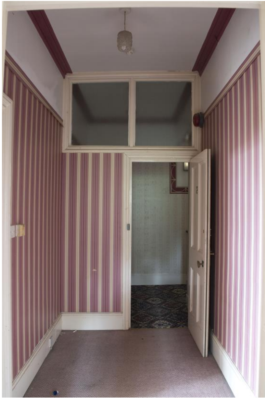
Plate 31: Small first floor rooms in north part of south range, facing west (WOD17-0084)
