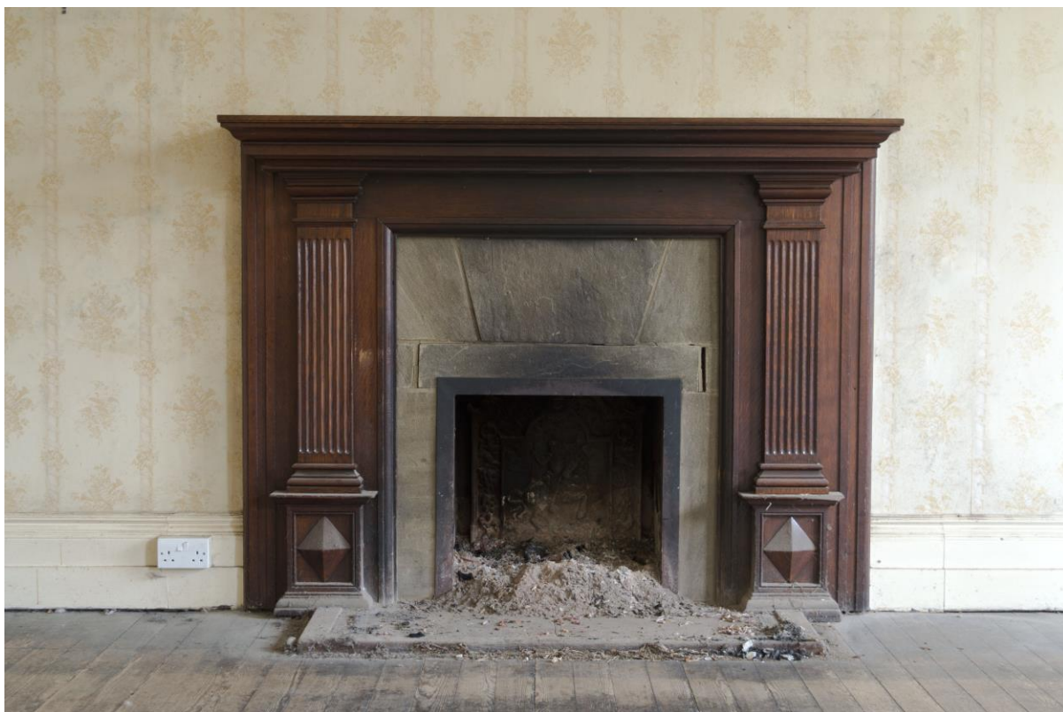
Plate 18: Fireplace in ground floor east room in south range of main building, facing east (WOD17-0047)
