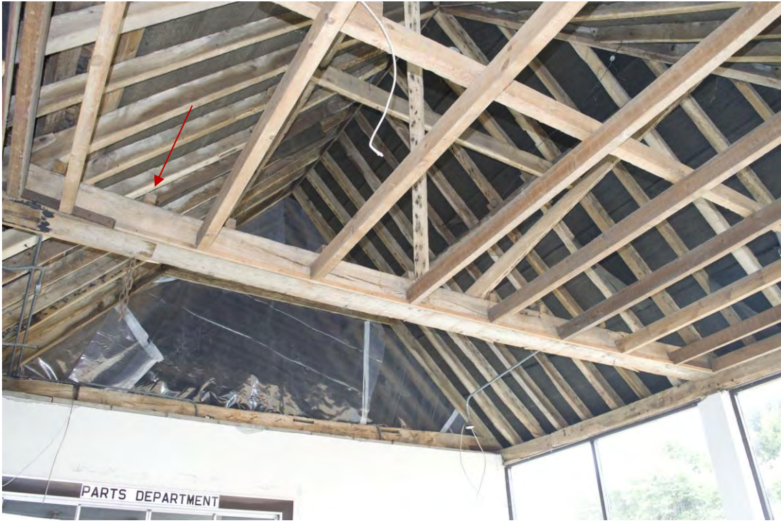
Plate 11 Detail of the retained floor joist sections above the tie-beam separating Bays 1 and 2 within Range 1, facing south-west (37)
