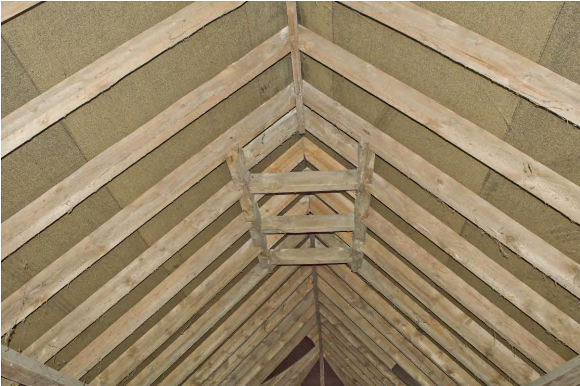
Plate 15 Detail of the central roof vent (now blocked) in Range 2, facing south (96)
