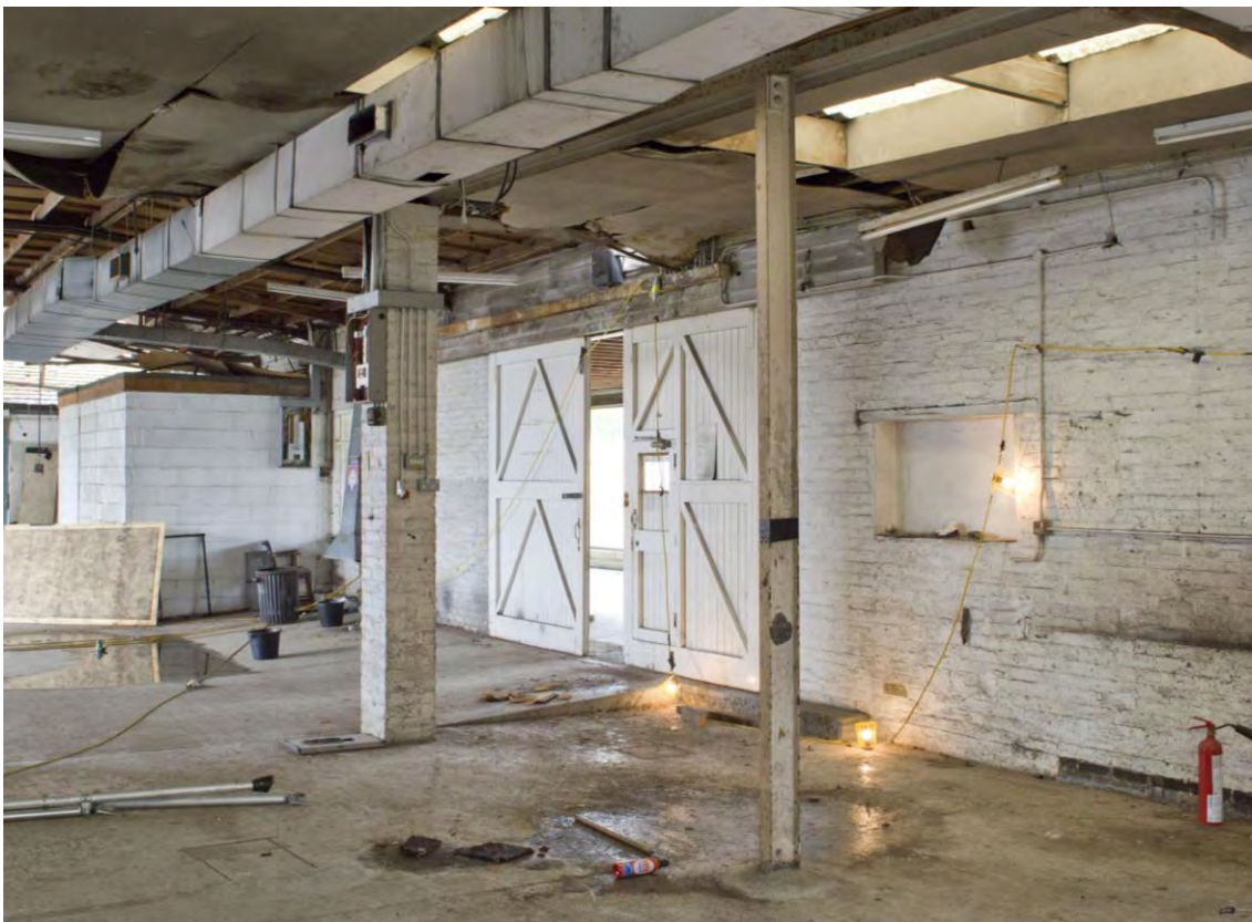
Plate 28 Detail of the sliding double doors providing access between the northern and southern halves of Range 3, facing north-east (54)
