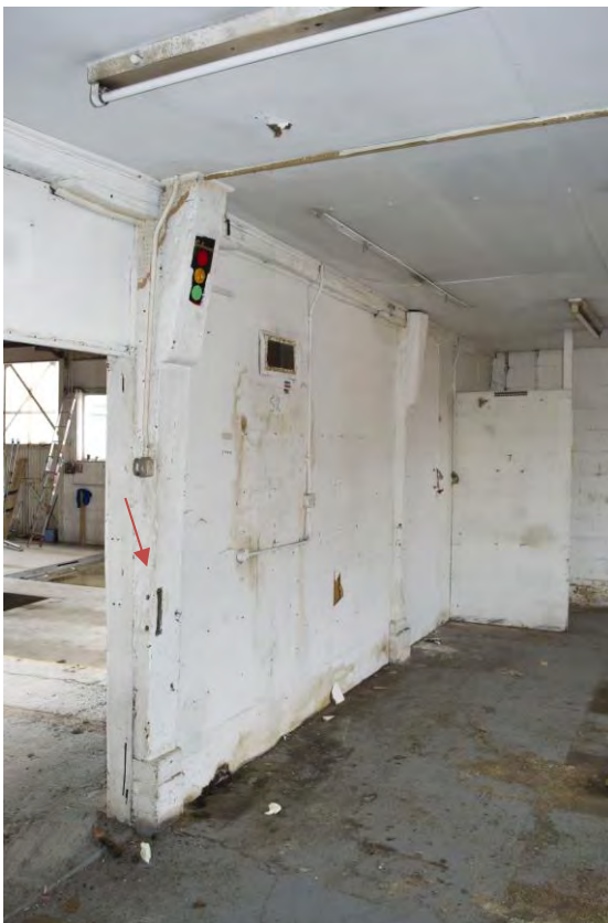
Plate 6 Detail of the posts within the east elevation of Range 1, note the redundant mortices for partitions, facing south-east (28)
