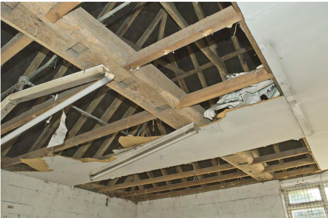
Plate 10 Detail of the redundant mortices within the southernmost tie beams within Range 1, facing south-west (78)
