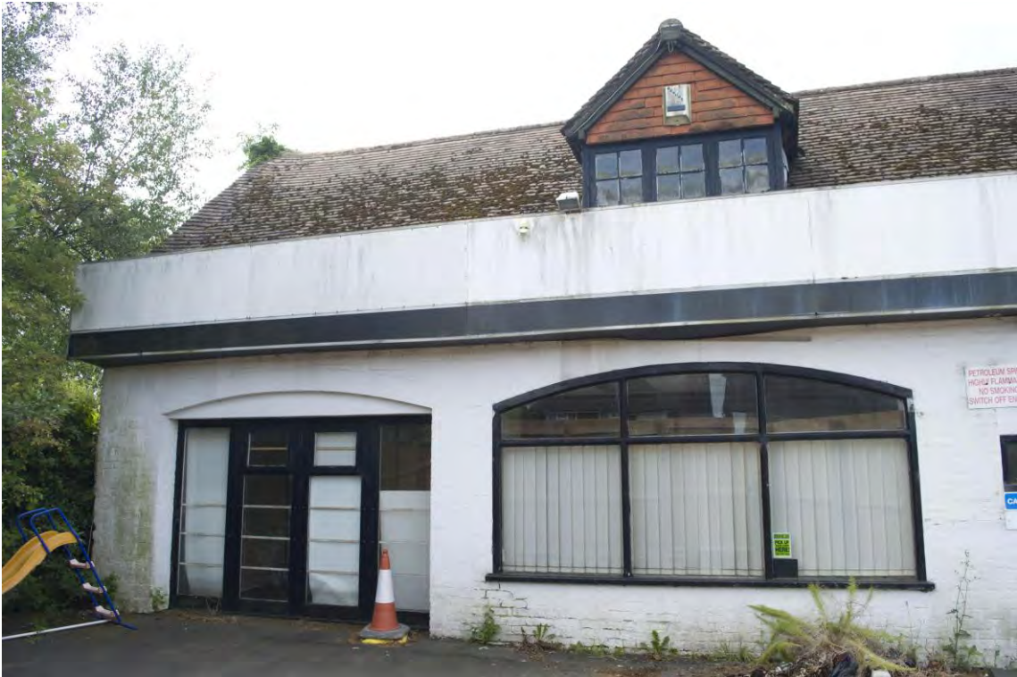
Plate 19 Detail of the original arched openings within the east end of the north elevation of Range 3, facing south (11)
