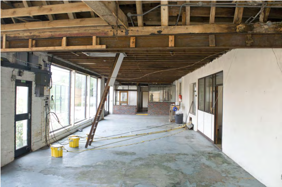
Plate 21 Interior ground floor view of the northern half of Range 3, facing east (59)
