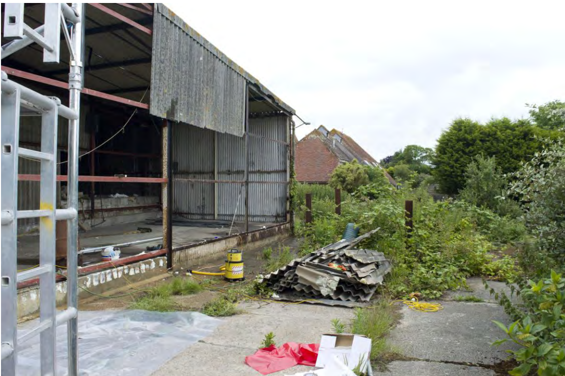
Plate 34 Concrete hardstanding and steel uprights found within the formerly developed south-east corner of the site, facing east (64)
