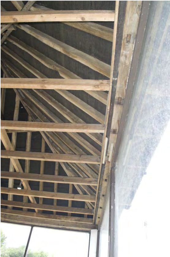
Plate 7 Detail of the redundant mortices within the wall-plate framing the north elevation of Range 1, facing west (40)
