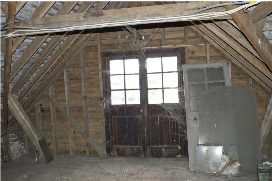
Plate 24 Detail of the central loading door within the attic above the northern half of Range 3, facing north (71)
