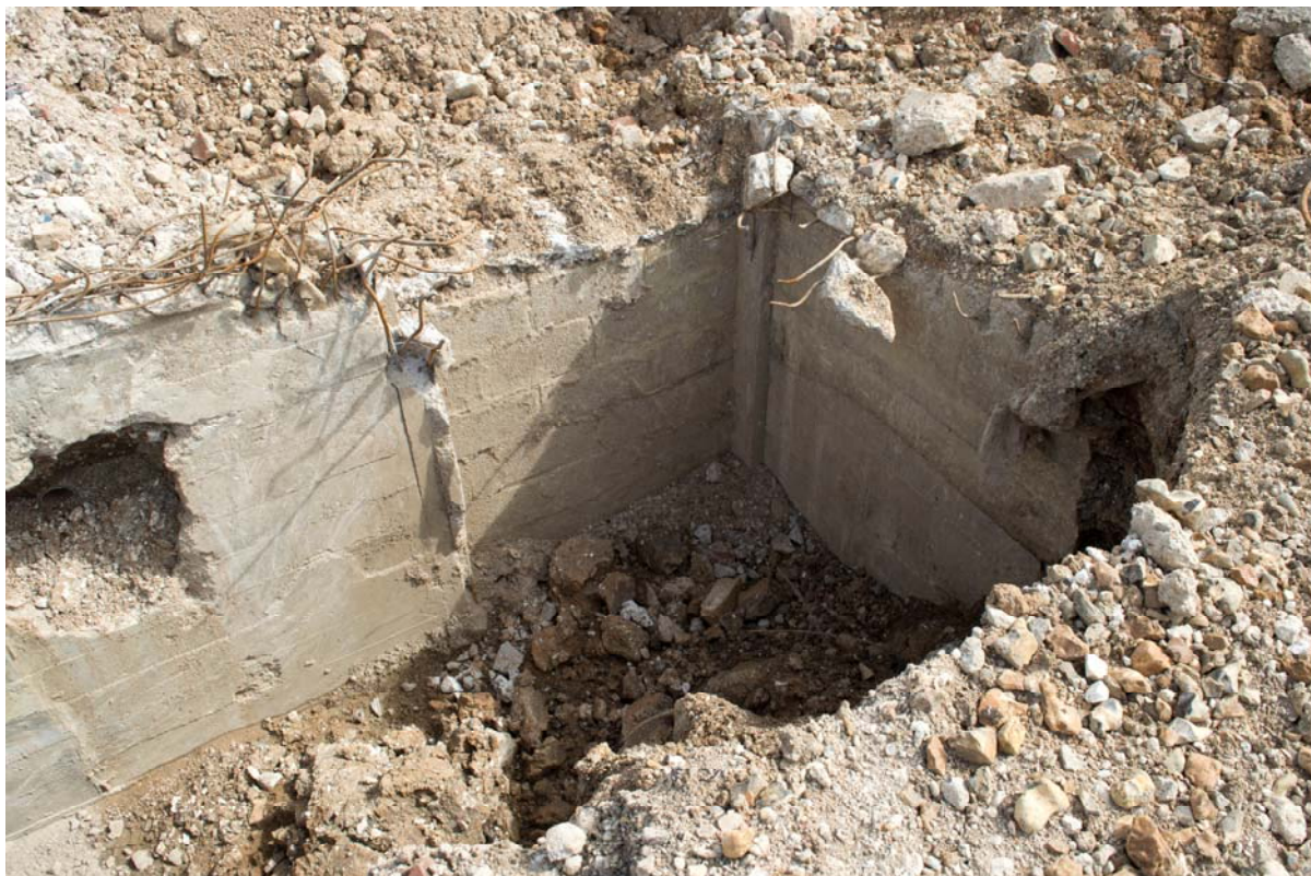
Plate 3: Blocked opening at north east corner of ARP shelter, facing north (RSP17-0007)
