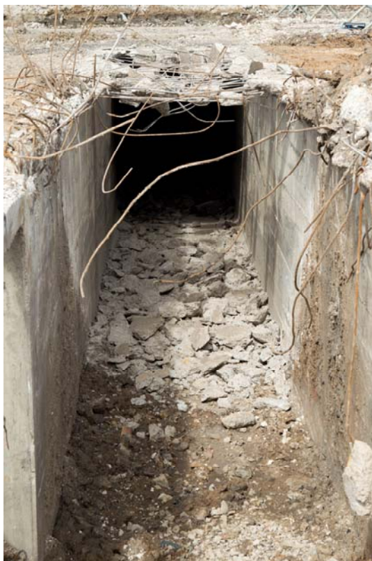
Plate 2: North trench of ARP shelter, showing construction of the structure, facing west (RSP17-0012)
