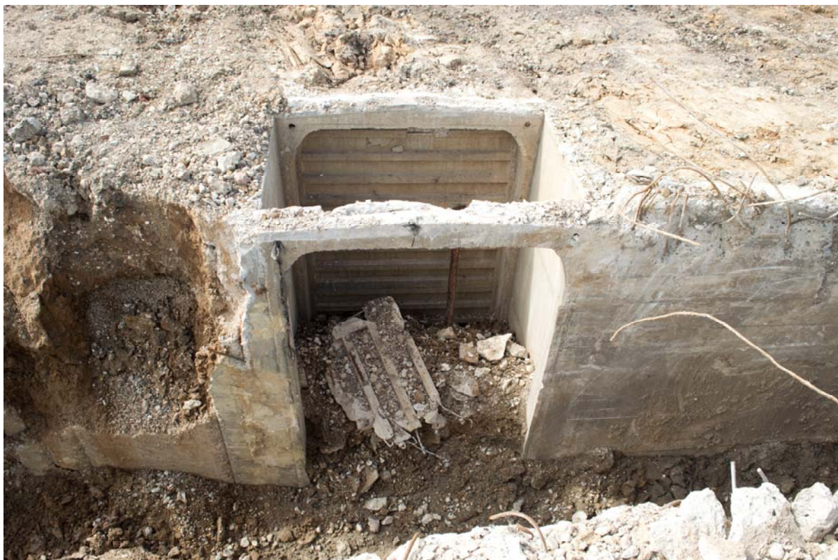
Plate 4: Blocked opening on south side of north trench with precast door frames, facing south (RSP17-0007)
