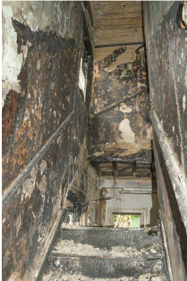
Plate 14 – Fire damaged interior of no.15 (HR117- 0104)
