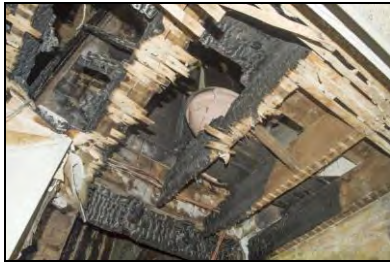
HR117-0091 Ceiling of room 3 showing fire damage
