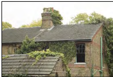
HRI17-0011 Detail of the roof from the rear of the building. Facing east
