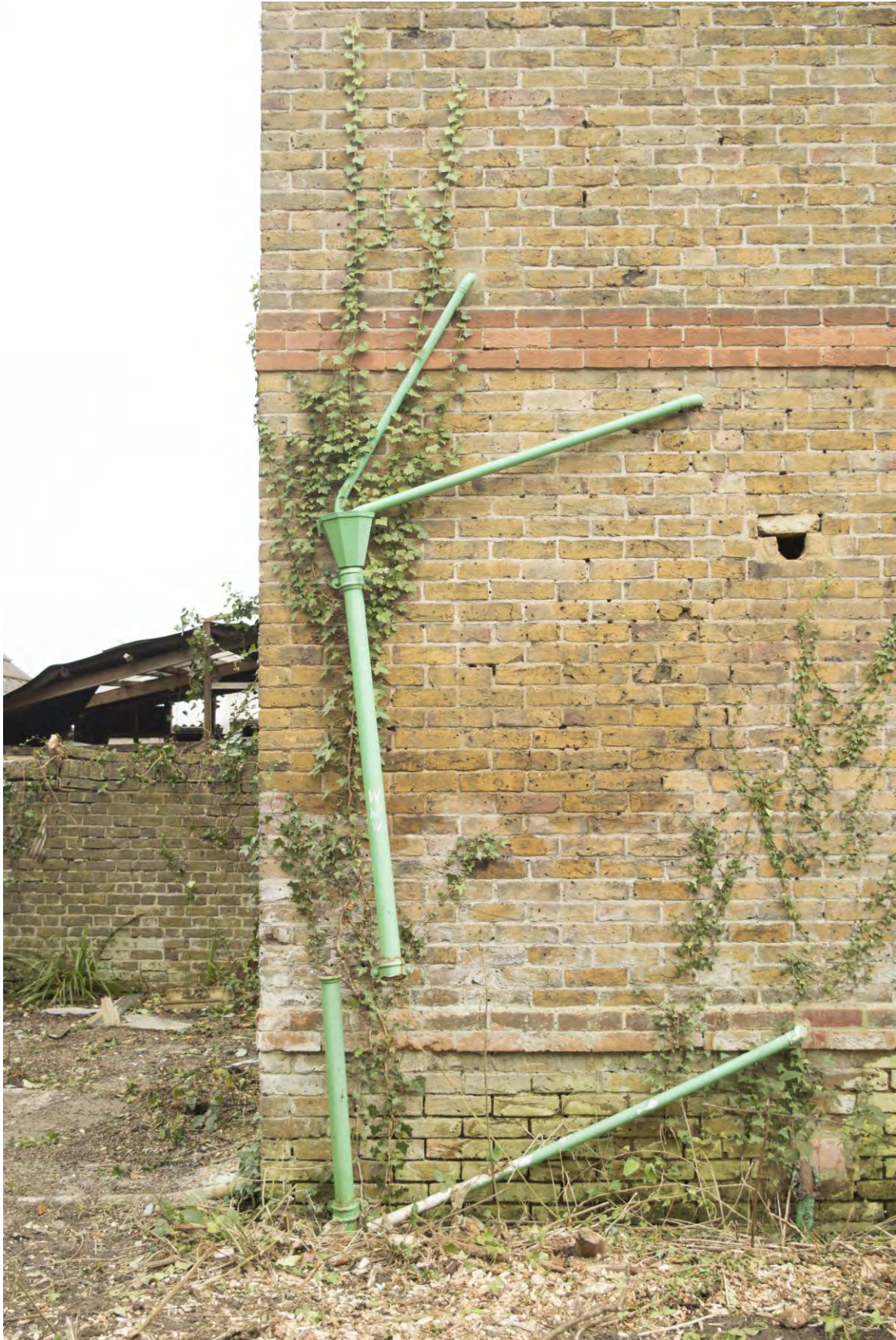
Plate 7 – Some of the external piping added to the building (HRI17-0015)
