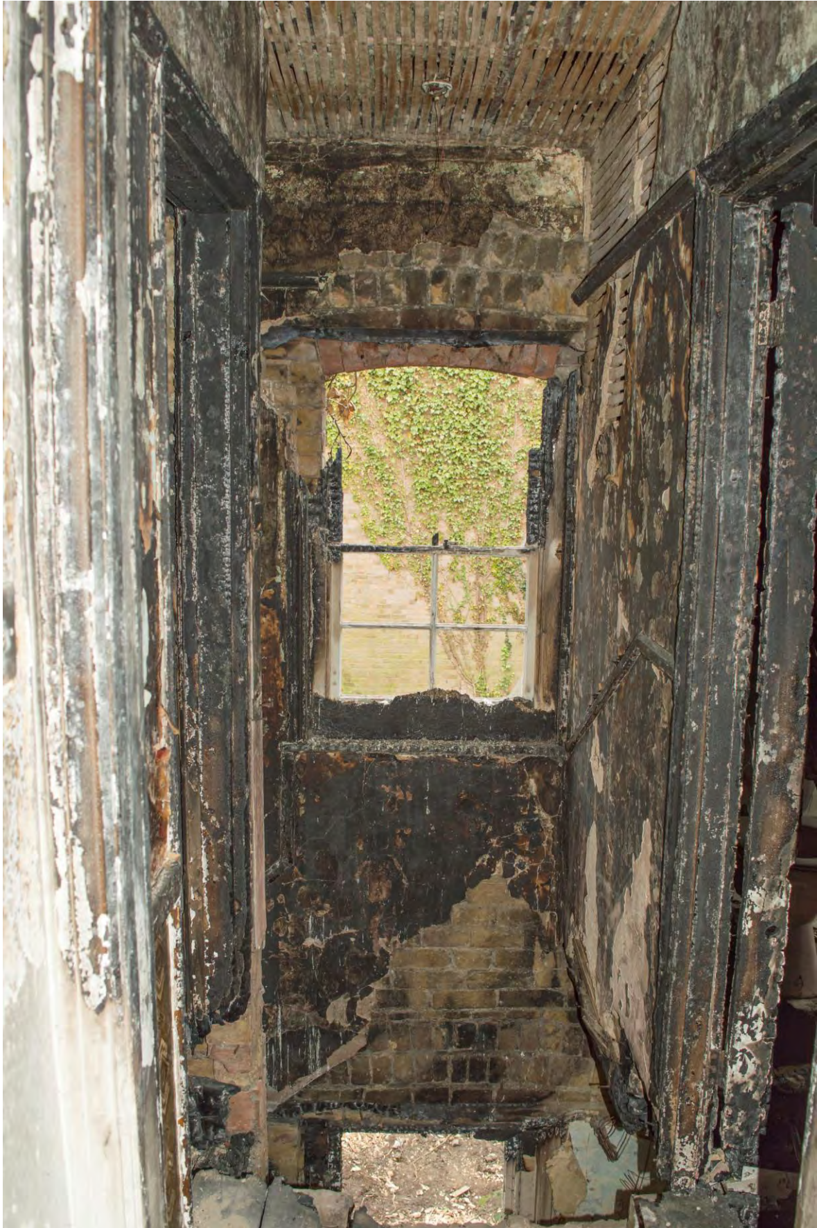
Plate 23 – Fire damage in no.15 revealed the construction methods used (HR117-0080)
