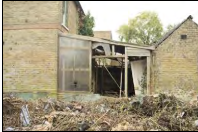
HR117-0034 NE elevation of the lean too structure at the rear of n. 17. Facing south-west
