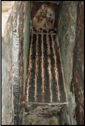
HR117-0094 Fire damage in room 3?
