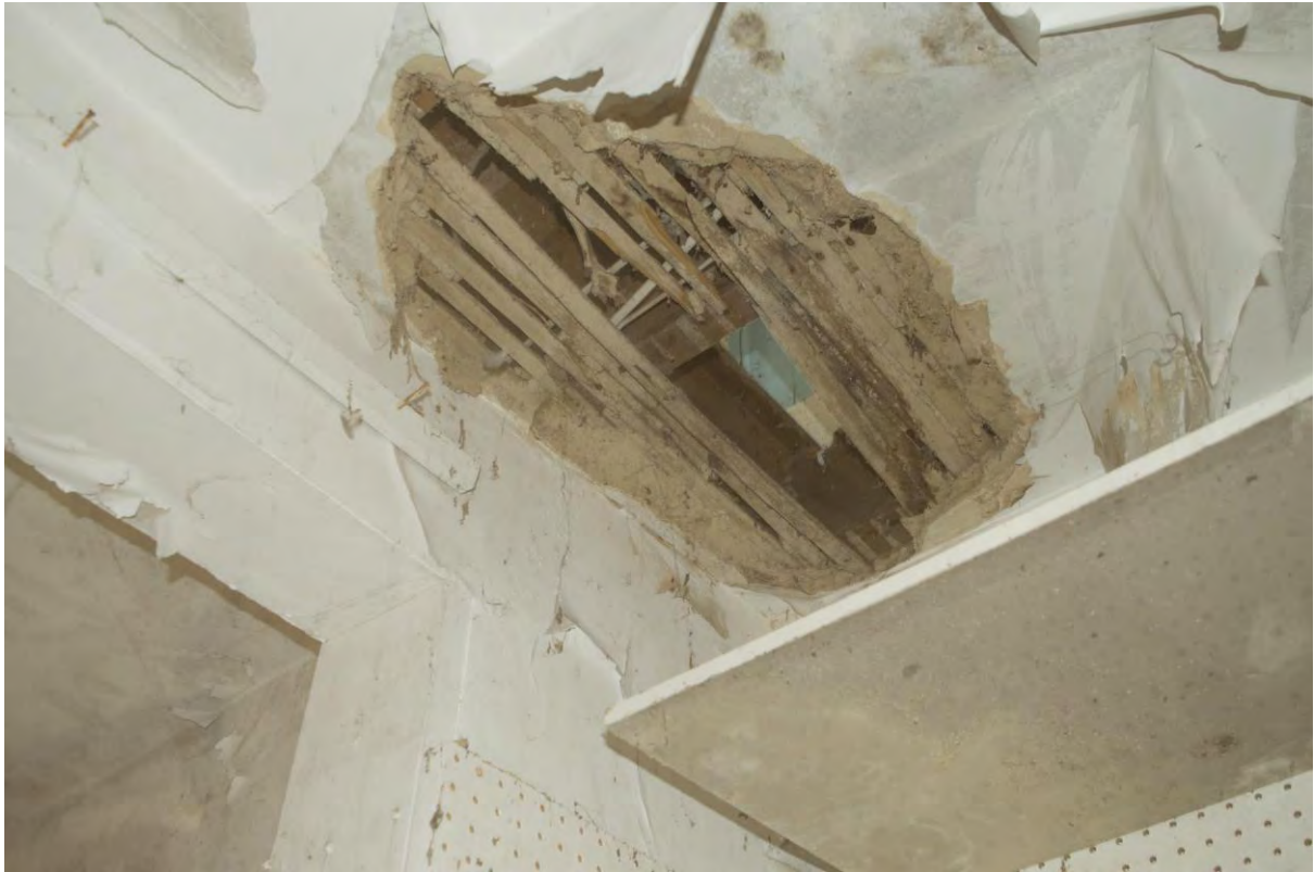
Plate 41 – Ceiling construction revealed by damage, (room 9), no. 17 (HR117- 0054)
