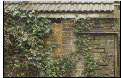
HRI17-0009 Detail of the outbuilding NW elevation showing blocked window. Facing south-east
