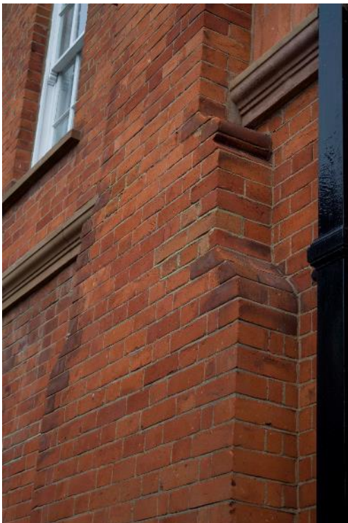
Plate 6: Station, Range 1, chimneystack and string course detail on the south-east elevation, facing north-west (170859_0049)
