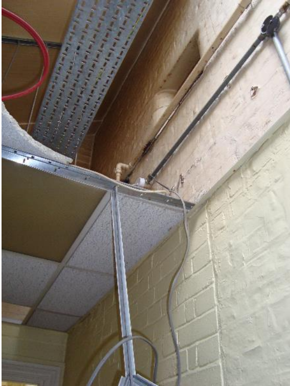
Plate 47: Station, Range 2, Room 19, air vent above Room 20 visible above the modern ceiling within the south-east wall, facing north-east (CgMs_0255)
