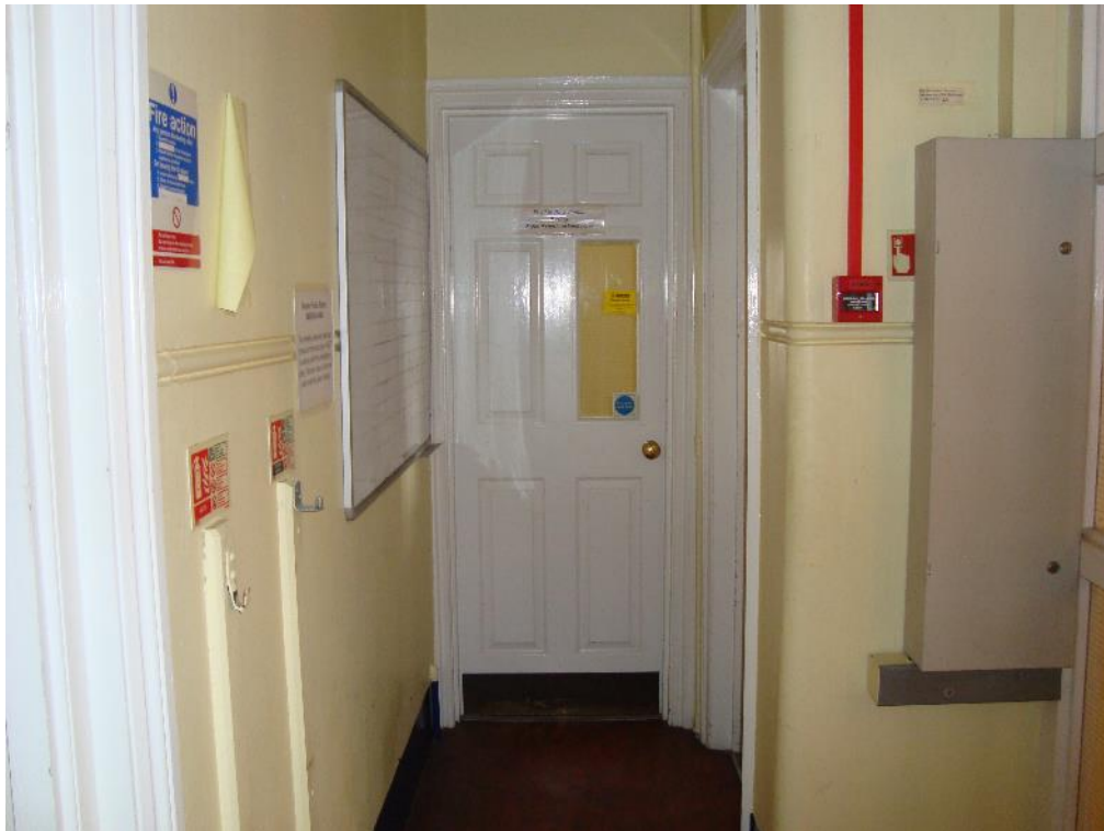
Plate 30: Station, Range 1, Room 9, bull-nosed wall reveals within the landing, facing north-east (CgMs_0143)
