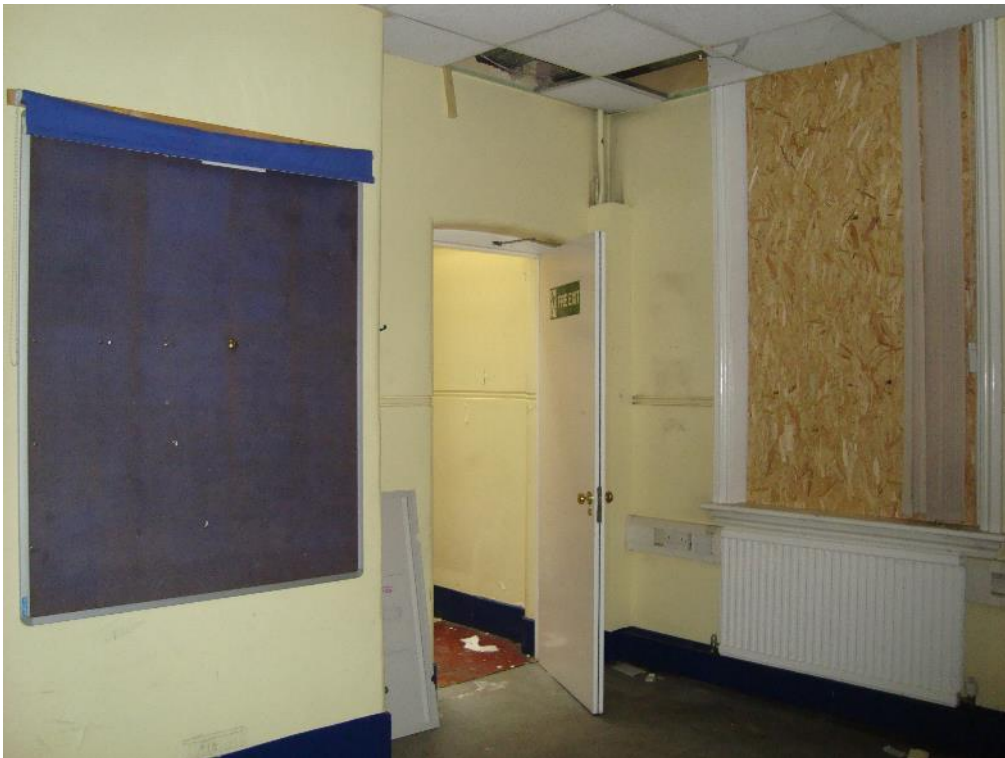
Plate 24: Station, Range 1, Room 5, note chimney stack and bull-nosing to the door jambs, facing west (CgMc_0104)
