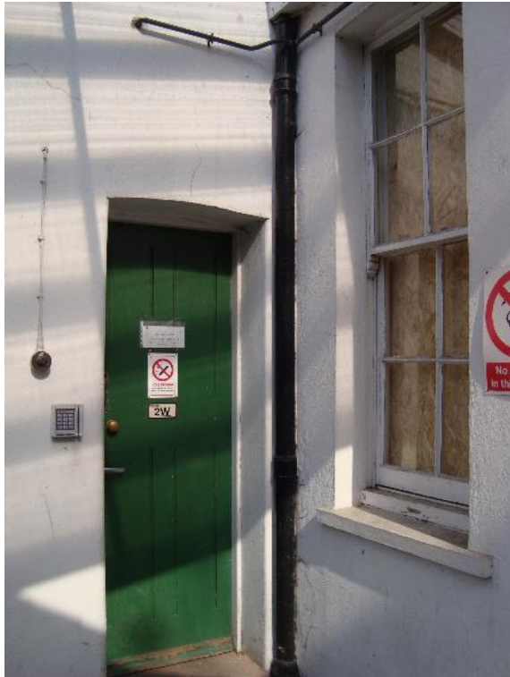
Plate 57: Station, Ranges 1 and 3, rendered finish to rear south-west elevation, facing north-east (CgMs_0172)
