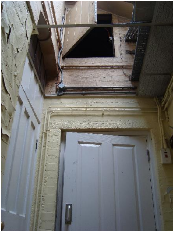
Plate 48: Station, Range 2, Room 19, doorway detailing at the south-west end of the corridor, facing south (CgMs_0249)
