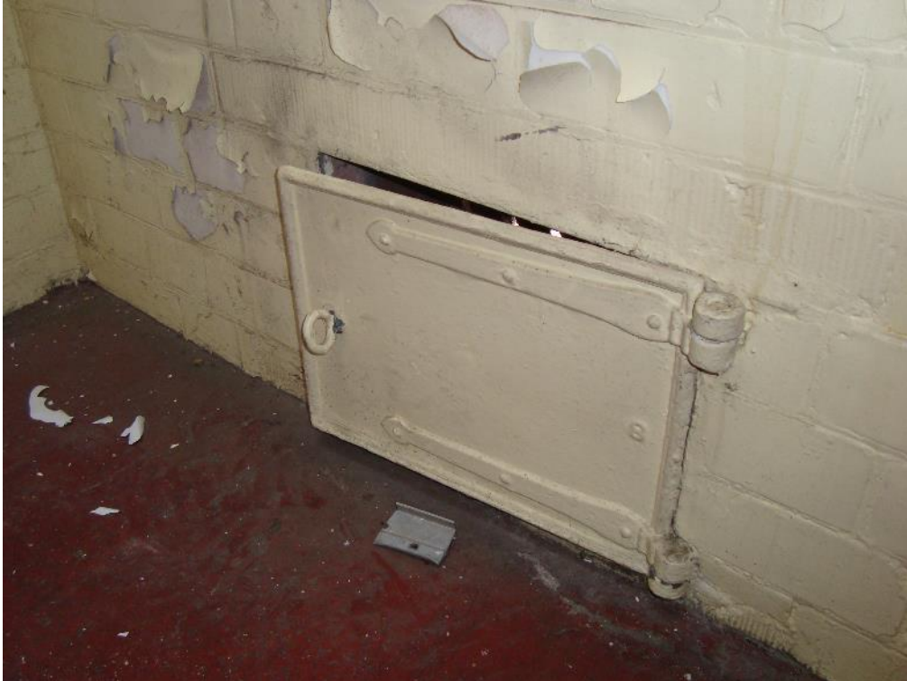
Plate 49: Station, Range 2, Room 19, ventilation grille hatch within the north-west wall, facing west (CgMs_0250)
