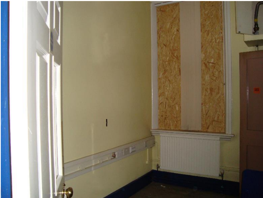
Plate 20: Station, Range 1, Room 3 interior noting inserted partition wall (left), facing west (CgMs_0107)
