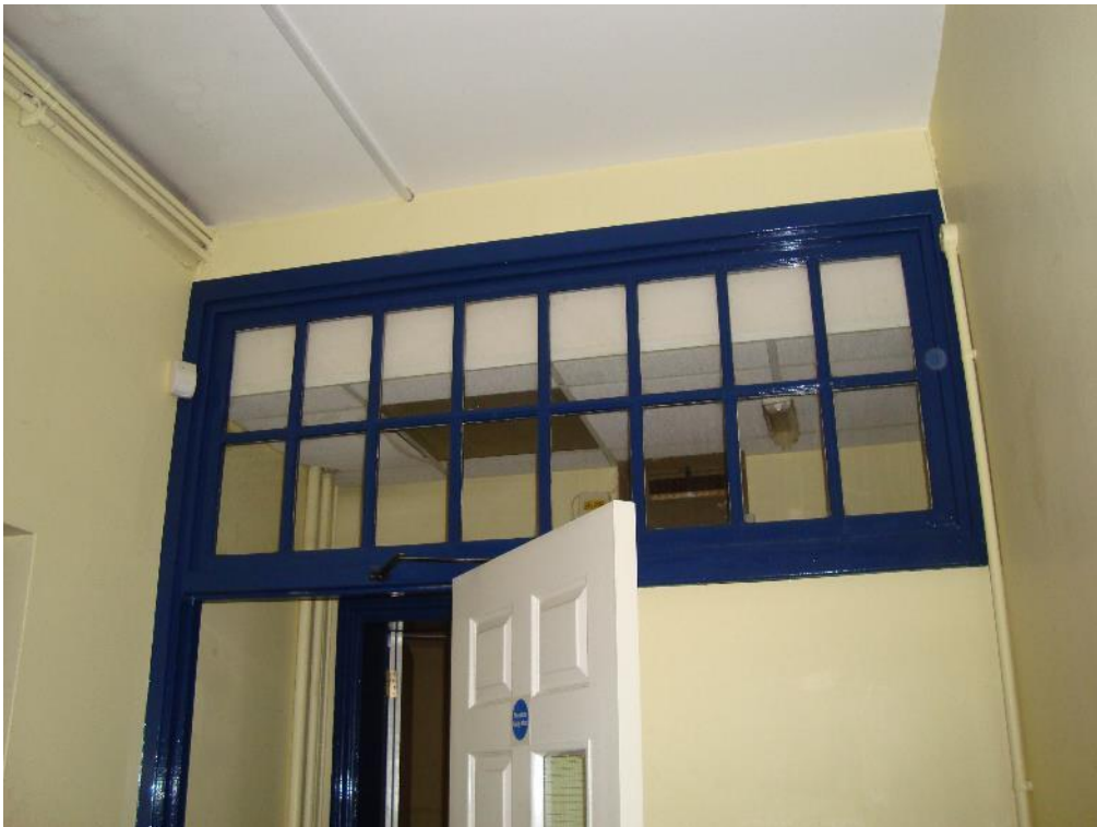
Plate 22: Station, Range 1, Room 3, detail of glazed partition separating the room from the inserted corridor, facing south-east (CgMs_0109)
