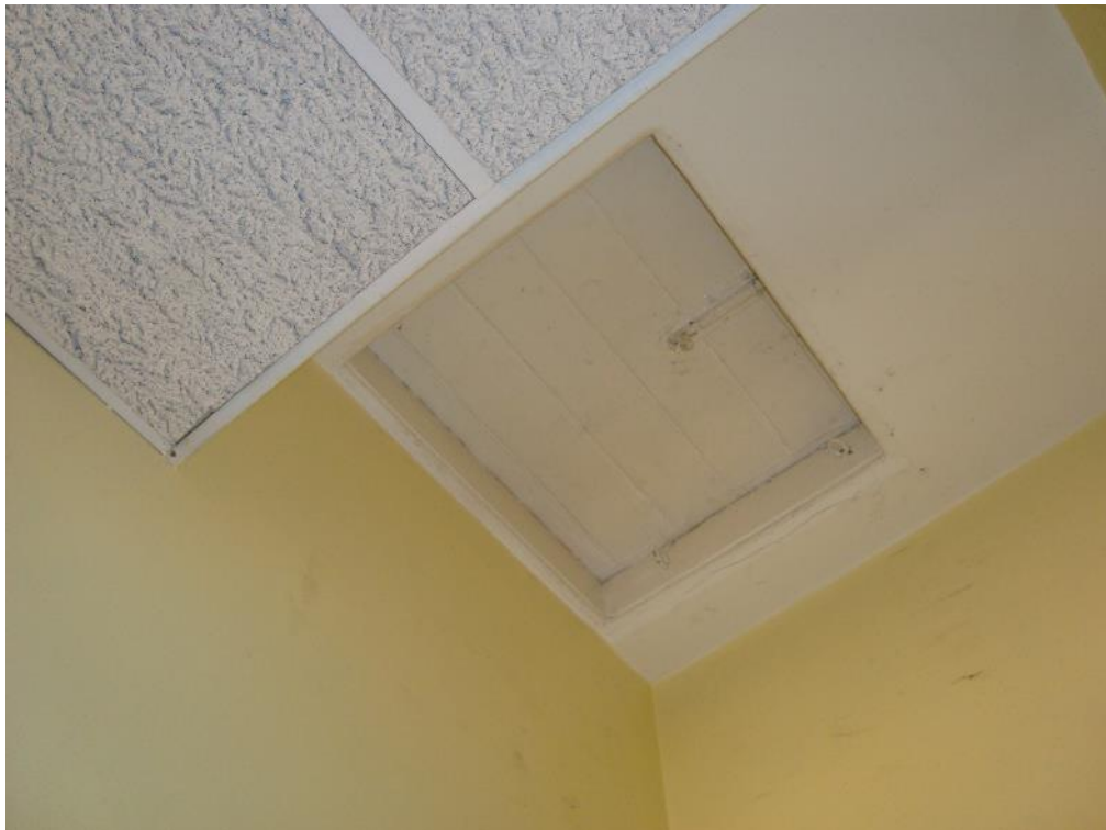
Plate 36: Station, Range 1, second floor level stairwell, roof hatch detail, facing north-west (CgMs_0163)
