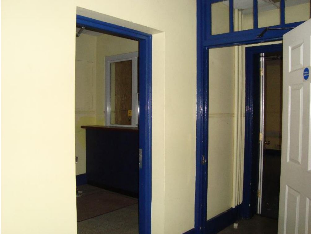
Plate 23: Station, Range 1, Room 4, corridor detail noting integral dado rail and door architraves, facing north-east (CgMs_0108)
