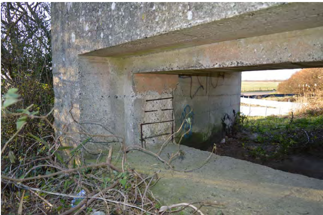
Plate 26: Structure 6, stepped embrasure, showing exposed steel reinforcing bars, looking south-east (0134)
