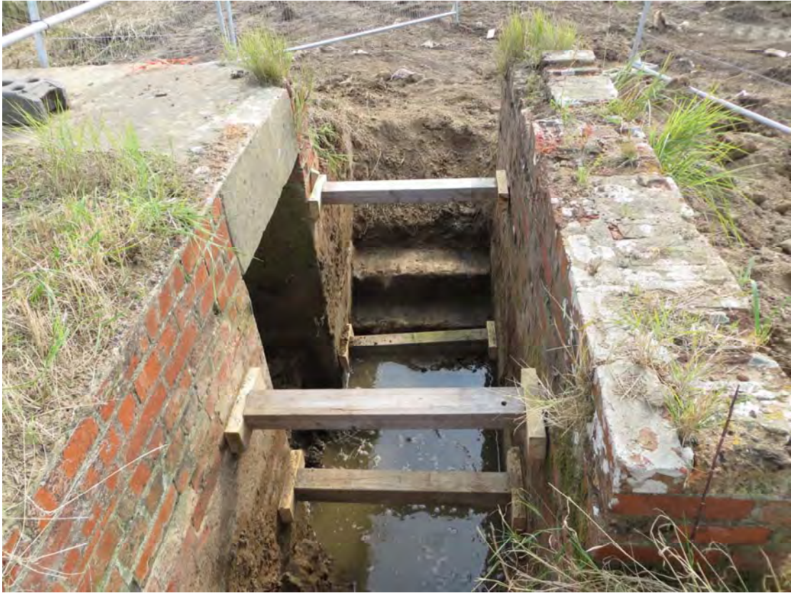
Plate 13: Structure 3, southern entrance, blast wall and steps, showing flooding, looking south (0045)
