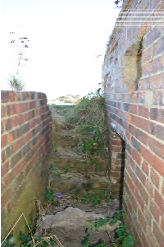
Plate 43: Structure 9, blast wall, access steps, entrance and loophole over entrance, looking east (0199)
