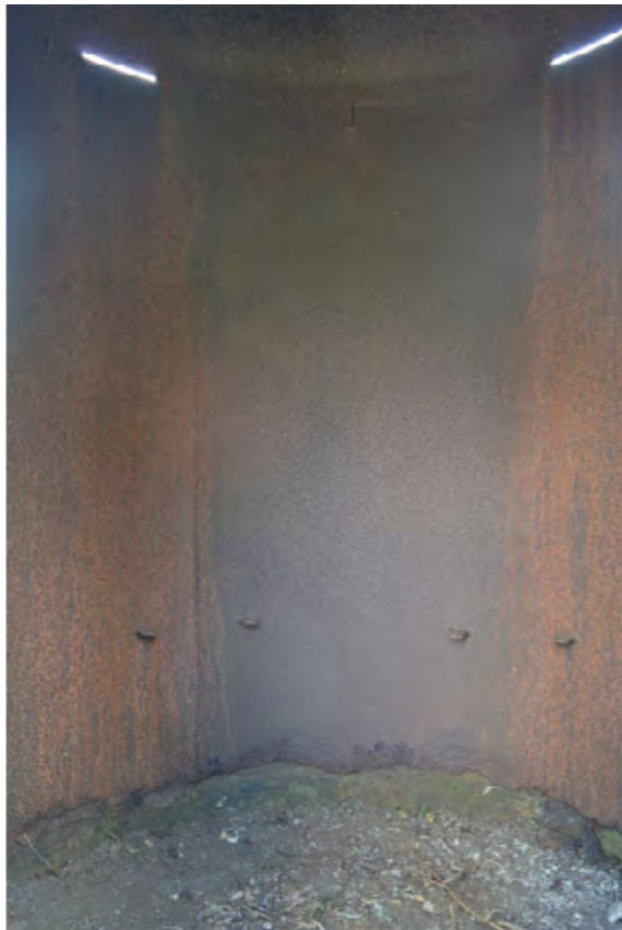
Plate 170: Internal view of the north-eastern sentry post, note the welded construction, facing south-west (619)
