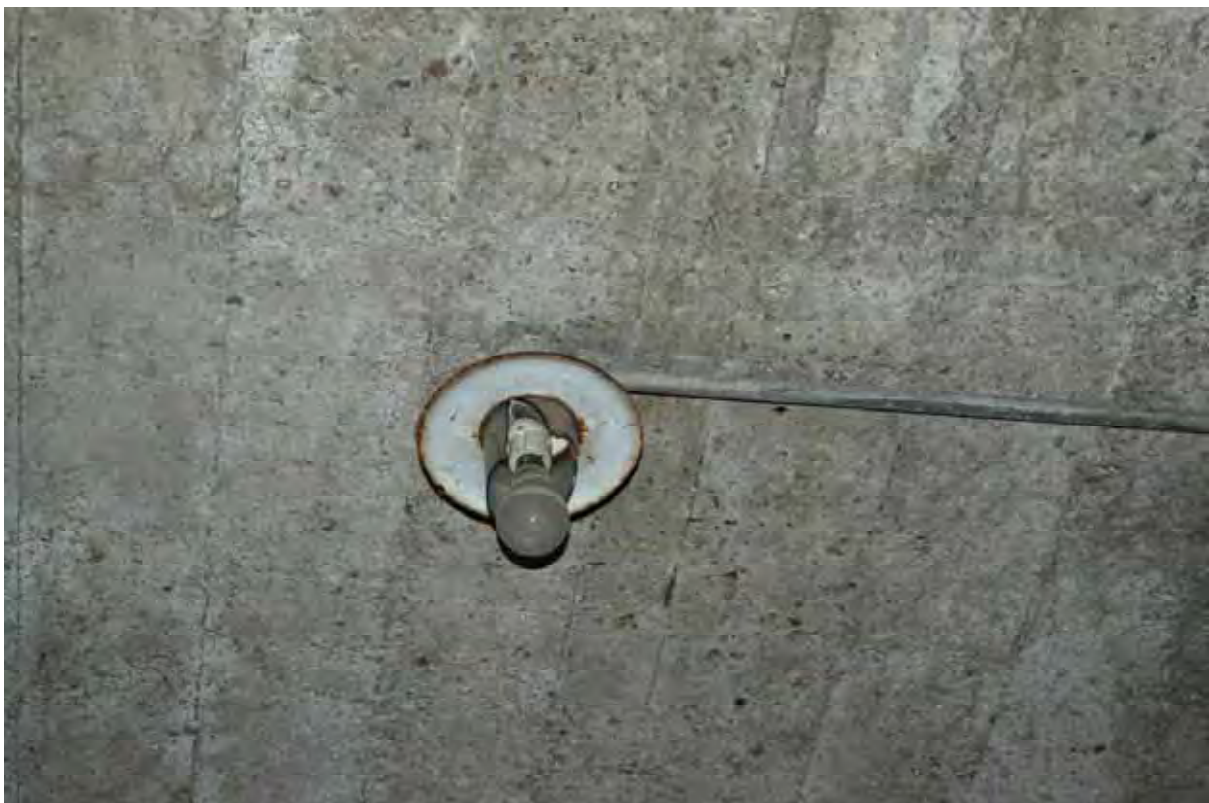
Plate 166: Store 14 – Detail of one of the retained light fittings within a number of the bays (eastern half), facing south (463)
