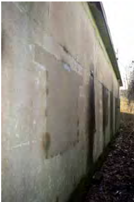
Plate 80: Store 6 – Detail of the blocked windows visible within the north-east elevation, facing north-west (359)
