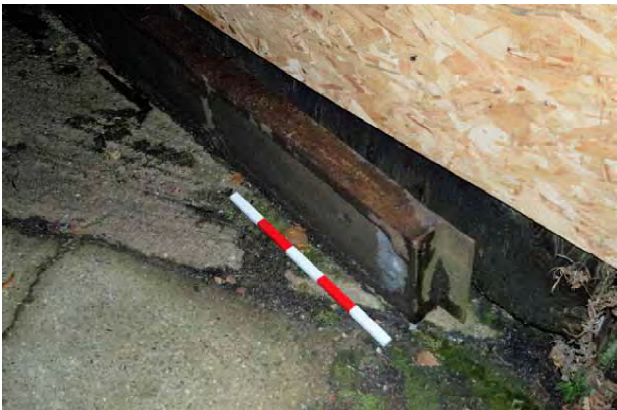
Plate 202: Detail of the displaced conveyor track element, situated adjacent to the south-east elevation of Building 2, facing south (552)
