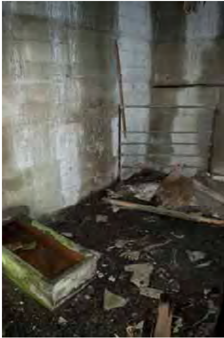
Plate 163: Store 14 – View of the alterations made within each of the eastern bays to accommodate the store's later use as a piggery, facing south-west (469)
