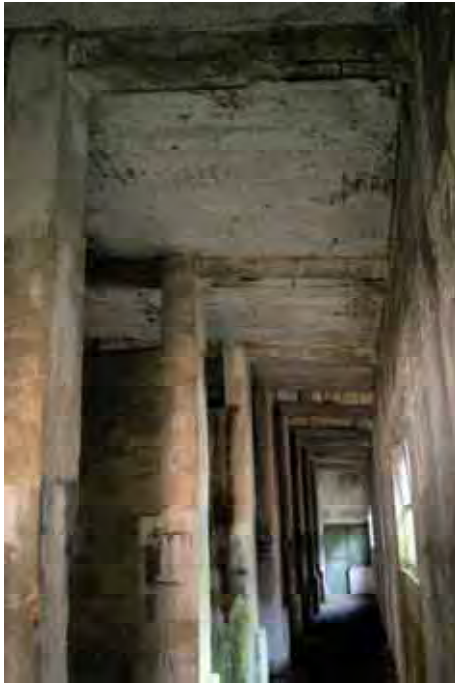
Plate 33: Store 4 – View of the store's roof construction above the western passage, facing south-east (263)
