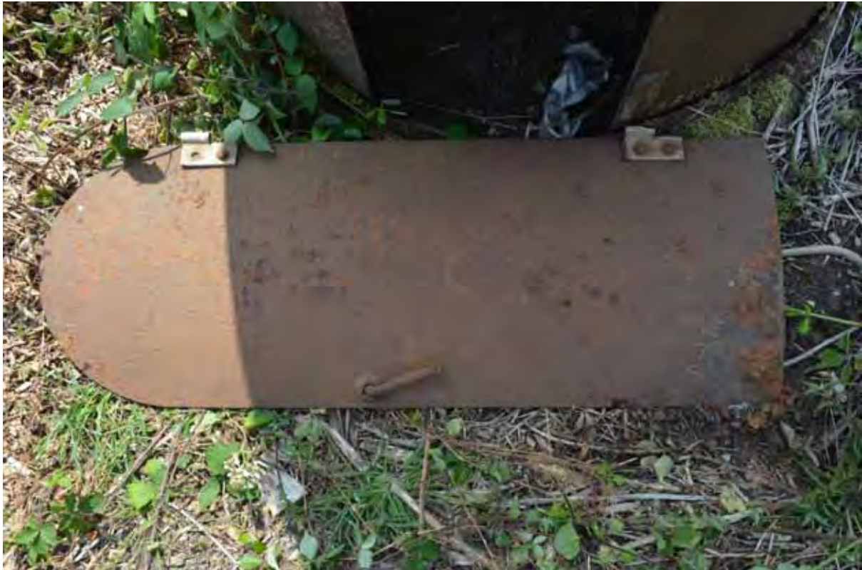
Plate 175: Detail of the detached door adjacent to the north-eastern sentry post, facing south-west (614)
