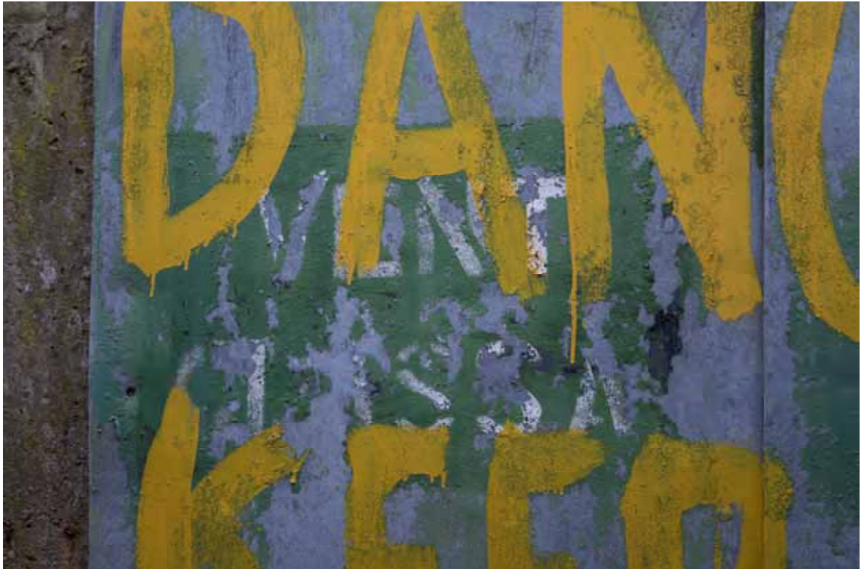
Plate 29: Store 4 – Detail of the 'Vent Class A' stencilling found on the external face of each store door (western door serving the northern loading bay), facing south-east (266)
