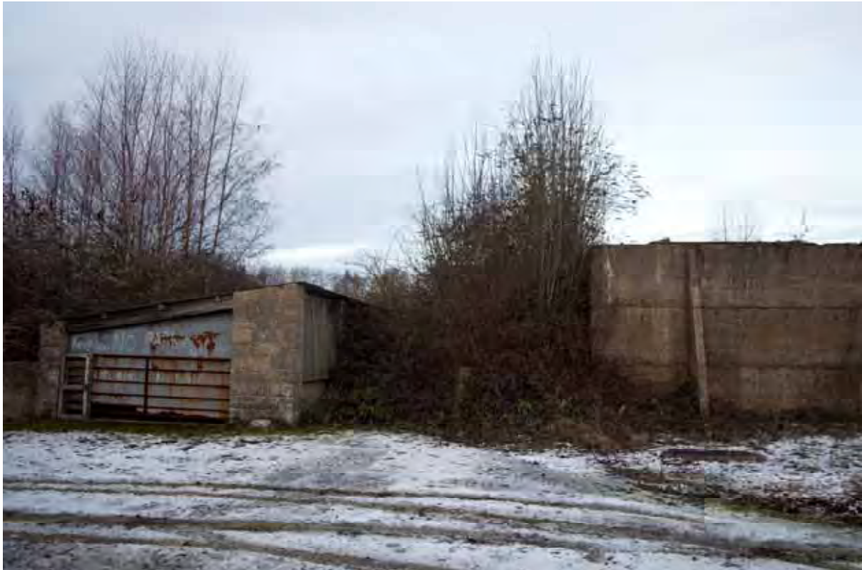
Plate 155: Store 14 / Building 13 – View of the northern loading bay, note the retained earth blast barrier, facing north-east (483)
