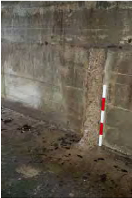
Plate 77: Store 6 – Detail of the retained footings of a former conveyor base situated in the western passage, facing south (346)
