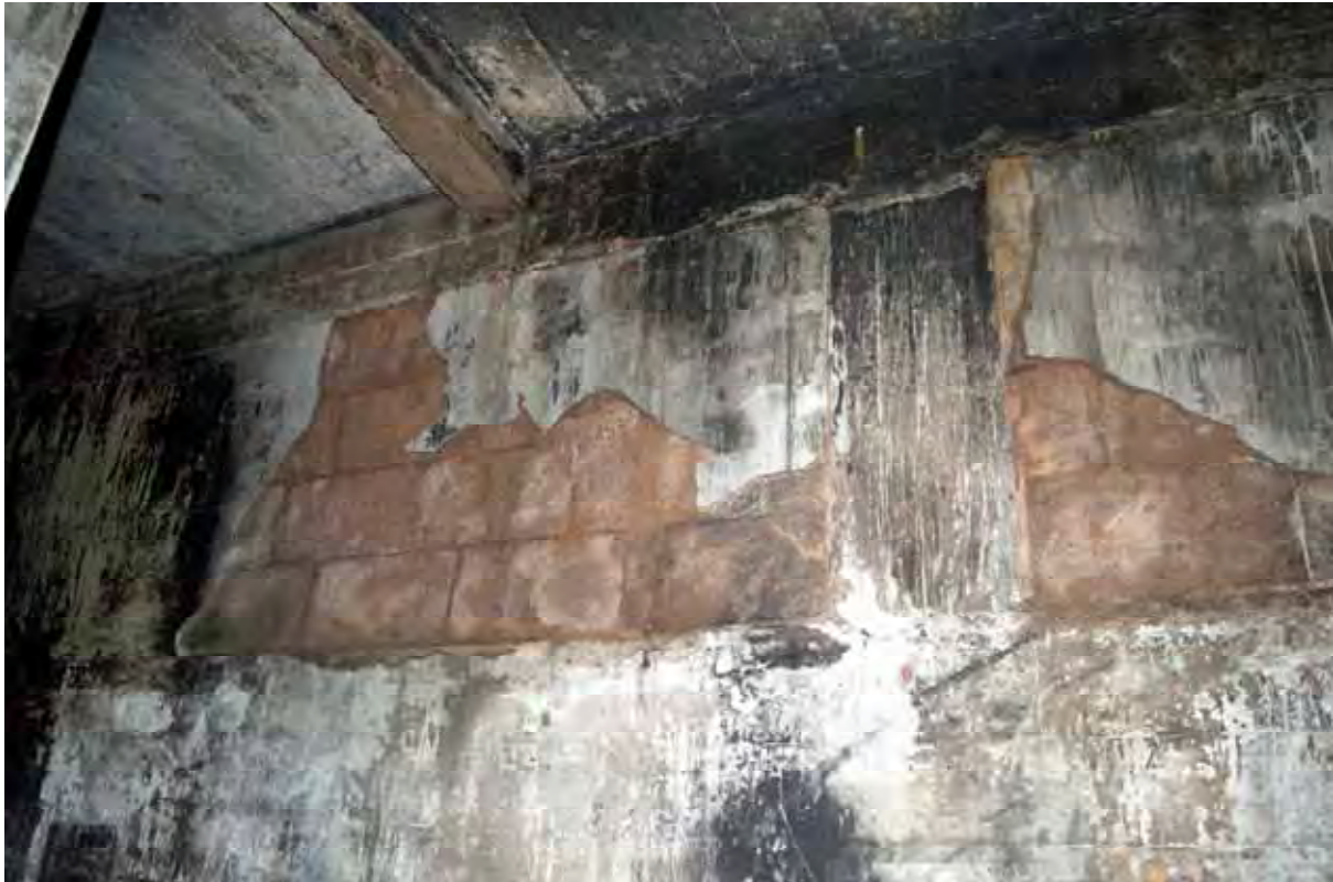
Plate 103: Store 8 – Detail of the fire damaged south-west wall within the western passage, note the concrete blocks used to fill the former openings, facing south (431)
