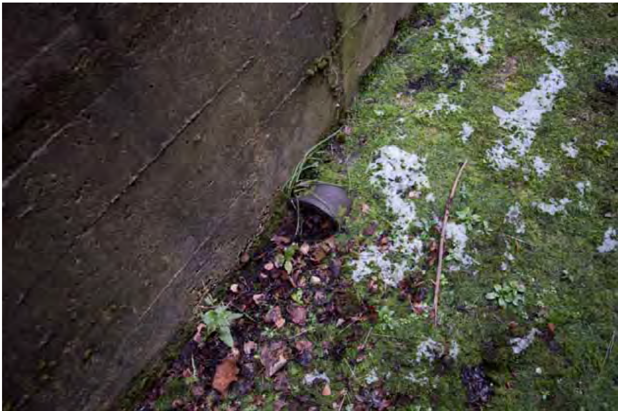
Plate 82: Store 6 – Detail of the drainage channels built into the inner walkway (south-east elevation), facing south (347)
