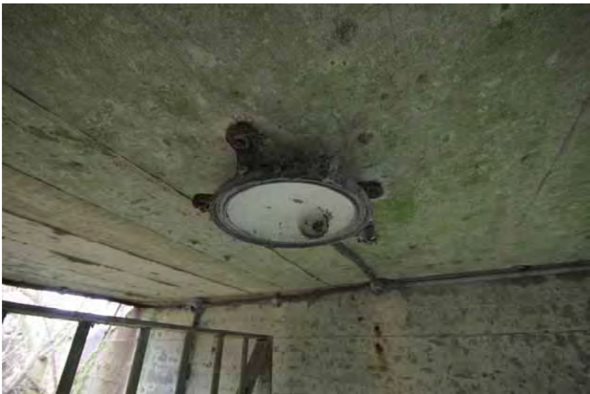
Plate 14: Store 4 – Detail of the Revo light fitting serving each covered entrance, facing west (64)
