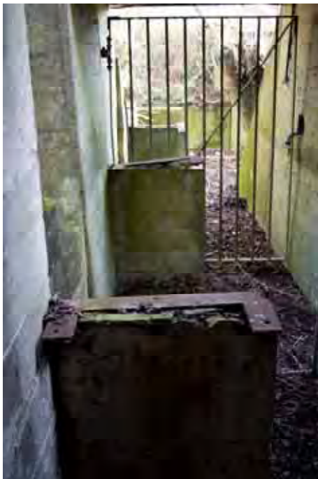
Plate 16: Store 4 – View of the southern loading bay serving the eastern half of the structure, note the complete nature of the bases and end platform (with brackets), facing south-east (277)
