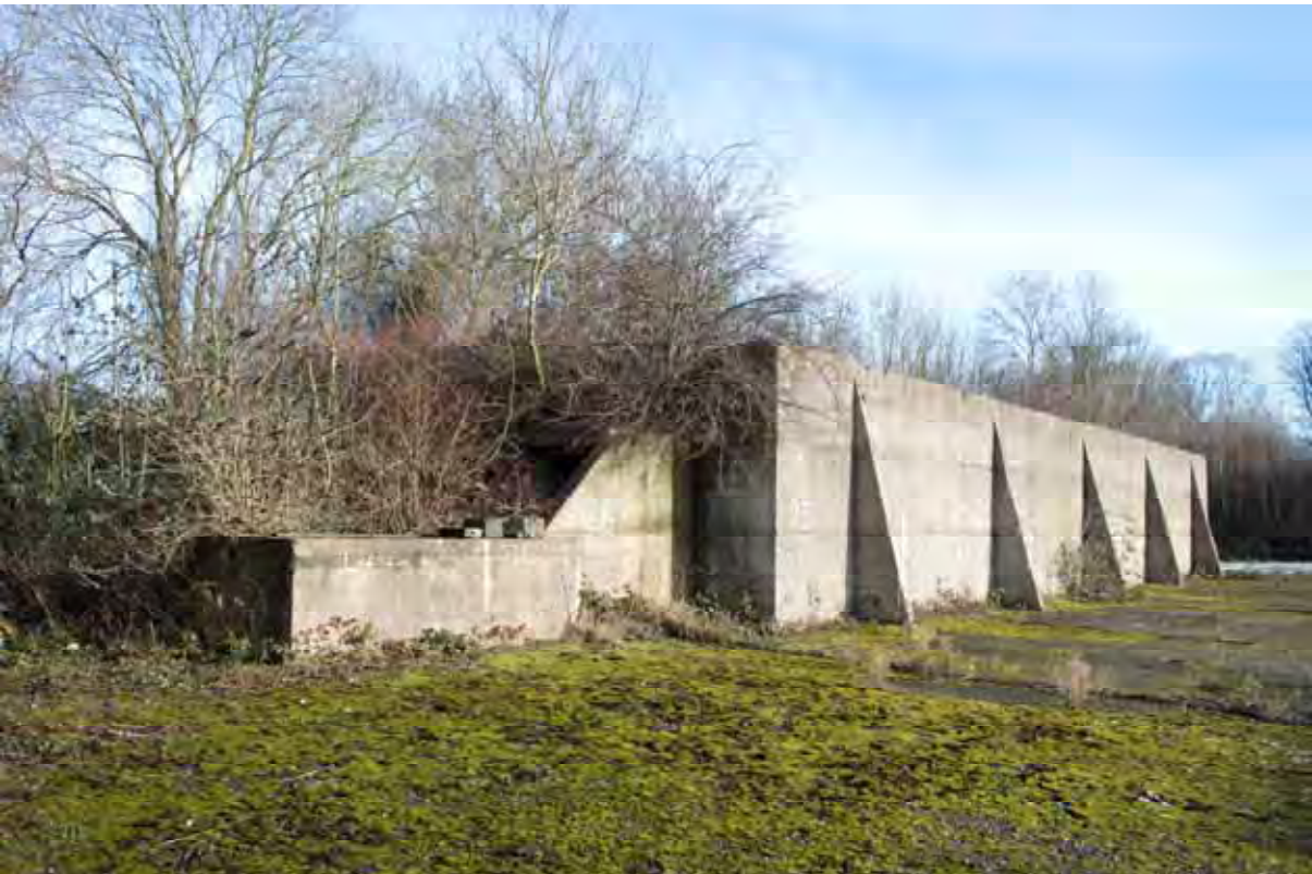
Plate 54: Store 5 – View of the north-west and south-west elevations of the outer blast wall, note the retained earth barrier along the north-west elevation, facing south-east (290)
