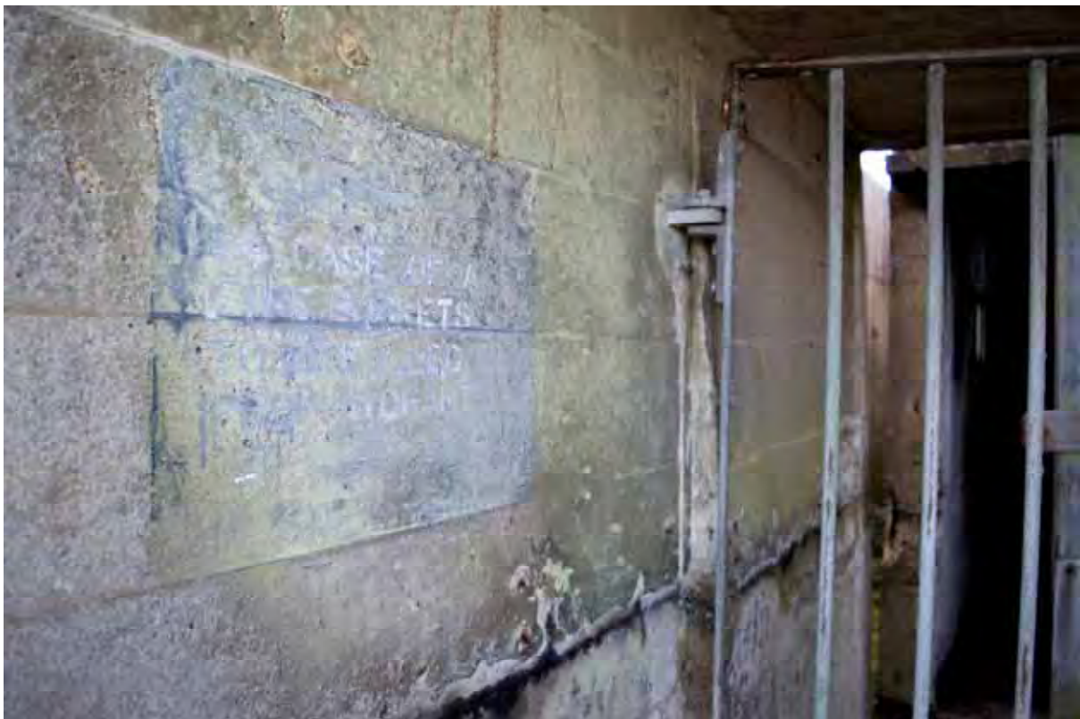
Plate 118: Store 9 – Detail of the fire hydrant signage found on the south-west wall of the western entrance serving the southern loading bay, facing north-west (377)
