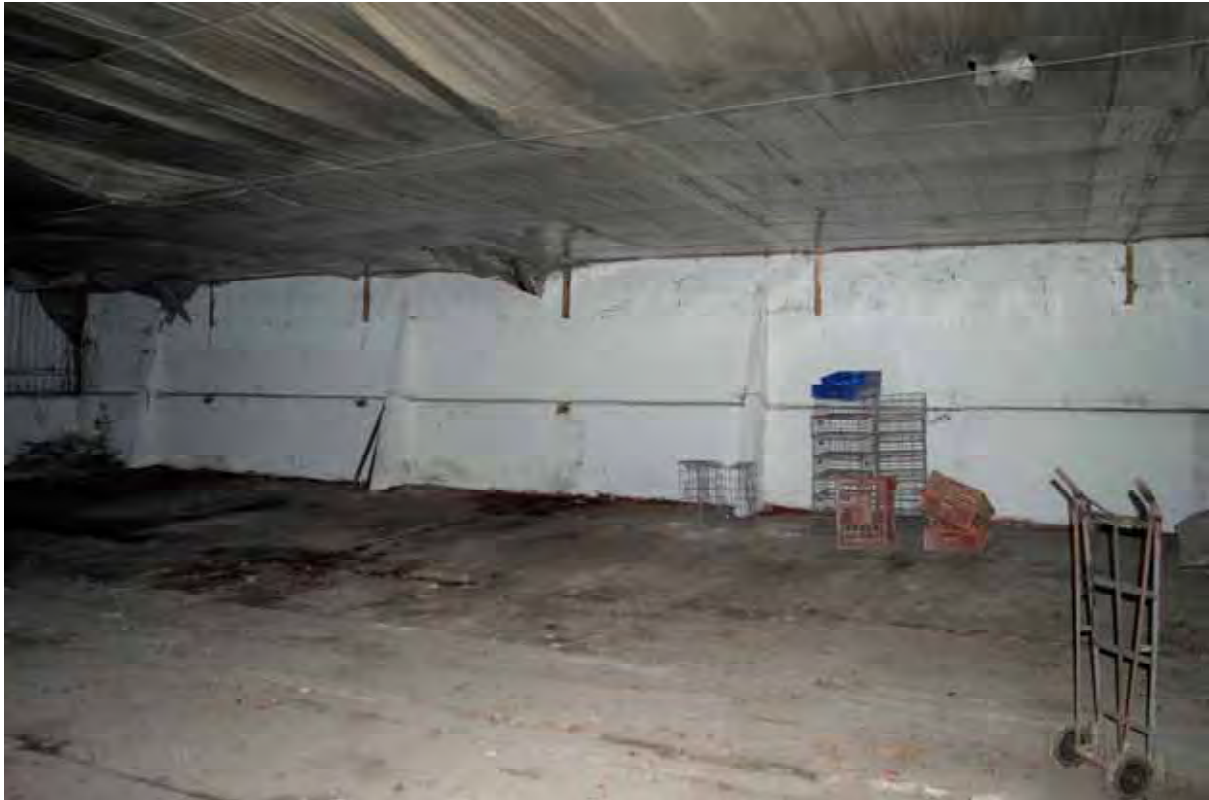
Plate 217: View of the north-east elevation of Store 10, situated within Building 10e, facing south-west (567)
