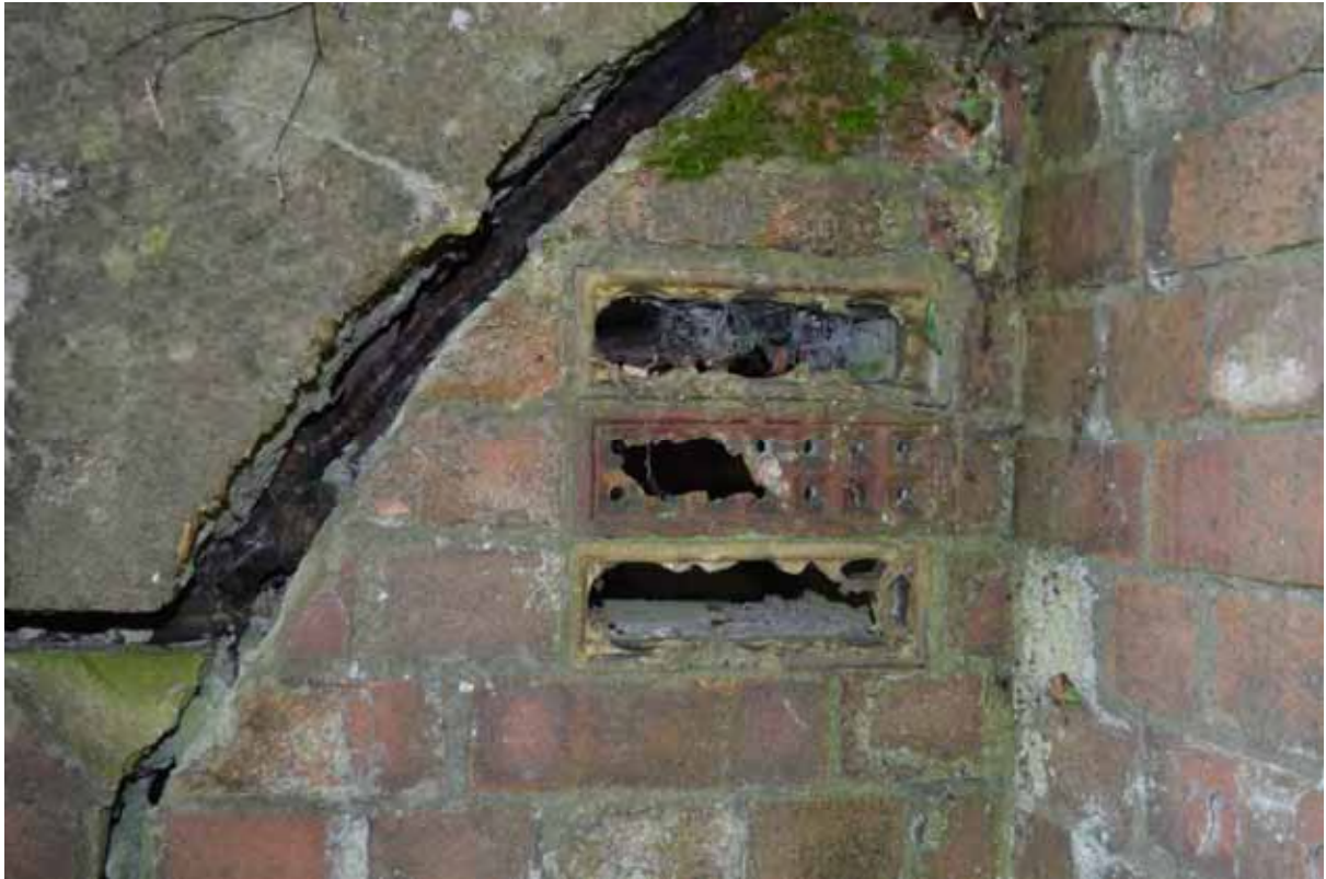
Plate 189: Detail of the air-bricks within the north-west elevation of the air-raid shelter, facing south-west (609)
