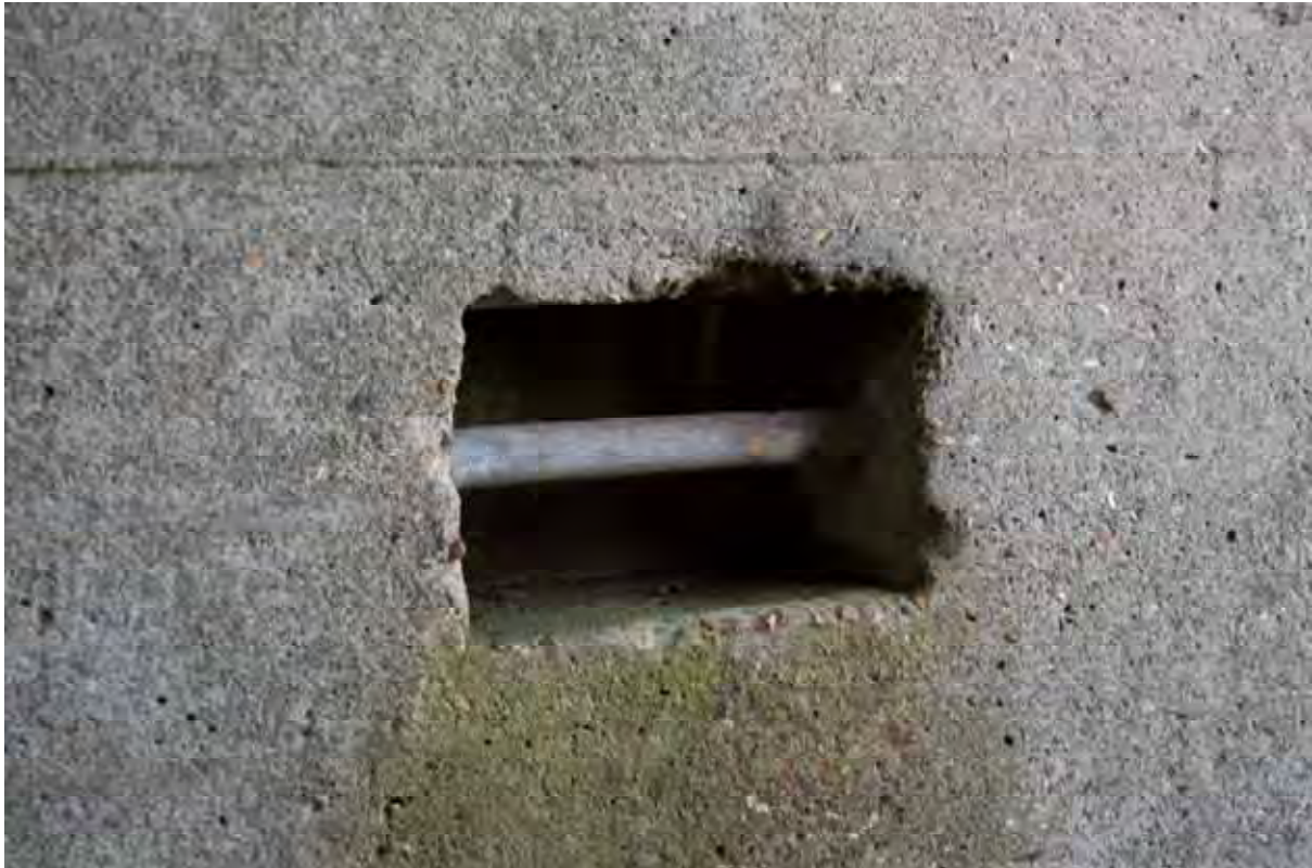
Plate 13: Store 4 – Detail of the integral locking bar for the gates within each covered entrance, facing east (334)
