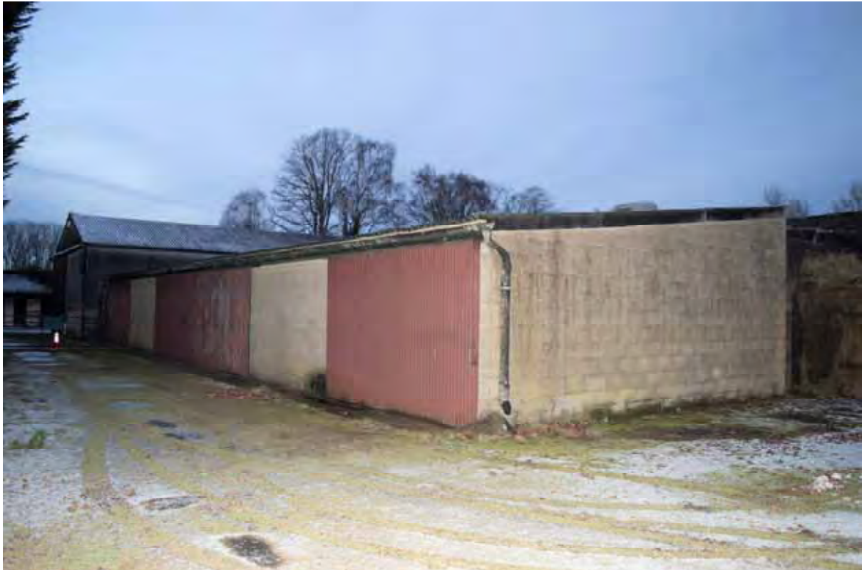
Plate 209: View of the south-west and south-east elevations of Building 10b, facing north (531)
