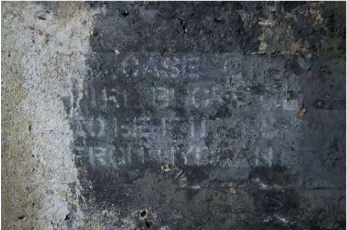
Plate 147: Store 12 – Detail of the fire hydrant signage situated on the south-west wall of the western entrance serving the southern loading bay, facing west (492)
