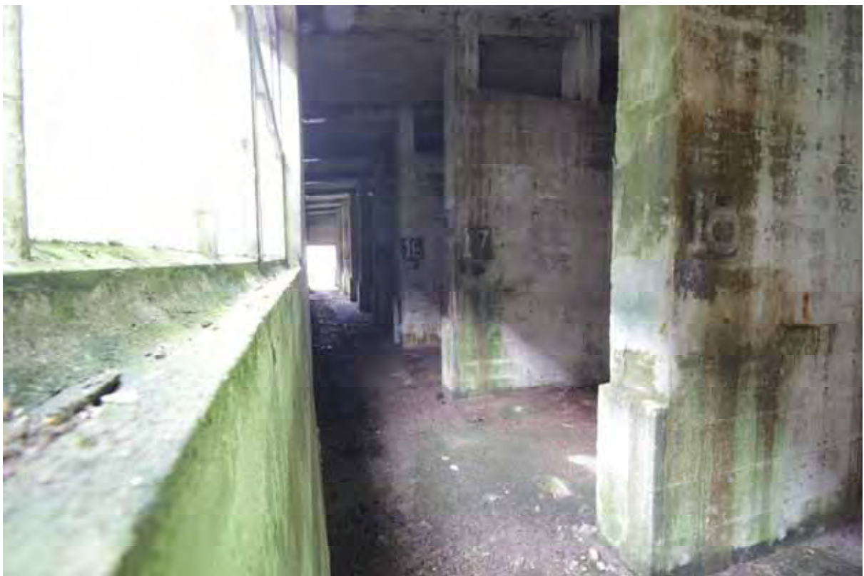
Plate 30: Store 4 – Internal view of the western passage and storage bays, facing north-west (1)
