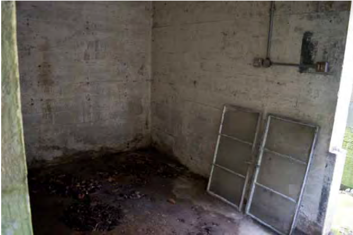
Plate 51: Store 4 – Displaced window casements within Bin 1 (eastern half), facing north-west (274)
