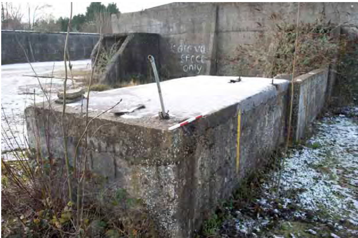
Plate 96: Store 8 – View of the eastern platform serving the southern loading bay, note the brackets and lamp fixture, facing west (413)
