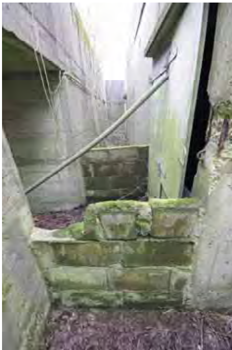
Plate 48: Store 4 – Later 20 th century alterations to the south-east walkway, comprising low level concrete block walls, facing south-west (11)
