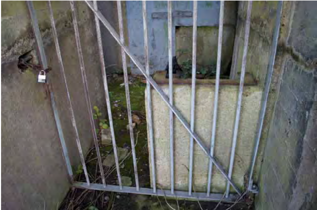
Plate 95: Store 8 – Detail of the conveyor bases retained within the western entrance serving the southern loading bay, facing north-west (409)
