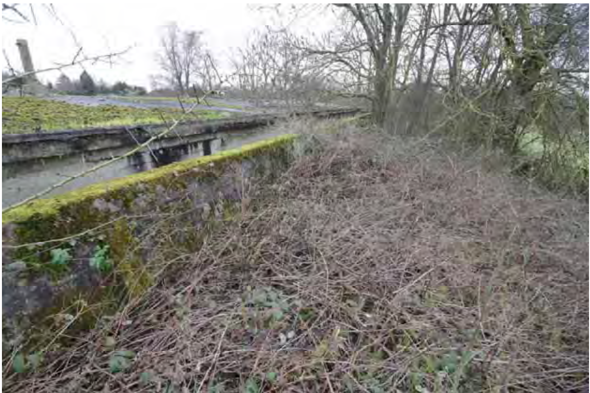
Plate 8: Store 4 - View of the earth blast barrier banking the north-east elevation of the outer blast wall, facing north (73)
