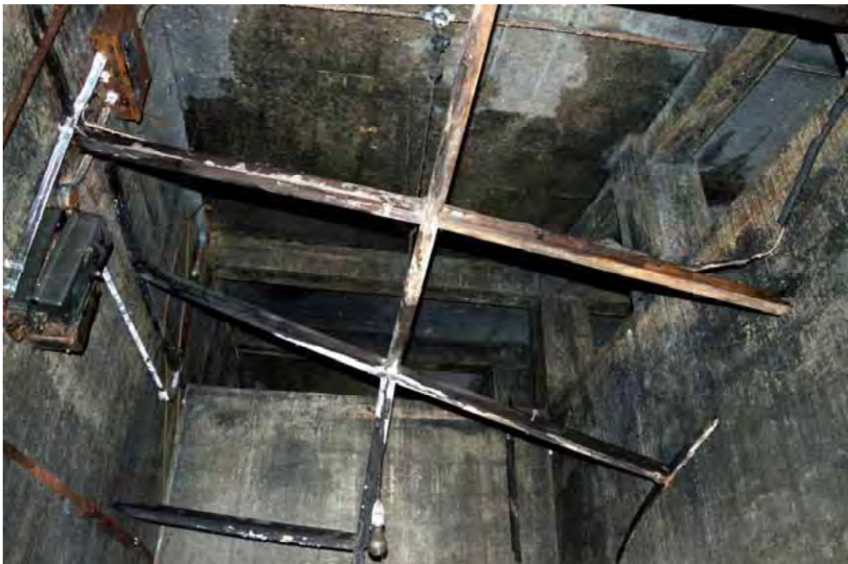
Plate 66: Store 5 – Detail of the inserted stud framework used to create lower ceilings in a number of the bays (Bin 10), facing north-east (308)
