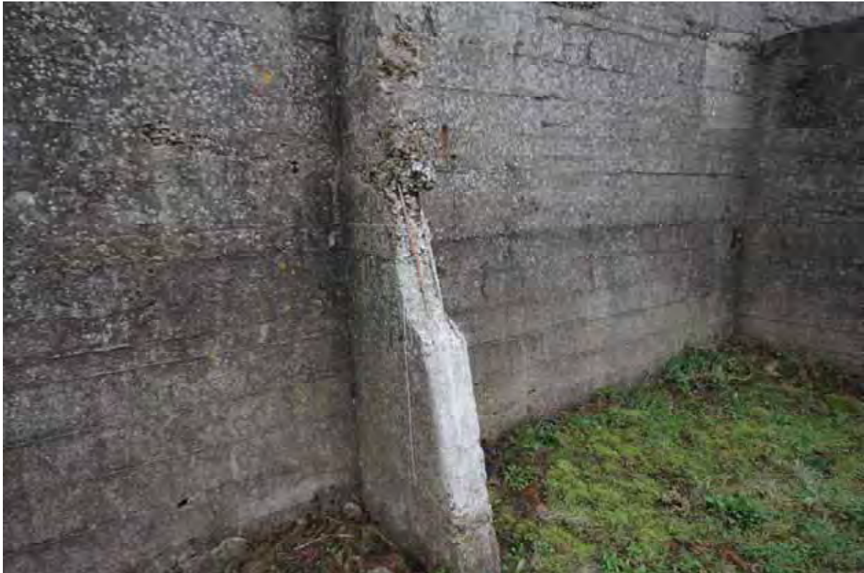
Plate 11: Store 4 – Detail of the concrete buttresses supporting each outer blast barrier wall, facing south-east (135)
