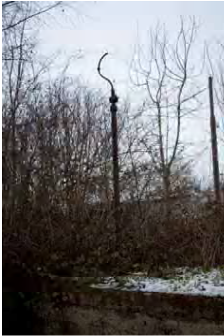
Plate 145: Store 12 – Detail of the retained lamp fitting upon the eastern platform in the northern loading bay, facing north-east (508)
