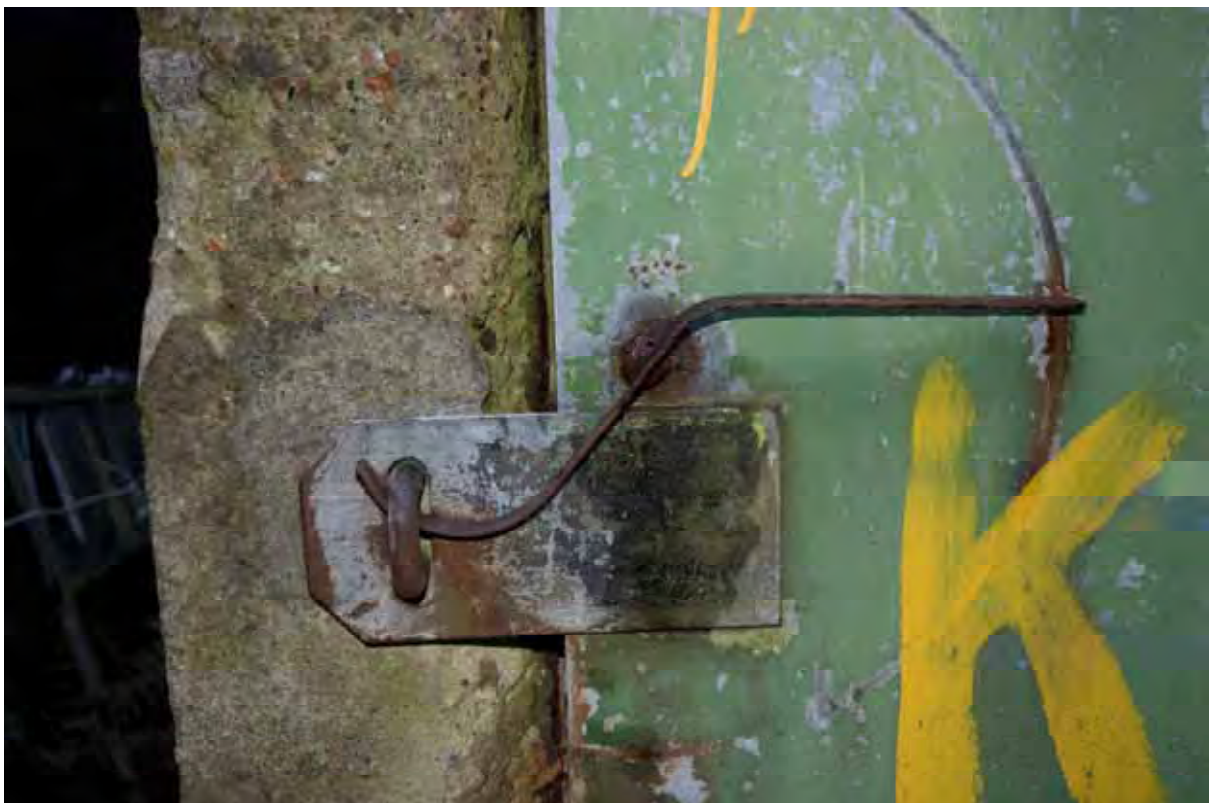
Plate 150: Store 12 – Detail of the door hook found on all doors within this store (western door serving the southern loading bay), facing north-west (495)
