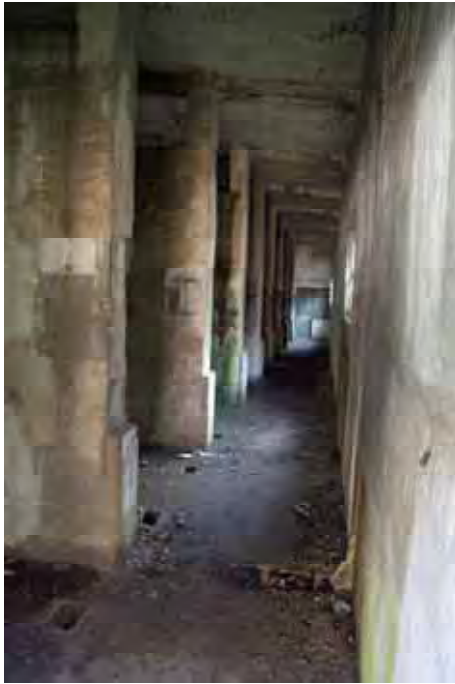
Plate 37: Store 4 – View of the store's western passage and bay divisions, facing south-east (245)
