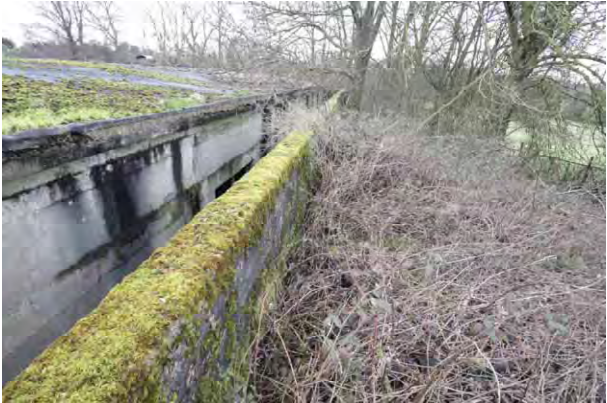
Plate 7: Store 4 – View of the open walkway separating the north-east elevation of the store from the outer blast wall, facing north (81)
