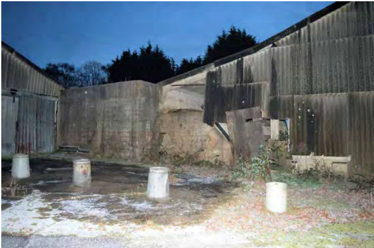
Plate 134: Store 10 – View of the northern end of the north-east elevation, note the encroachment of later 20 th century structures on all sides, facing south (562)
