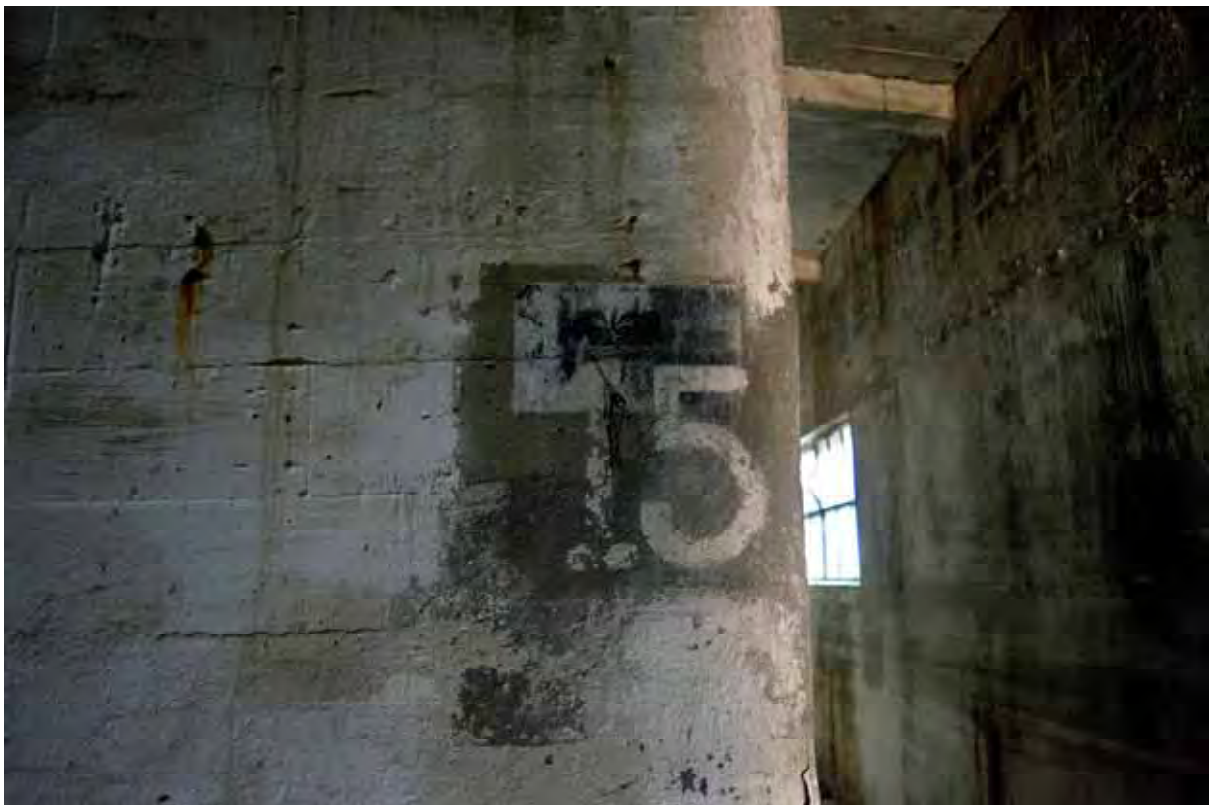
Plate 34: Store 4 – Detail of the storage bay signage, note the phasing (western half), facing south-east (257)
