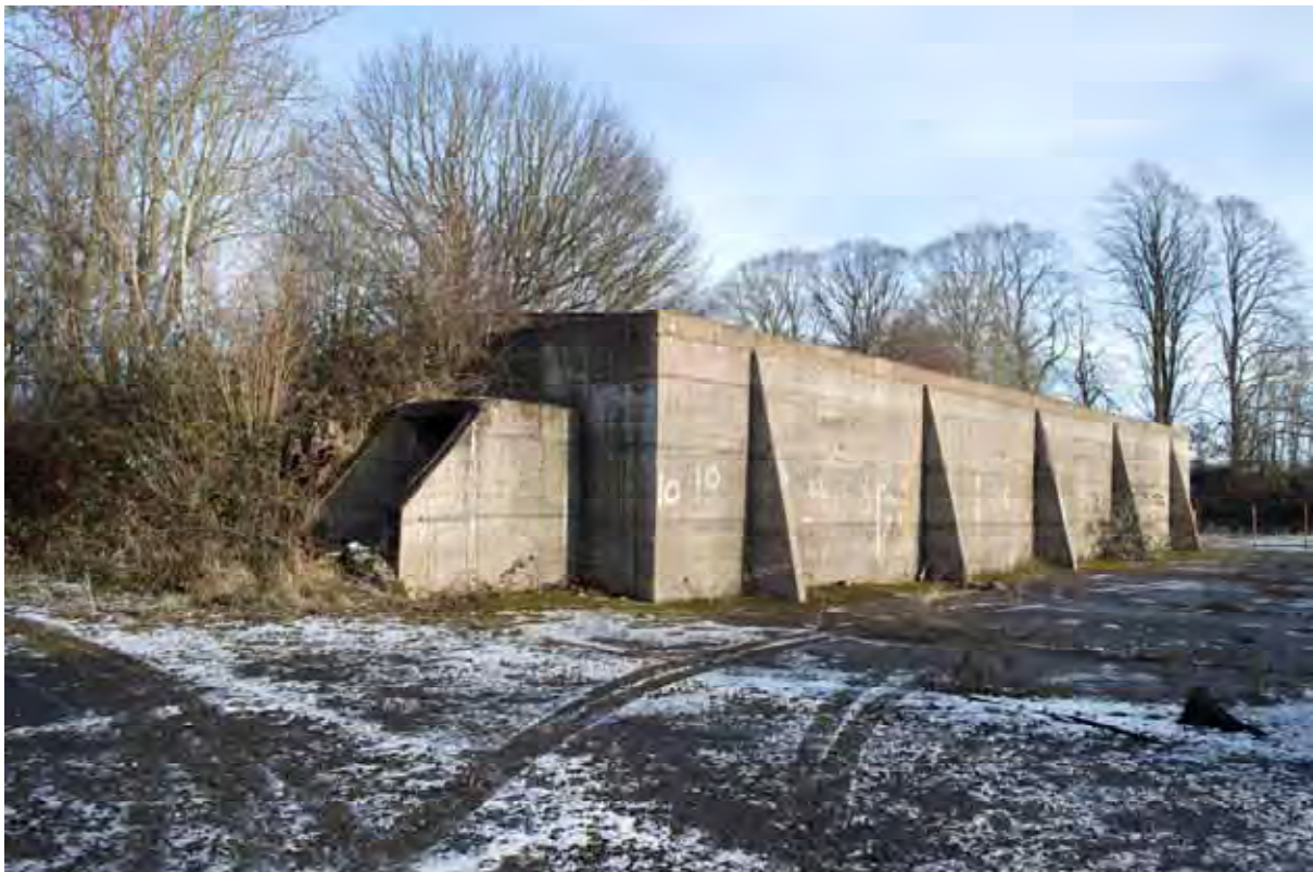
Plate 76: Store 6 – Detail of the removed loading platform to the western side of the northern bay, facing east (328)
