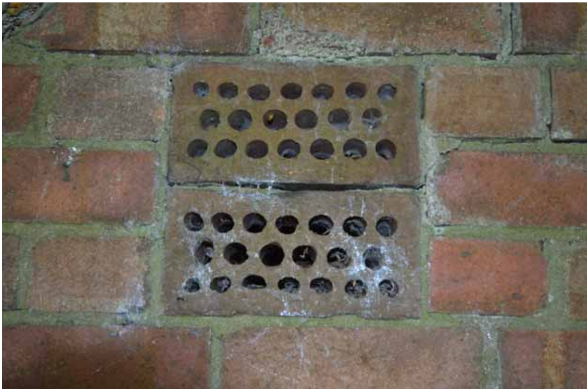
Plate 188: Detail of the air-bricks within the south-west elevation of the air-raid shelter, facing north-east (608)
