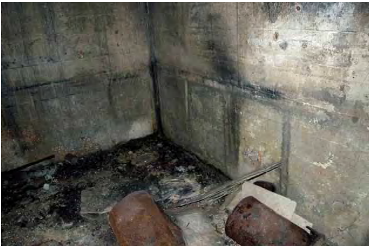
Plate 68: Store 5 – Soot staining left on the walls of Bin 4, facing west (322)
