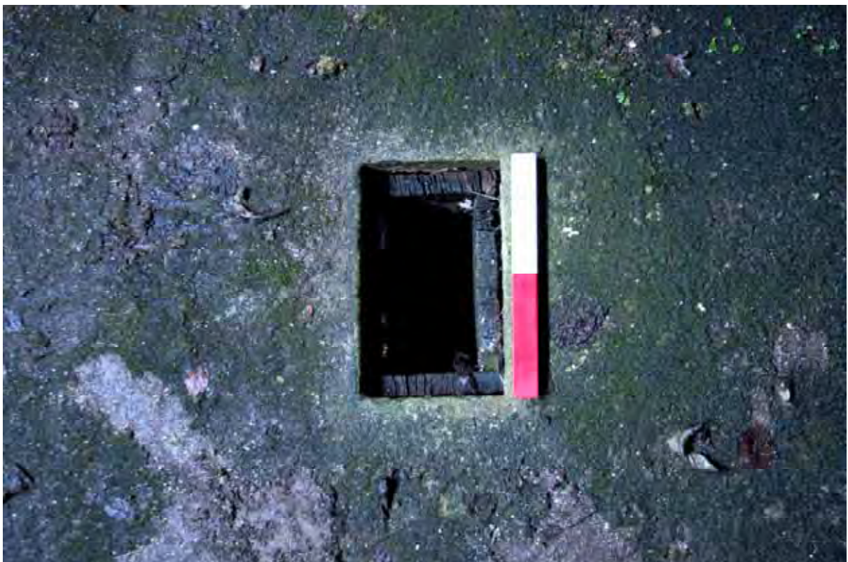
Plate 36: Store 4 – Detail of the floor sockets within each bay (eastern half), facing south-west (251)
