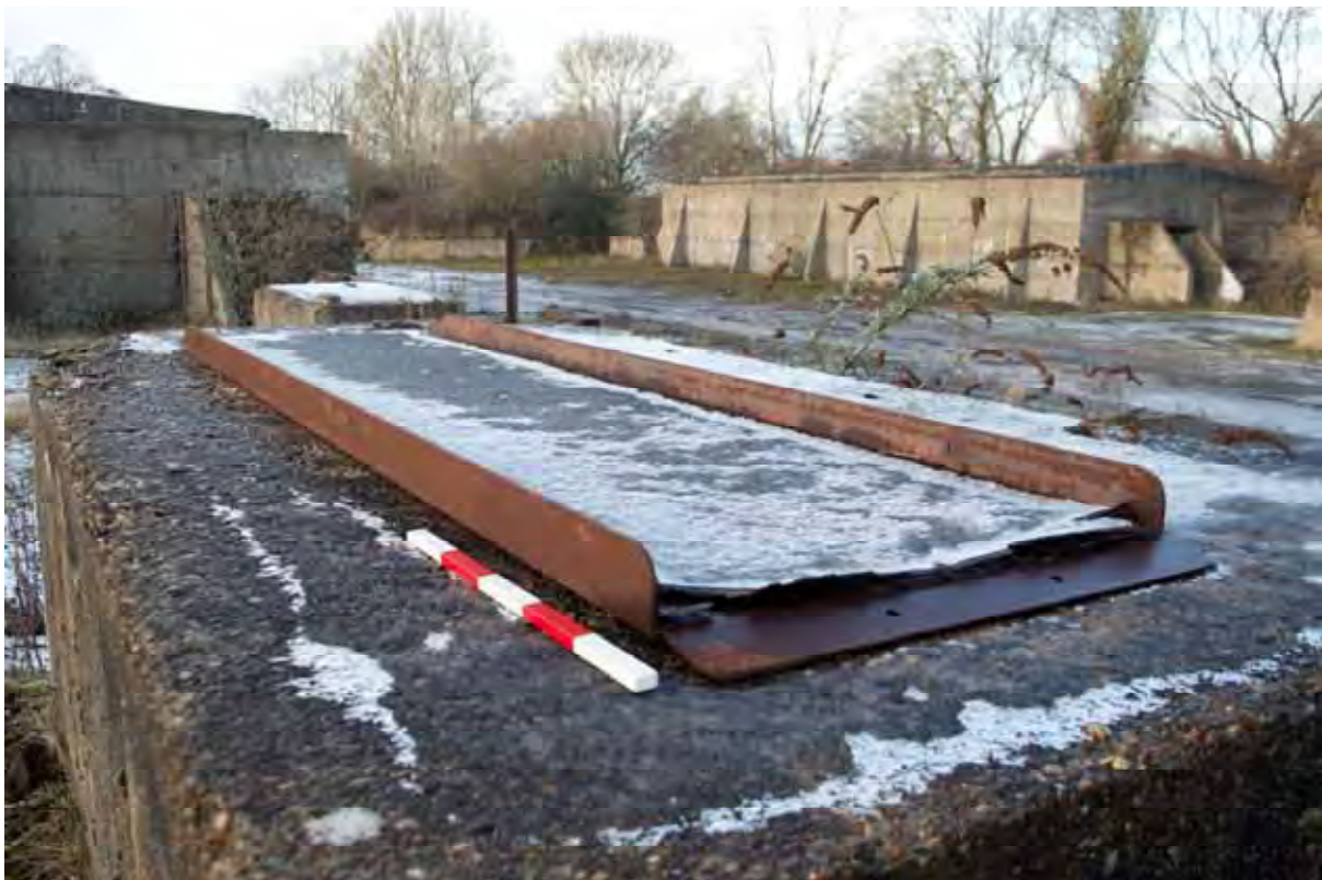
Plate 116: Store 9 – Retained conveyor track on the eastern platform within the northern loading bay, facing north (406)
