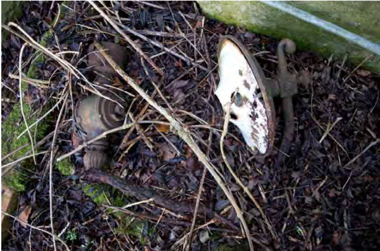
Plate 43: Store 4 – Detail of the displaced light fitting formerly situated on the eastern loading platform serving the southern loading bay, facing east (285)
