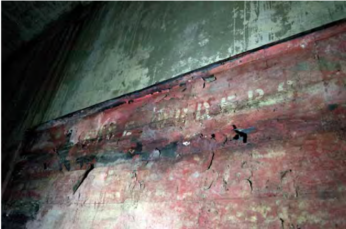
Plate 89: Store 6 – Detail of the retained timber notice board within the northern end of the western passage, entitled 'Fire Orders', facing south-west (342)
