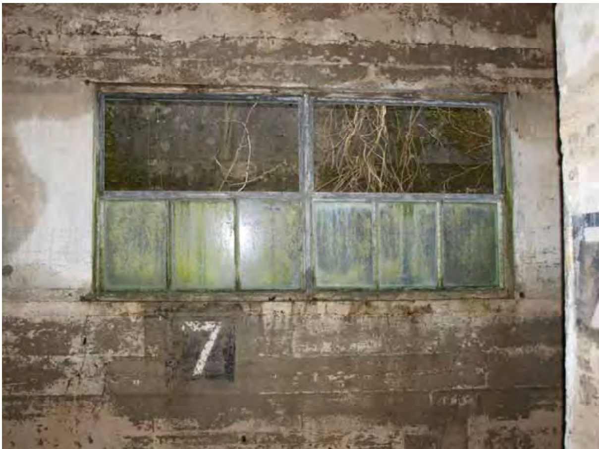
Plate 50: Store 4 – Missing window casements within the northern window in the eastern passage, facing north-east (201)
