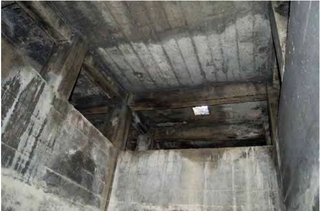
Plate 107: Store 8 – View of the bay roof arrangement and external vents situated above the central void, facing south-west (439)
