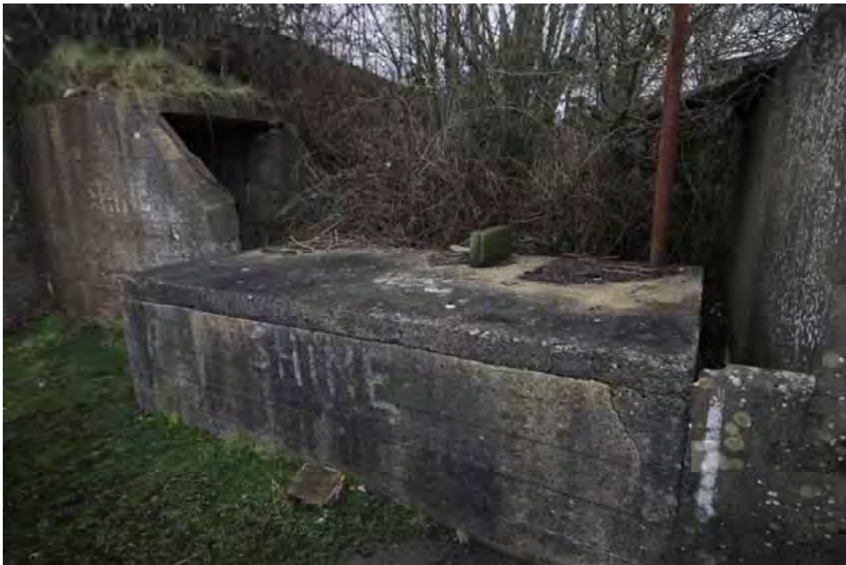
Plate 42: Store 4 – Detail of the western loading platform serving the southern loading bay, facing north (86)
