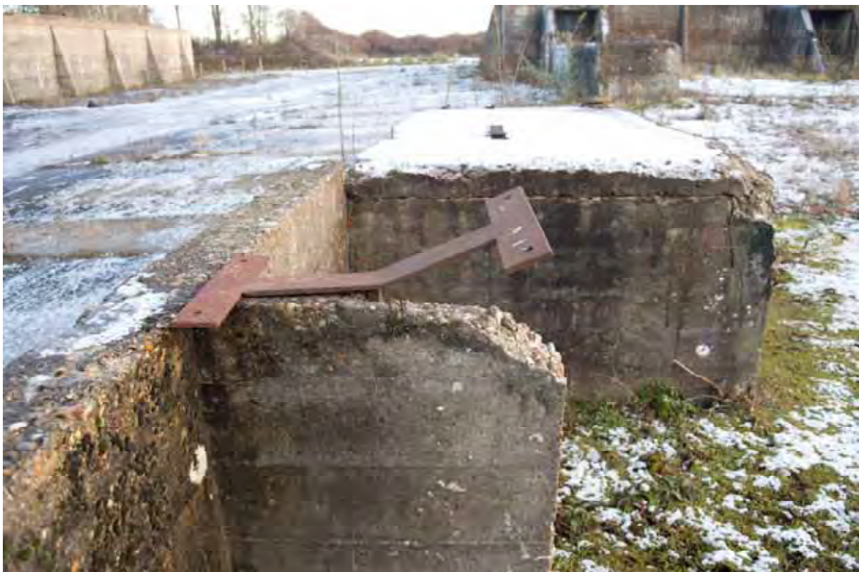
Plate 94: Store 8 – Detail of a retained conveyor base serving the eastern side of the southern loading platform, note the bracket fixing, facing south-east (414)
