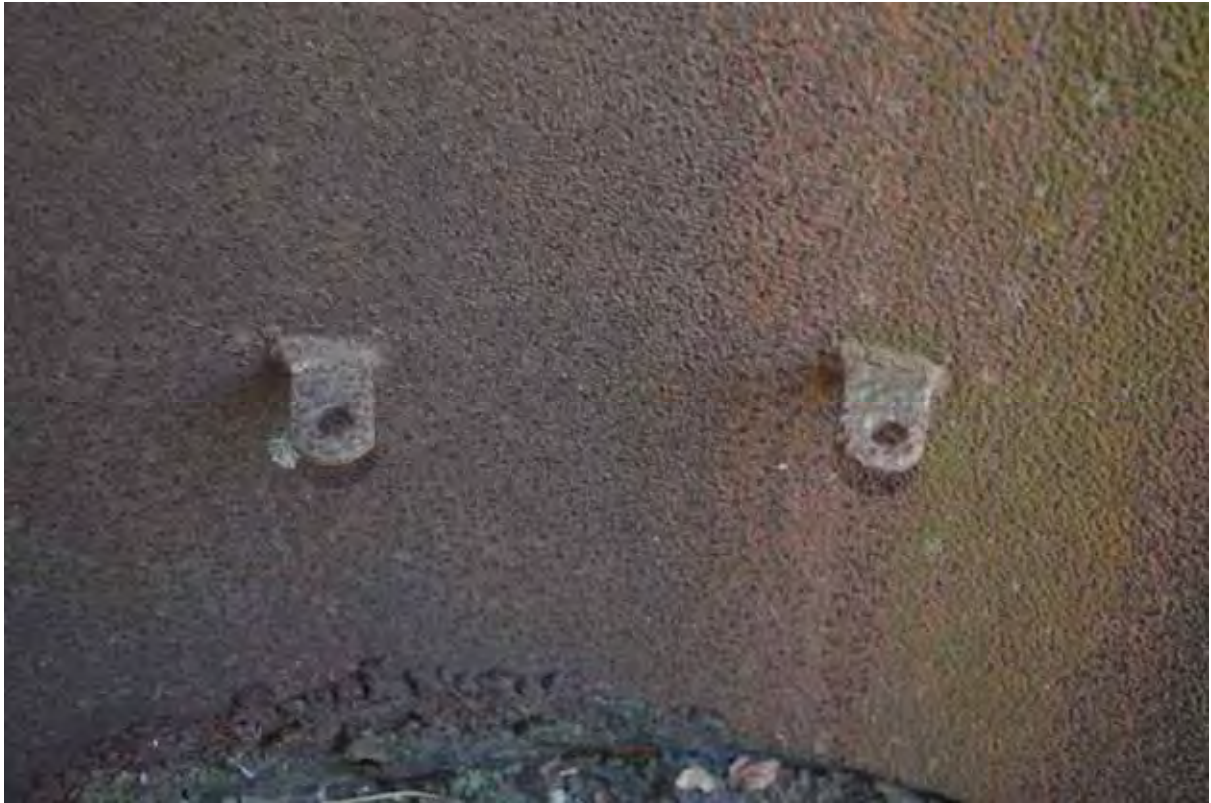
Plate 179: Detail of the bench brackets to either side of the north-eastern sentry post, facing south (617)
