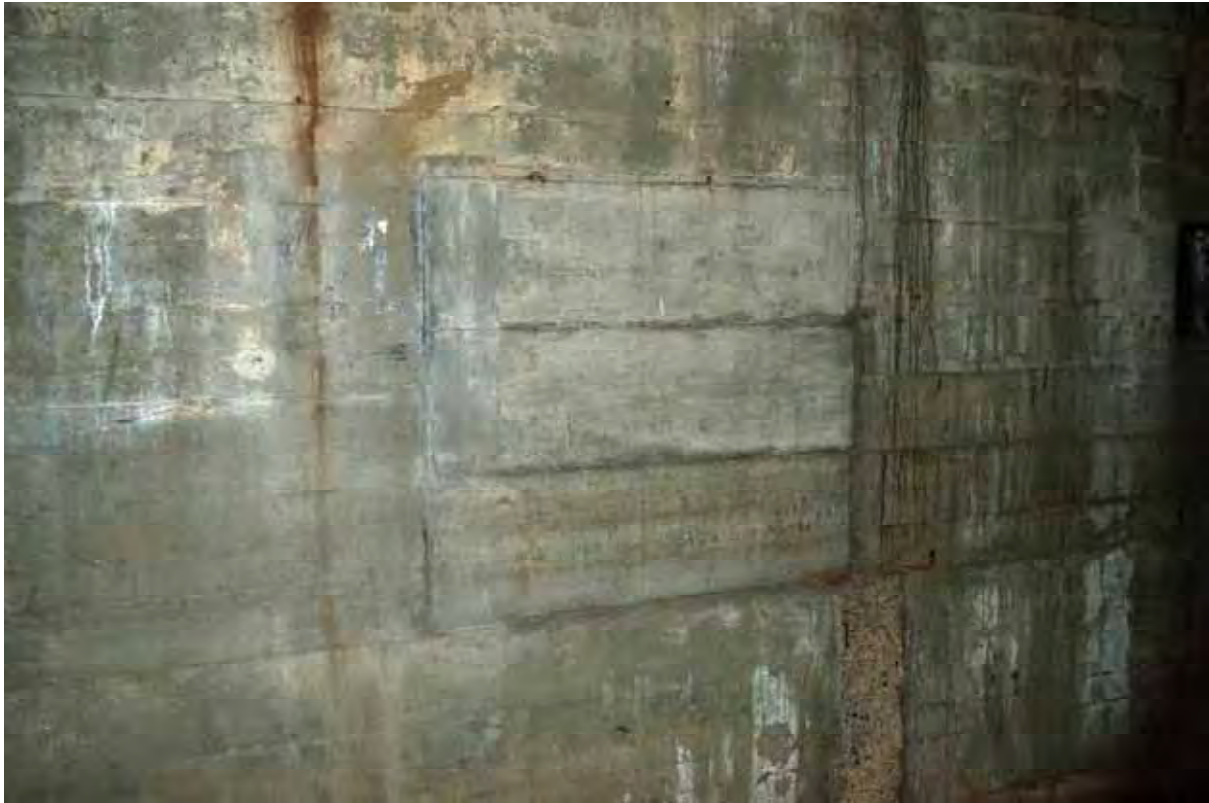
Plate 81: Store 6 – Evidence of the blocked window opening within the store's north-east wall, facing east (357)
