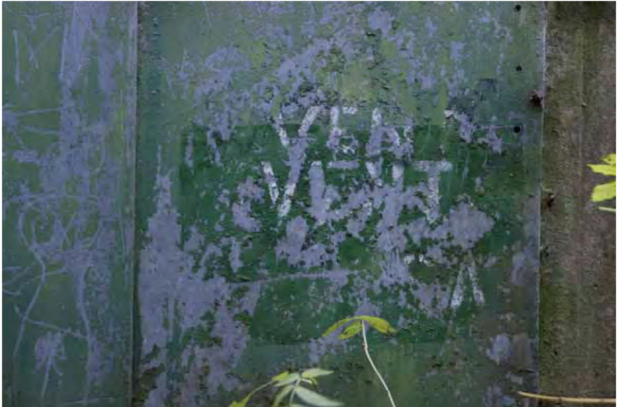
Plate 149: Store 12 – Detail of the door signage retained on the western doorway serving the northern loading bay, facing north-west (510)
