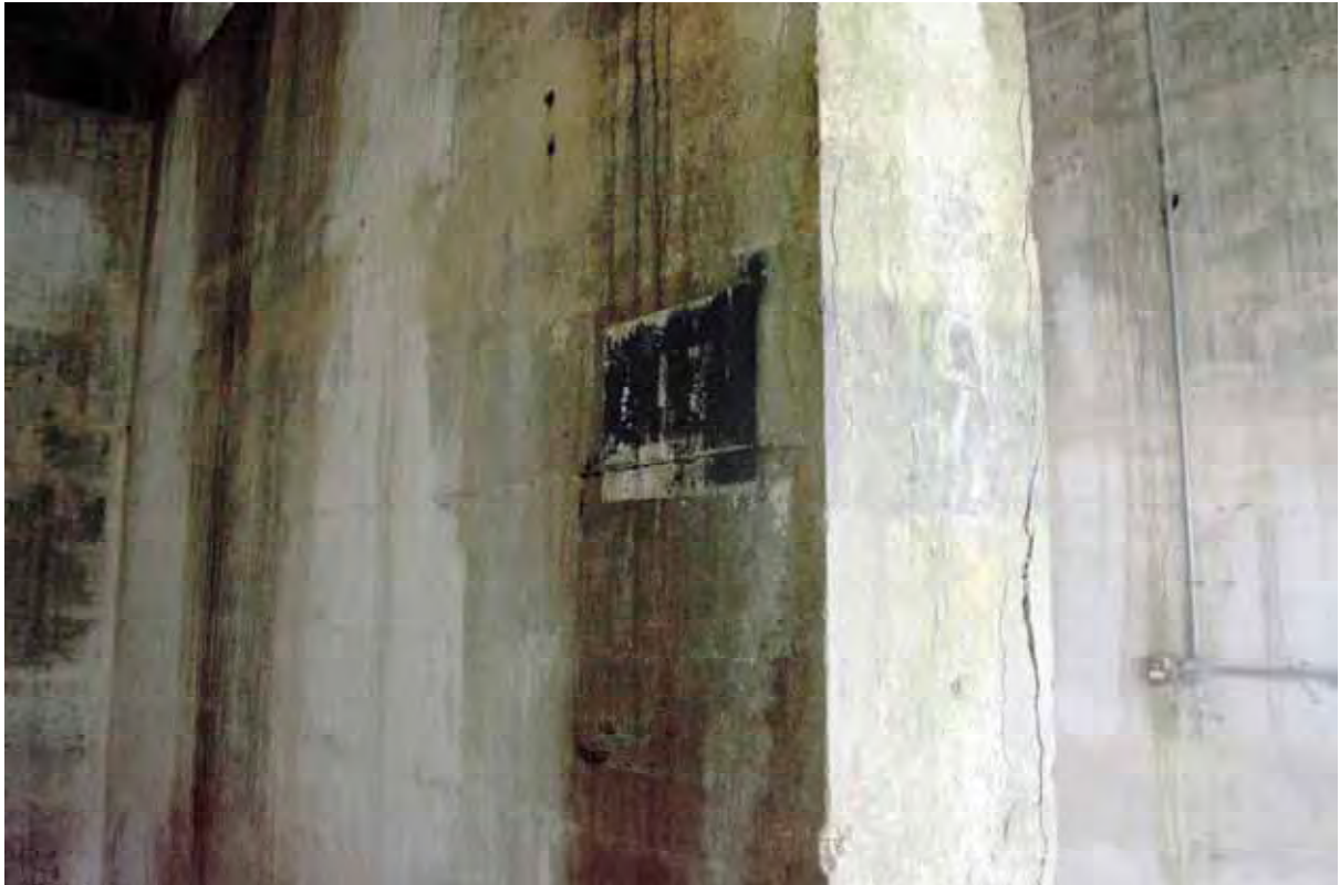
Plate 87: Store 6 – Detail of the signage visible on a number of the containment bay walls (Bin 9), facing north-west (340)
