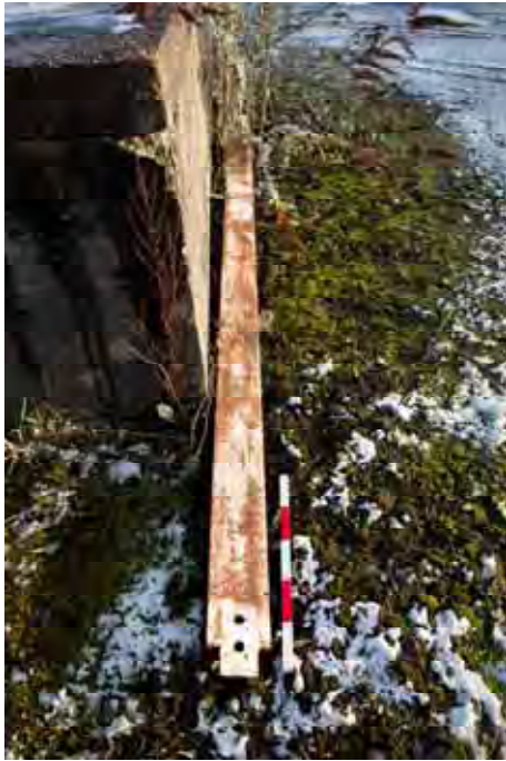
Plate 115: Store 9 – Detail of the displaced girder within the southern loading bay, facing south-east (372)
