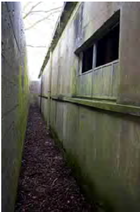
Plate 18: Store 4 – View of the inner walkway separating the north-east elevation of the inner structure and outer blast wall, facing south-east (270)
