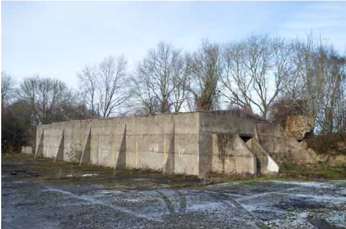
Plate 55: Store 5 – View of the south-west and south-east elevations of the outer blast wall, facing north (294)
