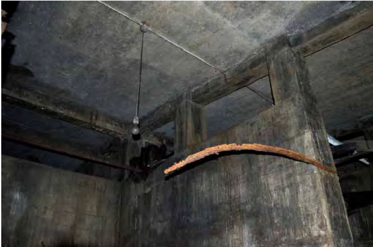
Plate 67: Store 5 – Detail of the metal brackets framing the containment wall of Bin 6, facing east (305)
