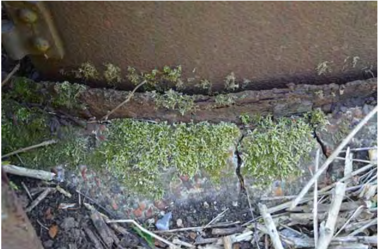
Plate 173: Detail of the hoop frame at the base of the north-eastern sentry post, facing south-west (621)
