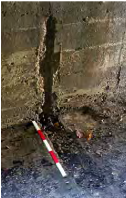
Plate 40: Store 4 – Detail of one of the removed conveyor bases within the western passage, facing west (250)
