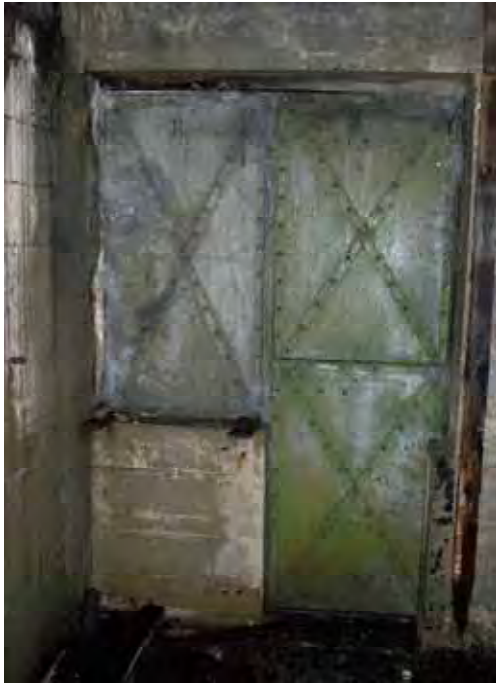
Plate 59: Store 5 – Detail of the conveyor base retained within the western doorway serving the northern loading bay, note the brackets, facing north-east (311)
