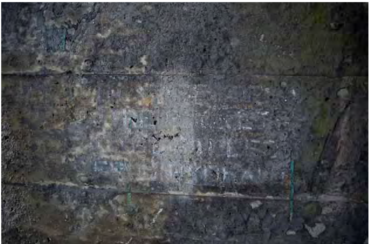
Plate 160: Store 14 – Detail of the fire hydrant signage on the south-west wall of the western entrance serving the southern loading bay, facing west (476)
