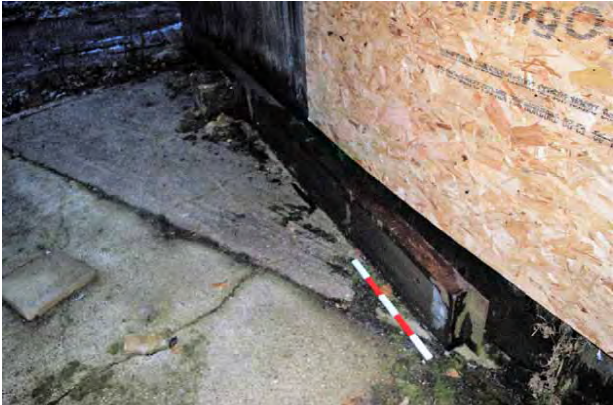
Plate 201: Detail of the displaced conveyor track element, situated adjacent to the south-east elevation of Building 2, facing south (551)
