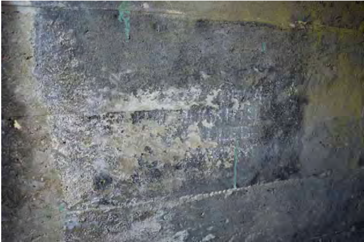
Plate 97: Store 8 – Detail of the fire hydrant signage visible on the south-west wall of the western entrance serving the southern loading bay, facing west (416)
