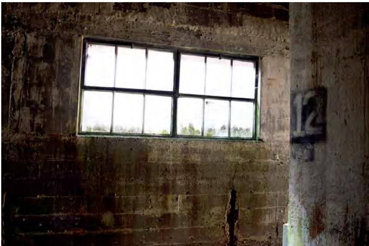
Plate 20: Store 4 – Detail of the current window detailing within the southern end of the store's south-west elevation, facing south-west (248)
