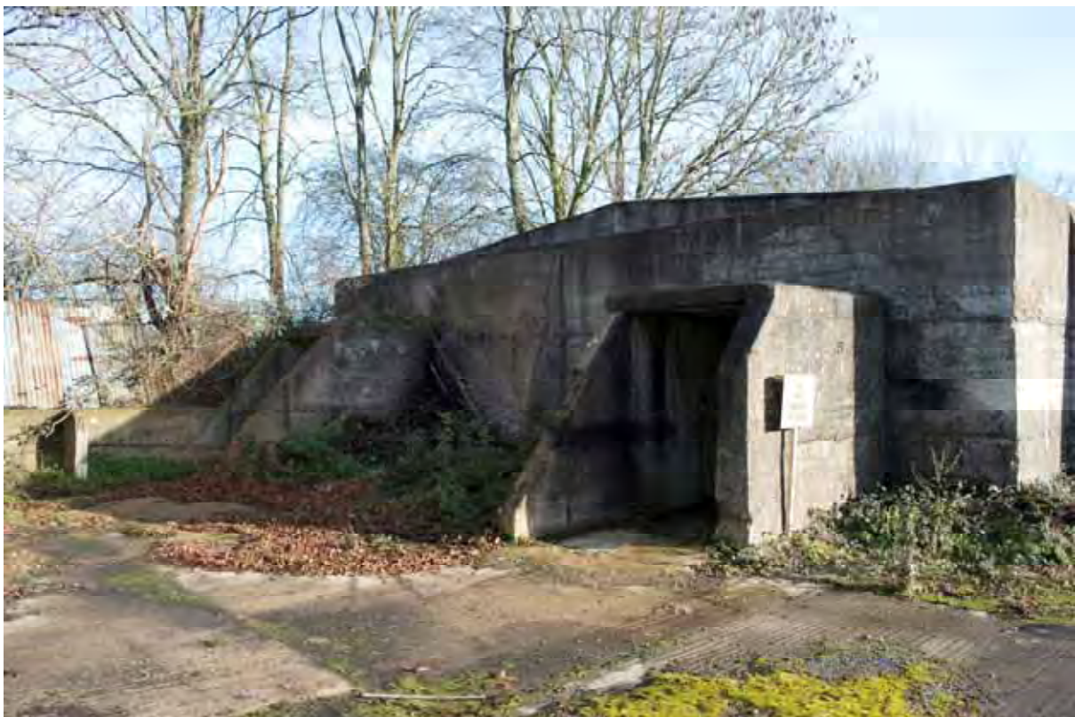
Plate 10: Store 4 – View of the northern loading bay, note the removed western platform, facing south-east (235)
