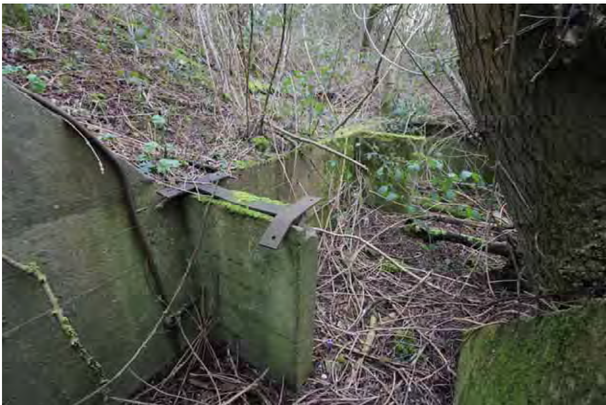
Plate 46: Store 4 – Detail of the retained conveyor bases within the southern loading bay (eastern side), note the metal brackets, facing north-east (66)
