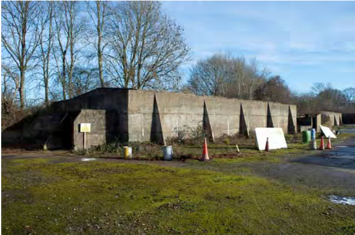
Plate 9: Store 4 – View of the north-west and south-west elevation of the outer blast wall, facing south-east (233)
