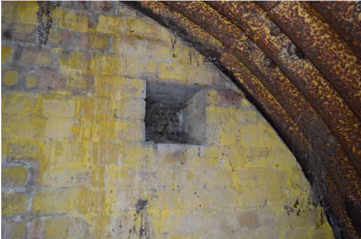
Plate 195: Detail of the air-brick within the south-west elevation of the air-raid shelter, facing west (603)
