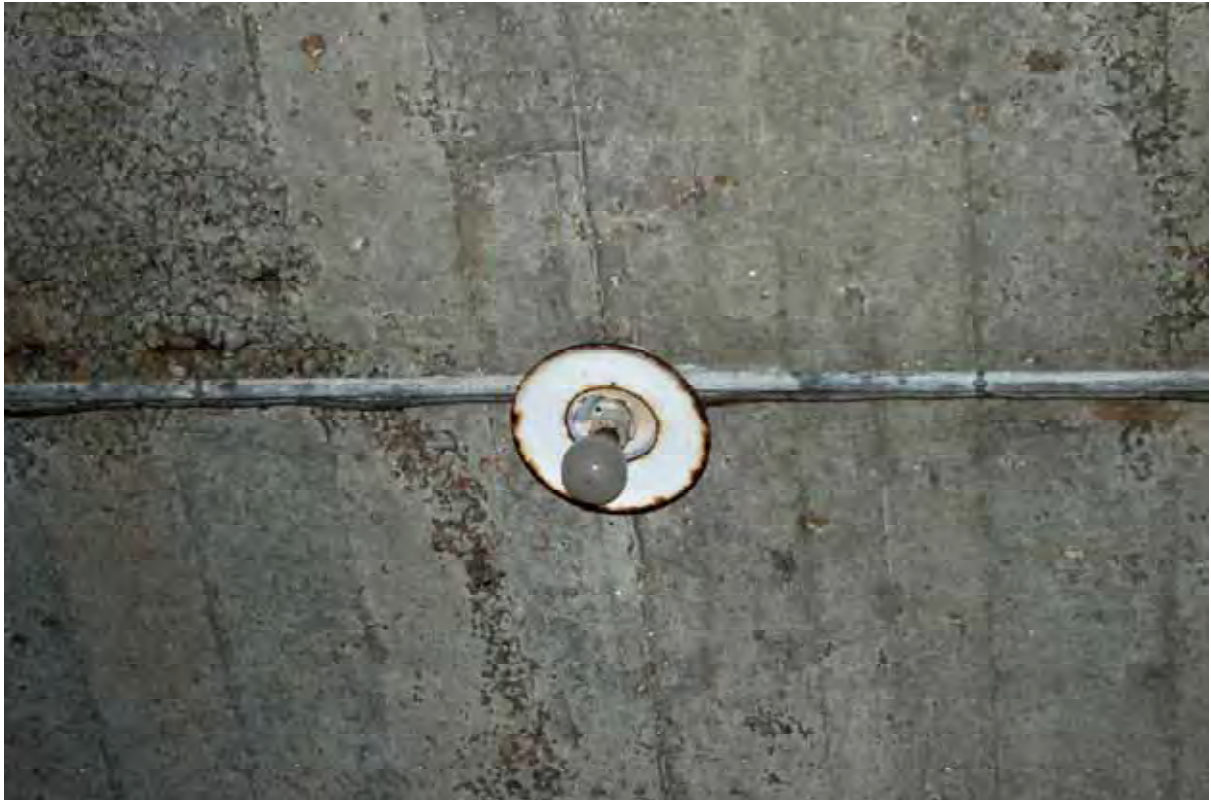
Plate 141: Store 10 – Detail of the retained light fitting within Bin 9, facing south-west (529)
