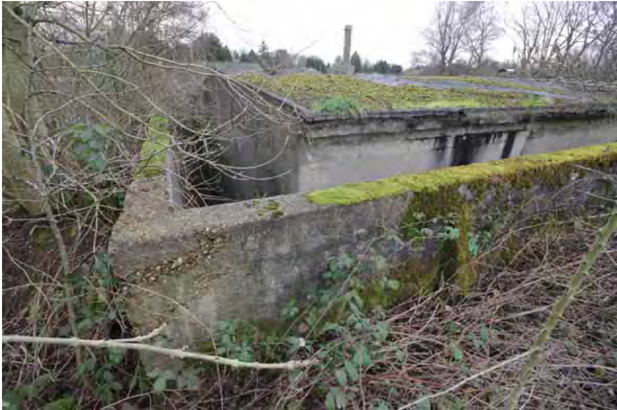
Plate 19: Store 4 – Detail of the roof and walkway separating the inner structure and outer blast walls, facing west (74)
