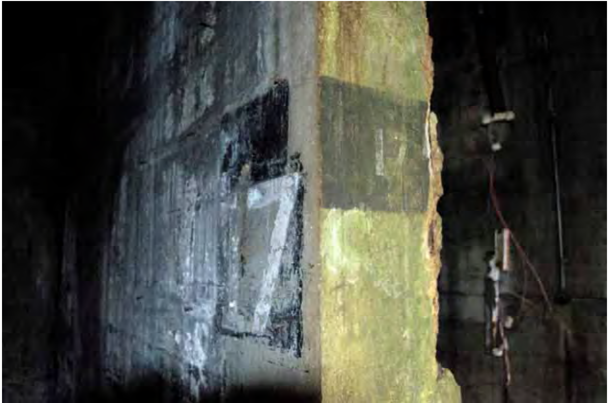
Plate 69: Store 5 –Detail of the phased bay signage visible throughout the structure (Bin 17), facing east (303)
