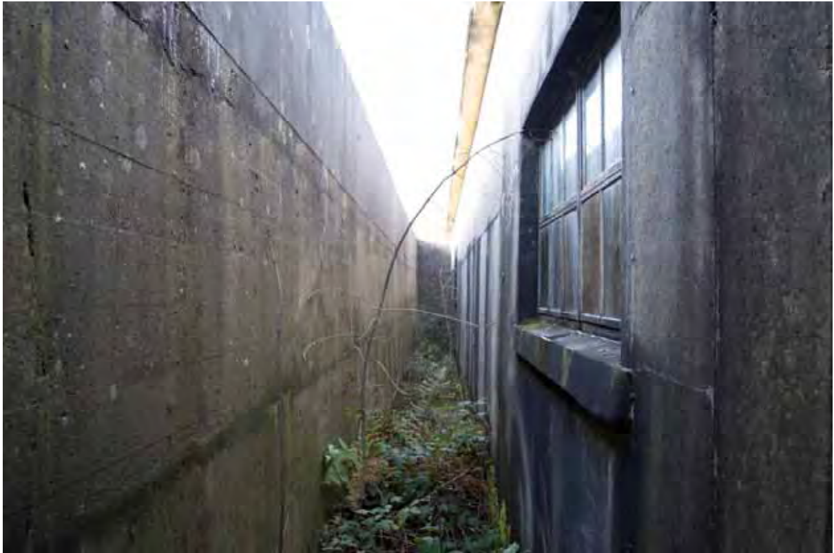
Plate 63: Store 5 – View of the western walkway, note the absence of a cill and high-set openings, facing north-west (297)
