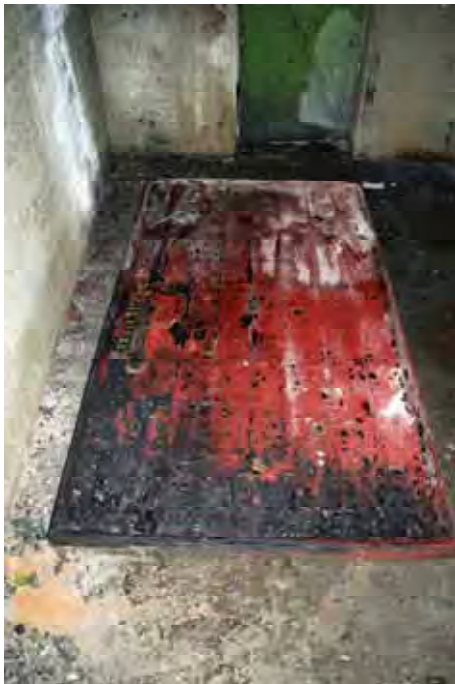
Plate 128: Store 9 – Detail of the timber notice board, entitled 'Regulations', situated at the northern end of the western passage, facing north-west (384)
