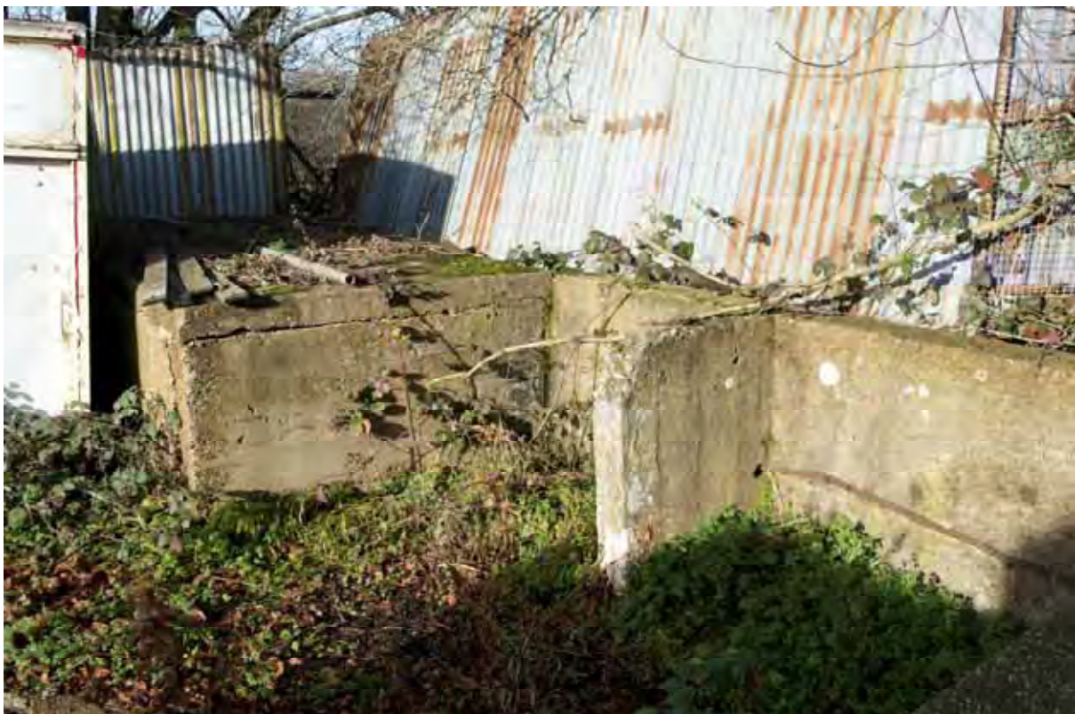
Plate 44: Store 4 – Detail of the eastern loading platform serving the northern loading bay, note retained conveyor base, facing north (281)
