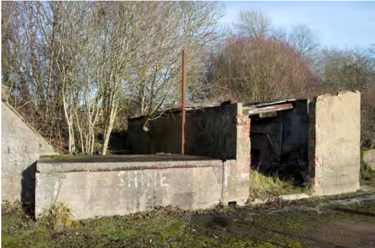
Plate 17: Store 4 / Building 15 – View of the southern loading platform serving the western half of the store, note the lamp post detailing, facing east (282)
