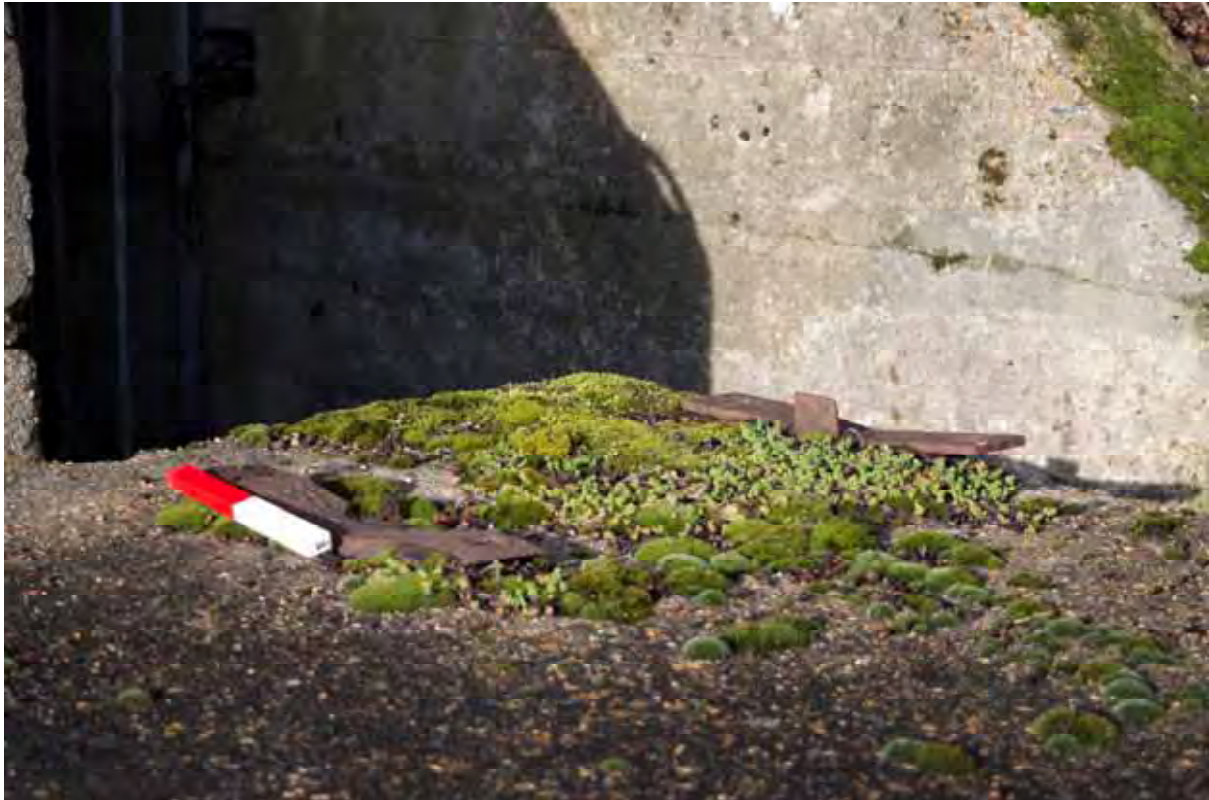
Plate 45: Store 4 – Detail of the conveyor system brackets on the western loading platform serving the southern loading bay, facing north (283)
