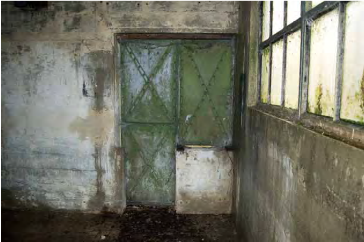
Plate 79: Store 6 – Detail of the doorway complete with conveyor base, set within the northern end of the western passage, facing south-east (351)
