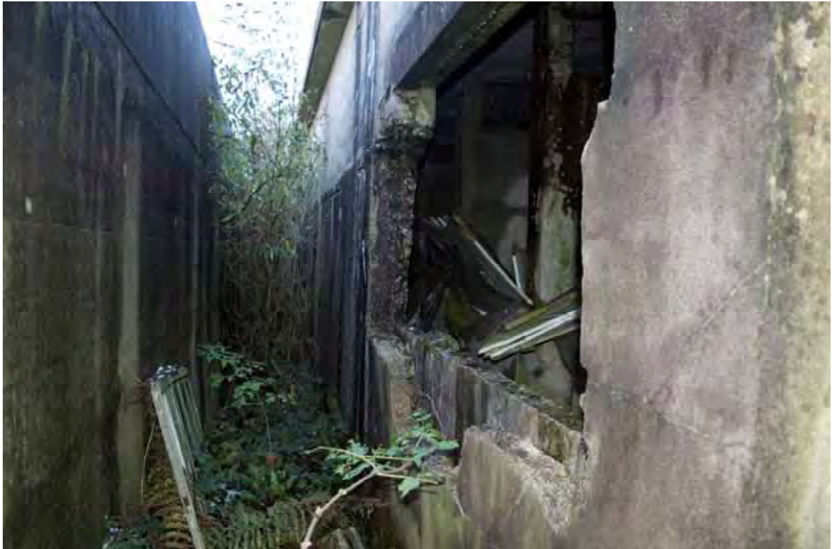
Plate 151: Store 12 – View of the western walkway, note the removal of the window from the south-west elevation of the inner structure, facing north-west (494)
