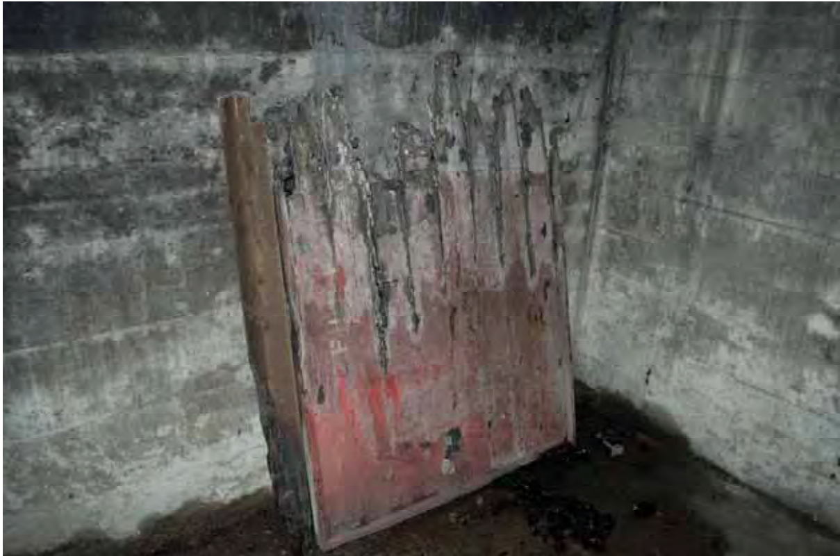
Plate 105: Store 8 – Detail of the fire damaged timber notice board within Bin 15 (western half), note the 'Fire Orders' title still visible, facing north (432)
