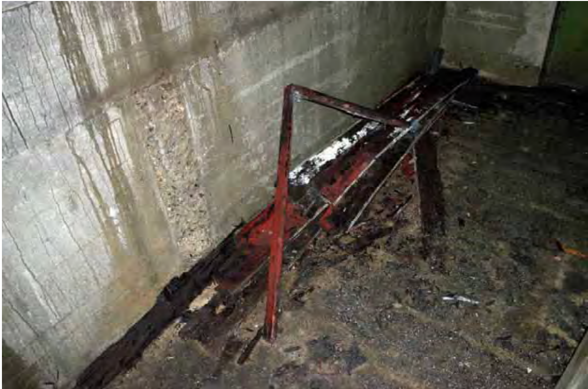
Plate 71: Store 5 – Detail of the degraded timber notice board within the northern end of the western passage, facing west (306)
