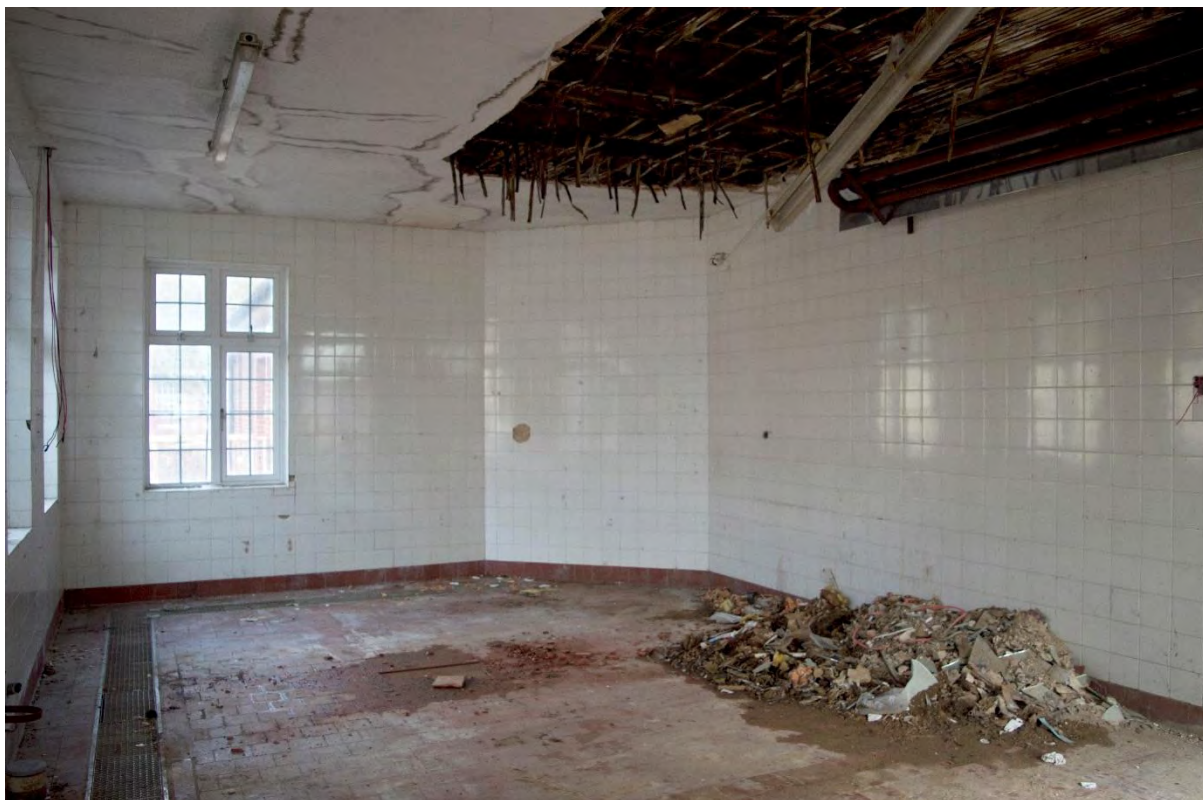
Plate 25 Building 1, central kitchen, food preparation area, possibly original servants' hall, facing north (FHH17-1166)
