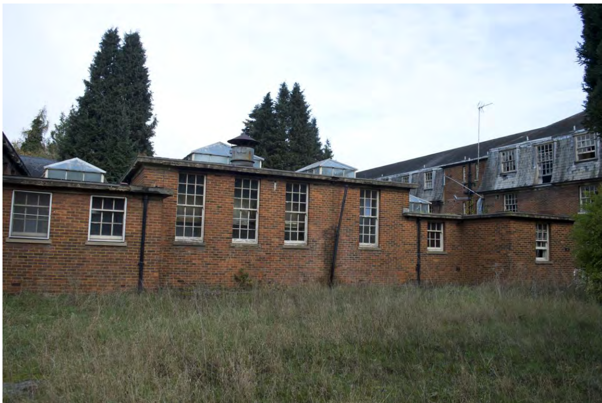
Plate 137 Building 26, nurses' home, courtyard elevations of kitchen, vegetable scullery and rooms for kitchen staff, facing north-east (FHH17-0747)
