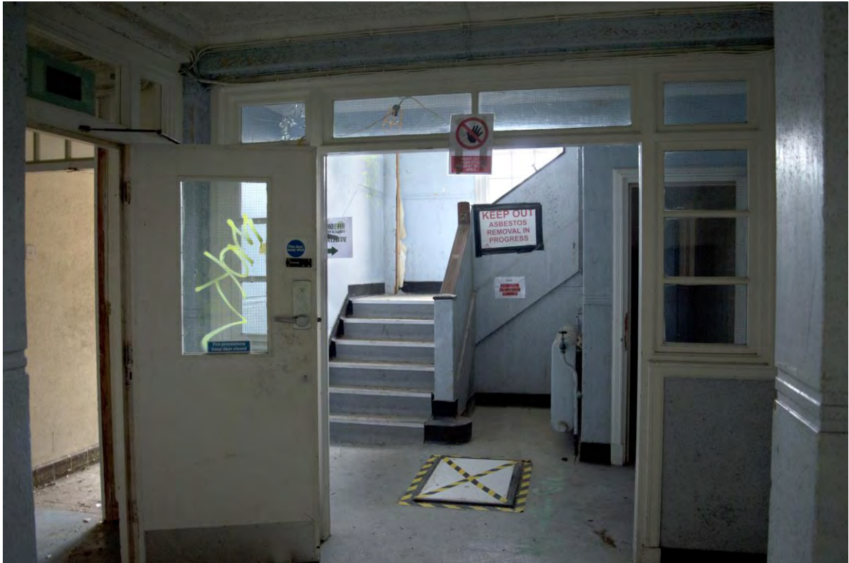
Plate 127 Building 28, nurses' home, principal stair at ground floor level, facing west (FHH17-0848)
