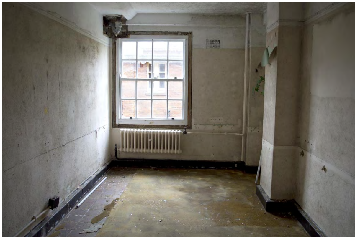
Plate 125 Building 28, nurses' home, ground floor kitchen in central entrance block, facing west (FHH17-0828)
