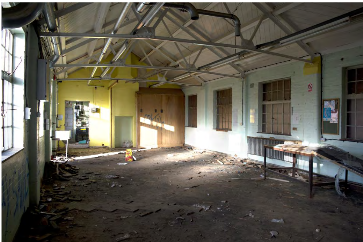
Plate 71 Building 7, carpenters' shop and garages, interior of southern part of range, facing north (FHH17-0670)
