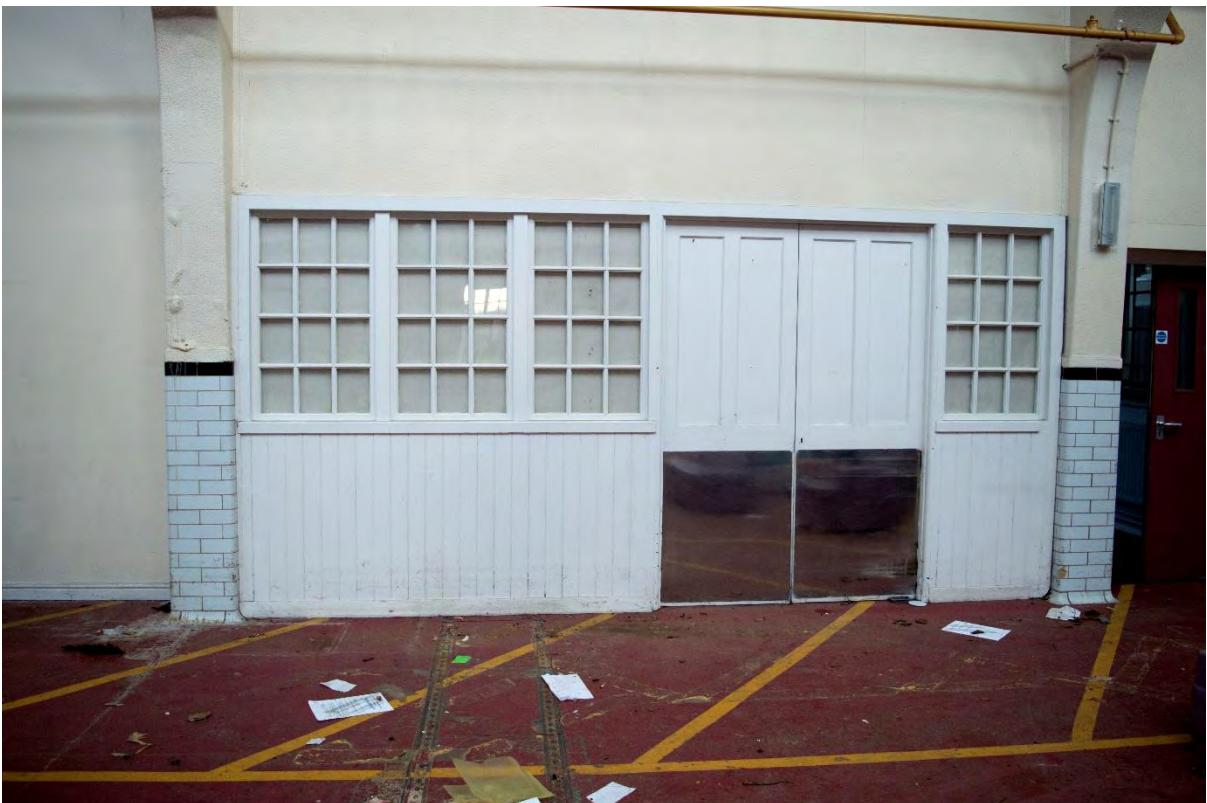
Plate 96 Building 11, general laundry, original partition on east side of main range, facing east (FHH17-0712)
