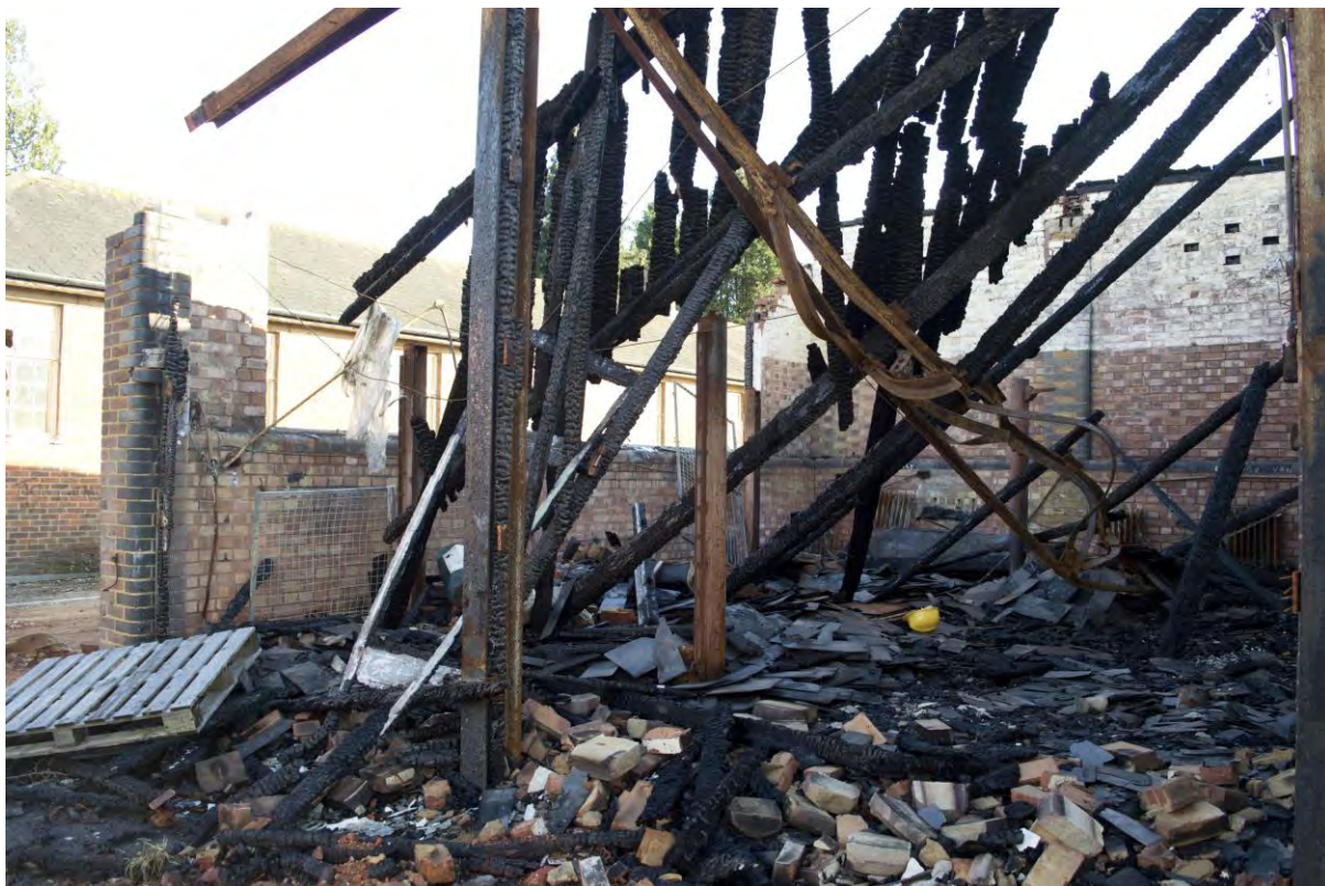
Plate 66 Building 6, fuel store, interior following 2017 fire, facing south-east (FHH17-0652)
