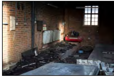
FHH17-0665 Building 06 post fire end
