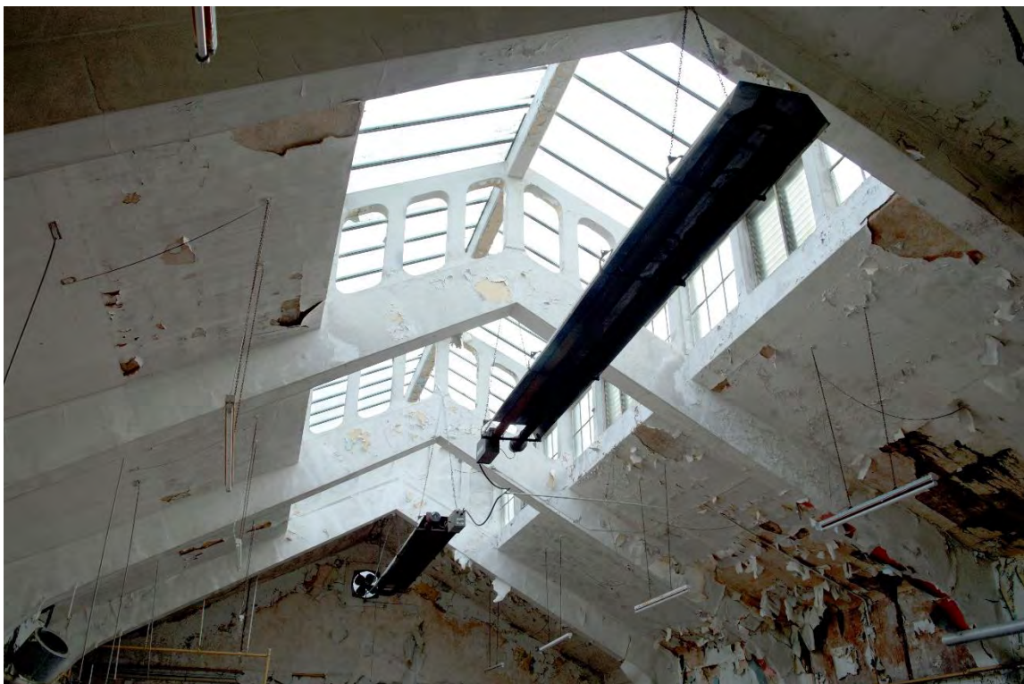
Plate 22 Building 1, central kitchen, detail of roof trusses and lantern light, facing south-east (FHH17-1165)
