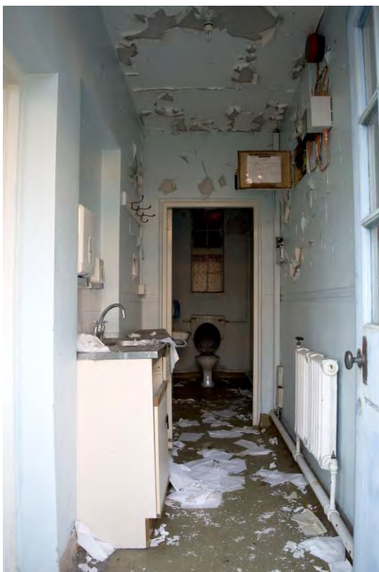
Plate 79 Building 9, workshop, lobby and WC to former clerk of works' office, facing west (FHH17-0685)
