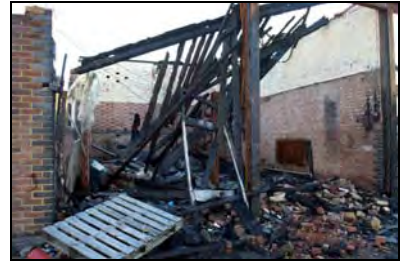
FHH17-0651 Building 06 post fire start
