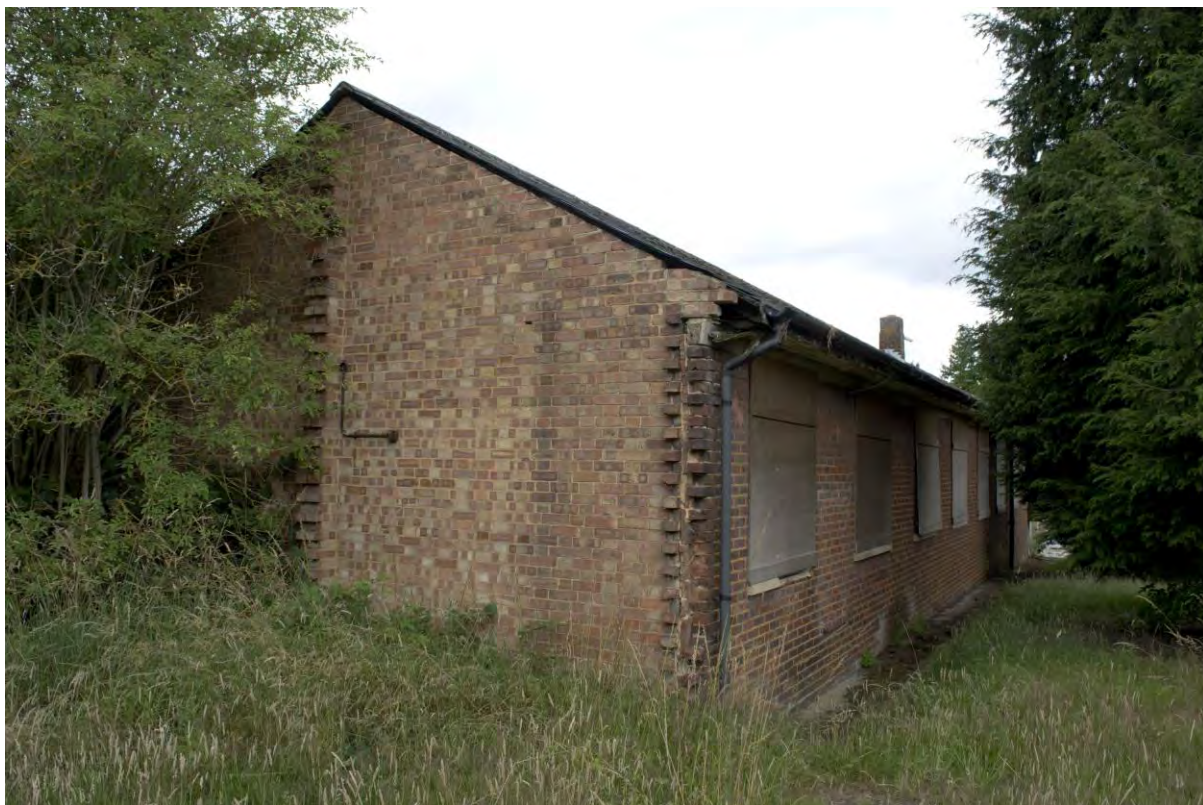
Plate 70 Building 7, carpenters' shop and garages, south elevation, showing brick tootinging for a planned range on the south side of the yard (FHH17-0492)
