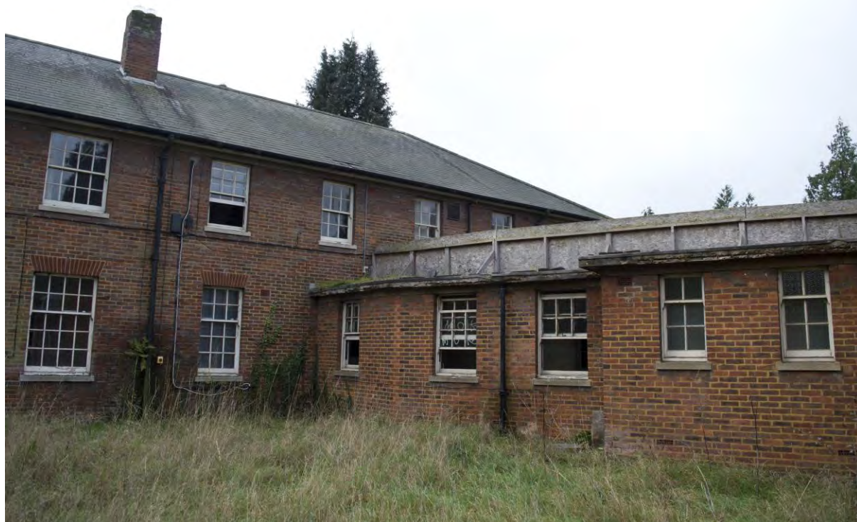
Plate 131 Building 25, nurses' home, north elevation where it meets the corridor to Building 26, facing south-west (FHH17-0736)
