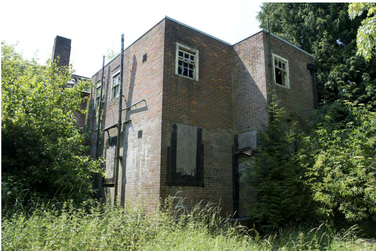
Plate 198 Building 42, male villa, rear sanitary annexe with flat roof, facing south-west (FHH17-0375)
