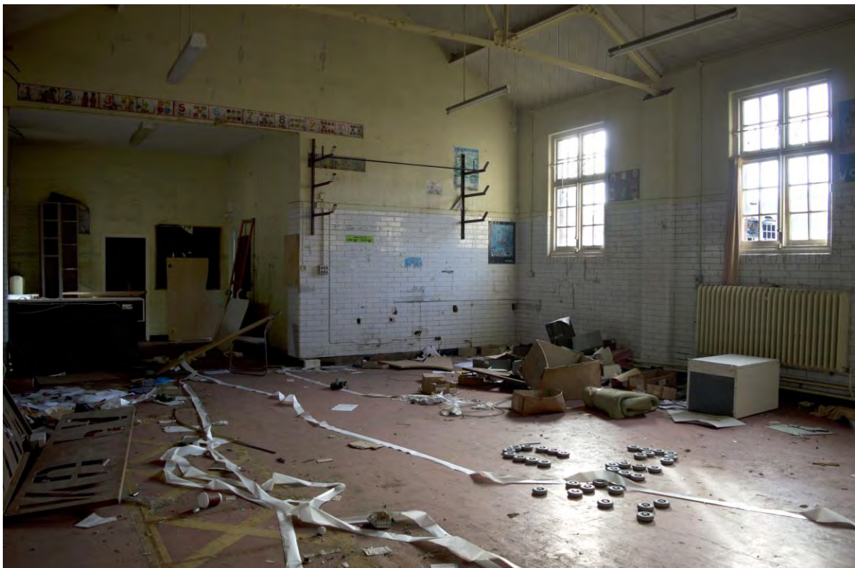
Plate 61 Building 5, bakery to east side of boiler house, facing south-east, showing the large recess which housed a drawplate oven (FHH17-0935)
