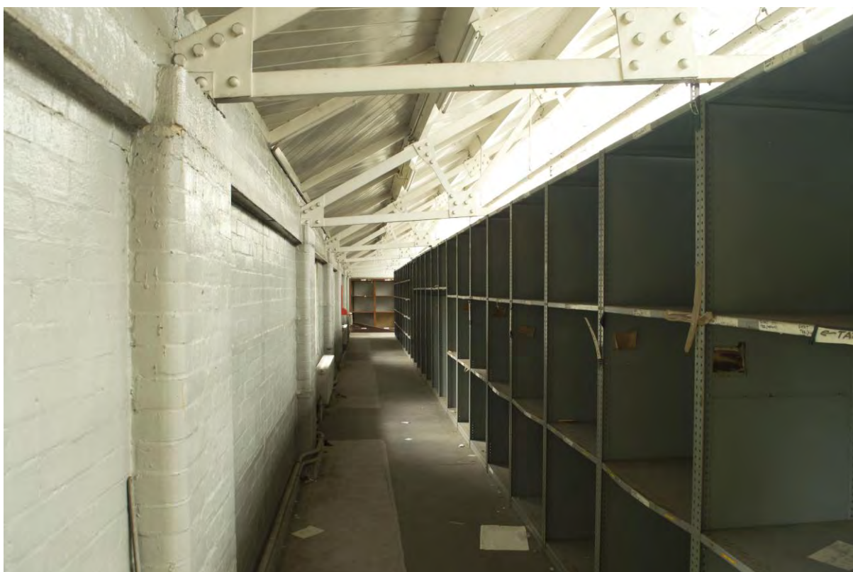
Plate 31: Building 3, main stores, roof truss resting on concrete wall-plate over brick pilaster-buttress, facing west (FHH17-0065)
