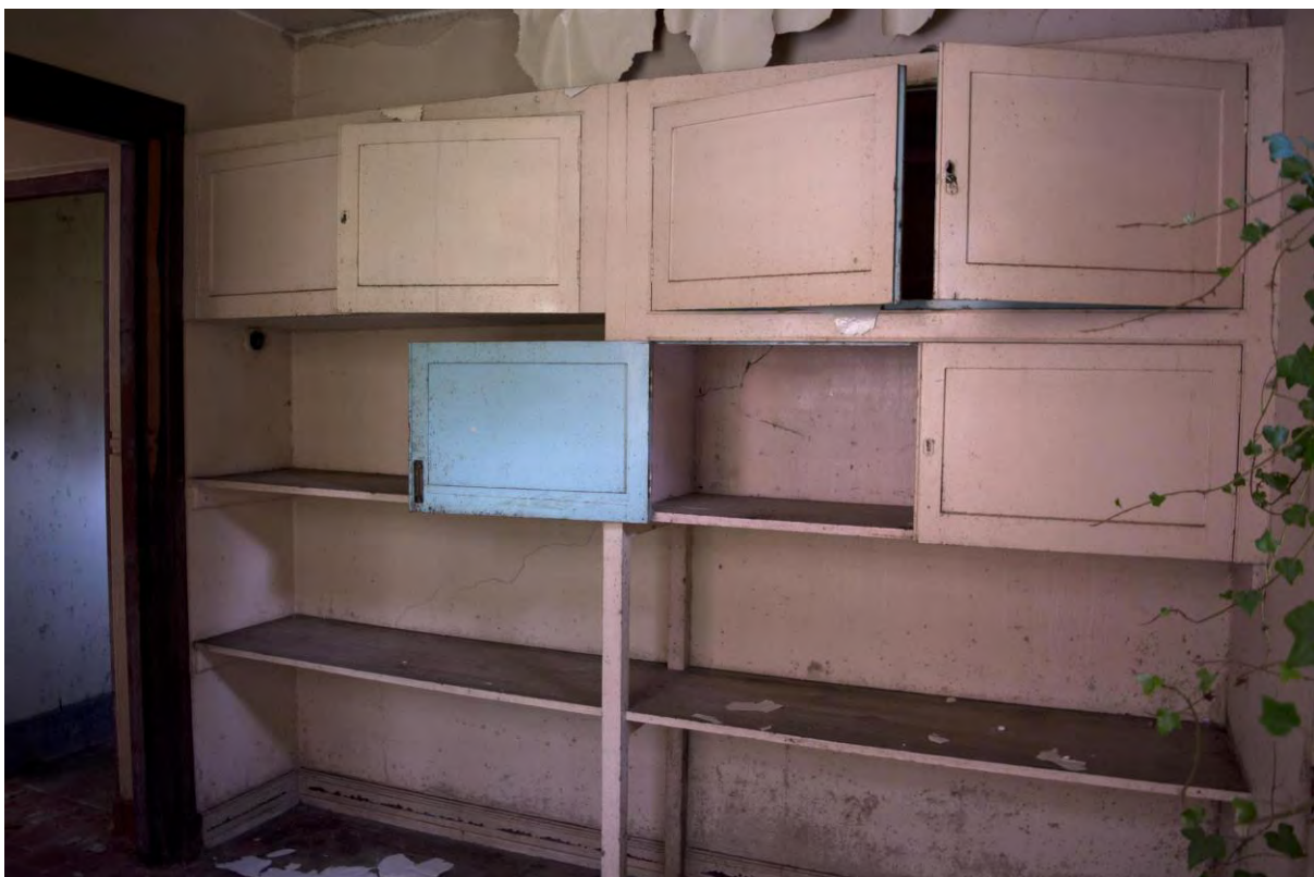
Plate 154 Building 26, nurses' home, shelves and cupboards in cook's room, facing west (FHH17-1266)
