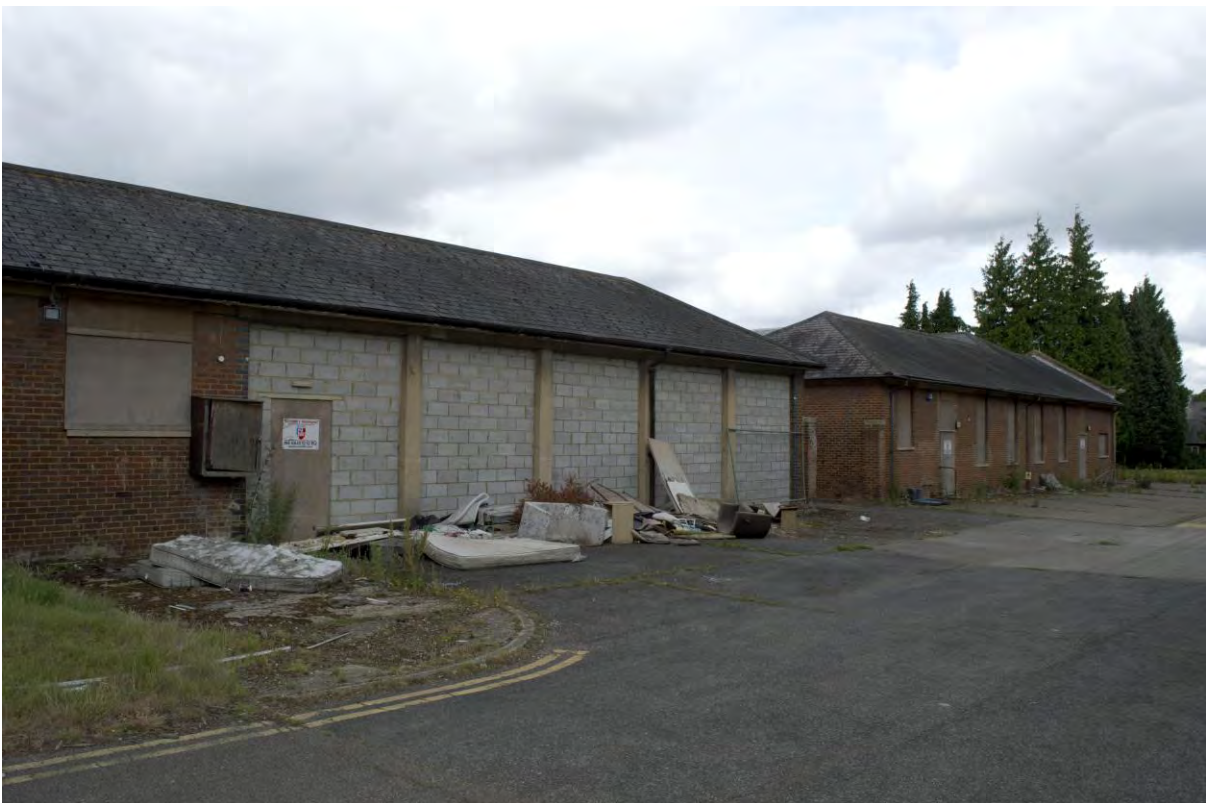
Plate 69 Building 7, carpenters' shop and garages, blocked doors to garages on east elevation, facing north-west (FHH17-0490)
