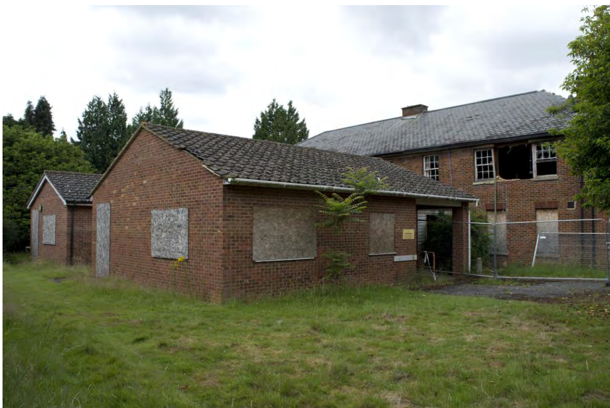
Plate 177 Building 34, male nurses' quarters, single storey addition to south, facing north-west (FHH17-0615)
