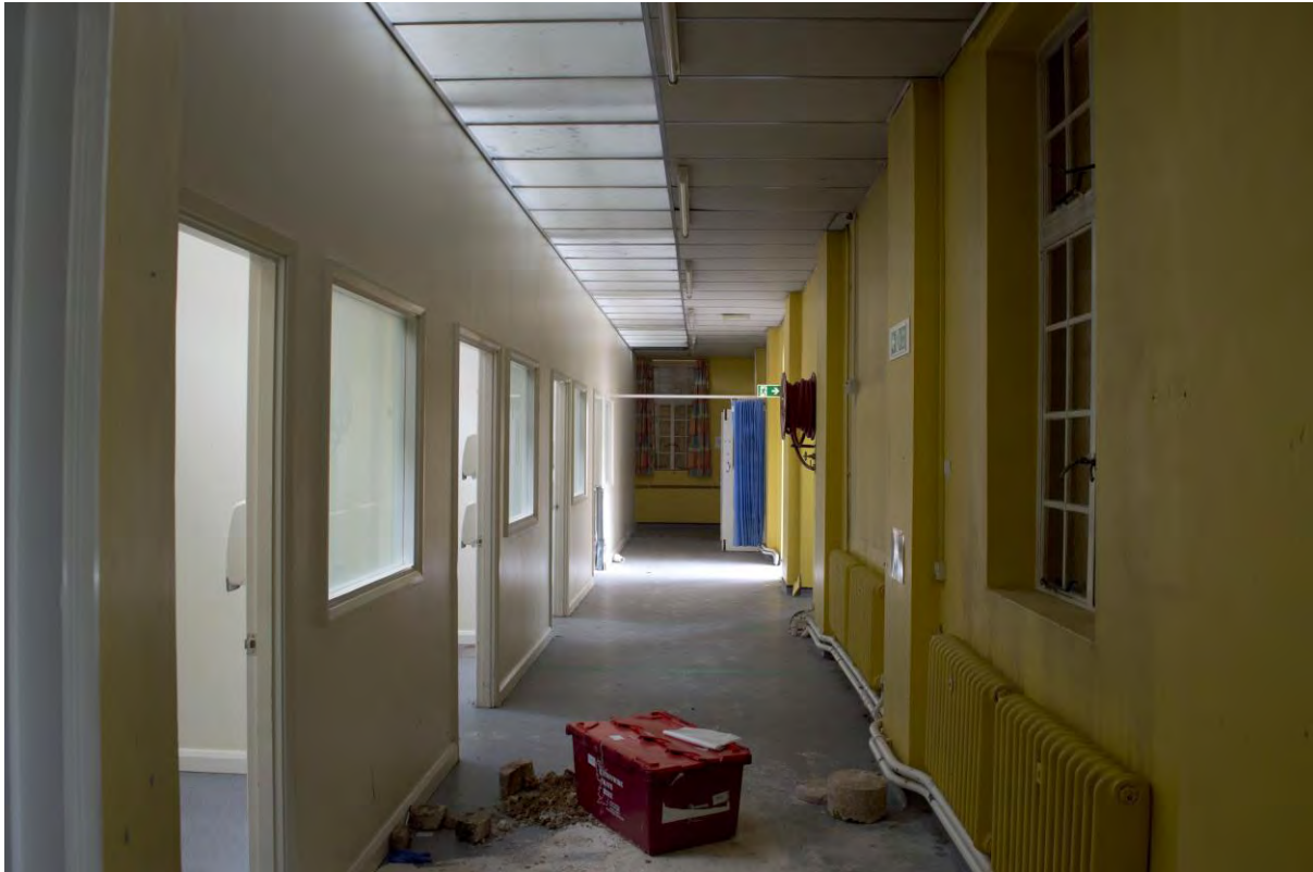
Plate 83 Building 10, staff laundry, interior of main range, facing west, showing inserted corridor and suspended ceiling (FHH17-0191)
