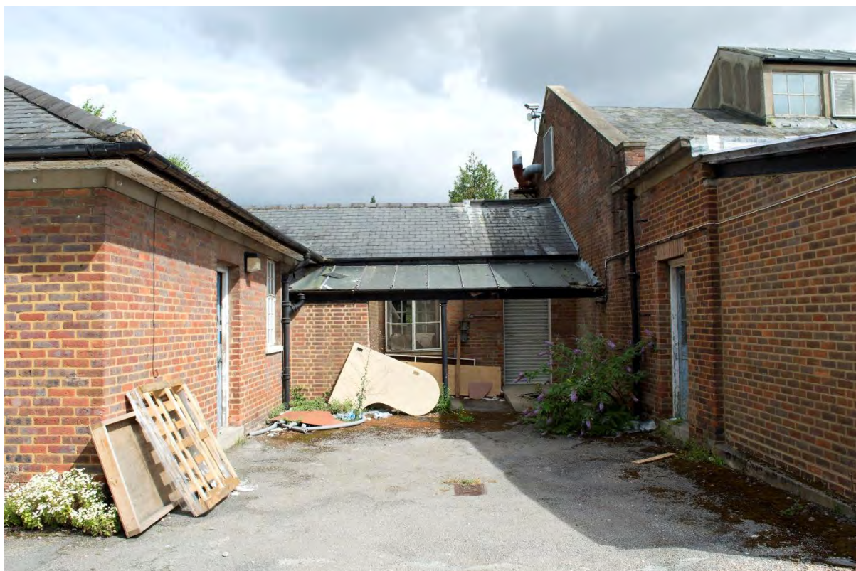
Plate 8 Building 1, central kitchen, covered walkway on south side of west flanking range, facing north (FHH17-466)
