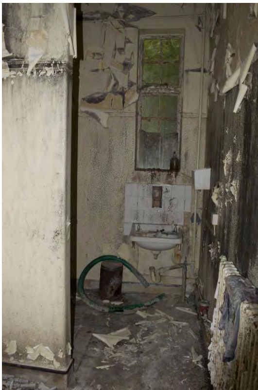
Plate 104 Building 12, disinfectant block, interior of WC/shower room at west end of building (FHH17-0237)
