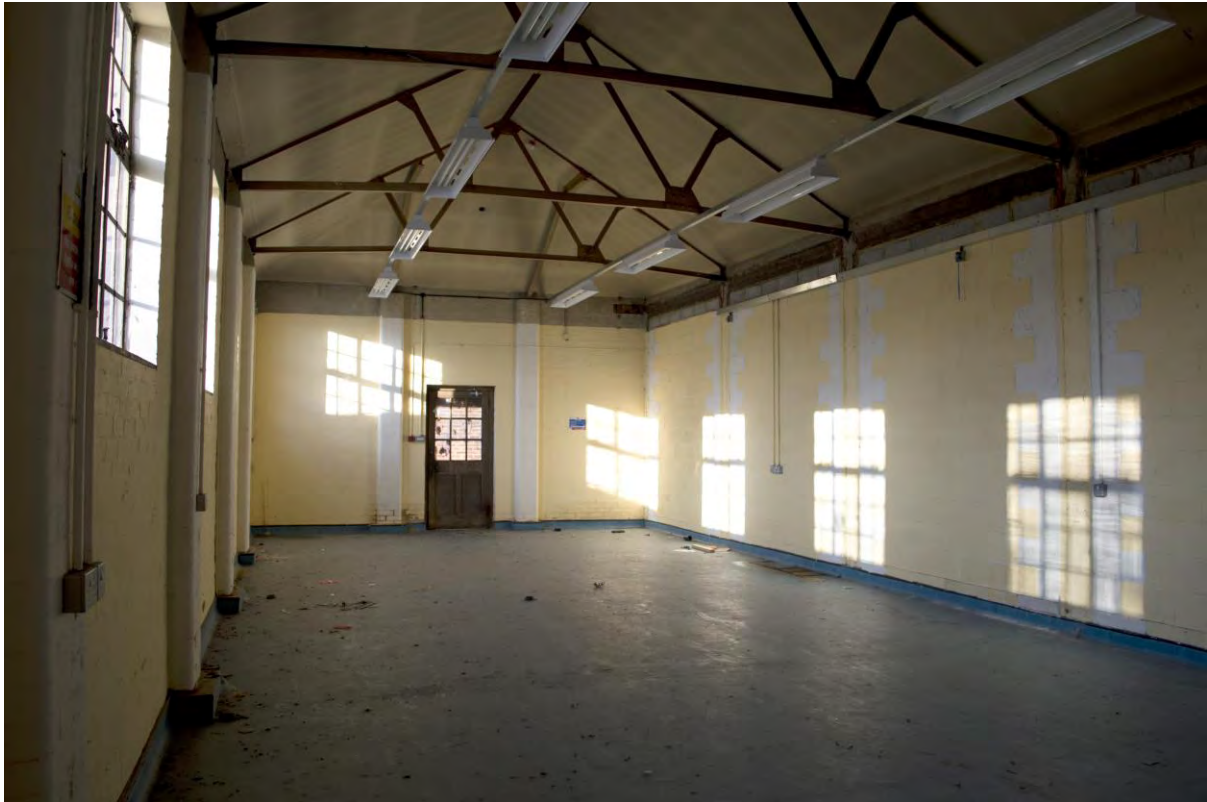
Plate 72 Building 7, carpenters' shop and garages, interior of the former garages in the northern part of the range, facing north (FHH17-0674)
