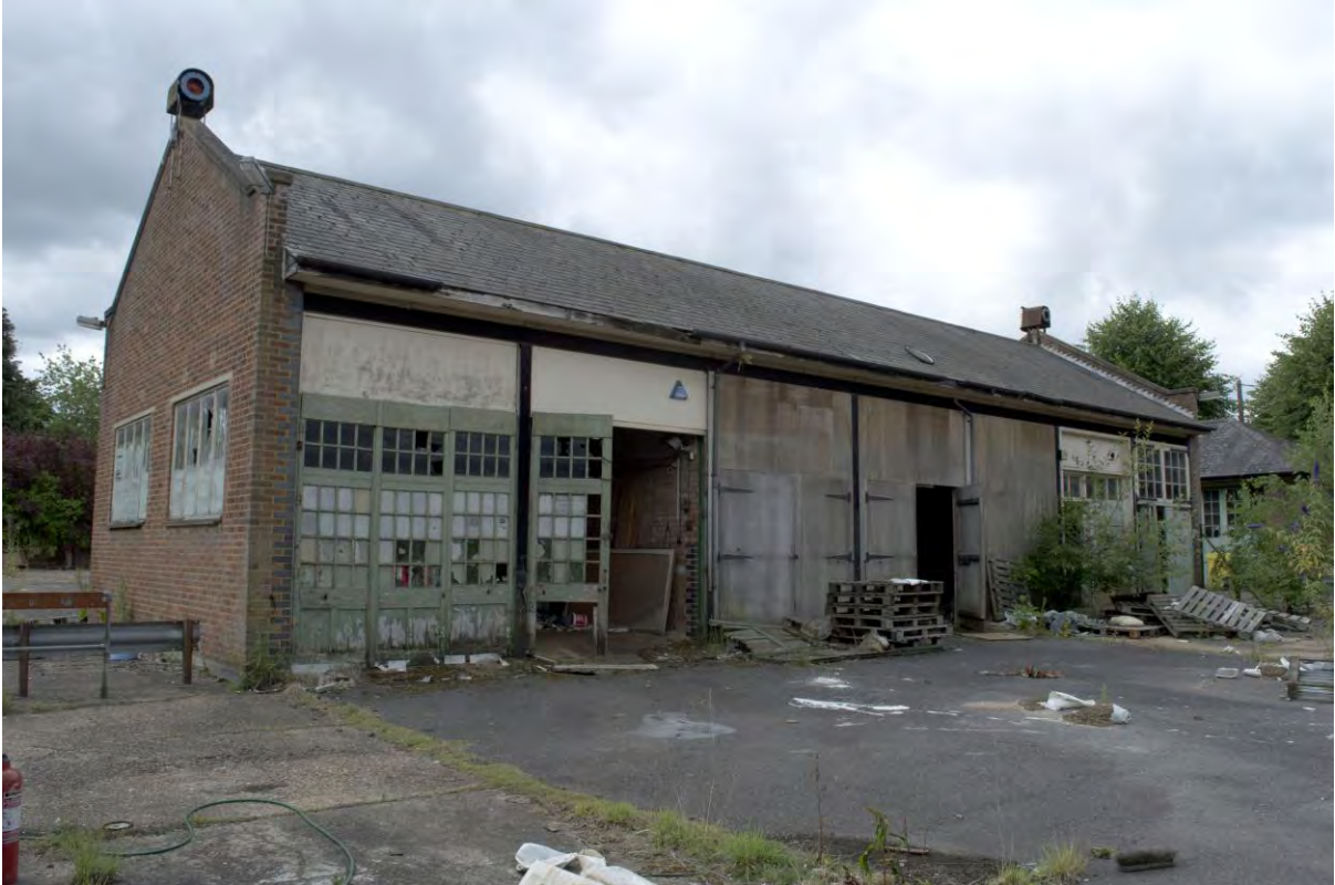
Plate 64 Building 6, fuel store, facing south-west (FHH17-0508)
