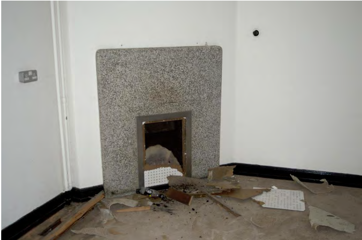
Plate 161 Building 27, nurses' home, polished concrete fire surround in suite, ground floor (FHH17-0951)
