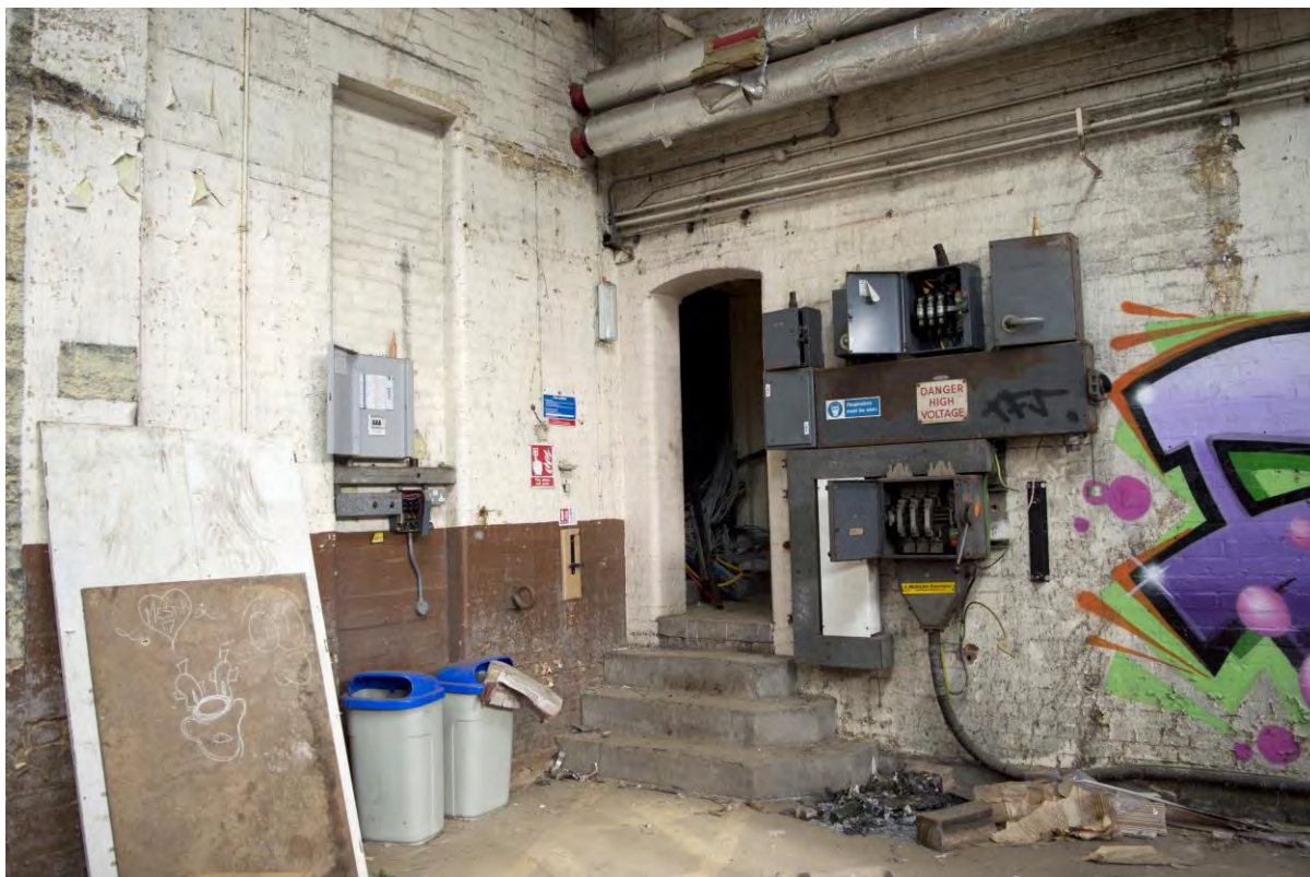
Plate 56 Building 5, boiler house, inserted steps and doorway to 1960s extension, facing north-west (FHH17-0894)
