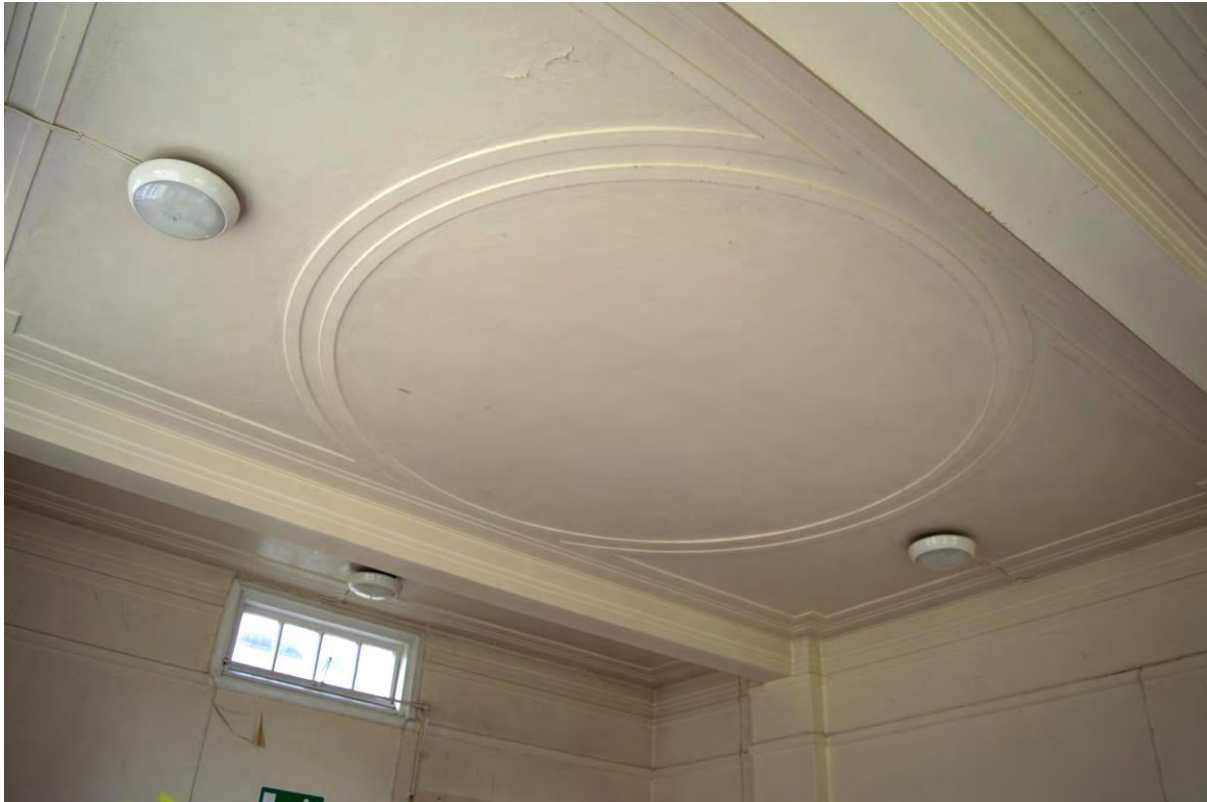
Plate 147 Building 26, nurses' home, detail of ceiling rose in senior staff dining room/lounge (FHH17-1212)
