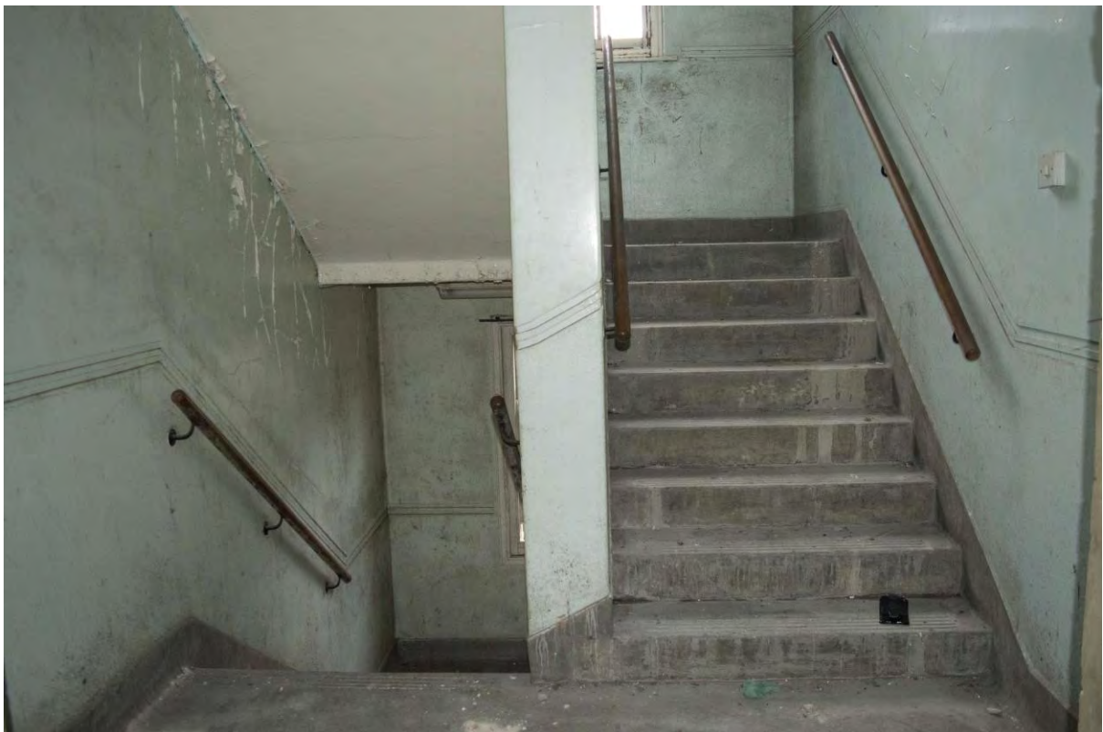
Plate 128 Building 28, nurses' home, north secondary stair at first floor level, facing west (FHH17-1415)
