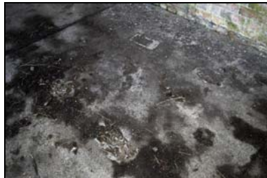
GIL18-0041 Scars in the concrete floor from machinery
