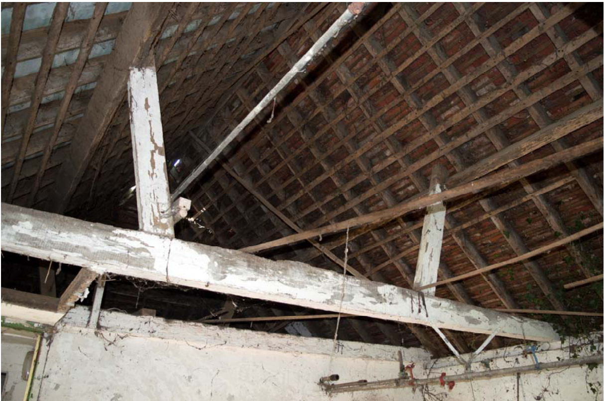
Plate 28 – Representative truss in the dairy (foreground) and that with the struts removed, facing north-west (GIL18-0093)
