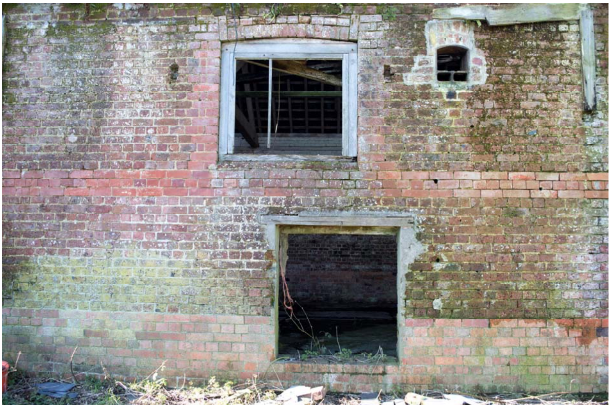
Plate 6 – Inserted windows and openings on the east elevation of the barn, facing west (GIL18-0006)
