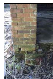
GIL18-0012 Detail of truncated older brickwork at the midstre opening. Facing south
