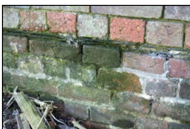
GIL18-0011 Detail of the likely older brickwork below the DPC. Facing south-west
