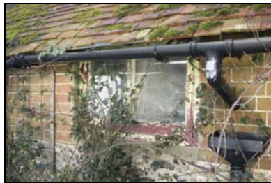
GIL18-0065 Inserted window in the north facing elevation of the dairy. Facing north
