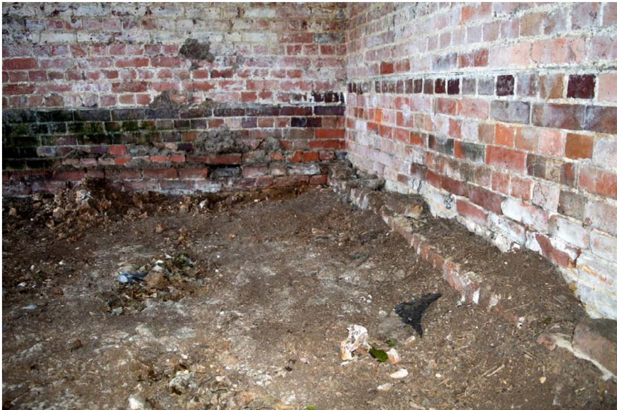
Plate 18 – Earlier brickwork visible below the damp-proof course, facing north-west (GIL18-0032)
