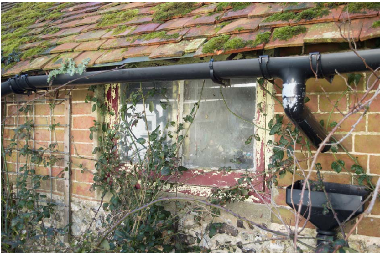
Plate 26 – Window inserted into the north elevation of the dairy, facing south-east (GIL18-0065)
