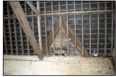
GIL18-0033 Detail of the roof where the barn and dairy join. Facing west
