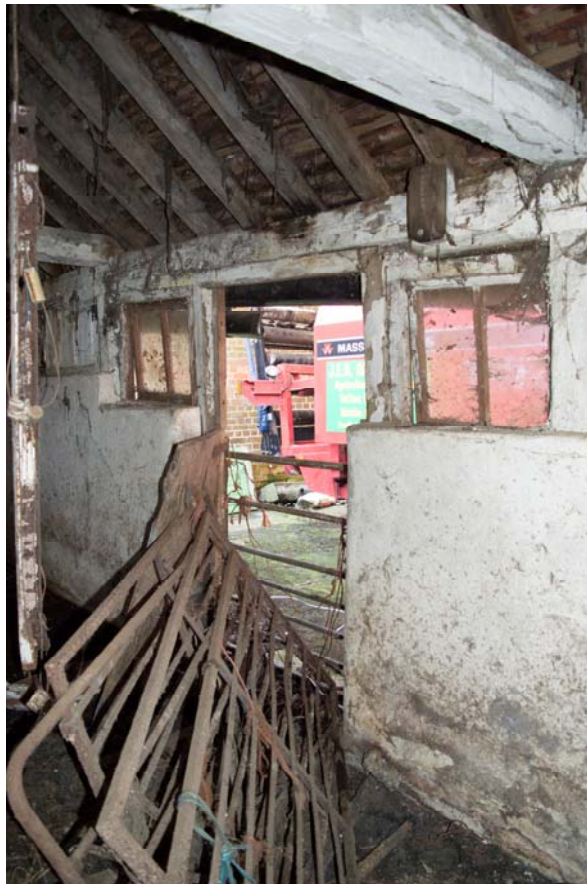
Plate 38 – Infilled original open front of the eastern part of the dairy, facing south-east (GIL18-0103)
