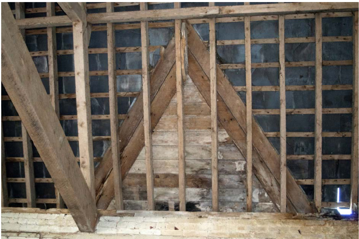
Plate 16 – Boarding replacing the barn's roofing slates where the dairy was added, facing west (GIL18-0034)
