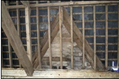
GIL18-0034 Detail of the roof where the barn and dairy join. Facing west
