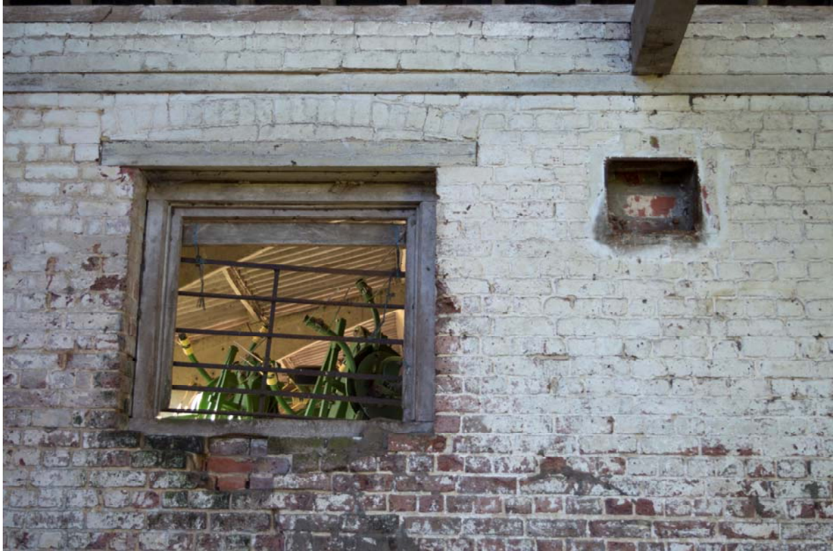
Plate 17 – Inserted window and machinery housing in the barn wall, facing west (GIL18-0040)
