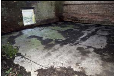
GIL18-0037 Concrete scree floor at the southern end of the barn. Facing south-east
