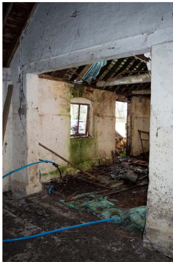
Plate 36 – Inserted opening in the brick wall between Rooms 3 and 4 of the dairy, facing south-west (GIL18-0102)
