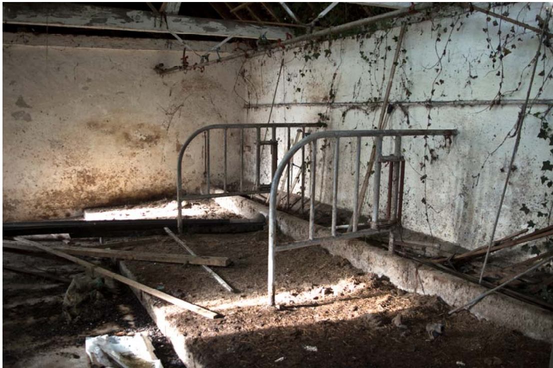
Plate 37 – Stall partitions and feeding trough in the dairy (Room 3), facing north-west (GIL18-0095)
