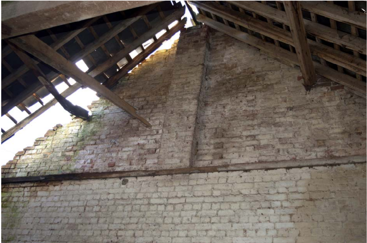
Plate 15 – Internal view of the southern gable end of the barn, facing south-east (GIL18-0051)
