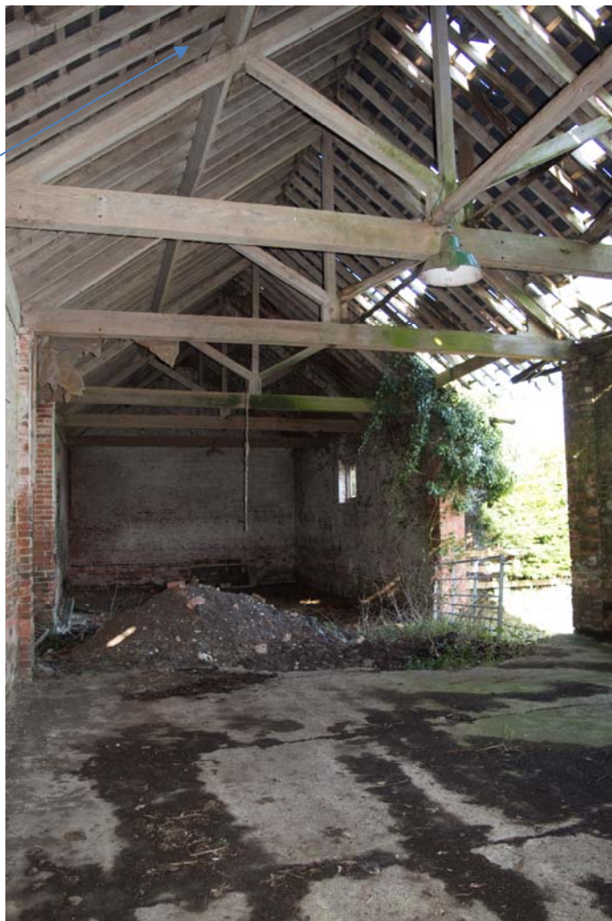
Plate 13 – Interior of the barn looking north-east. Location of E carved into the rafter is indicated by the arrow (GIL18-0043)
