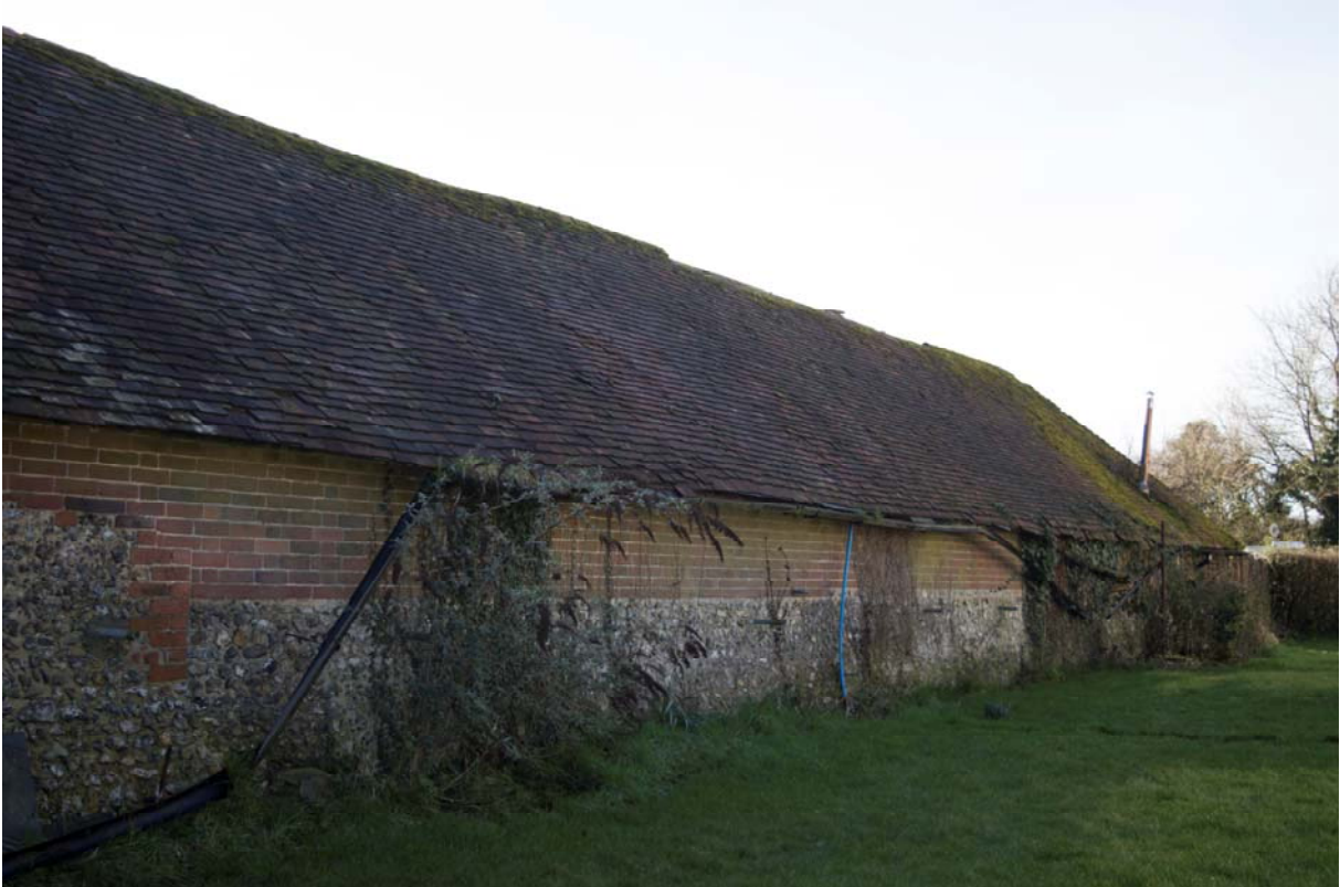
Plate 25 – North elevation of the dairy showing the incorporated flint yard wall, facing south-east (GIL18-0062)
