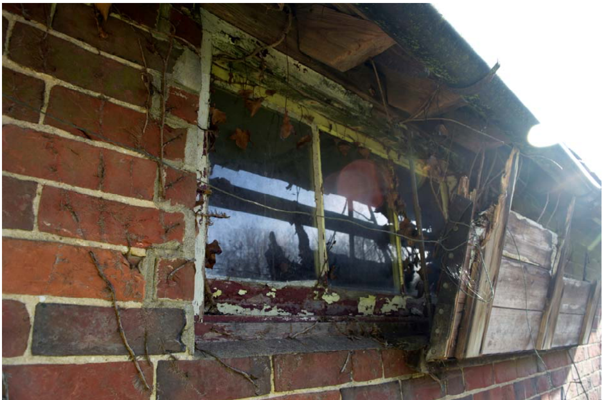
Plate 24 – Window inserted into the west elevation of the dairy, facing south-east (GIL18-0068)
