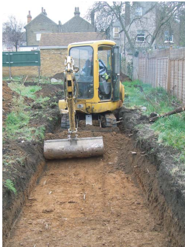
© Archaeology South-East The Brent, Dartford Fig. 5 Project Ref: 3291 March 2008 Excavating Trench 1 Report Ref: 2008019 Drawn by: SM
