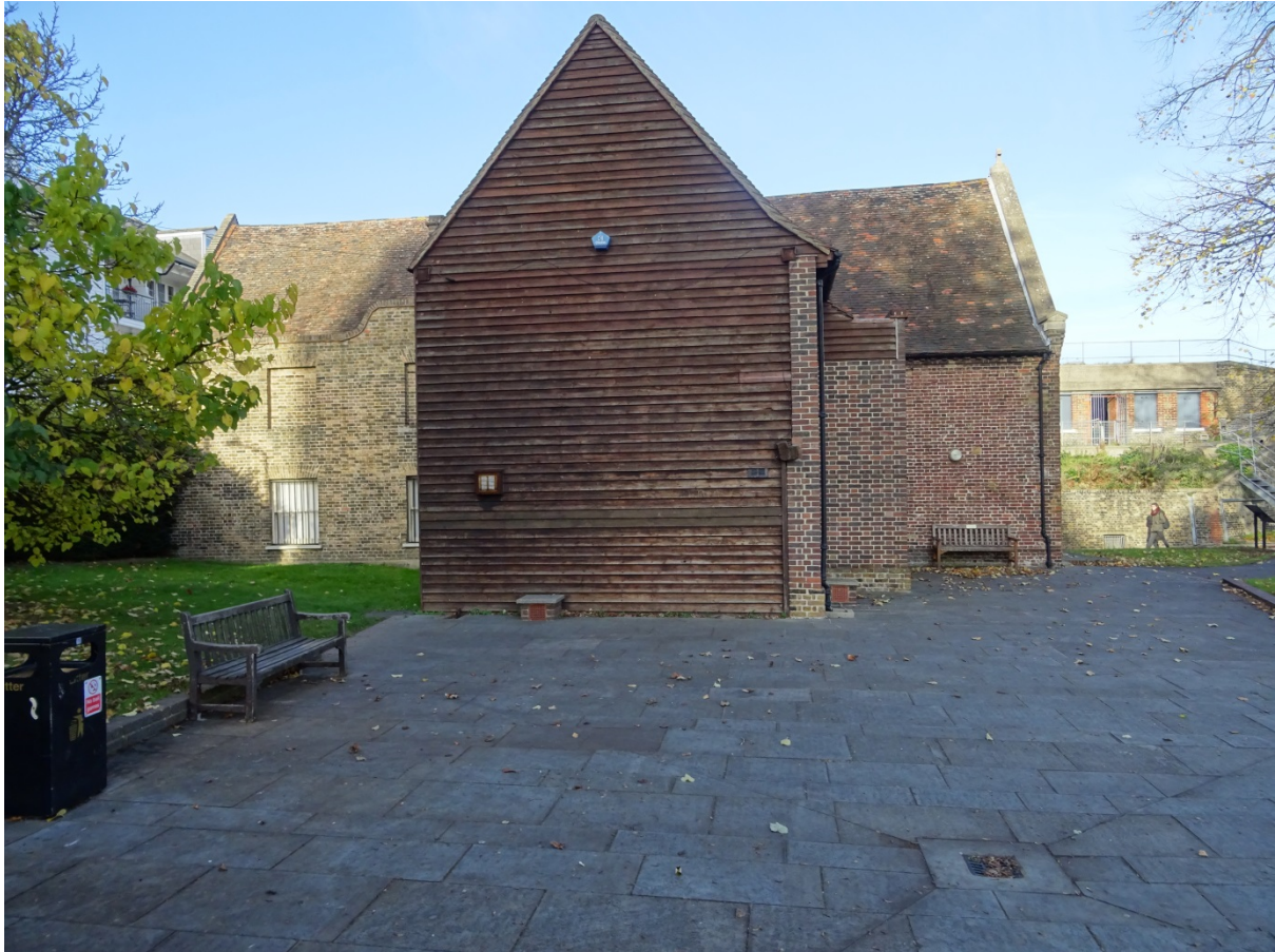
Milton Chantry, view looking north. Weather-boarded south wall of south block at centre with brick-faced medieval chantry beyond. Water pipe subject to works passes below lawn to left, in angle between buildings.
