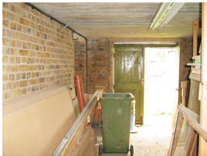
Plate 6: Interior of the north room with later inserted double doors in the north end wall, shows the un-painted brickwork
